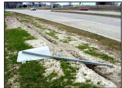
Figure 1: Improper Sign Removal
