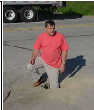
Figure 3: Improper pothole restoration
