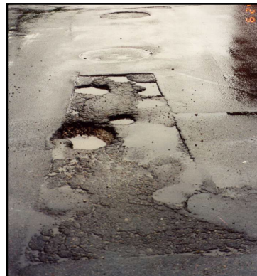
Figure 5: Both patches improperly backfilled/compacted, and not patched to nearest joint or seam
