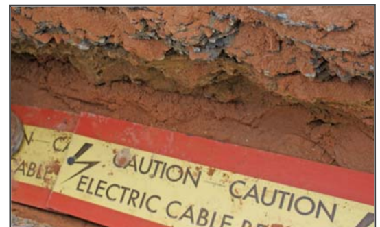
Underground utilities are one example of the hazards to be identified in the ITCP (Source: Interserv).
