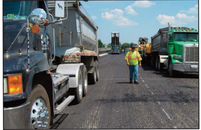
An ITCP should provide rules for workers if they must pass vehicle paths (Source: ARTBA).
