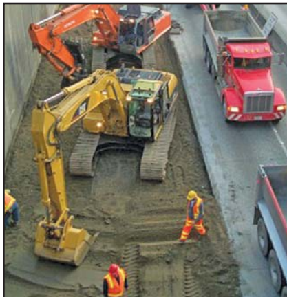
An internal traffic conflict between workers on foot and equipment (Source: pavementinteractive.org ).
