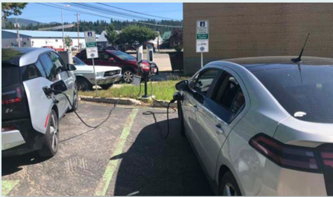
EV Charging Station in Newport
