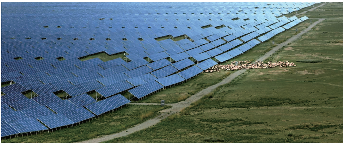
Renewable energy hub in Gonghe, Qinghai, built with the support of Huawei's smart PV solution: Herding sheep under solar panels and supplying green electricity to Henan Province, more than 1,500 kilometers away, via an UHVDC line
