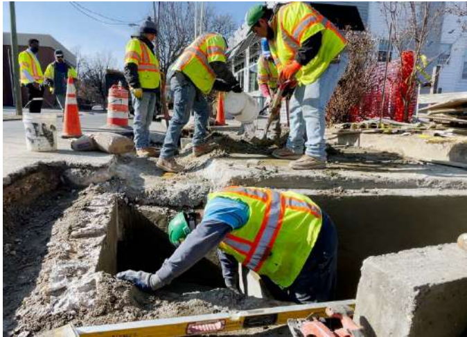
A crew pours concrete to form the catch basins for the new, wider inlets on Hume Avenue.
