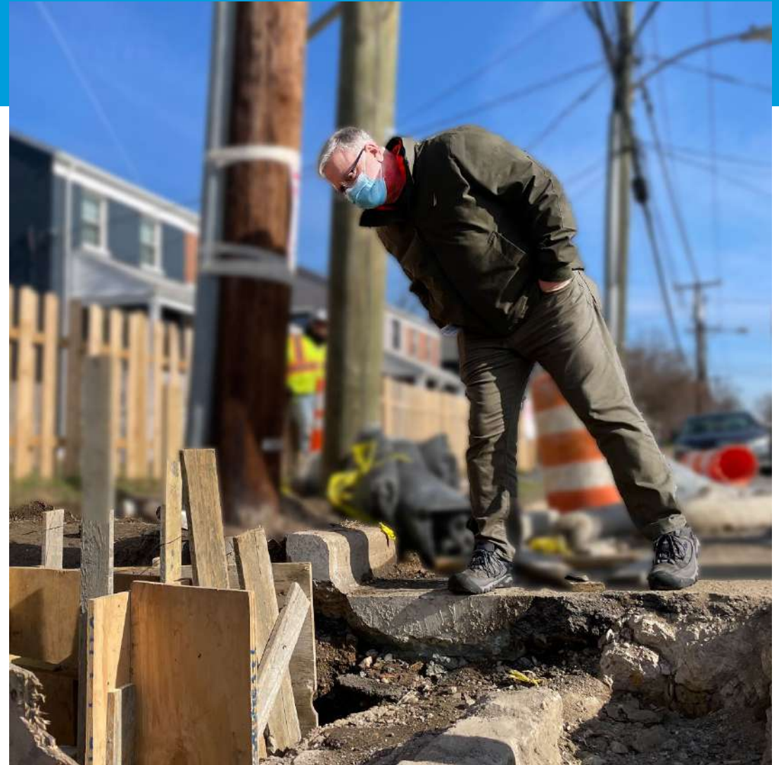
Engineer Brian Rahal, of the Stormwater Management Division, monitors progress on larger inlet installation on Hume Avenue on Jan. 24, 2022
