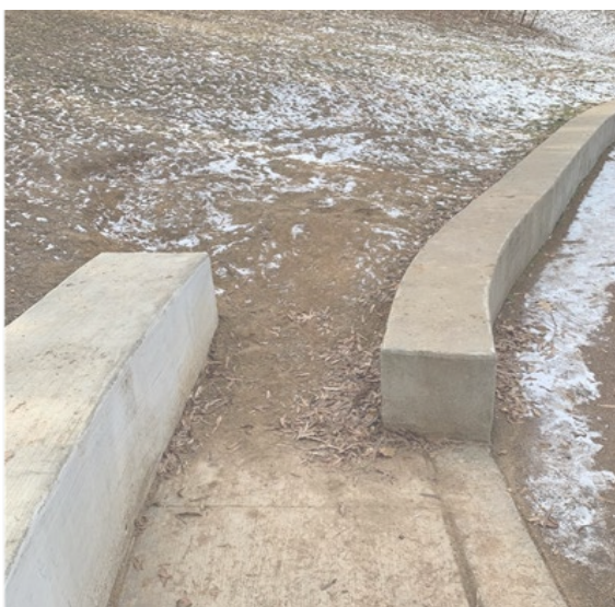
New stone steppers and plantings (not shown) to address soil erosion between the seating walls
