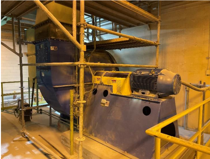
Figure 7: New LN fan for Unit 3
