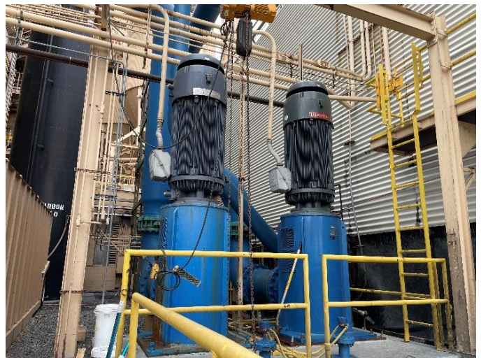
Figure 36: Cooling Tower Circulating Water Pumps
