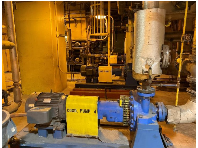
Figure 26: Turbine Condensate Pumps
