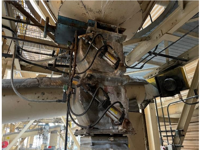
Figure 8: Double dump valves both failed open – allows for air in-leakage
