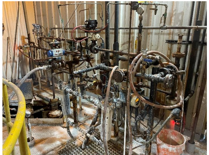
Figure 34: Scrubber Penthouse Lime Slurry Station
