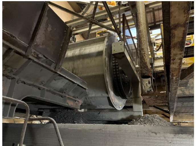
Figure 4: New ferrous magnet installed in Feb. 2022
