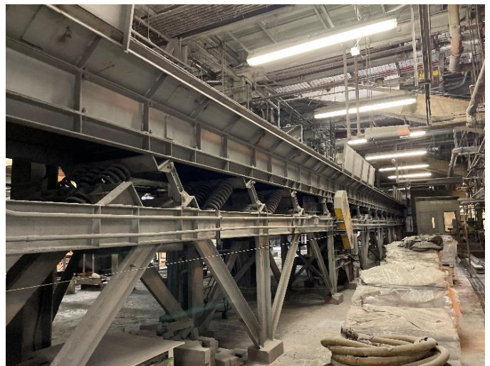
Figure 22: Main Ash Vibrating Conveyor
