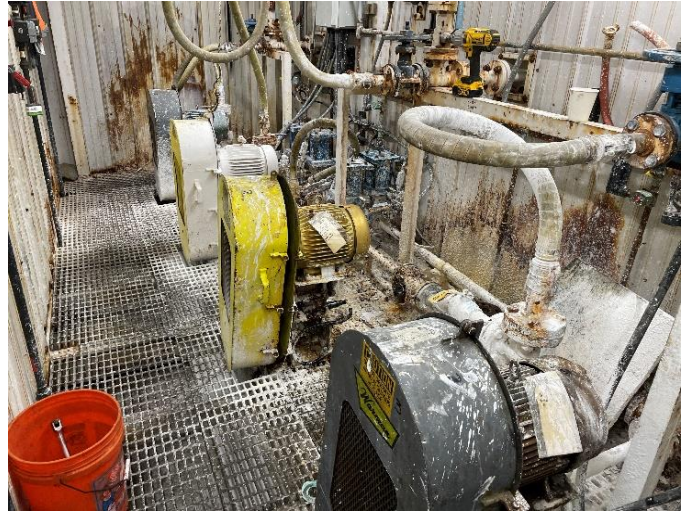
Figure 32: Lime Slurry Pumps
