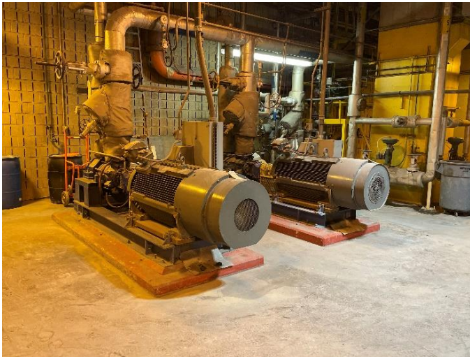
Figure 25: Boiler Feedwater Pumps
