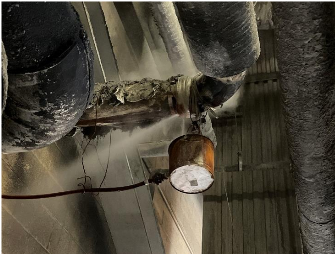
Figure 1: Feedwater pipe leak (photo from Feb. 2022)
