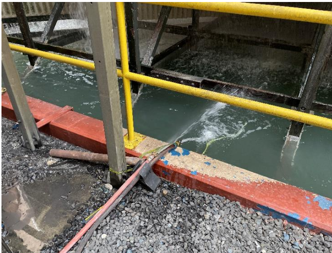
Figure 3: Heavy water discharge from feedwater pipe leak was being diverted to the cooling tower basin instead of the settling basin
