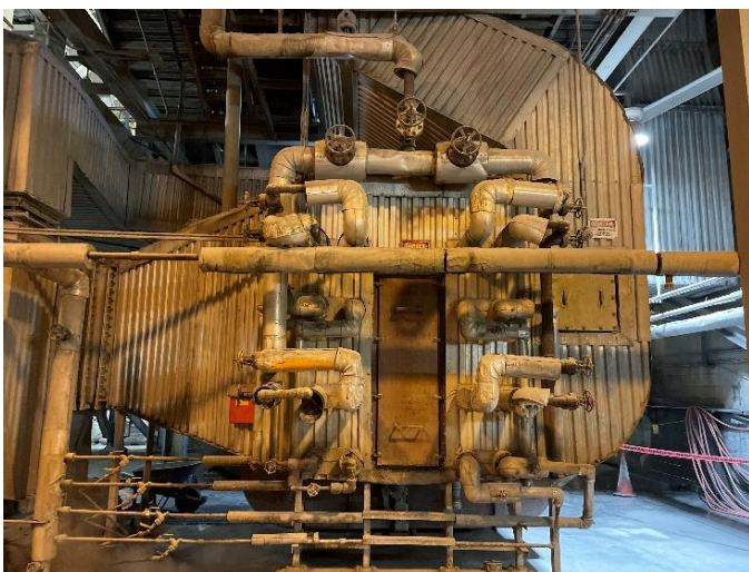
Figure 23: Combustion Air Pre-Heater
