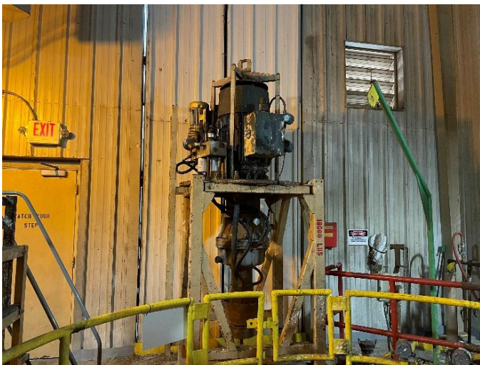
Figure 35: Scrubber Lime Slurry Atomizer
