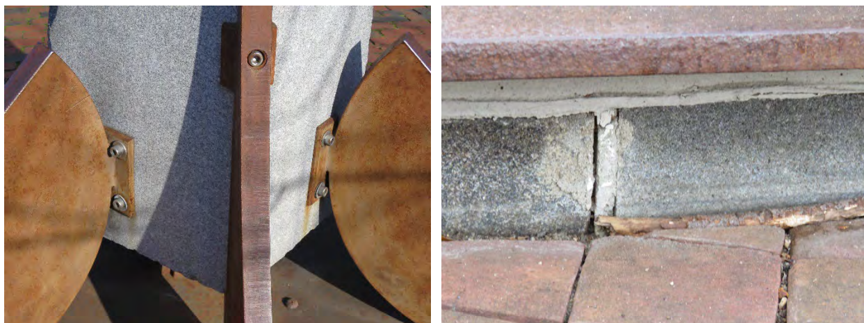
(Left) Minor localized ferrous staining on the granite, in areas where the metal has contact with the masonry. (Right) Deterioration of the mortar within the joints on the base.
