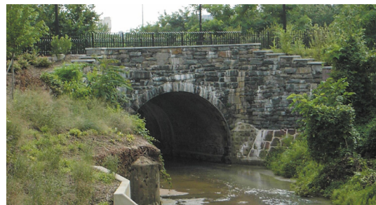
Hooffs Run Bridge is the last surviving stone structure of the Orange and Alexandria Railroad.
