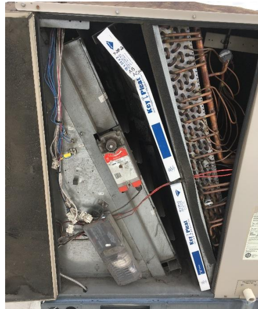
Figure 6. Picture of filter not seated correctly.
