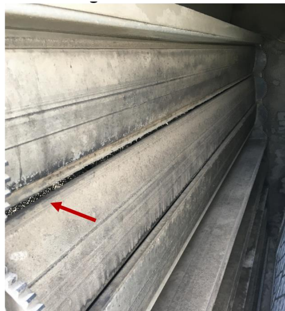
Figure 5. Picture of a warped damper blade unable to close.
