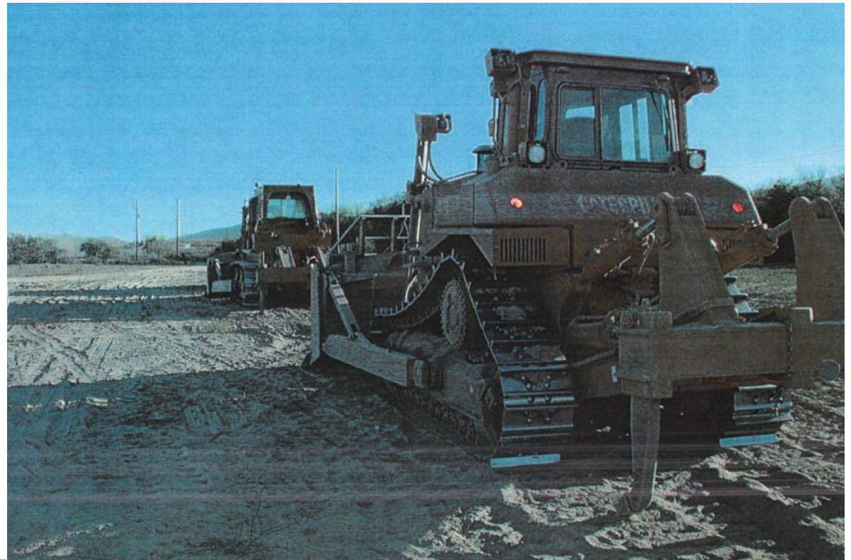
These were among the bulldozers used to clear hundreds of acres of land in violation of state environmental laws.
