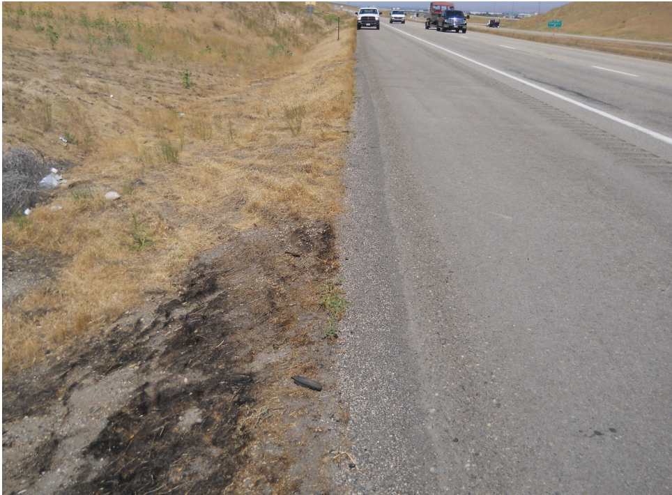
Example of a typical fire started on the roadside in an untreated area (MM 66 Fire in 2012).
