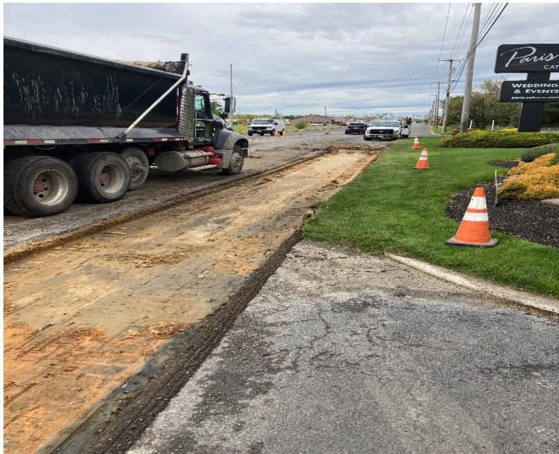
Figure 1: Contractor milling north of New Freedom rd. on Berlin Cross Keys Rd.
