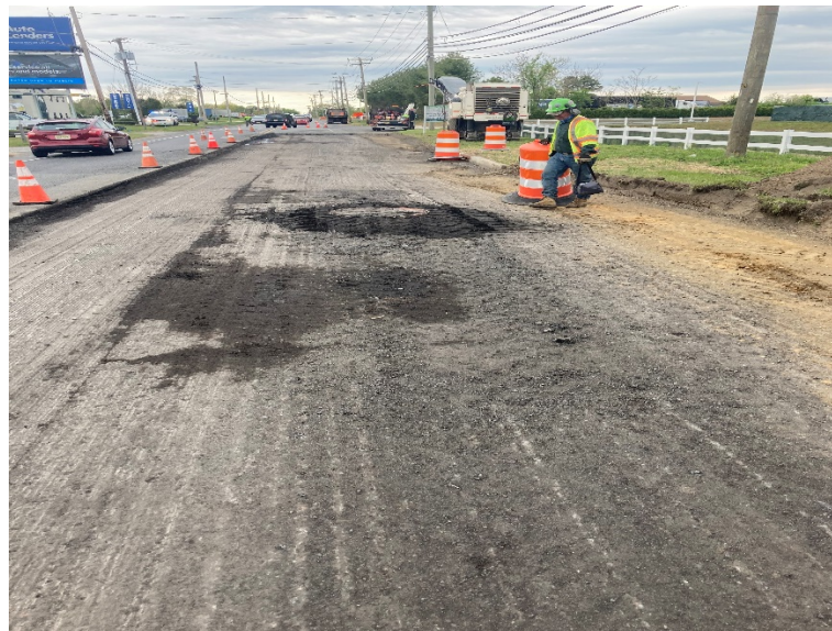
Figure 6&7: Southbound lane and shoulder milled by contractor south of New Freedom Rd.
