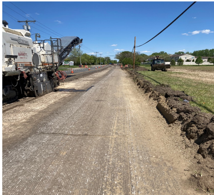
Figure 2&3: Contractor hit cement in the entire roadway except the shoulder after 4" of asphalt was removed.
