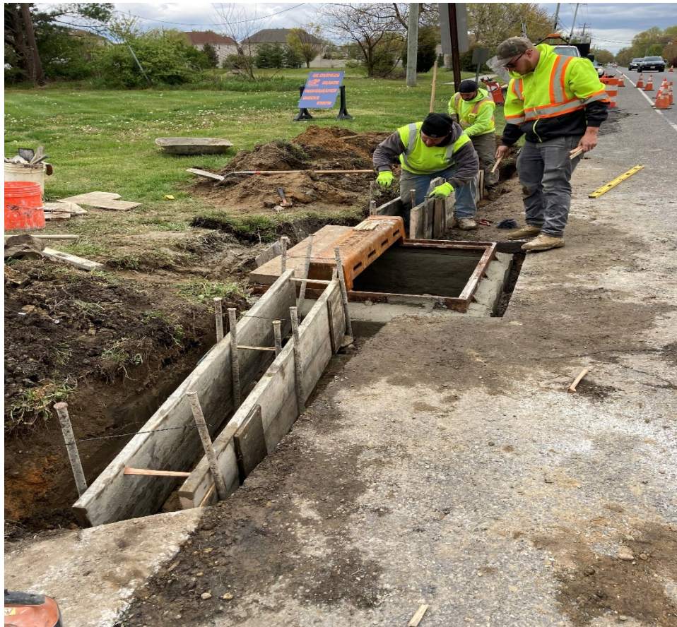
Figure 1: Contractor installed Bicycle Safe Grate and Curb Piece, adding forms for concrete.
