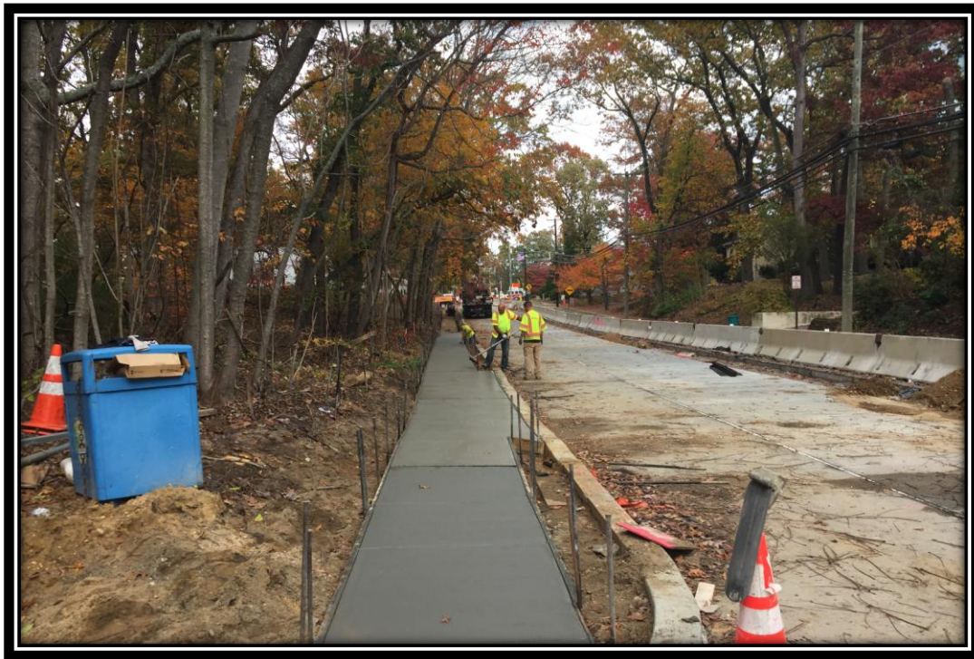
Figure: 1 – Installation of concrete sidewalk and driveway apron along the southbound lane in the vicinity of the intersection with Cloverdale Avenue
