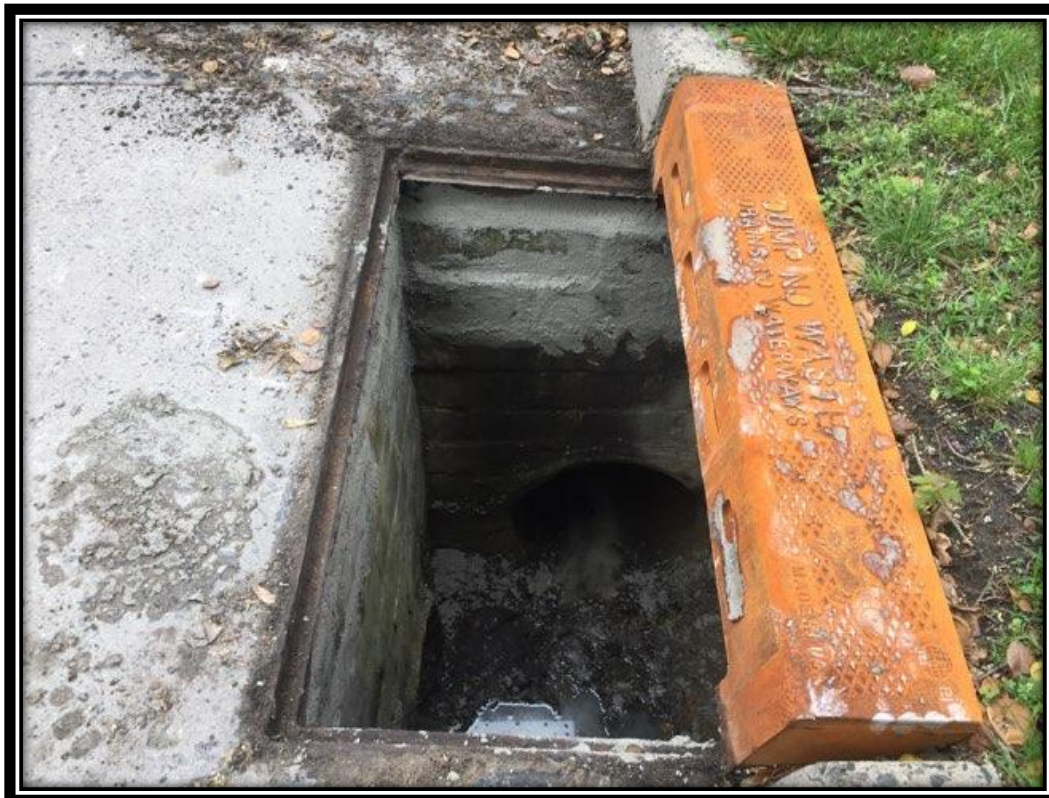
Figure: 1 – Resetting of an existing type 'B' inlet casting in the northbound lane approaching the intersection with Turnersville-Hickstown Road
