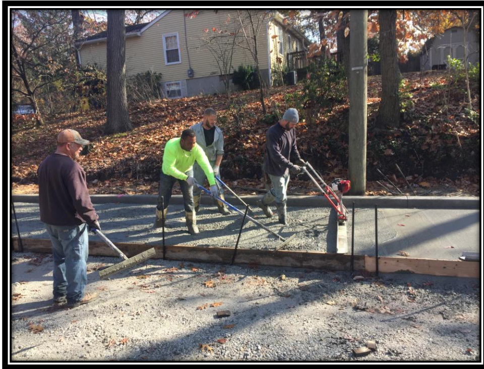
Figure: 2 – Installation of concrete surface course in the northbound shoulder in the vicinity of the intersection with Cloverdale Avenue
