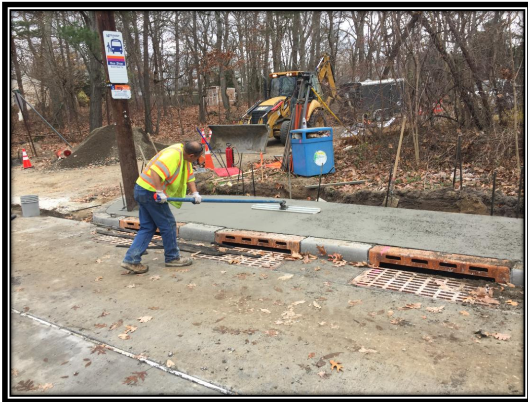
Figure: 1 – Installation of concrete sidewalk along the northbound lane at the intersection with Cloverdale Avenue
