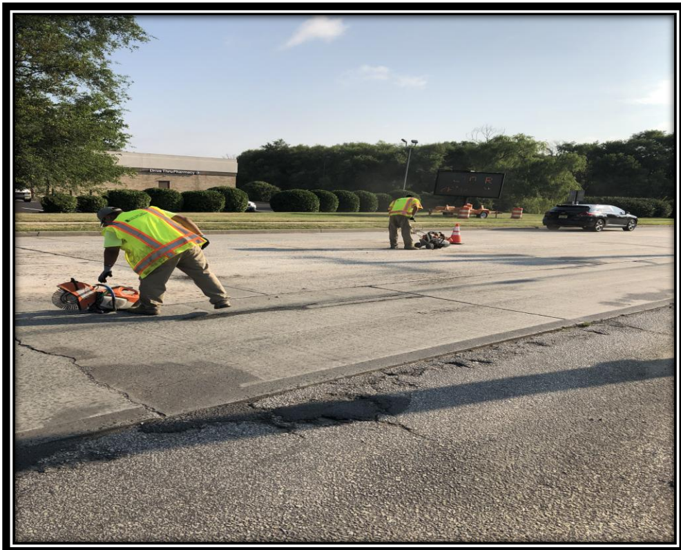
Figure: 1 – Sawcutting of existing joints in preparation for sealant installation in the northbound lane at the intersection with Erial New Brooklyn Road
