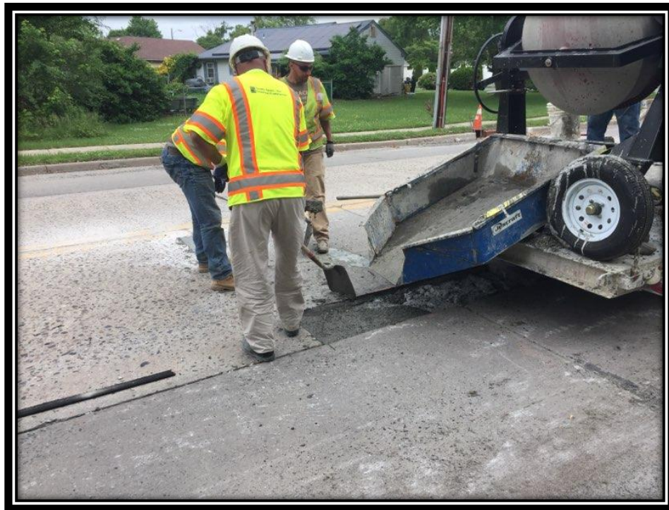
Figure: 3 – Partial depth concrete slab repairs in the northbound lane between Danbury Drive and Shultz Avenue
