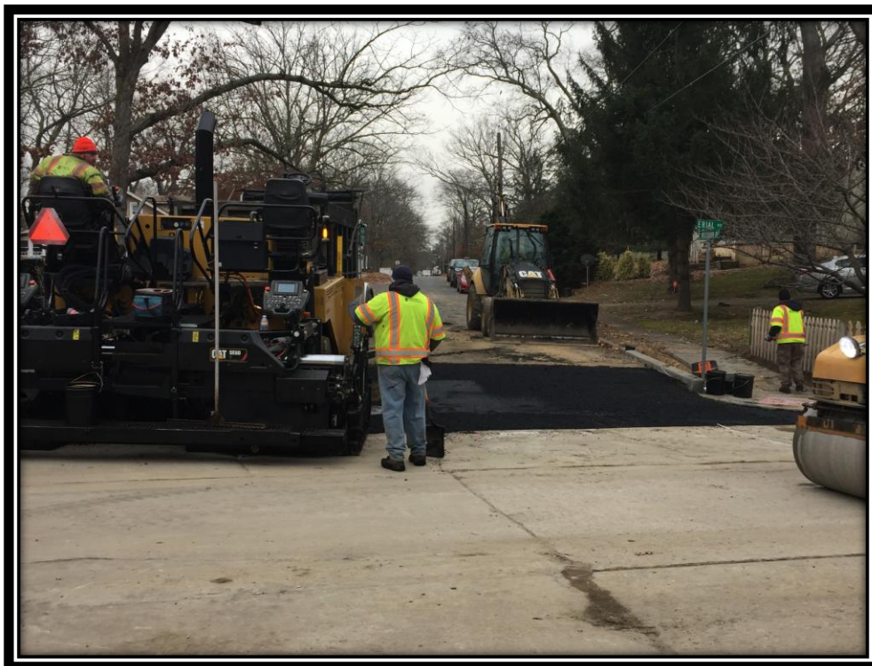
Figure: 3 – Installation of HMA 19M64 base course at the intersection with Woodburn Avenue
