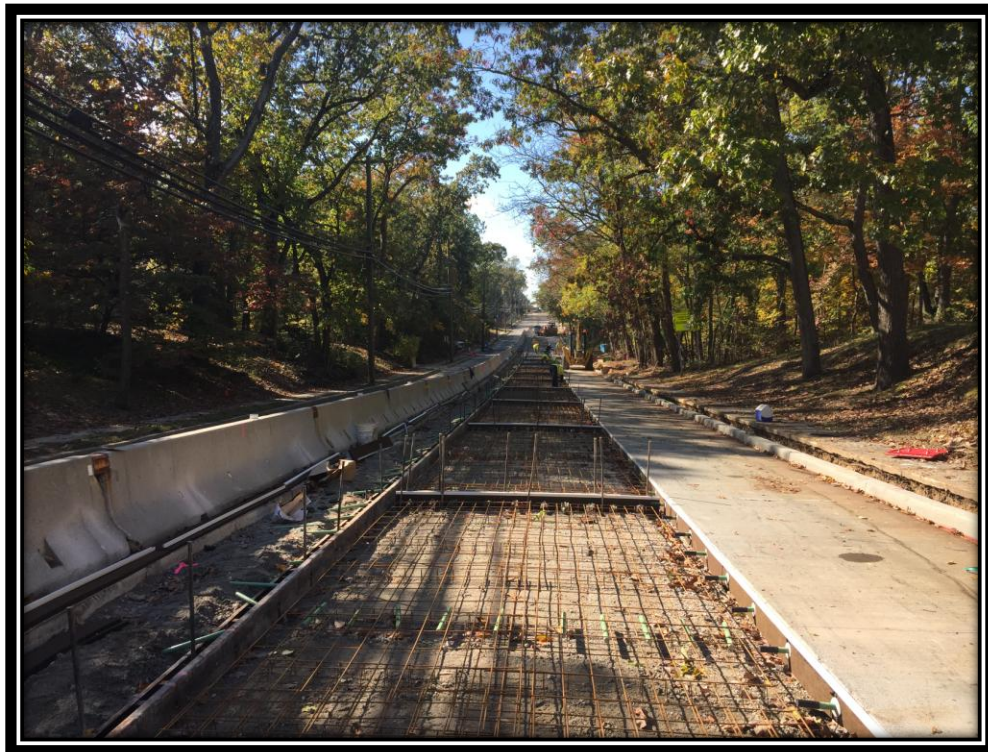
Figure: 1 – Installation of reinforcement and expansion joint material prior to the installation of concrete surface course in the southbound travel lane in the vicinity of the intersection with Cloverdale Avenue
