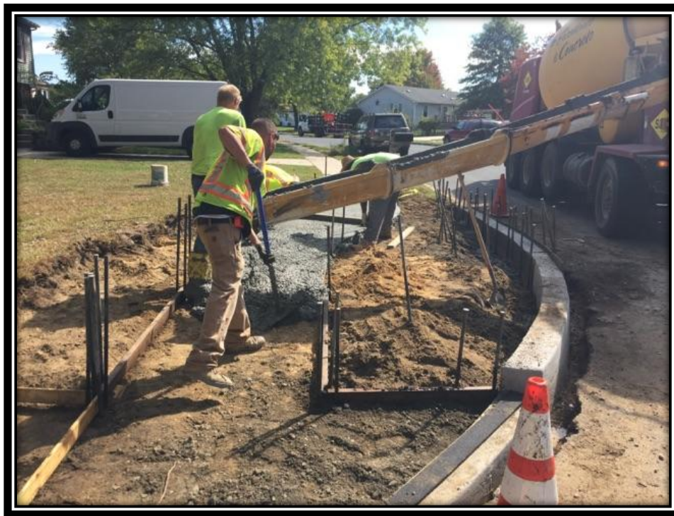
Figure: 3 – Installation of concrete sidewalk along the eastbound lane at the southwest corner of the intersection with Danbury Drive
