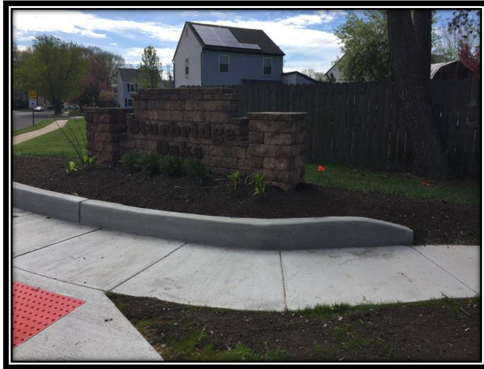
Figure: 2 – Topsoil and seed restoration at the newly installed ADA ramp at the intersection with Bromley Drive
