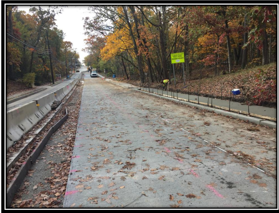
Figure: 2 – Installation of concrete sidewalk along the southbound travel lane in the vicinity of the intersection with Cloverdale Avenue
