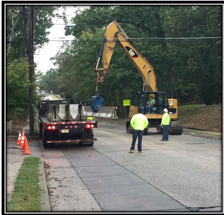
Figure: 1 – Installation of traffic control measures in the vicinity of the intersection with Cloverdale Avenue
