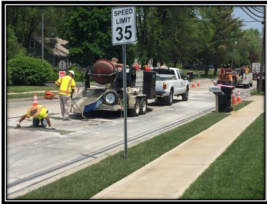
Figure: 2 – Partial depth concrete slab repairs in the northbound lane between Erial New Brooklyn Road and Pleasantview Drive
