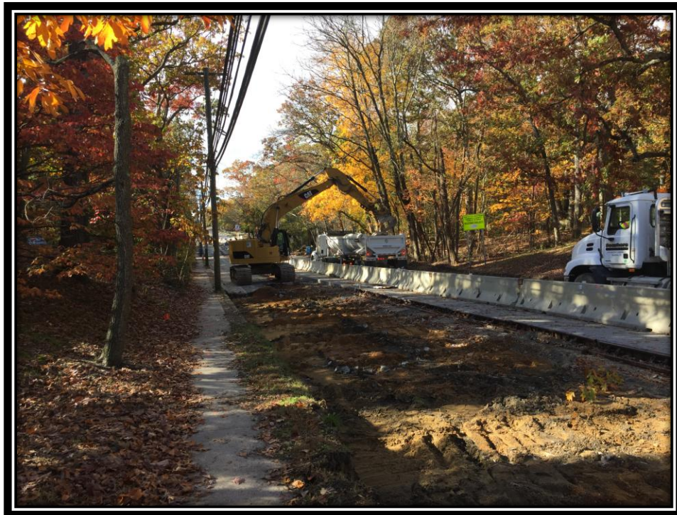
Figure: 3 – Removal of existing concrete roadway in the northbound lane in the vicinity of the intersection with Cloverdale Avenue
