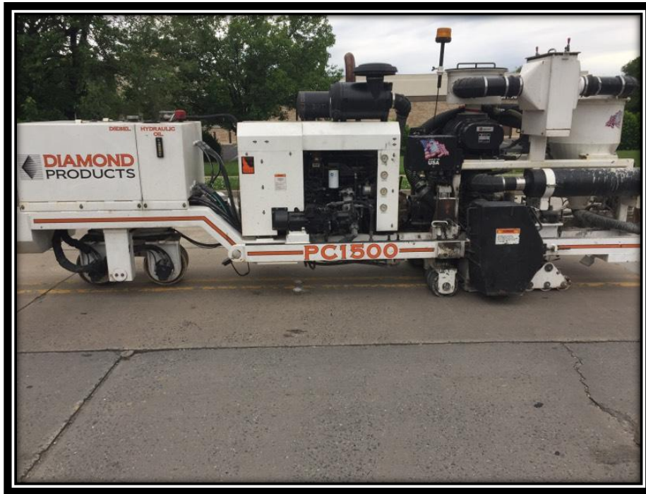
Figure: 2 – Diamond grinding of the concrete surface course in the northbound lane between Erial New Brooklyn Road and Pleasantview Drive
