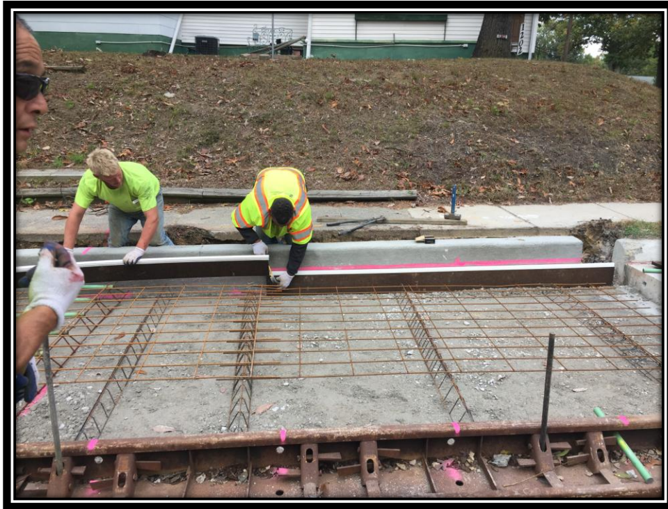
Figure: 2 – Installation of reinforcement and expansion joint prior to the installation of concrete surface course in the southbound lane in the vicinity of the intersection with Cloverdale Avenue
