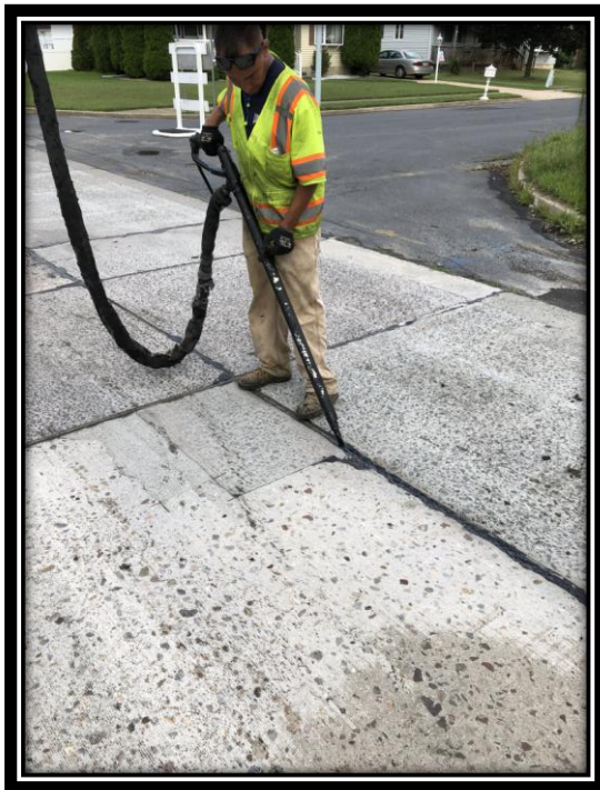
Figure: 3 – Sealing of the existing joints in the northbound lane between Bromley Drive and Turnersville Hickstown Road
