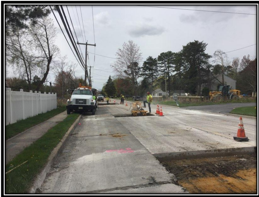
Figure: 1 – Preparation of full depth concrete slab repair along the northbound lane between Shultz Avenue and Bromley Drive
