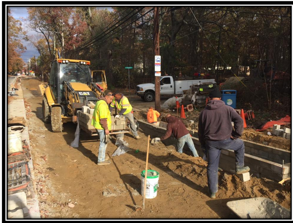
Figure: 1 – Reconstruction of existing drainage structure along the northbound lane at the intersection with Cloverdale Avenue
