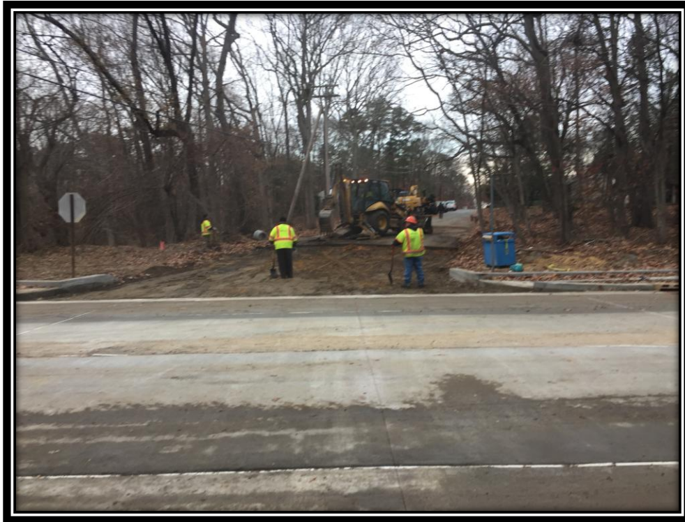
Figure: 2 – Excavation of the existing roadway at the intersection with Cloverdale Avenue
