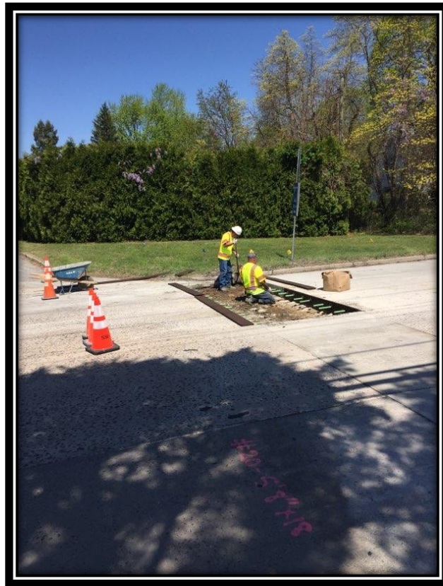
Figure: 1 – Preparation of full depth concrete slab repair along the southbound lane between Bromley Drive and Shultz Avenue
