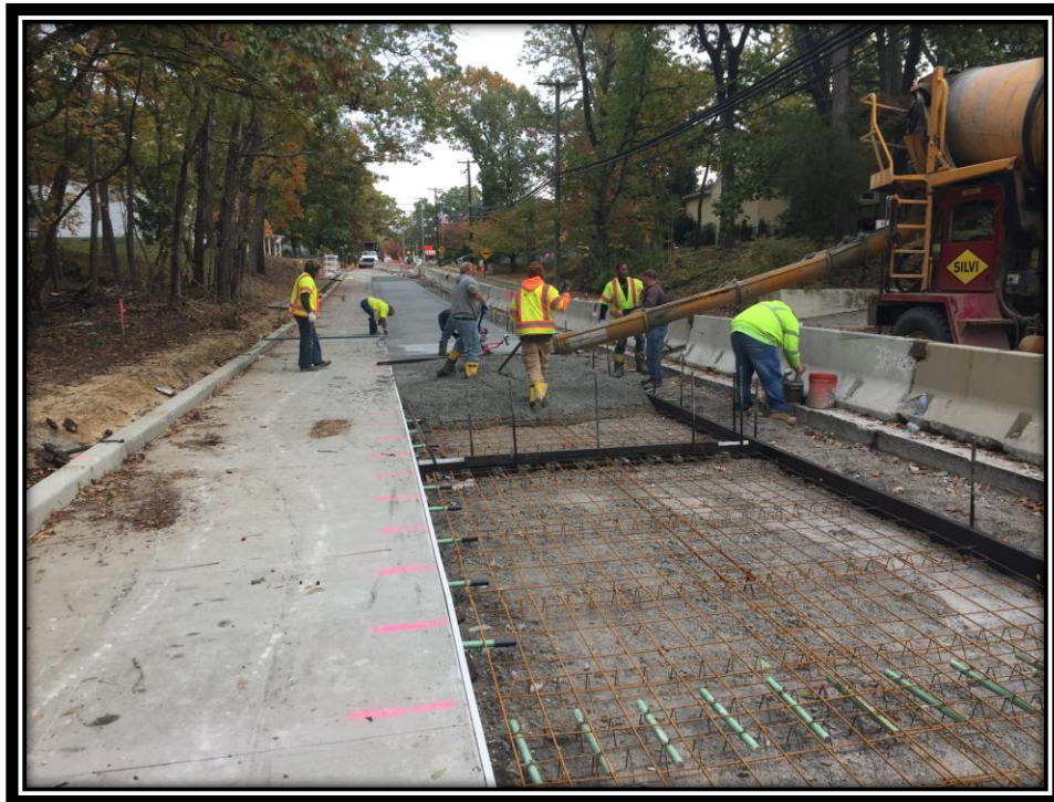
Figure: 3 – Installation of 8” thick concrete surface course in the southbound travel lane in the vicinity of the intersection with Cloverdale Avenue
