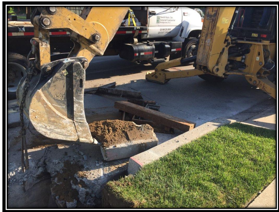
Figure: 3 – Removal of existing concrete slab in preparation of full depth concrete slab repair along the southbound lane between Bromley Drive and Shultz Avenue
