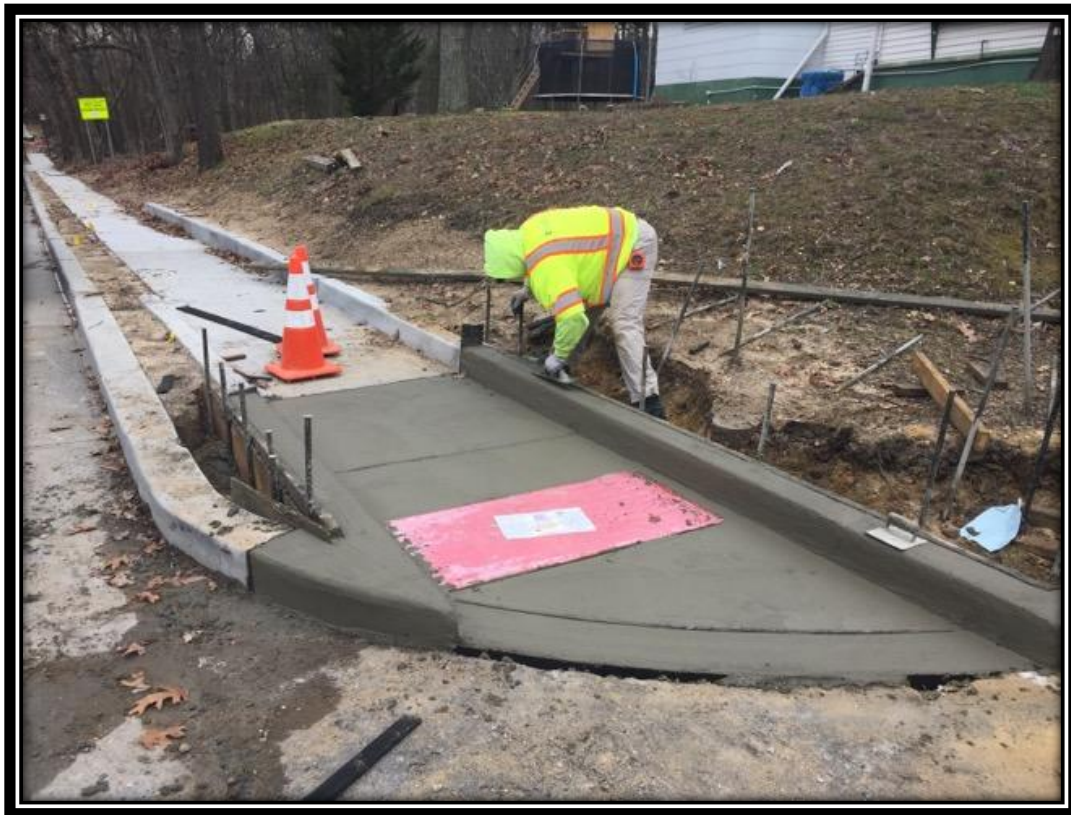
Figure: 1 – Installation of ADA ramp along the southbound lane at the intersection with Woodburn Avenue
