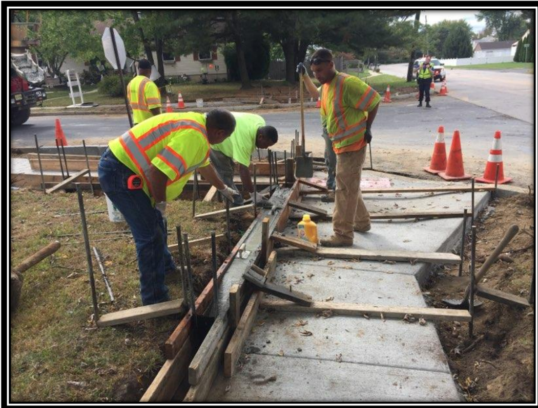
Figure: 1 – Installation of ADA ramp along the eastbound lane at the southwest corner of the intersection with Danbury Drive
