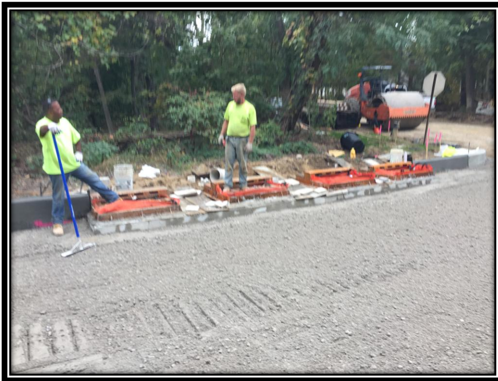
Figure: 1 – Installation of 8” thick dense graded aggregate base course in the southbound lane in the vicinity of the intersection with Cloverdale Avenue
