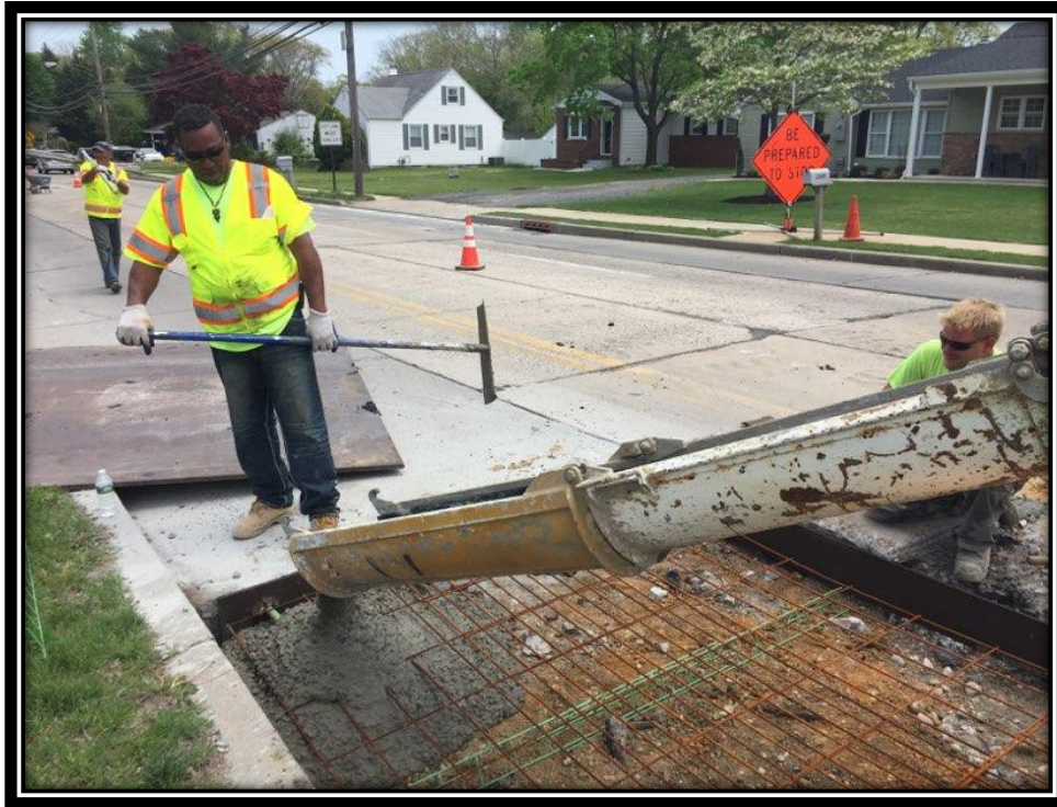
Figure: 2 – Full depth concrete slab repair along the southbound lane between Bromley Drive and Shultz Avenue
