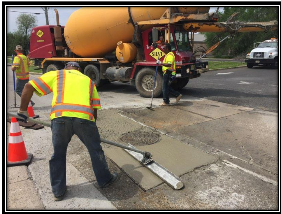
Figure: 3 – Full depth concrete slab repair along the southbound lane at the intersection with Pleasantview Drive
