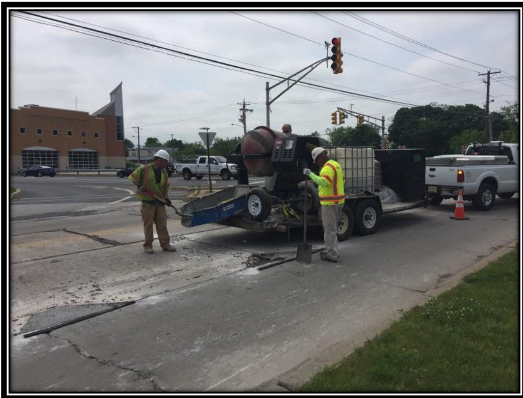
Figure: 1 – Partial depth concrete slab repairs in the southbound lane approaching the intersection with Erial New Brooklyn Road
