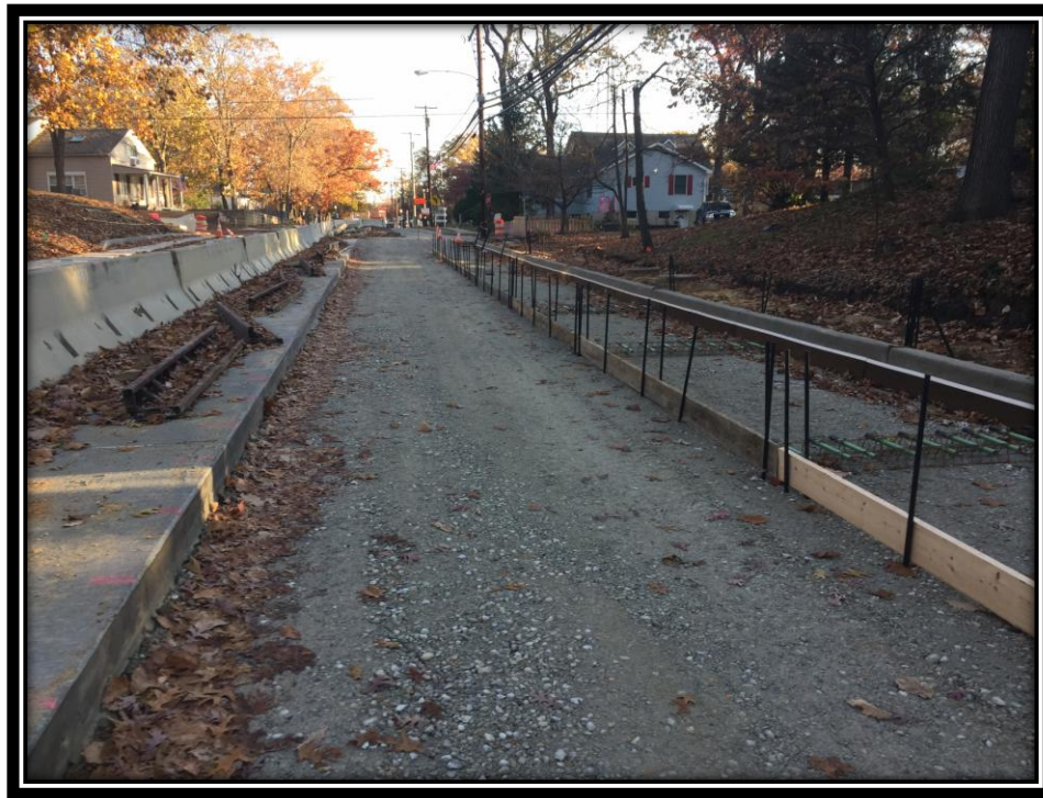
Figure: 1 – Installation of dowels in preparation of concrete surface course installation in the northbound shoulder in the vicinity of the intersection with Cloverdale Avenue
