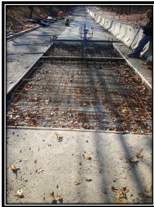
Figure: 1 – Wire mesh and dowel reinforcement of concrete surface course installation in the northbound travel lane in the vicinity of the intersection with Cloverdale Avenue
