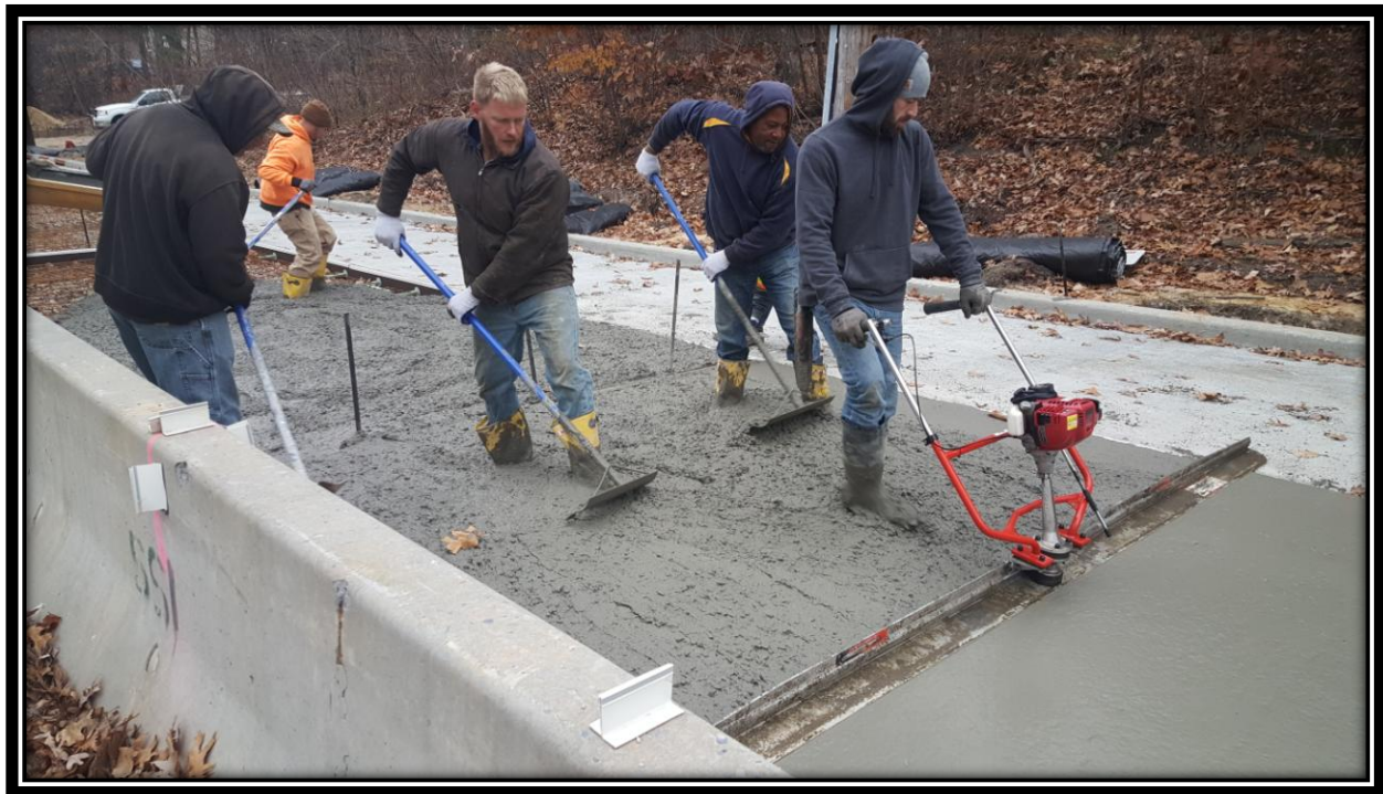
Figure: 3 – Finishing of concrete surface course in the northbound travel lane in the vicinity of the intersection with Cloverdale Avenue
