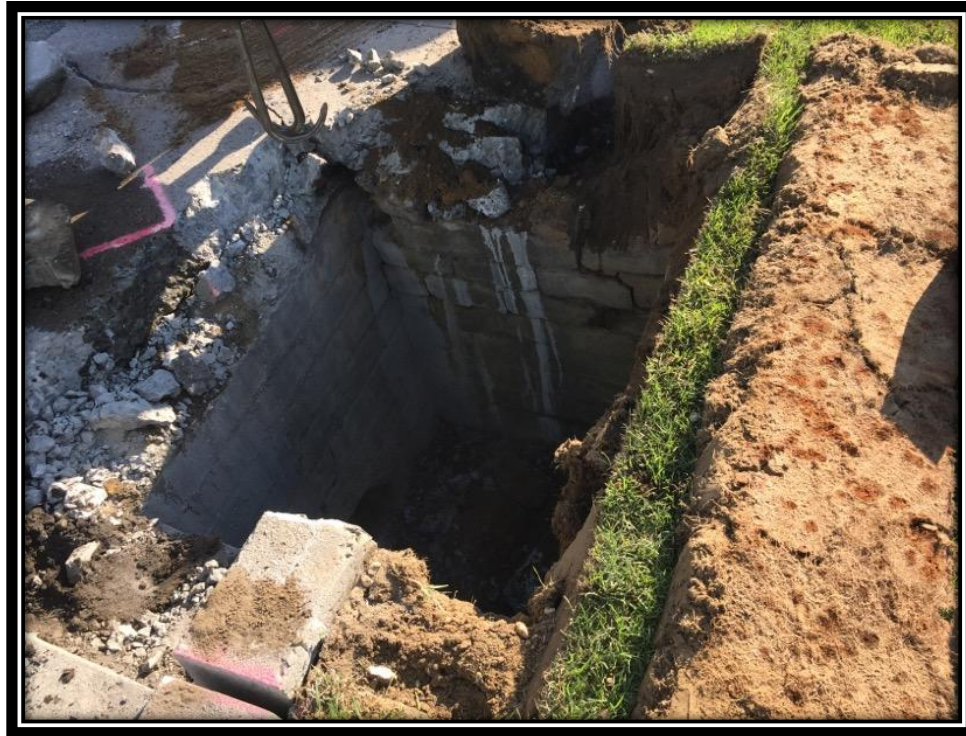
Figure: 2 – Inlet reconstruction including a new casting along the southbound lane between Bromley Drive and Shultz Avenue
