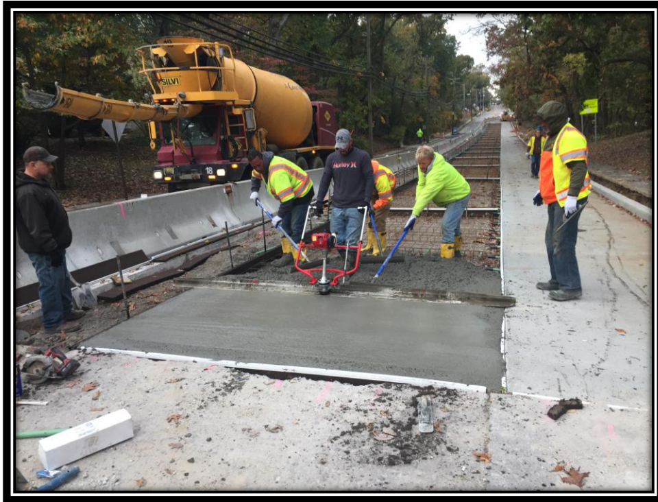
Figure: 2 – Installation of 8” thick concrete surface course in the southbound travel lane in the vicinity of the intersection with Cloverdale Avenue
