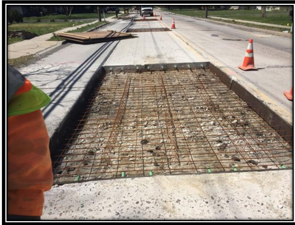
Figure: 2 – Full depth concrete slab repair along the northbound lane between Erial - New Brooklyn Road and Pleasantview Drive
