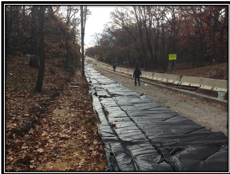
Figure: 3 – Installation of thermo blankets to protect the newly installed concrete surface course in the northbound shoulder in the vicinity of the intersection with Cloverdale Avenue
