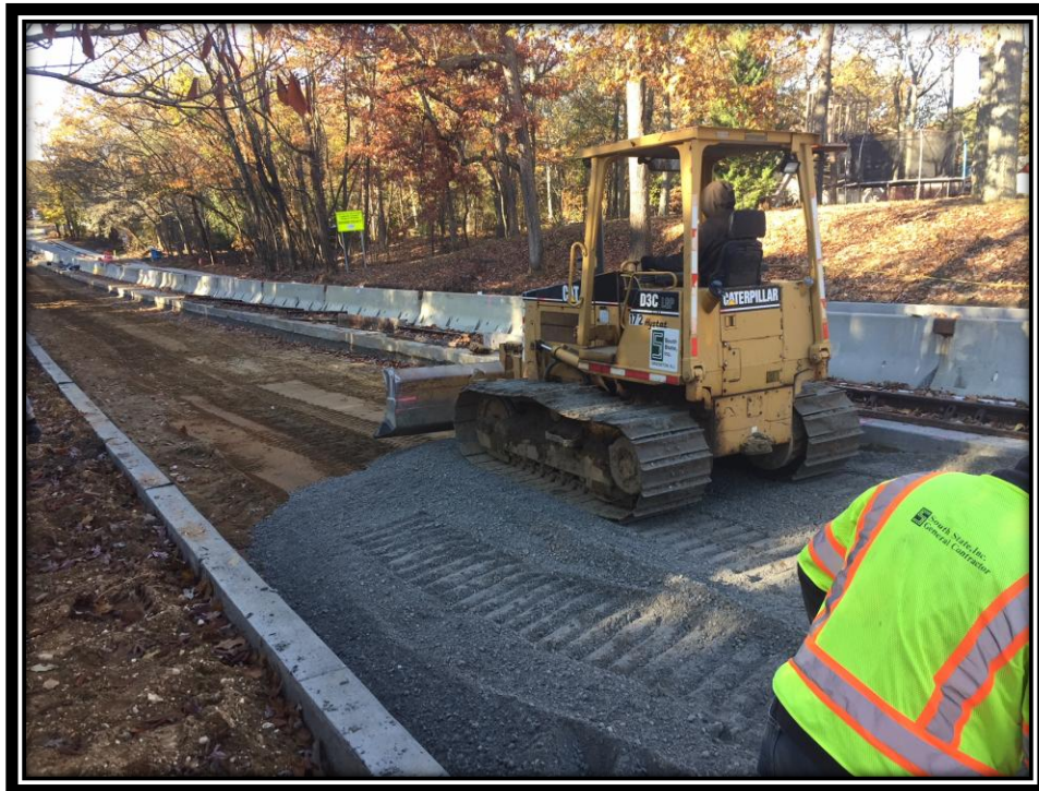
Figure: 3 – Installation of 8" thick dense graded aggregate along the northbound lane between Woodburn Avenue and Cloverdale Avenue
