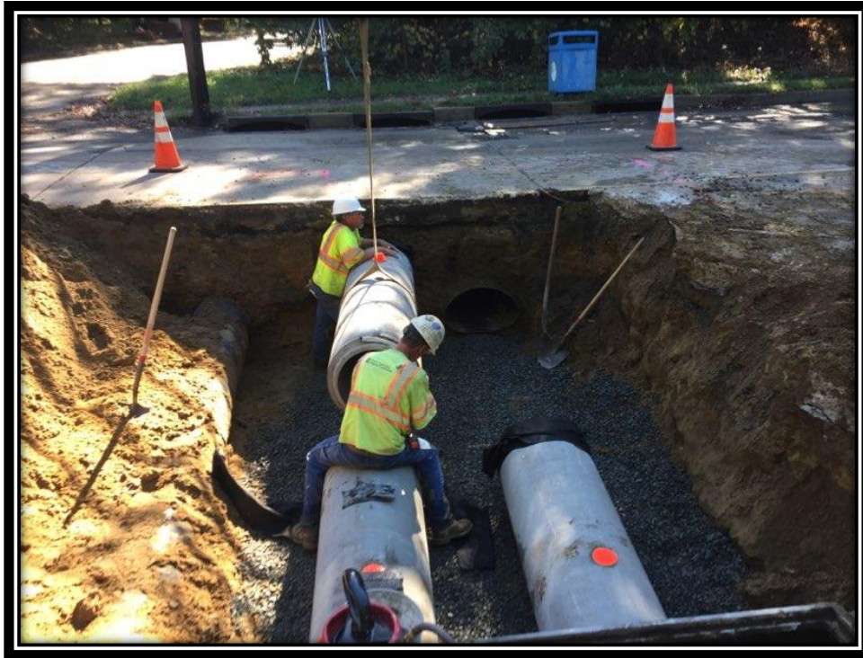
Figure: 2 – Installation of triple 18” RCP storm sewers at the intersection with Cloverdale Avenue
