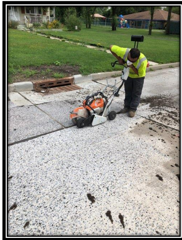
Figure: 1 – Sawcutting of existing joints in preparation for sealant installation in the southbound lane between Turnersville Hickstown Road and Erial New Brooklyn Road
