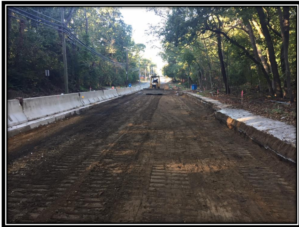
Figure: 3 – Rough grading of the roadway subbase in the southbound lane in the vicinity of the intersection with Cloverdale Avenue
