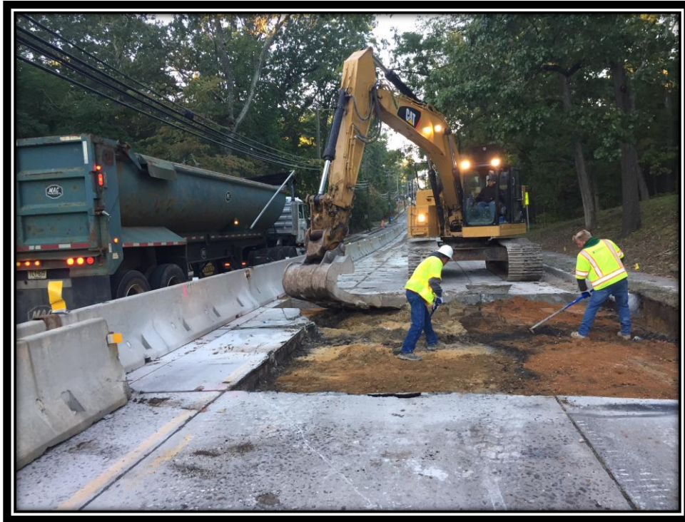
Figure: 2 – Removal of existing concrete surface course in the southbound lane in the vicinity of the intersection with Cloverdale Avenue
