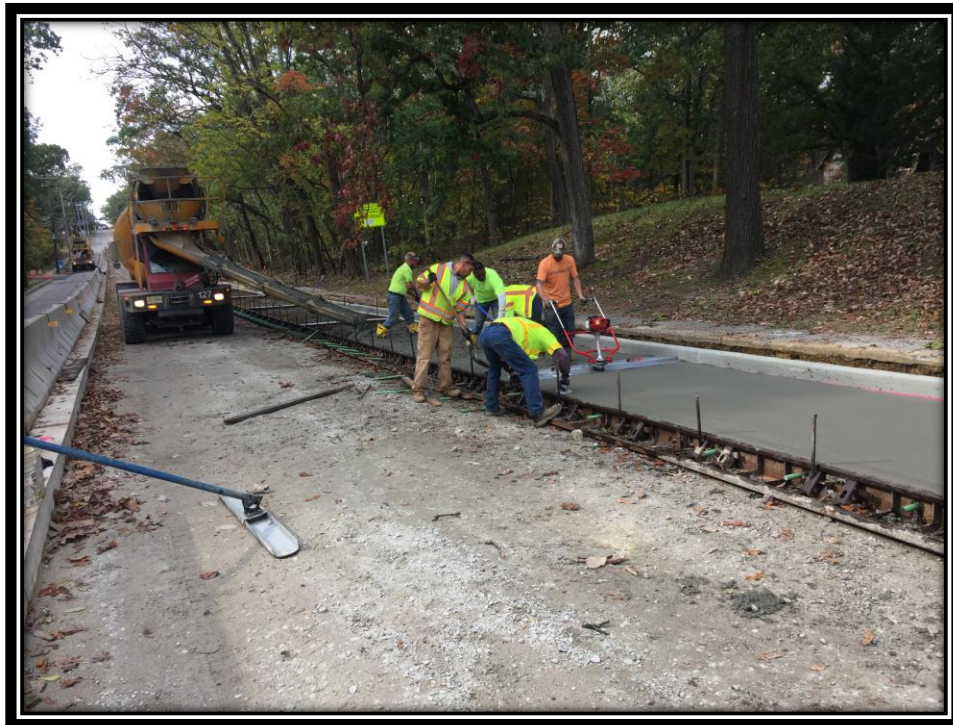
Figure: 3 – Installation of 8” thick concrete surface course in the southbound lane in the vicinity of the intersection with Cloverdale Avenue
