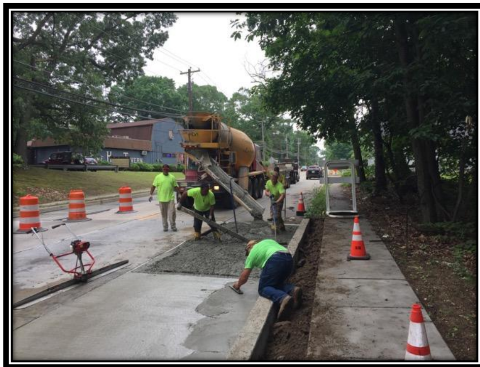
Figure: 3 – Full depth concrete slab replacement in the southbound lane between Cloverdale Avenue and Buttonwood Avenue
