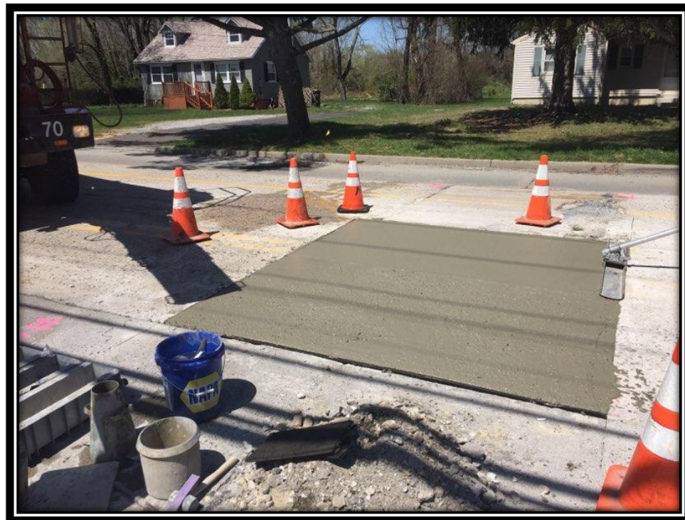
Figure: 3 – Full depth concrete slab repair along the northbound lane between Erial - New Brooklyn Road and Pleasantview Drive
