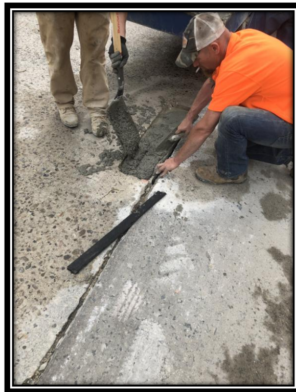
Figure: 3 – Partial depth concrete slab repairs in the southbound lane between Pleasantview Drive and Erial New Brooklyn Road
