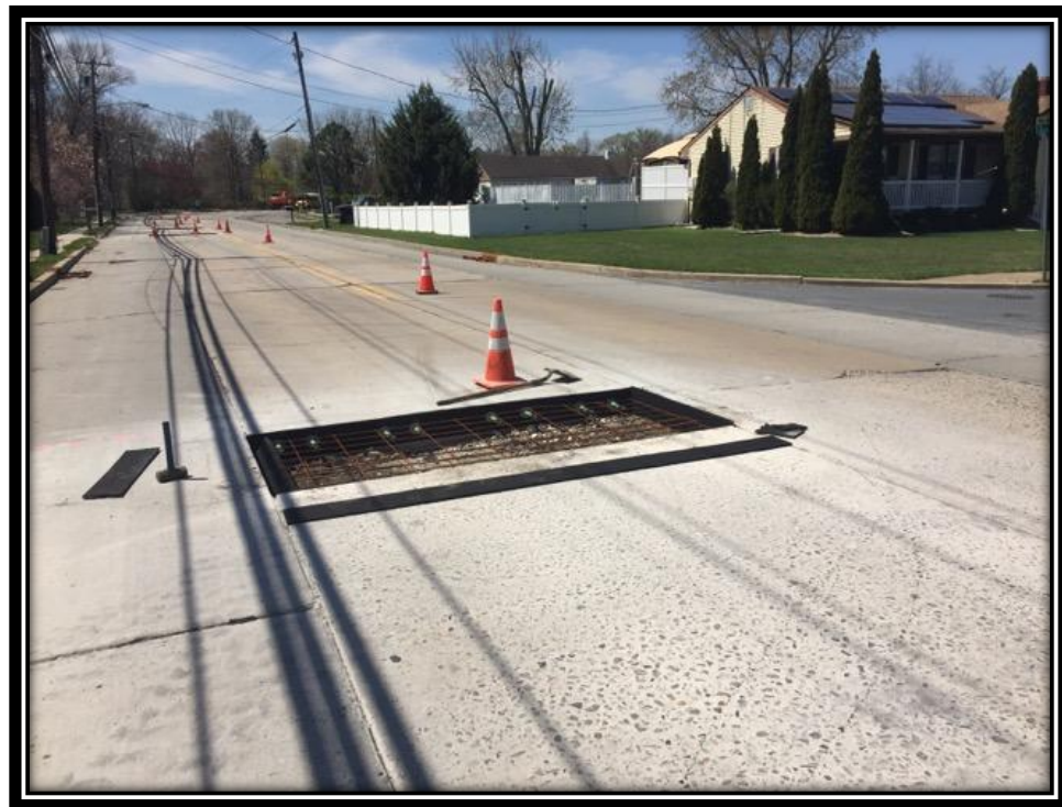
Figure: 3 – Full depth concrete slab repair along the northbound lane between Pleasantview Drive and Lee Lane
