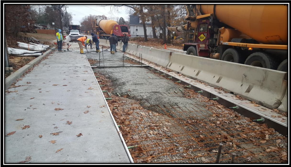
Figure: 2 – Installation of concrete surface course in the northbound travel lane in the vicinity of the intersection with Cloverdale Avenue
