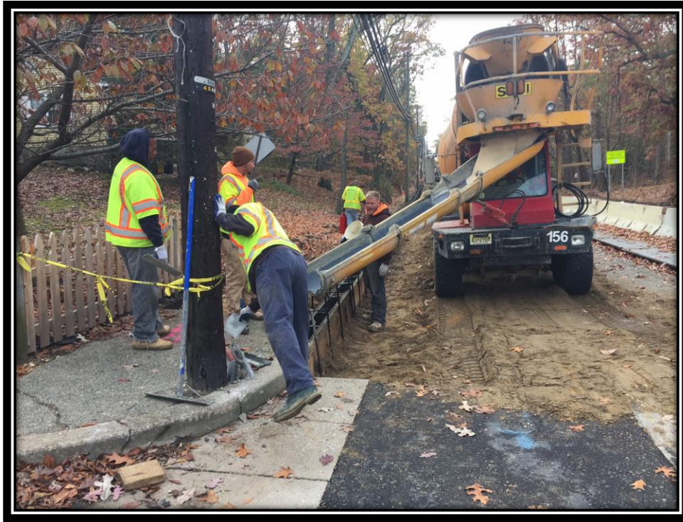
Figure: 2 – Installation of concrete curb along the northbound lane between Woodburn Avenue and Cloverdale Avenue
