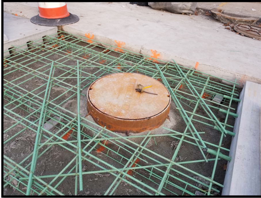
Slab K60 rebar set for poured in place slab replacement due to unforeseen condition of manhole.
