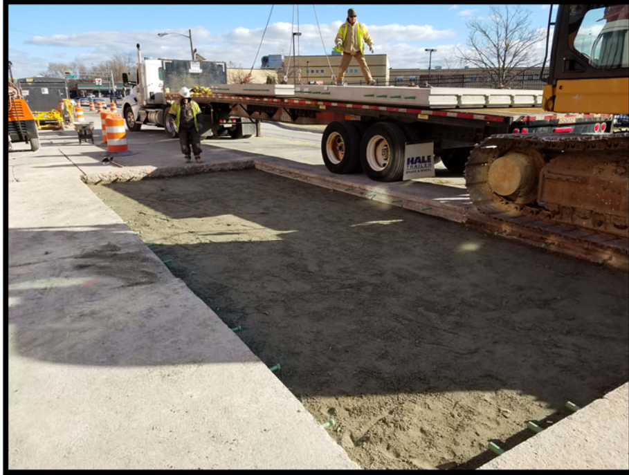
Phase 2 subbase prepared, dowels installed and new prefabricated slabs ready to be installed.
