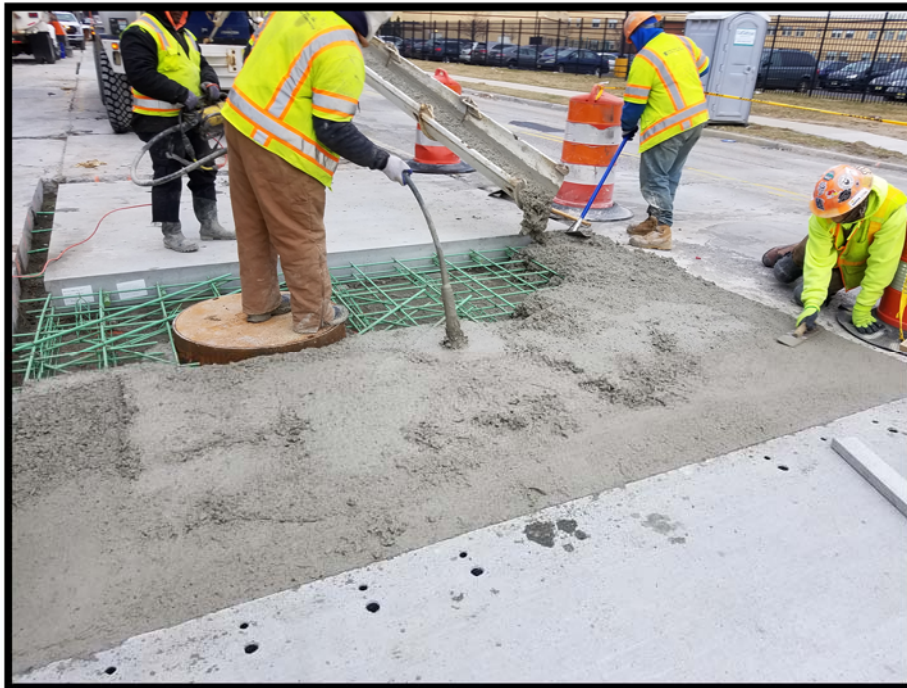
Slab K60 rebar set and concrete being poured in place per work directive associated with unforeseen condition of manhole.
