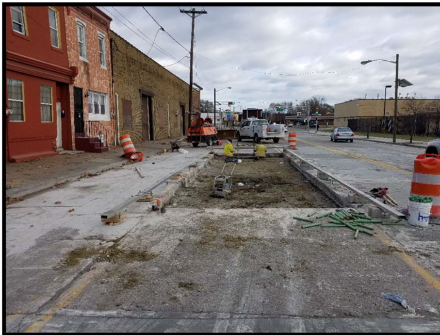
Phase 2 Slab preparation underway. Note work area encroaching on westbound travel lane resulting in police mandated lane closure and detour.
