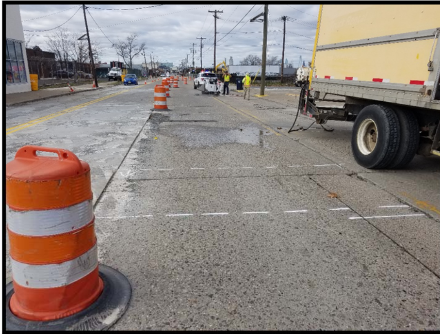
Phase 2 Temporary Traffic Striping and Drums installed. Traffic shifted to southernmost lanes and work zone in northernmost lanes. Sawcutting of Phase 2 slabs underway.
