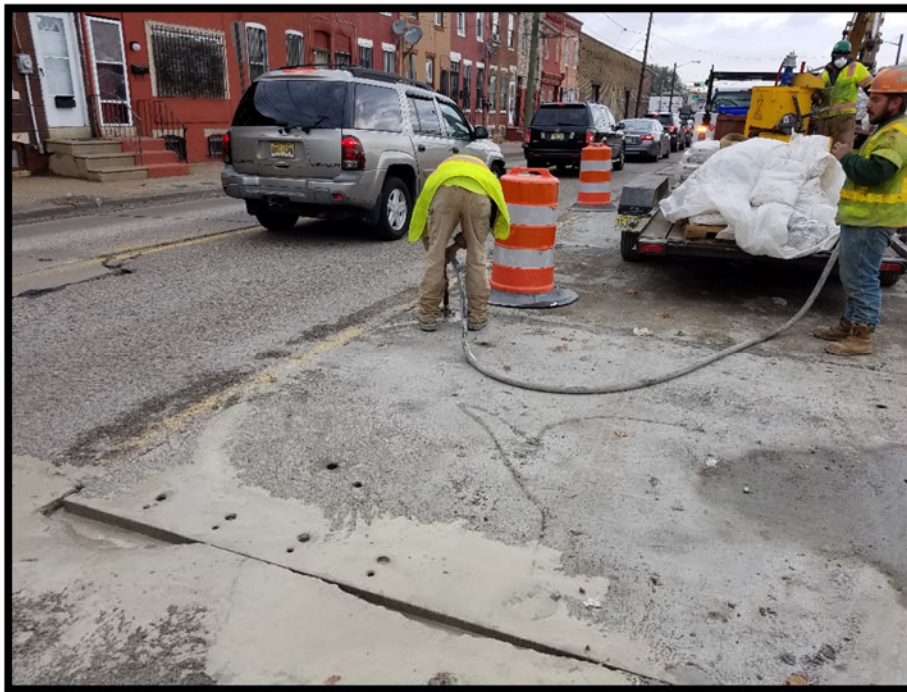
Pressure grouting of slab underside, joints and dowel pockets underway in Phase 1 work area.
