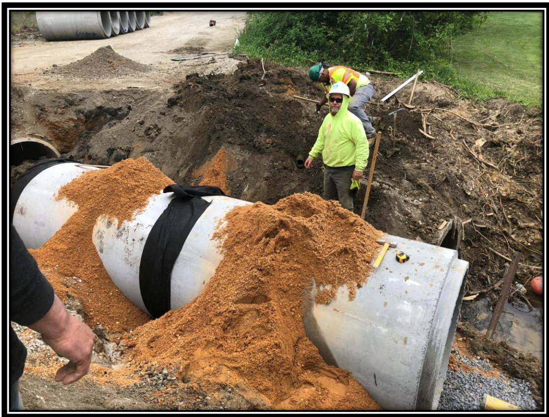
Figure: 1 – Installation of 48” RCP at the culvert replacement adjacent to the Merchantville Country Club
