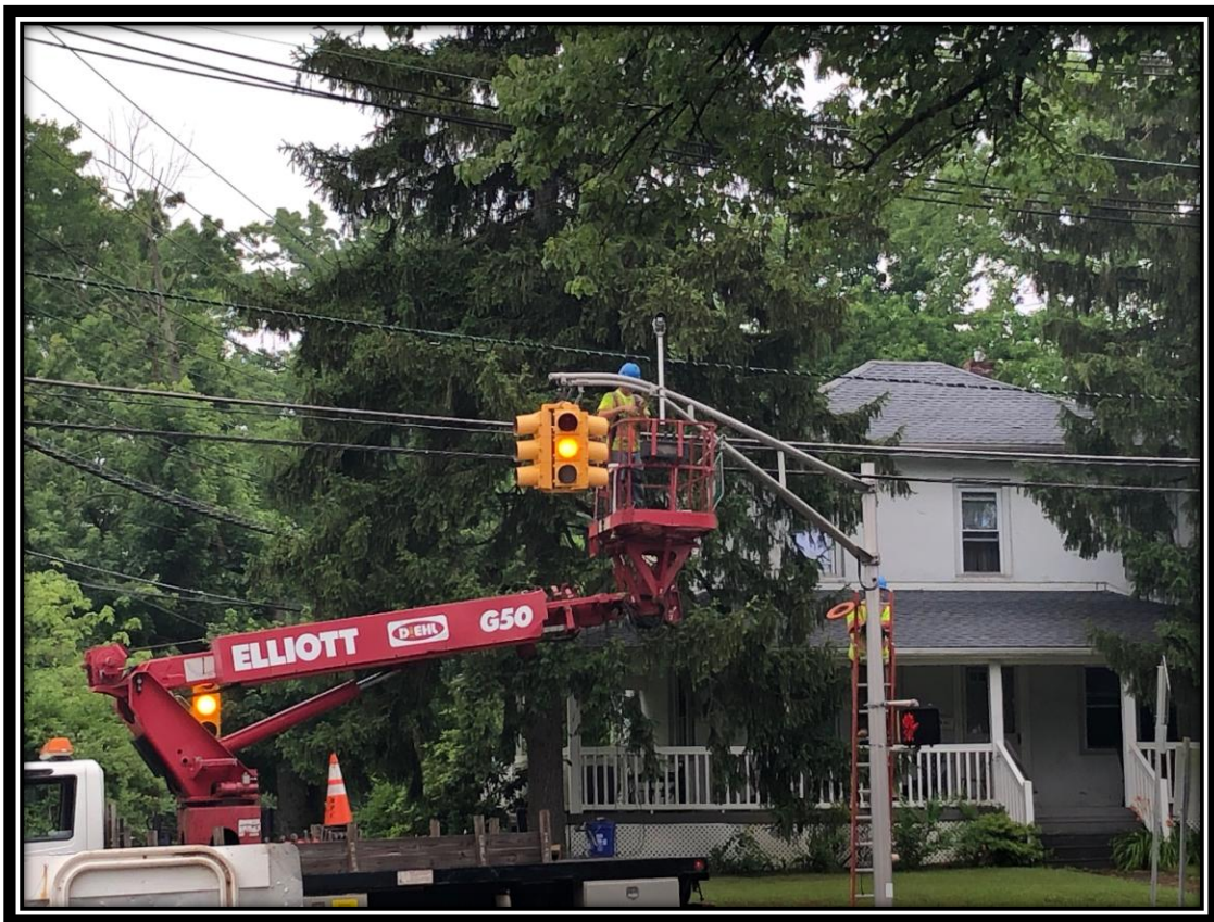
Figure: 1 – Installation of image detector camera at the intersection of Hampton Road and Chapel Avenue
