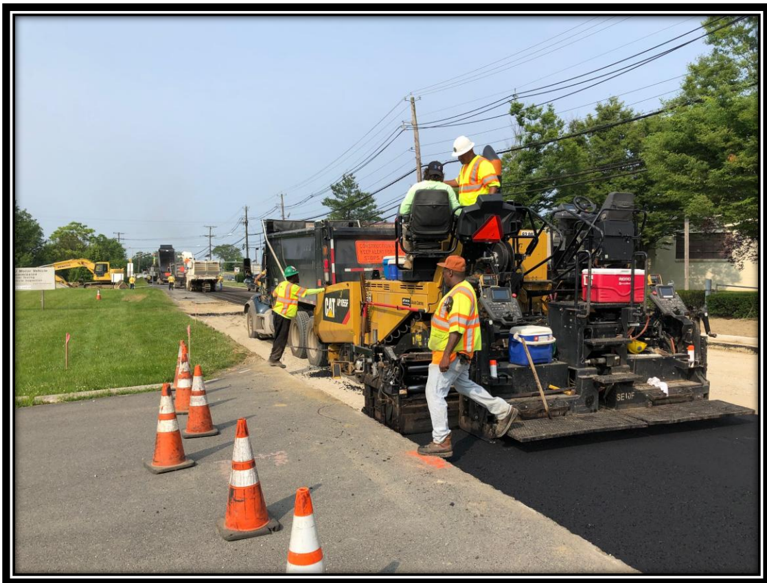
Figure: 1 – Installation of HMA 25M64 Base Course in the eastbound lane along the frontage of the Department of Motor Vehicles
