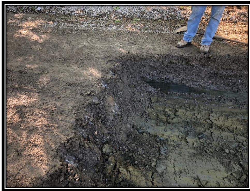
Figure: 2 – Over excavation of unsuitable subbase prior to installation of additional dense graded aggregate
