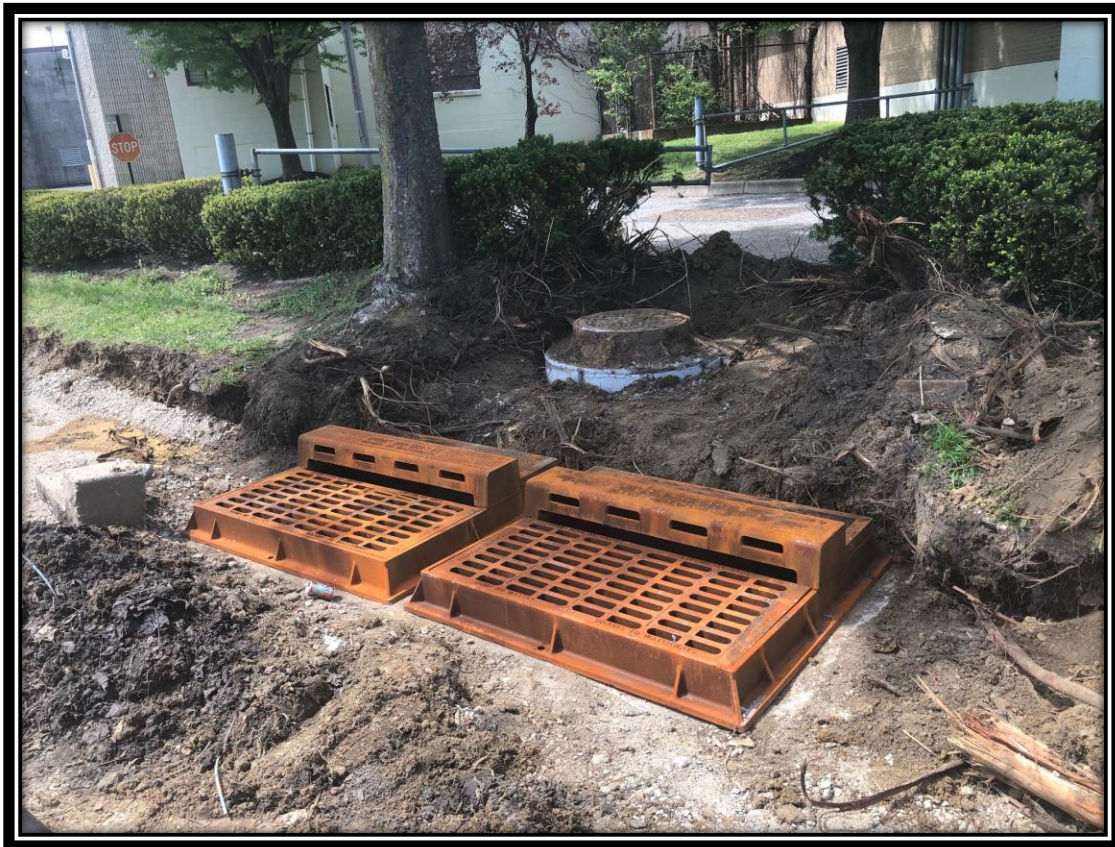
Figure: 1 – Reconstruction of storm sewer manhole and replacement of double 'B' castings along the northbound lane approaching Cuthbert Boulevard
