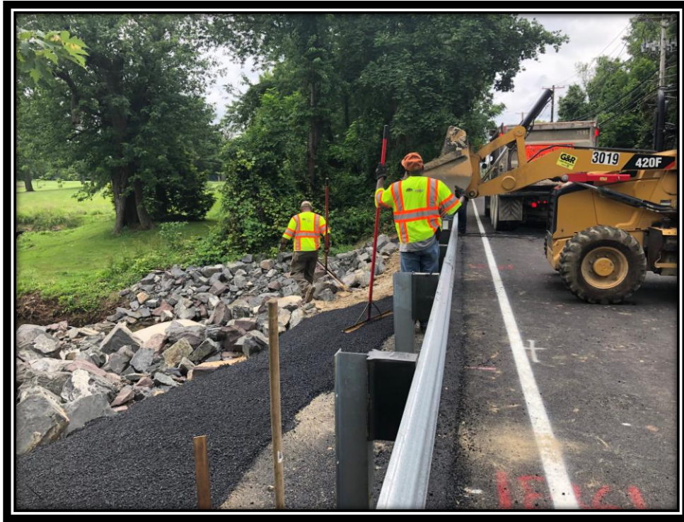
Figure: 2 – Installation of non vegetative surface behind newly installed guiderail over the twin 48” RCP culvert
