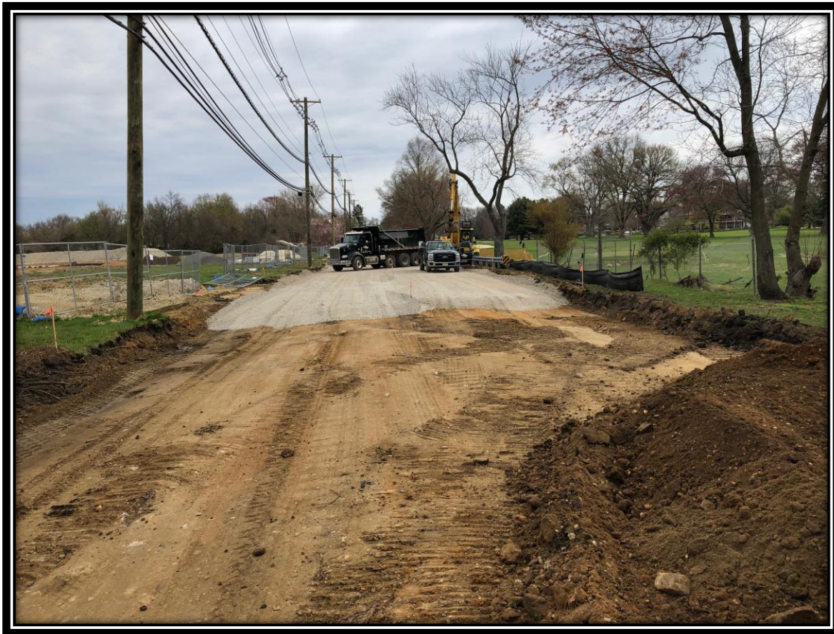
Figure: 1 – Roadway excavation and installation of 6” thick dense graded aggregate base course
