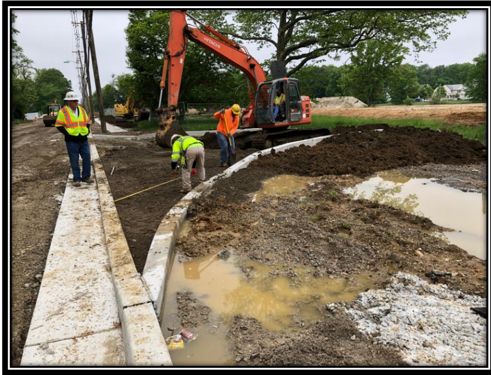
Figure: 2 – Installation of concrete curb & gutter and concrete vertical curb at future entrance to the proposed development along the westbound lane
