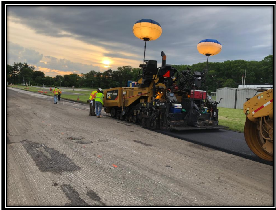
Figure: 3 – Installation of HMA 12.5M64 Surface Course in the eastbound lane along the frontage of the Department of Motor Vehicles
