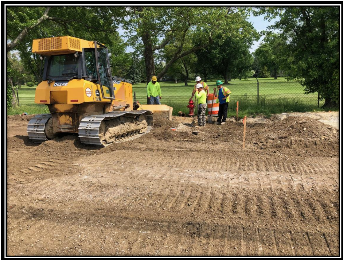
Figure: 1 – Fine grading of previously installed dense graded aggregate in preparation for base paving
