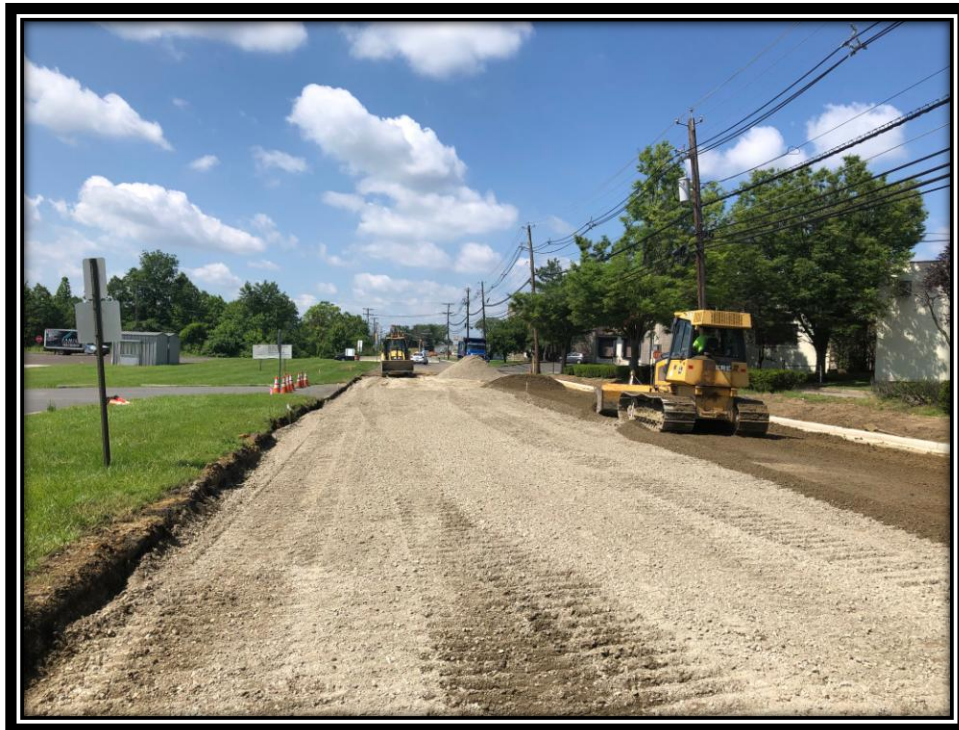
Figure: 3 – Installation of 6” thick dense graded aggregate base course along the frontage of the Department of Motor Vehicles
