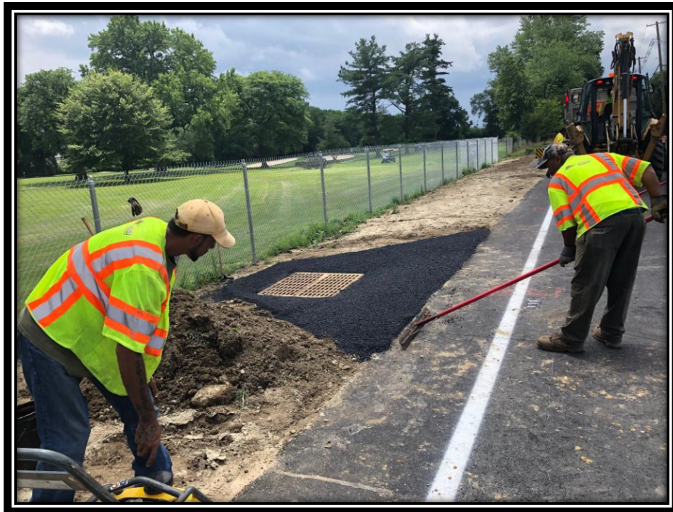
Figure: 3 – Installation of asphalt swale around newly installed ‘E’ inlet along the eastbound lane adjacent to the Merchantville Country Club
