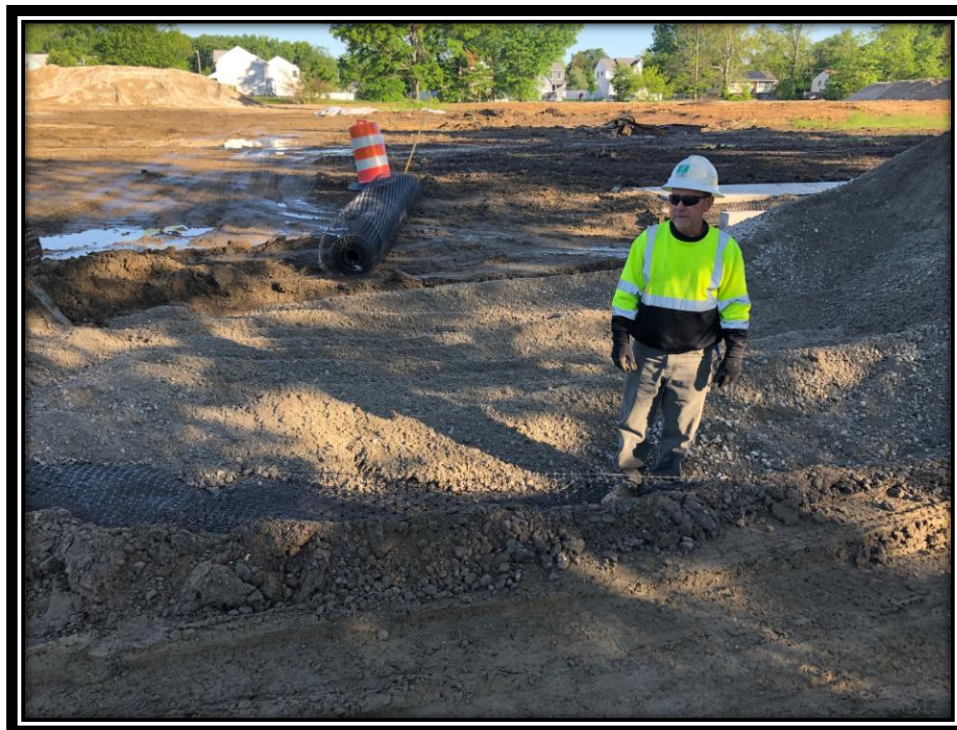
Figure: 3 – Installation of dense graded aggregate and geogrid prior to fine grading
