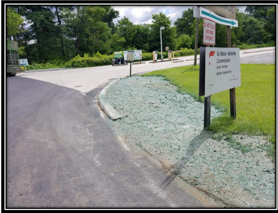
Figure: 2 – Installation of topsoil and hydro seed along the eastbound lane at the main entrance to the department of motor vehicles
