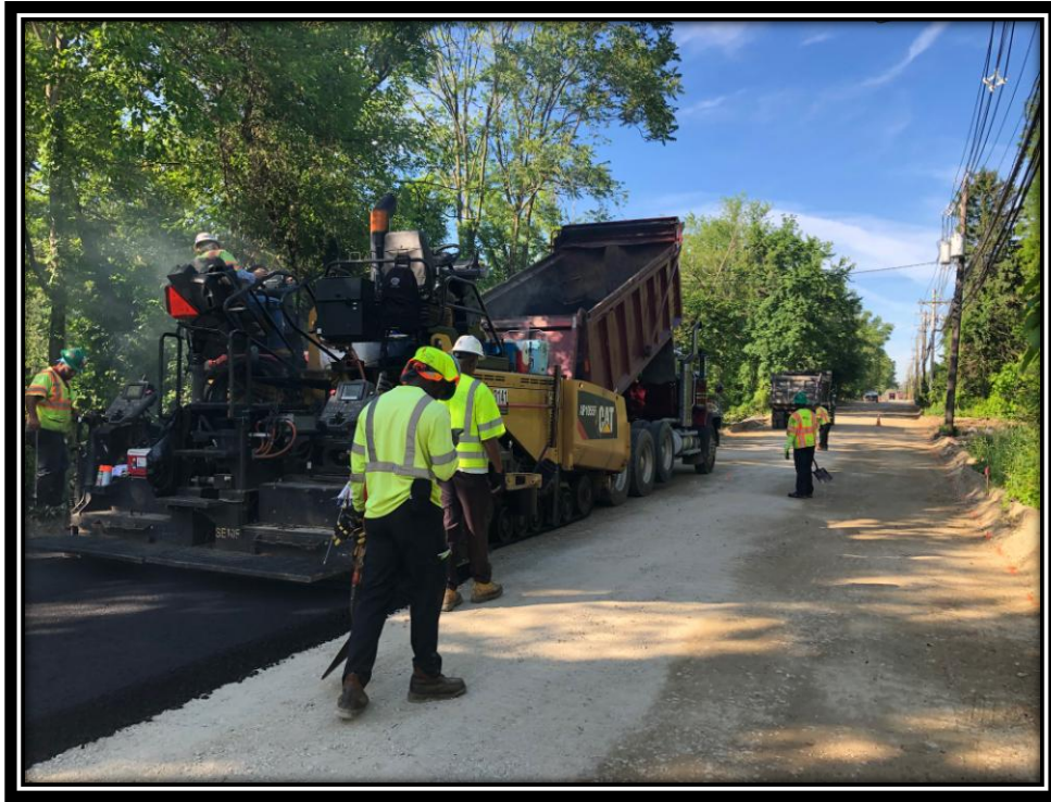
Figure: 2 – Installation of HMA 25M64 base course along the eastbound lane between Chapel Avenue and the Department of Motor Vehicles entrance
