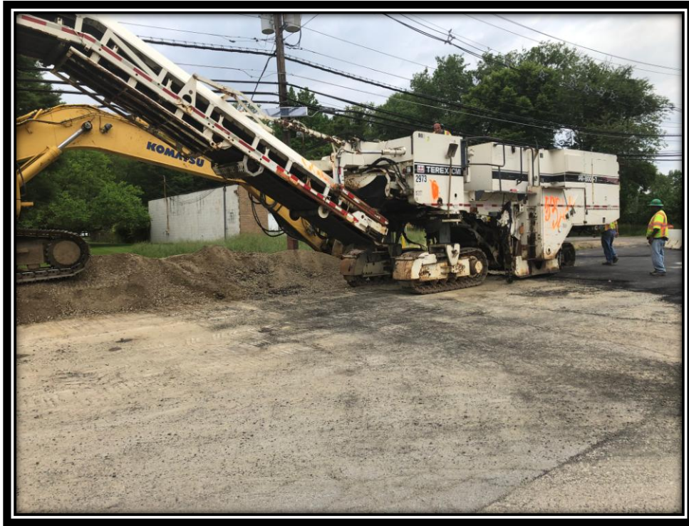
Figure: 2 – Milling of existing asphalt along the westbound lane along the frontage of the Department of Motor Vehicles
