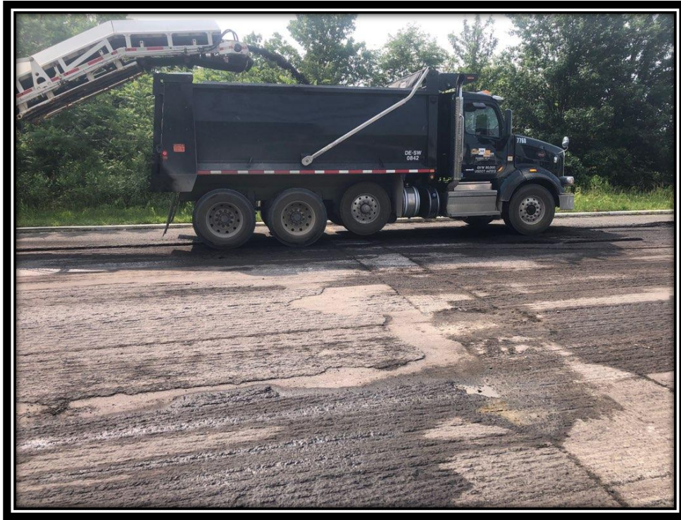
Figure: 2 – Milling of existing asphalt in the eastbound lane approaching the intersection with Cuthbert Boulevard
