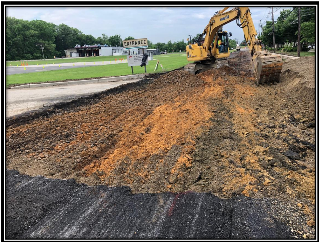
Figure: 1 – Roadway excavation along the frontage of the Department of Motor Vehicles
