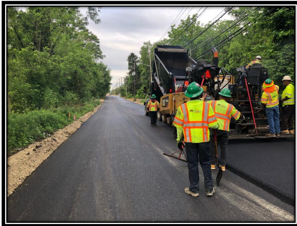
Figure: 3 – Installation of HMA 12.5M64 intermediate course along the westbound lane between Chapel Avenue and the Department of Motor Vehicles entrance
