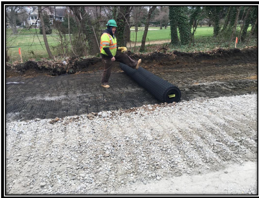
Figure: 3 – Installation of 6” thick dense graded aggregate base course in the southbound lane and pavement reinforcing geogrid along the northbound lane
