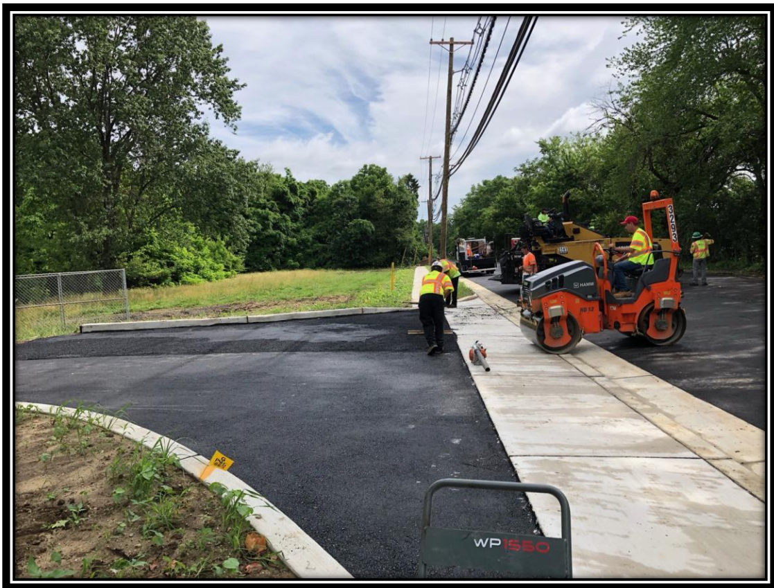
Figure: 1 – Installation of HMA driveway along the westbound lane at the eastern entrance to the proposed First Montgomery Development
