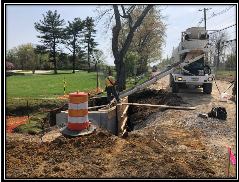
Figure: 2 – Installation of extended concrete wing wall off of previously installed headwall along the northbound lane
