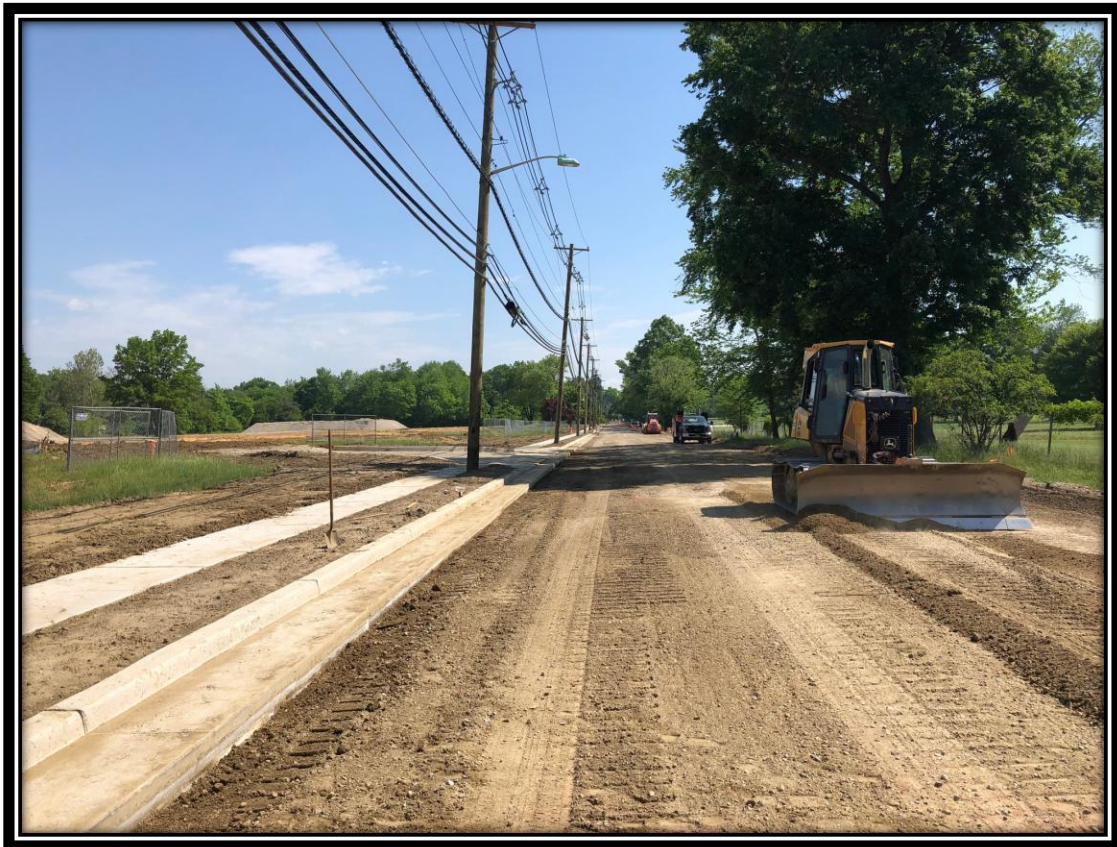
Figure: 1 – Fine grading of previously installed dense graded aggregate in preparation for base paving
