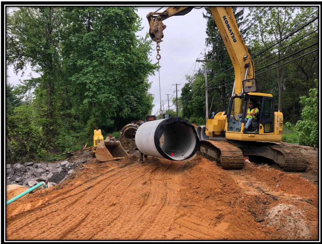
Figure: 1 – Installation of 48” RCP at the culvert replacement adjacent to the Merchantville Country Club
