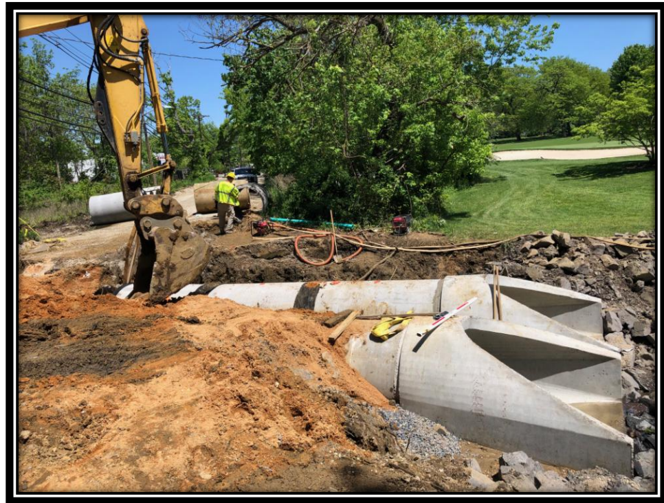
Figure: 3 – Installation of 48" RCP at the culvert replacement adjacent to the Merchantville Country Club
