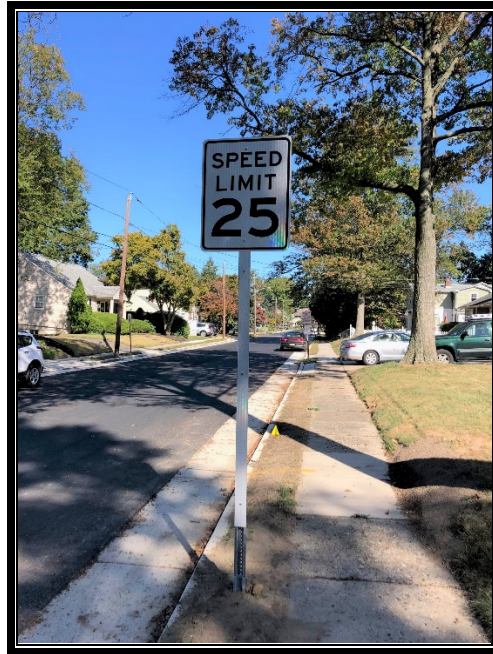
Figure 2: Contractor installed new speed limit signs with reflective posts on Avondale Avenue.
