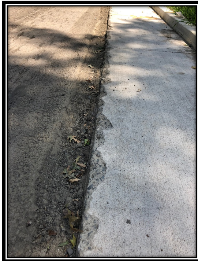
Figure 1: New gutter damaged by milling machine.
