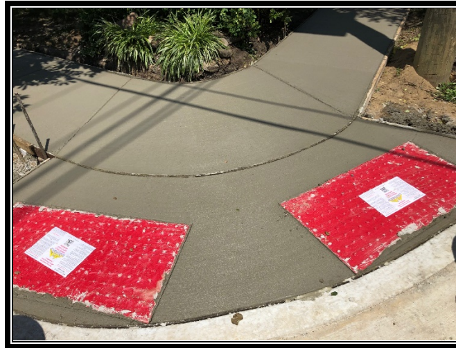
Figure 2: New handicap ramps at the intersection of Crystal Lake and Avondale Avenues.
