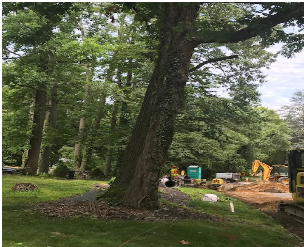
Figure: 1 – Utility pipe reconstruction on Central Ave on lake Blvd (Looking East side).
