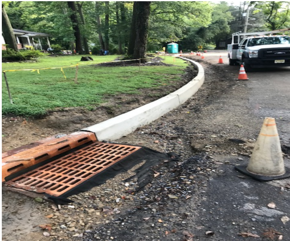
Figure: 2 – Reconstruct Curb and Handicap Ramp starting near Spring Landing Road (If and where directed)
