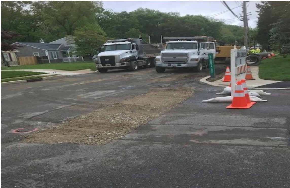
Figure: 3 – Utility pipe and 8” Water Main relocated Columbia Ave on lake Blvd (Looking North side).
