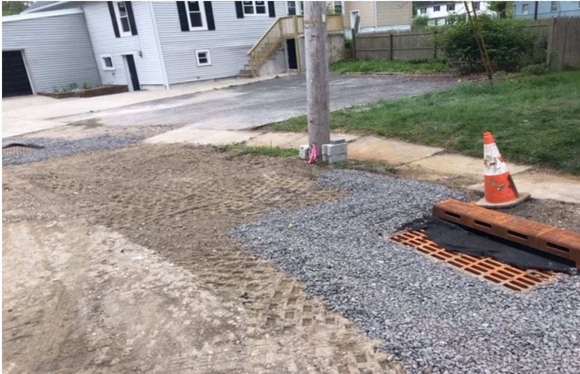
Figure: 3 – Utility structure rebuild near W.park Ave on lake Blvd (Looking East South side).
