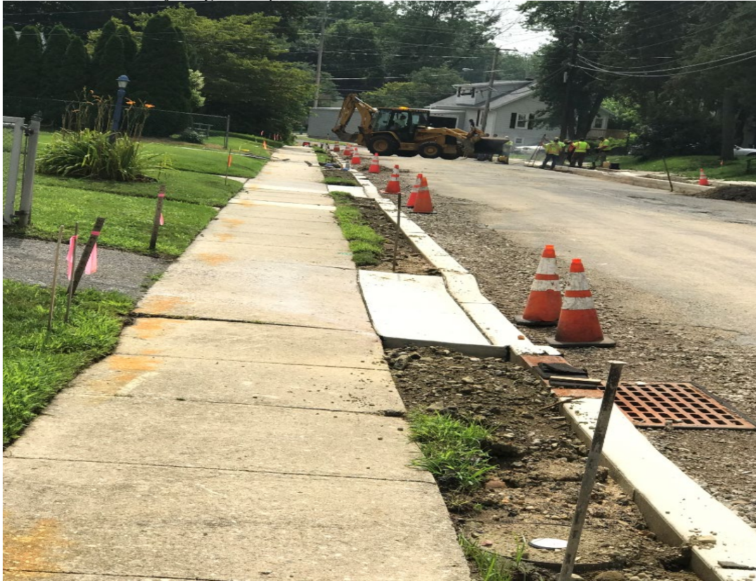
Figure: 2 – Reconstruct Curb and Handicap Ramp starting near W. park Ave (If and where directed)
