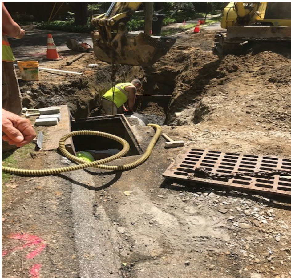
Figure: 1 – Reconstruct Pipe and inlet structure near Central Ave on lake Blvd.
