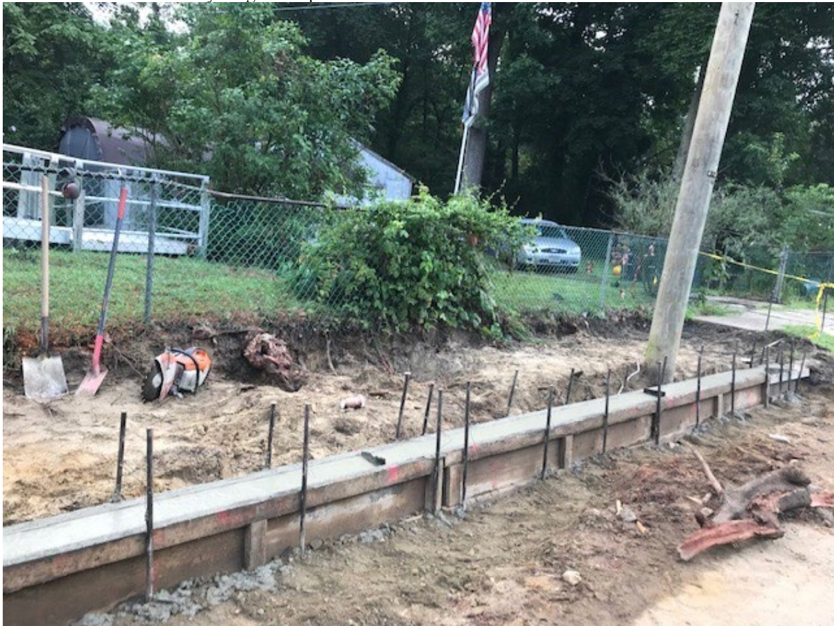
Figure: 2 – Reconstruct Curb and Handicap Ramp starting near Cottage Ave and Scott ave (If and where directed)
