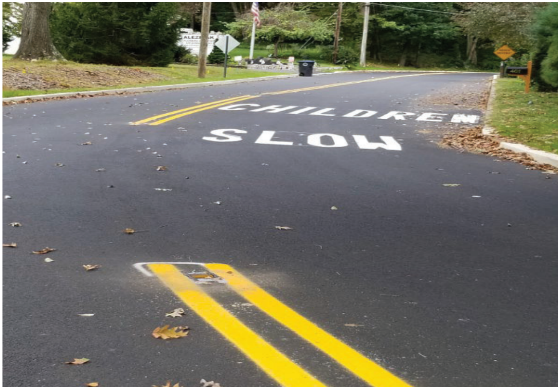
Figure: 2 –Repaint Centerlines and Traffic control and Signage installed for entire road (If and where directed)
