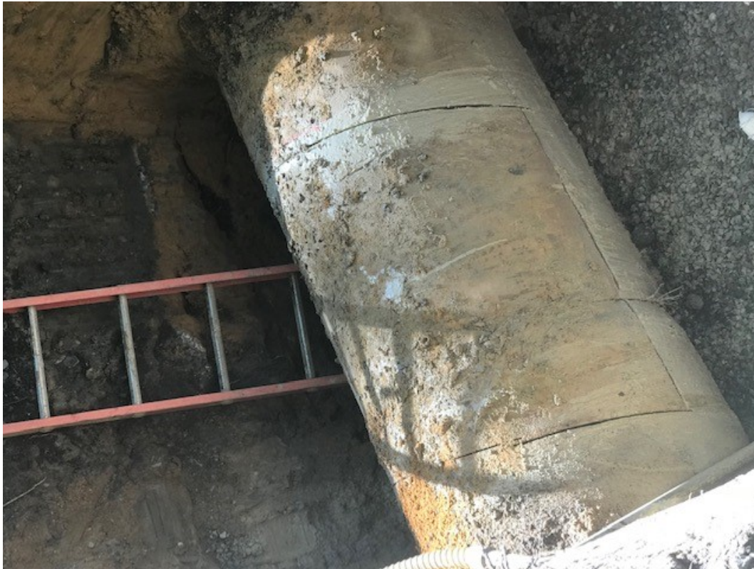
Figure: 2 – Utility pipe reconstruction on Central Ave on lake Blvd (Looking North side).
