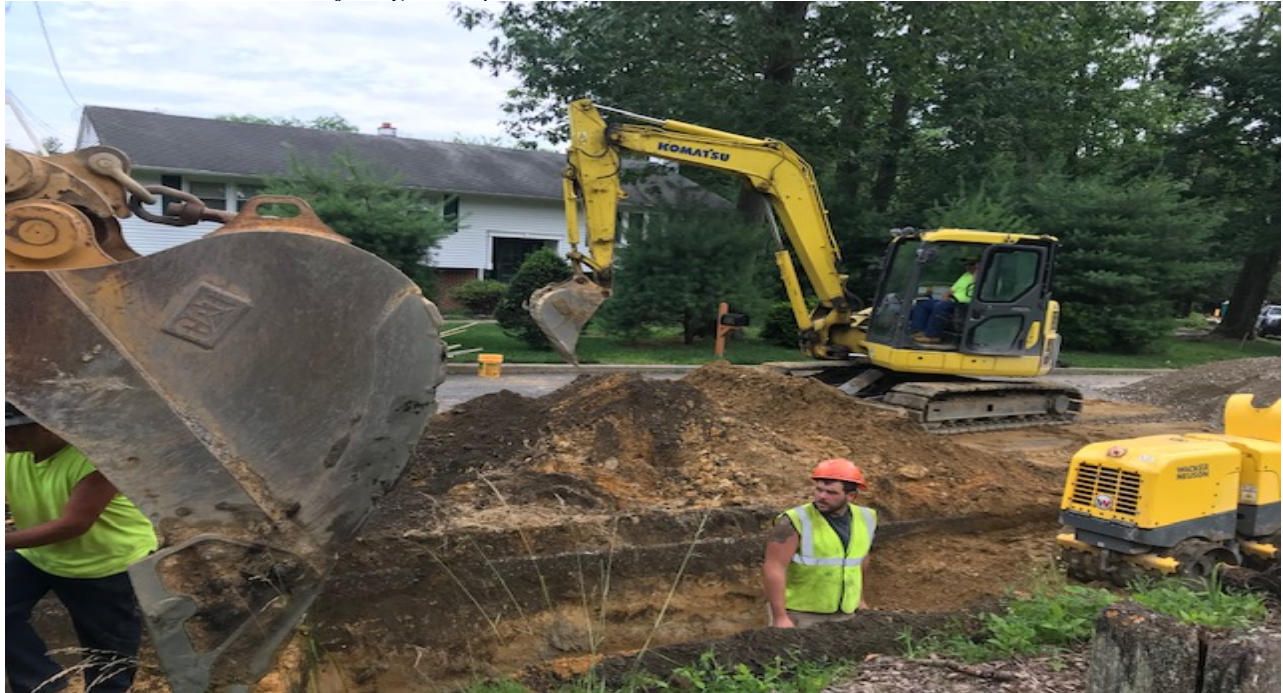
Figure: 2 – Reconstruct Pipe and inlet structure near Spring Landing Rd on lake Work Completed the Week of June 12, 2019
