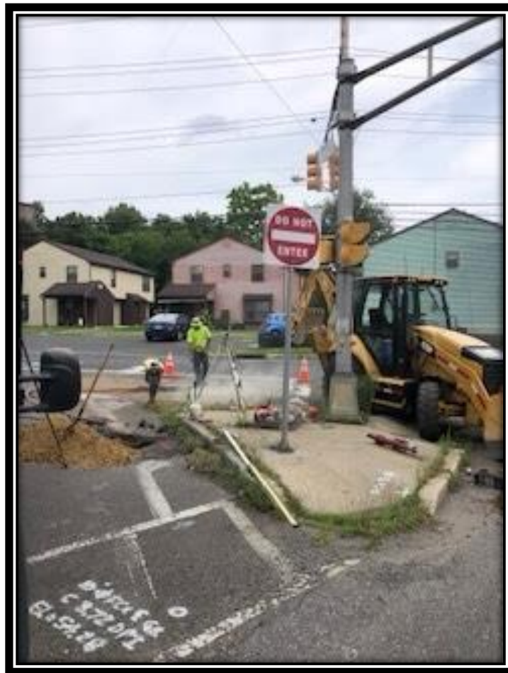
Figure: 1 – APS digging excavation test pits at the intersection of Almonesson Road and Lower Landing Road (CR 681) to locate gas, water, sanitation and force main lines.
