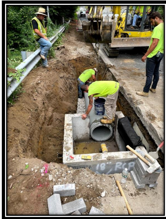
Figure: 2 – APS pipe crew installing B inlet and 18” RCP drainage pipe at STA 81+55 along the Southbound Lane of Lower Landing Road (CR 681).
