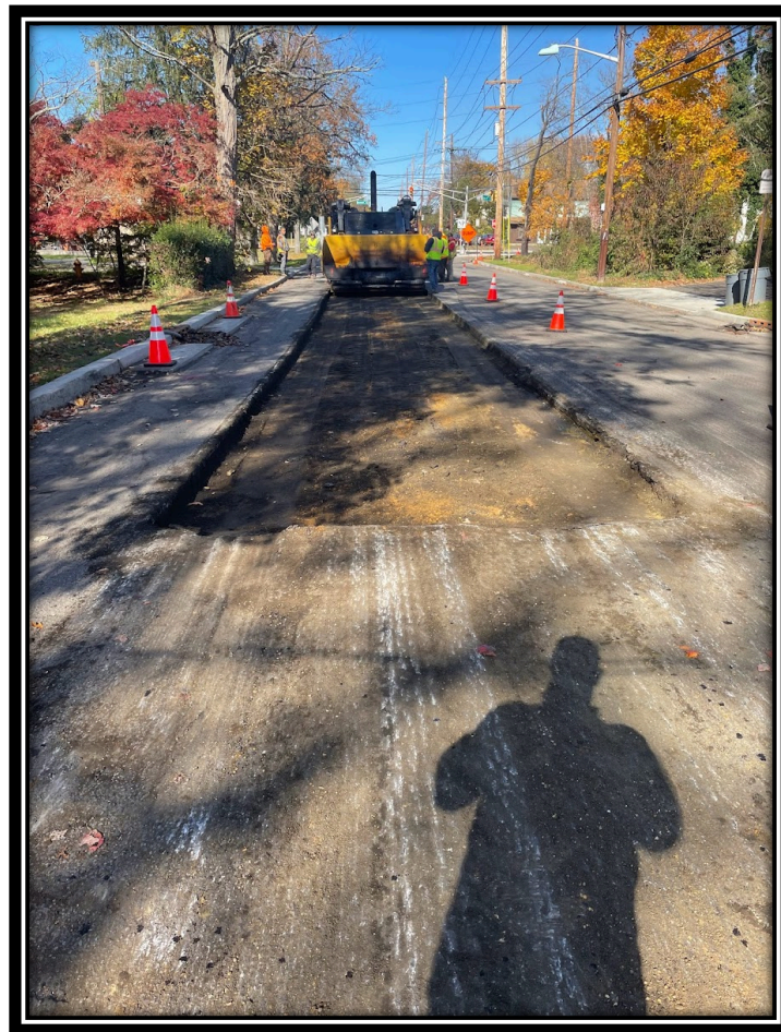
Figure: 1 – Example of APS performing a base repair along Lower Landing/Good Intent Road (CR 681) prior to installing HMA9.5M64 surface course.
