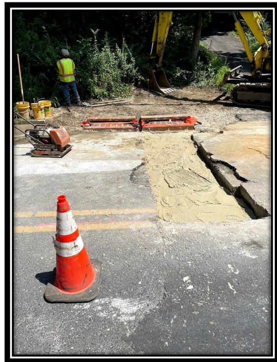
Figure: 3 – APS pipe crew filling in crossing at STA 82+00 with Flowable Fill before restoring asphalt and opening lane up to traffic along the Northbound lane of Lower Landing Road (CR 681).
