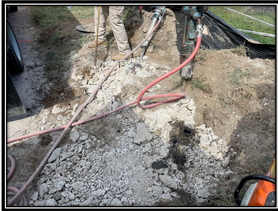
Figure: 2 – Techna-Pro jackhammering out the old traffic signal foundations at the Northeast corner of Lower Landing/Almonesson Road Intersection.
