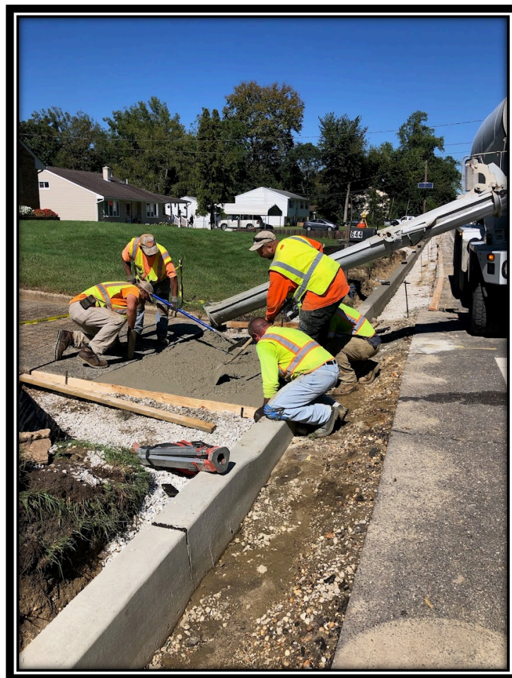
Figure: 1 – APS pouring concrete apron with welded wire along Lower Landing/Good Intent Road (CR 681).
