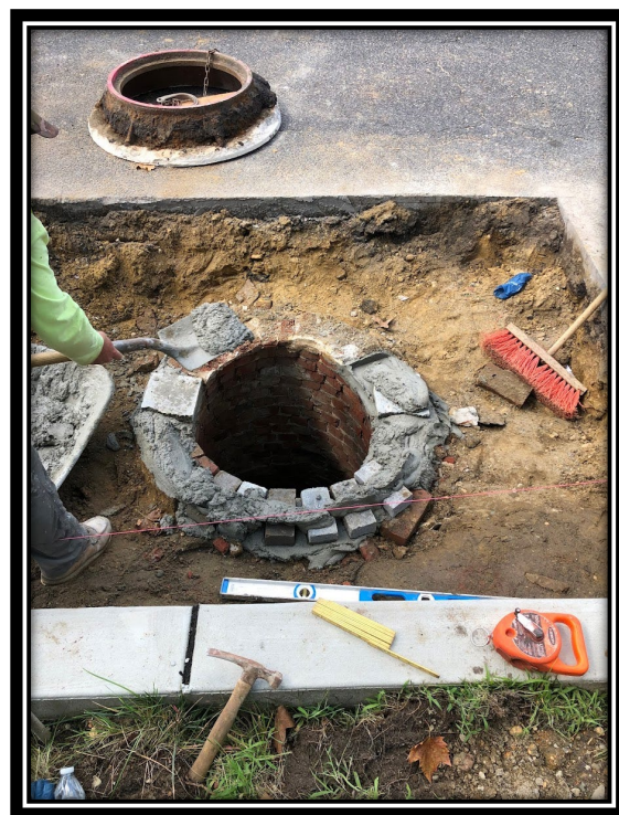
Figure: 3 – Manhole casting being reset along Lower Landing Road (CR 681) by the contractor APS.
