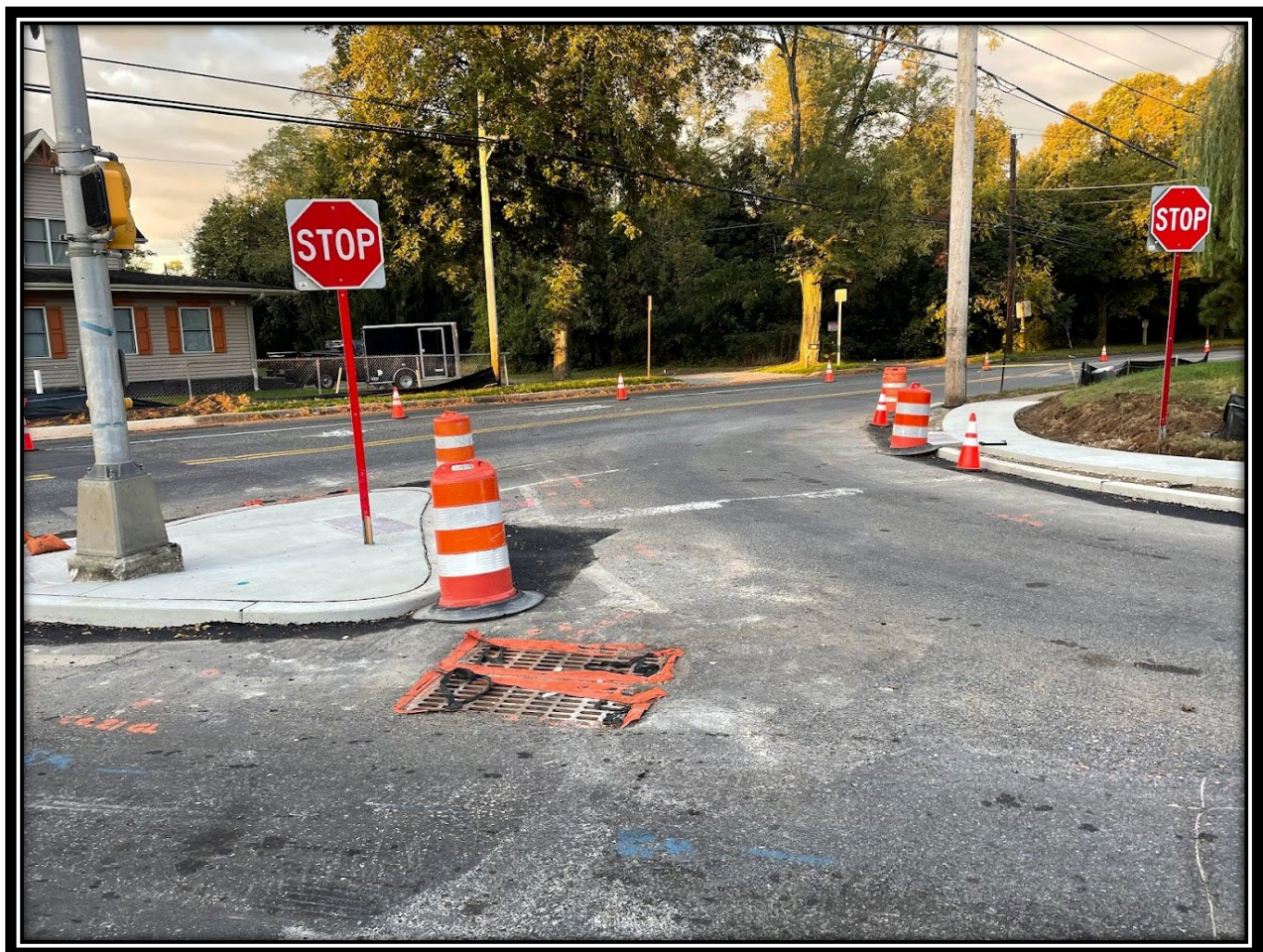
Figure: 1 – APS re-installed Stop/Do Not Enter signs at the NW island at the Almonesson/Lower Landing Intersection along with asphalt restoration (CR 681).
