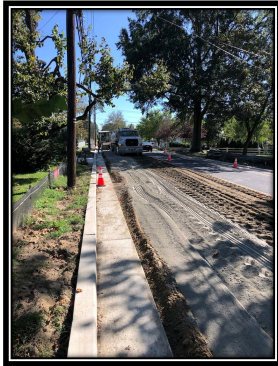
Figure: 2 – APS applying cement during the FDR process on Lower Landing Road (CR 681).
