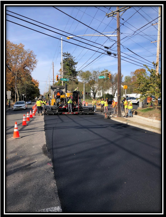
Figure: 3 –APS installing HMA9.5M64 surface course at the intersection of Almonesson Road and Lower Landing/Good Intent Road (CR 681).
