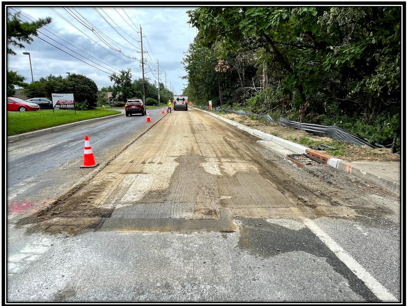
Figure: 1 – APS pulverizing existing asphalt and mixing with Portland Cement and water 14” deep for the base of the road.
