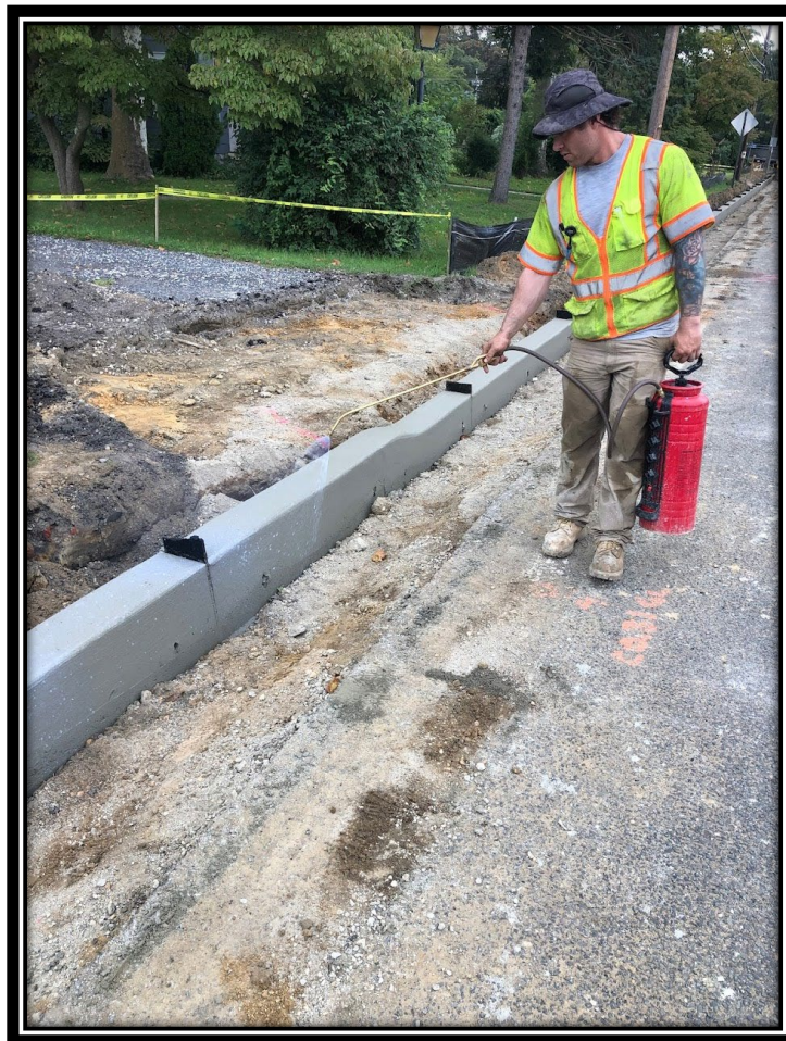
Figure: 1 – APS Laborer applying curing compound to mix poured that morning on Lower Landing Road (CR681).
