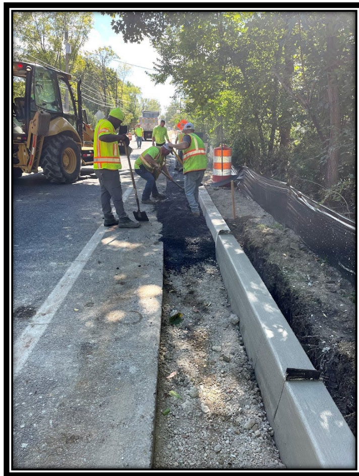
Figure: 1 – APS restoring asphalt around concrete curbs along Lower Landing/Good Intent Road before opening road up to traffic (CR 681).
