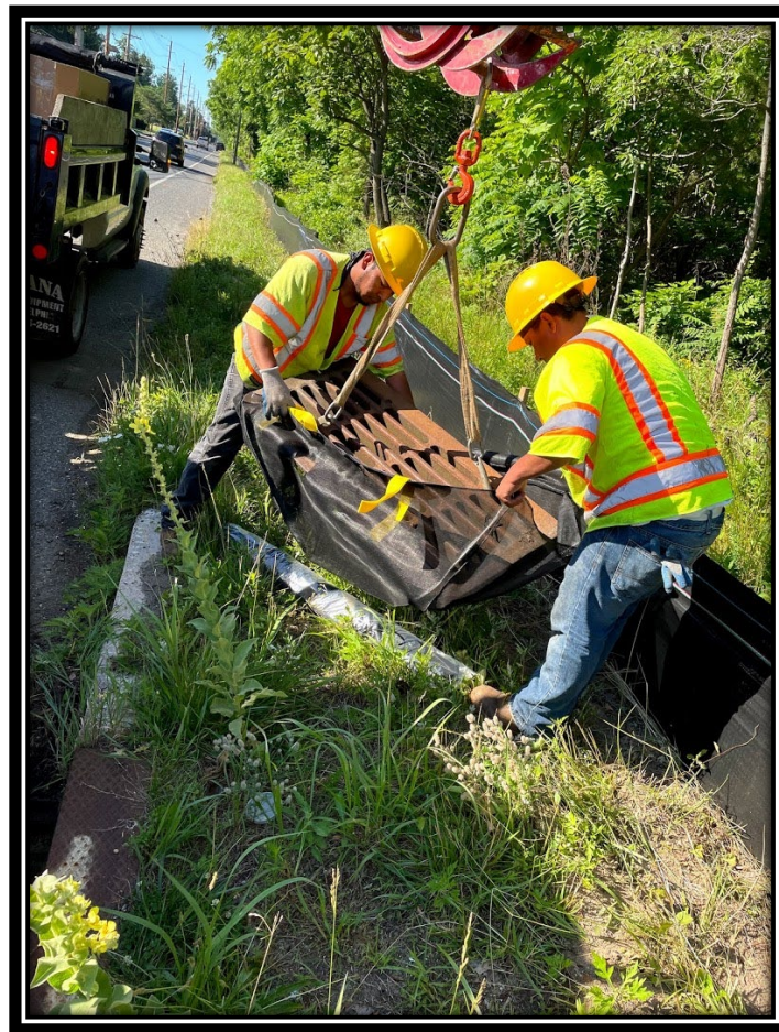
Figure: 1 – Installation of Inlet Filters along south bound lane of Lower Landing Road (CR 681) between Route 42 ramp and Poplar Ave (Station 16+50).
