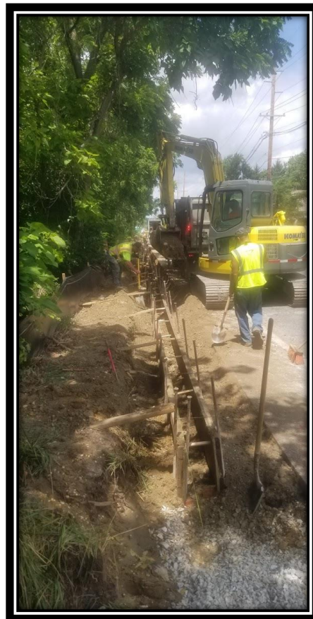
Figure: 1 – Concrete Vertical forms being installed on Southbound land of Lower Landing Road (CR 681) between Stations 28+00 to Station 25+00 (Apple Ave to Poplar Ave). Forms needed to be started 10 feet from proposed location of Double B inlet because the inlet is under construction. APS will tie the curb into the inlet upon completion.
