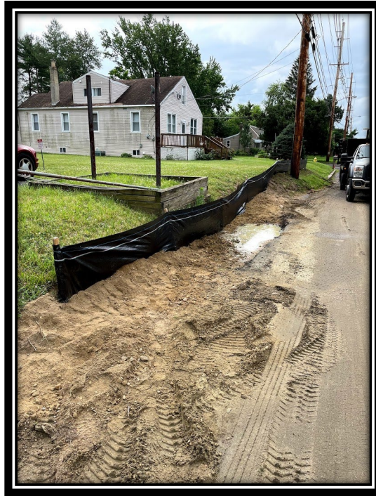
Figure: 2 – Installation of silt fence in front of residential properties between Highland Ave and Apple Ave along the north bound lane of Lower Landing Road (CR 681).
