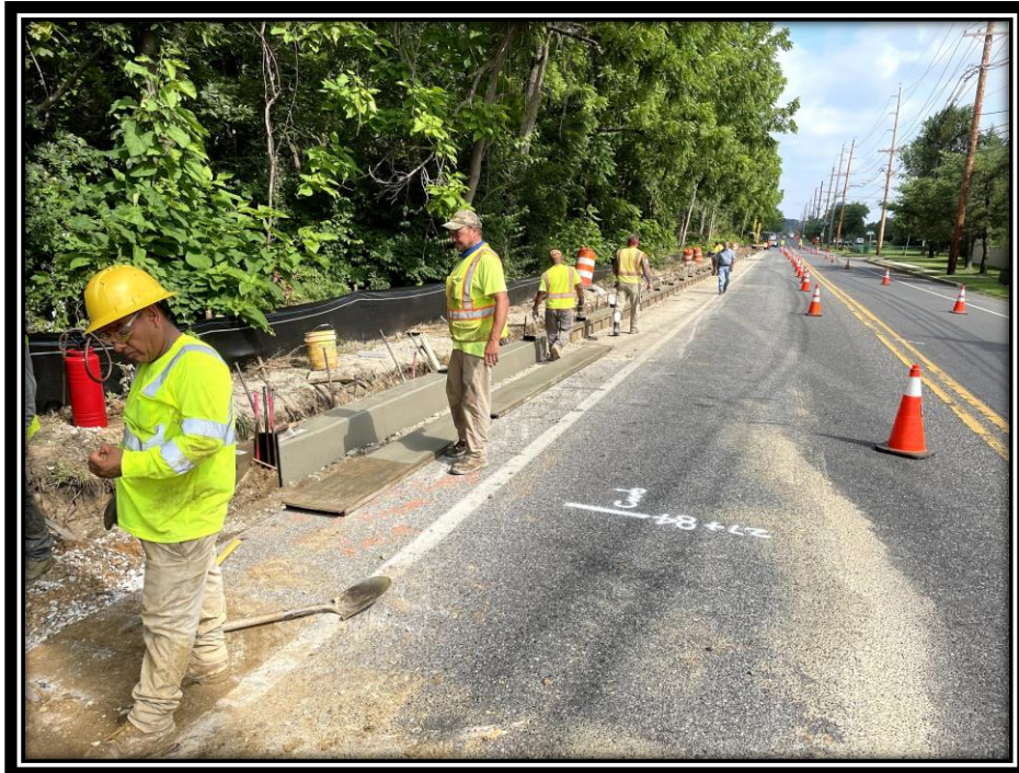
Figure: 2 – Striping of forms from poured 9” x 16” concrete vertical along the Southbound Lane of Lower Landing Road (CR 681).
