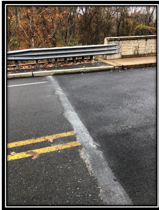
Figure: 2 – Sealed joint at the end of project limits by the bridge along Lower Landing/Good Intent Road (CR 681).
