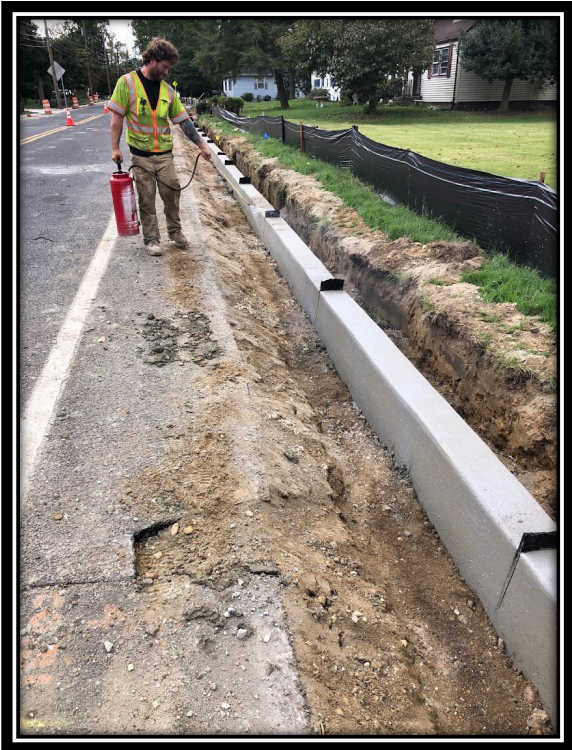
Figure: 2 – APS applying curing compound to concrete curb along Lower Landing Road (CR 681).
