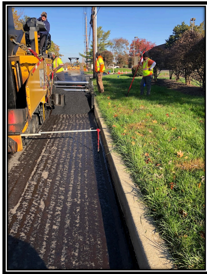
Figure: 1 – APS installing HMA9.5M64 surface course along Lower Landing/Good Intent Road (CR 681).
