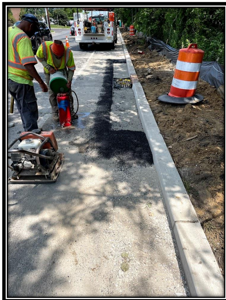
Figure: 1 – Gutters poured around inlets and asphalt filled in excavation areas so traffic can drive over the area along Southbound Lane of Lower Landing Road (CR 681).
