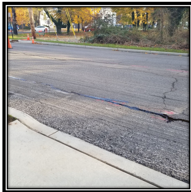
Figure: 3 –APS filling crack with polymerized joint adhesive in milled area along Lower Landing/Good Intent Road (CR 681).
