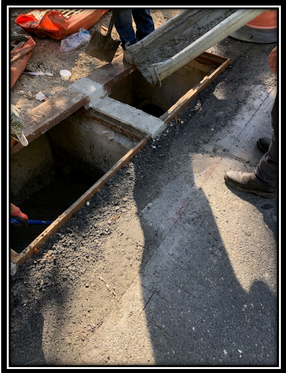
Figure: 3 – Pouring channels for inlets along Lower Landing Road/Good Intent Road (CR 681).
