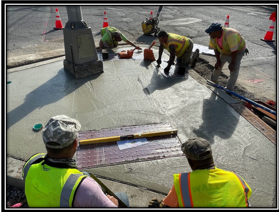
Figure: 2 – APS finishing concrete and adjusting for the appropriate slope at the NW island in the Almonesson/Lower Landing Road intersection.
