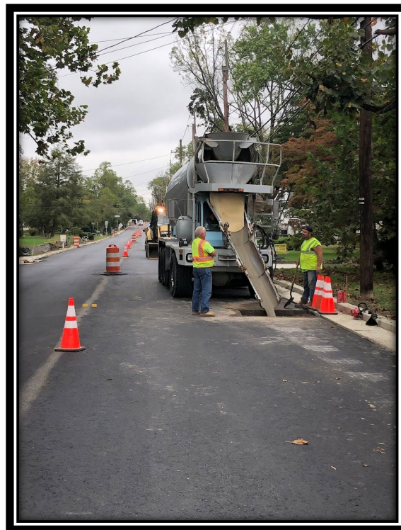
Figure: 3 – APS pouring flowable fill in the abandoned sewer drainage pipe along Good Intent Road.
