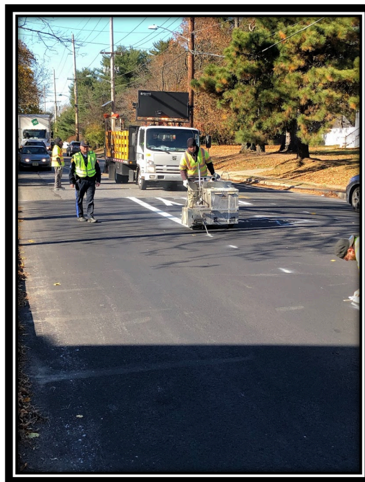
Figure: 3 – APS sub-contractor (Zone Striping Inc) striping at the Lower Landing and Almonesson Intersection.
