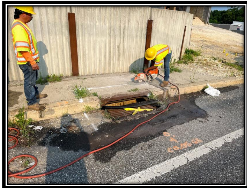
Figure: 3 – APS Subcontractors, Clean Earth Matters, cutting perimeter of inlets for excavation and construction of new inlets along Southbound Lane of Lower Landing Road (CR 681) across from 42 ramp at Station 11+00.
