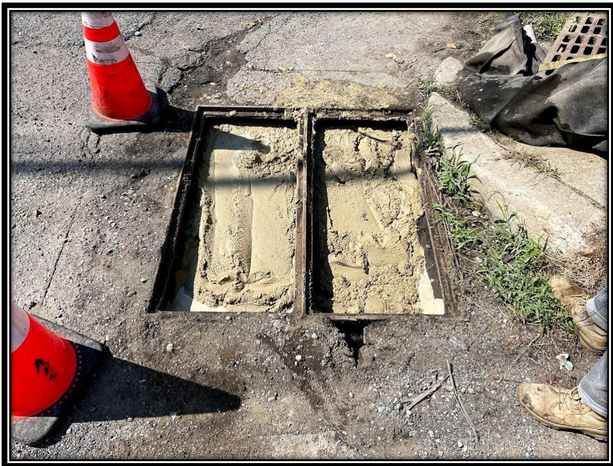
Figure: 1 – APS infilled existing E inlet and existing drainage pipe at Almonesson and Lower Landing Intersection with flowable fill.
