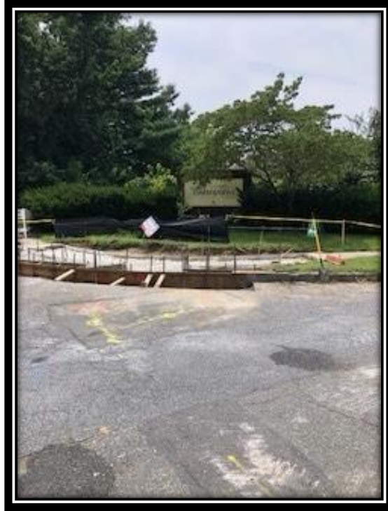
Figure: 2 – APS setting forms for curb and apron for ADA compliant ramps at the corner of Hemlock Drive along the Southbound Lane of Lower Landing Road (CR 681).
