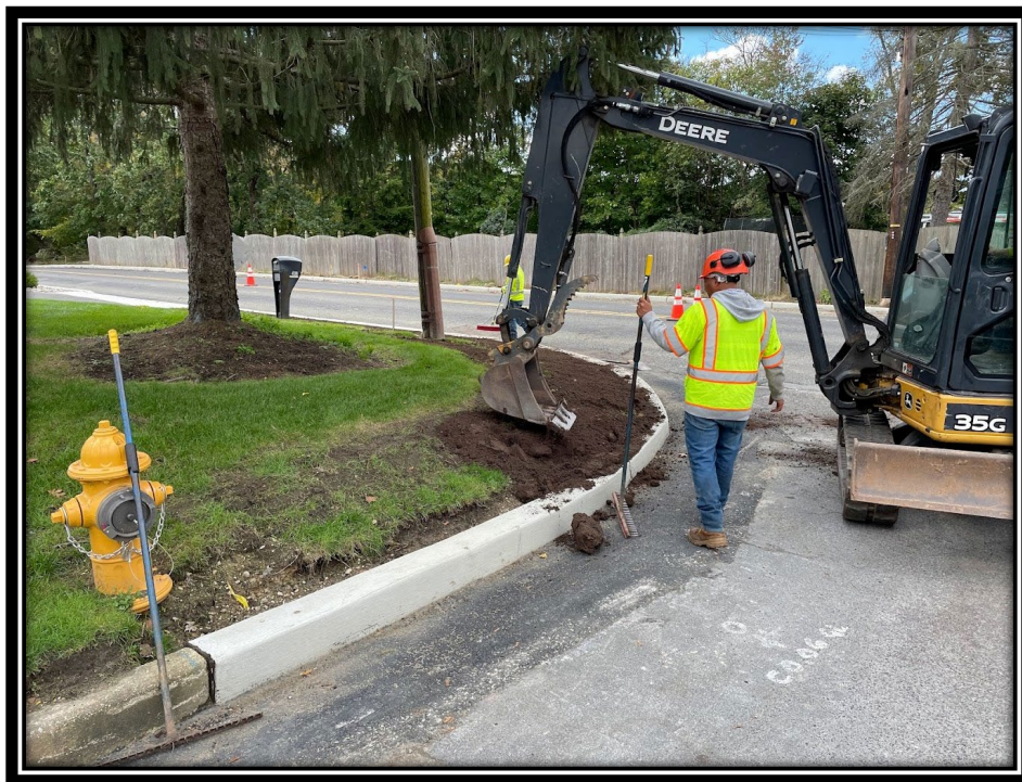
Figure: 3 – Clean Earth Matters applying topsoil 4” Thick along Lower Landing/Good Intent Road (CR681).
