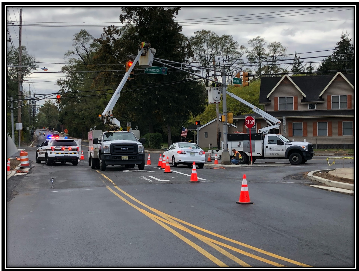
Figure: 1 – Techna-Pro at the intersection of Almonesson and Lower Landing/Good Intent Road installing image detectors and push buttons for crosswalks.
