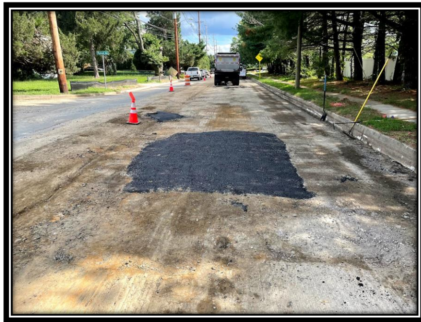
Figure: 3 – Example of APS FDR crew repairing a spot where the soil was soft after pulverization. Area is filled with DGA and compacted and then covered with asphalt prior to base course of paving.
