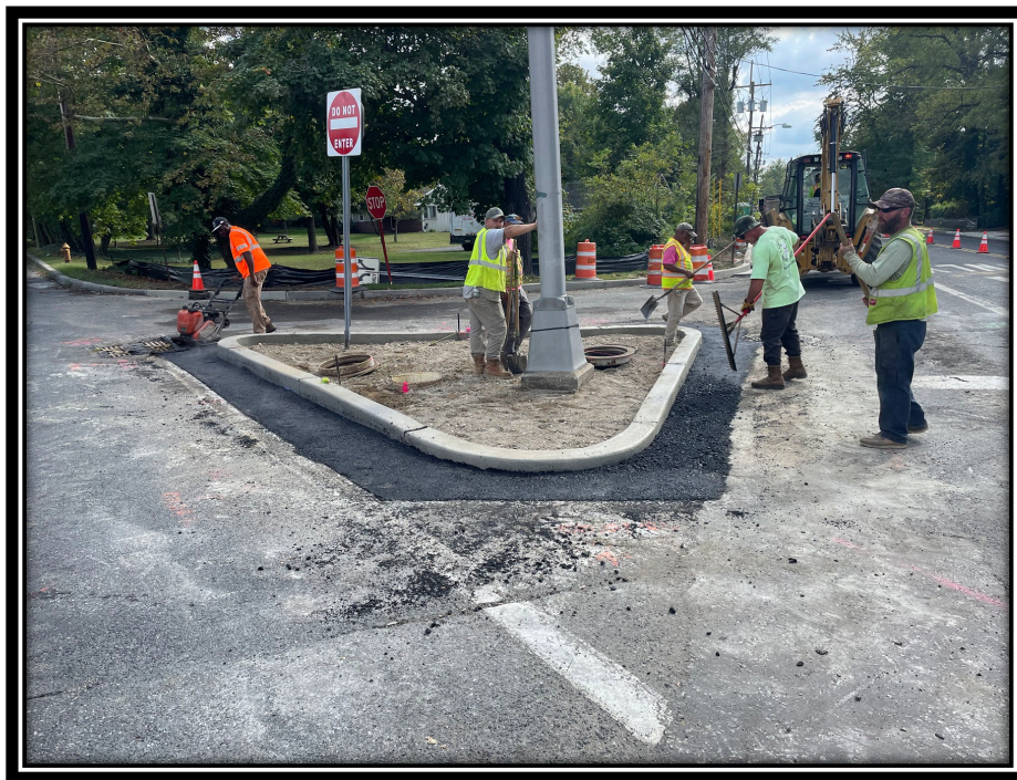
Figure: 3 – APS backfilling curb and restoring asphalt at the Southeast Island in the Lower Landing/Almonesson Road intersection before opening road up to traffic.
