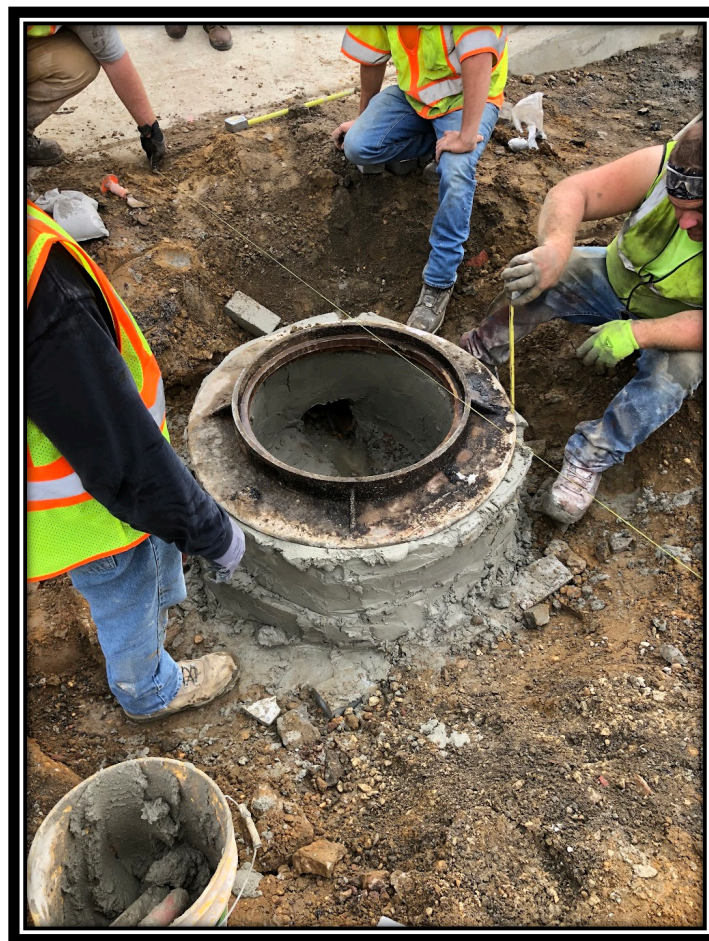
Figure: 1 – APS resetting existing manhole casting along Lower Landing/Good Intent Road before installing base course of asphalt (CR 681).
