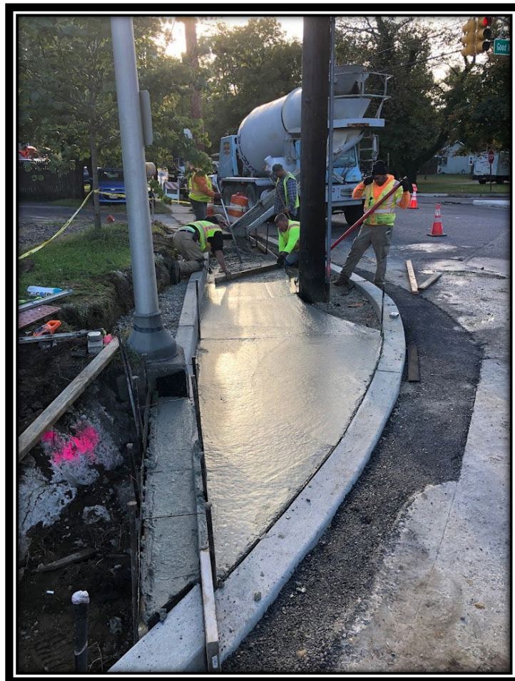
Figure: 1 – APS pouring sidewalk at the NE corner of the Almonesson/Lower Landing Intersection (CR 681), implemented header curb also visible in this photo.
