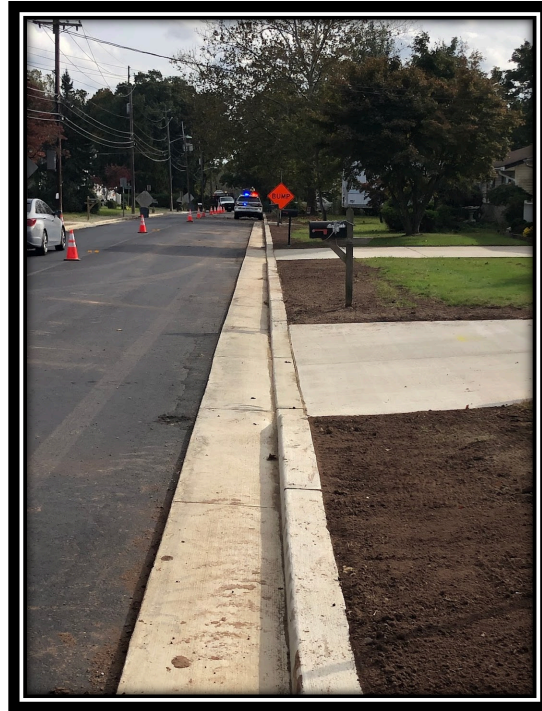
Figure: 2 – Clean Earth Matters laying topsoil 4” thick along Lower Landing/Good Intent Road (CR 681).
