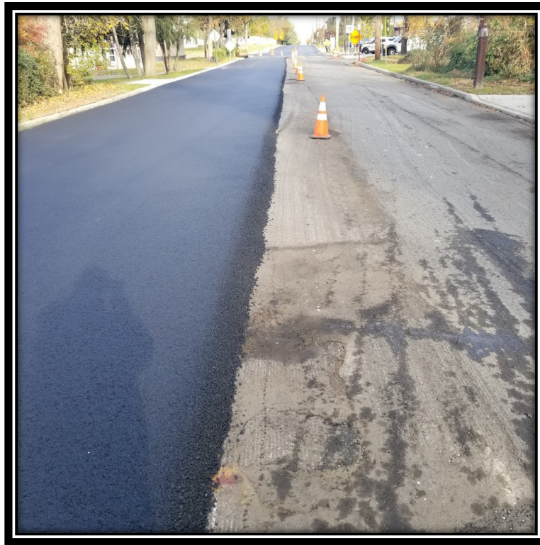
Figure: 2 –APS installing HMA9.5M64 surface course along Lower Landing/Good Intent Road (CR 681) between the bridge and the Almonesson Intersection.
