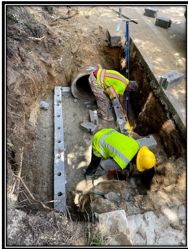
Figure: 1 – Type Double B inlet, Complete Construction at Station 28+00 across from Apple Ave on West Side of (Southbound Lane) of Lower Landing Road (CR 681). APS subcontractor, Clean Earth Matters, poured foundation of inlet and built block on top, expecting to pour the channel at a later date.
