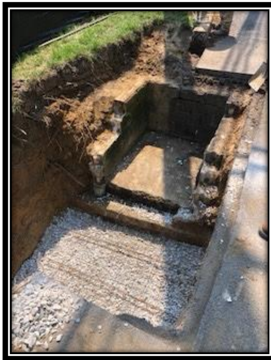
Figure: 3 – Clean Earth Matters building a new Type B inlet next to an existing B inlet to make it a “Double B” inlet along Lower Landing Road (CR 681).
