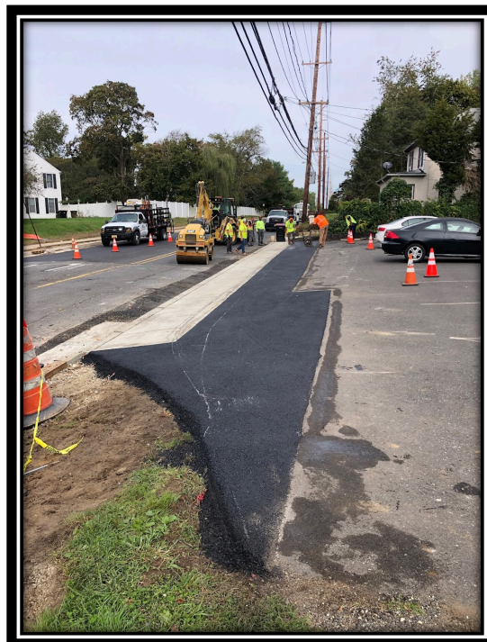
Figure: 3 –APS milled and restored asphalt on a driveway at STA 51+00 LT right before the Almonesson and Lower Landing/Good Intent Road intersection.
