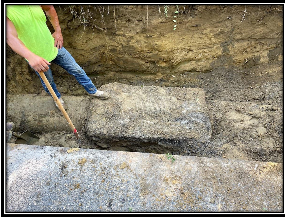
Figure: 2 – APS excavated around existing pipe at STA 52+14 – 52+24 Left side of Lower Landing road to make repair according to plans. Repair already made in the past and pipe was found to be in good condition so infilled around existing repair with flowable fill.
