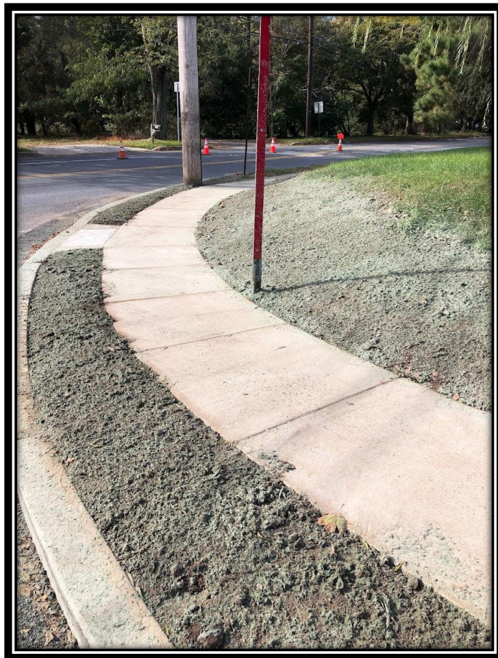
Figure: 1 – APS sub-contractor, Clean Earth Matters, hydroseed application at the NW corner of Almonesson and Lower Landing/Good Intent Road (CR 681).
