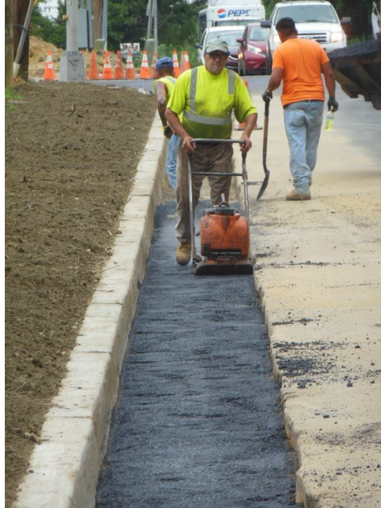
Figure 4 Bituminous material was placed in the front side of the newly installed curb
