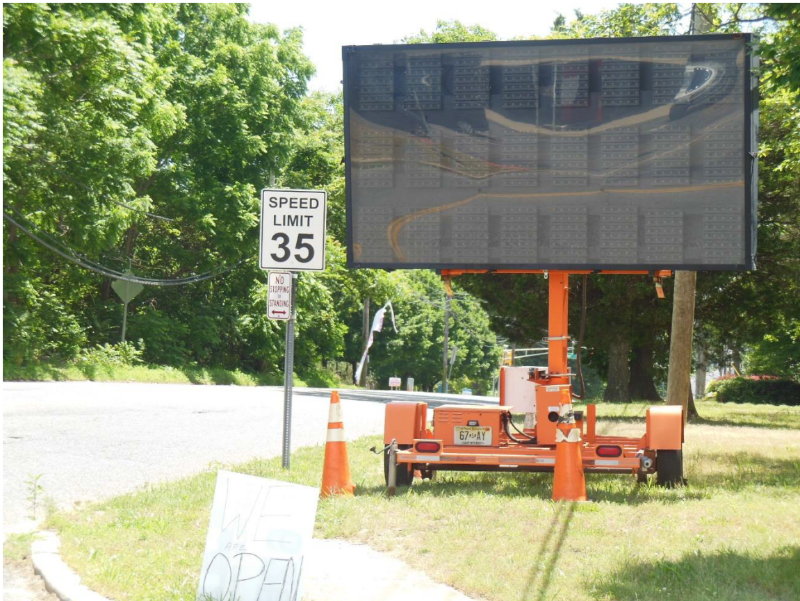
VMS installed at each end of the project.
