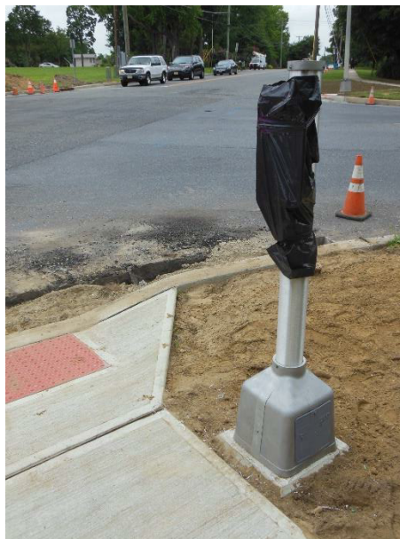
Figure 5 Contractor graded and dressed up the area where new Push button poles were installed
