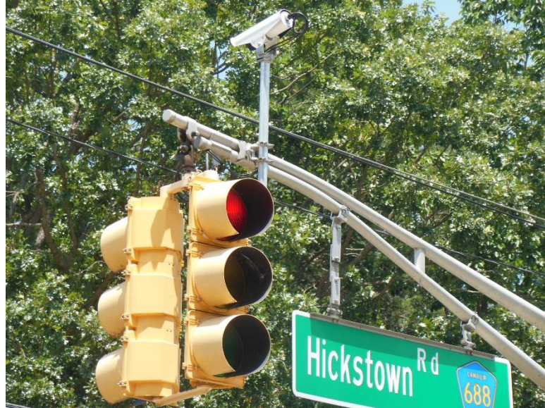
Figure 2 Image Detector installed at the intersection of Hickstown and Peter Cheeseman
