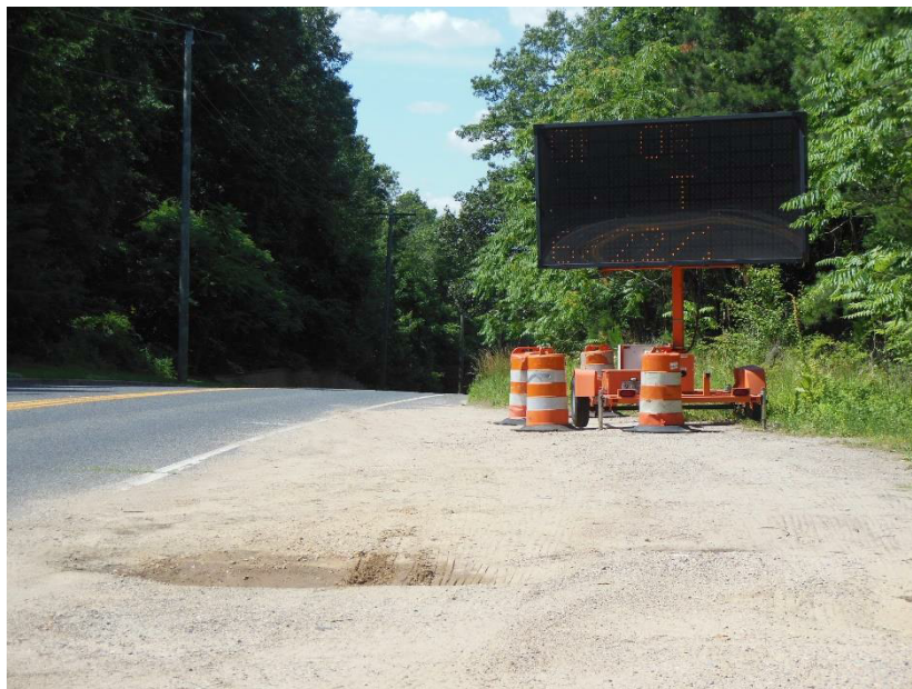
Figure 3 VMS was moved to a safer location around Sta. 67+00 Lt.
