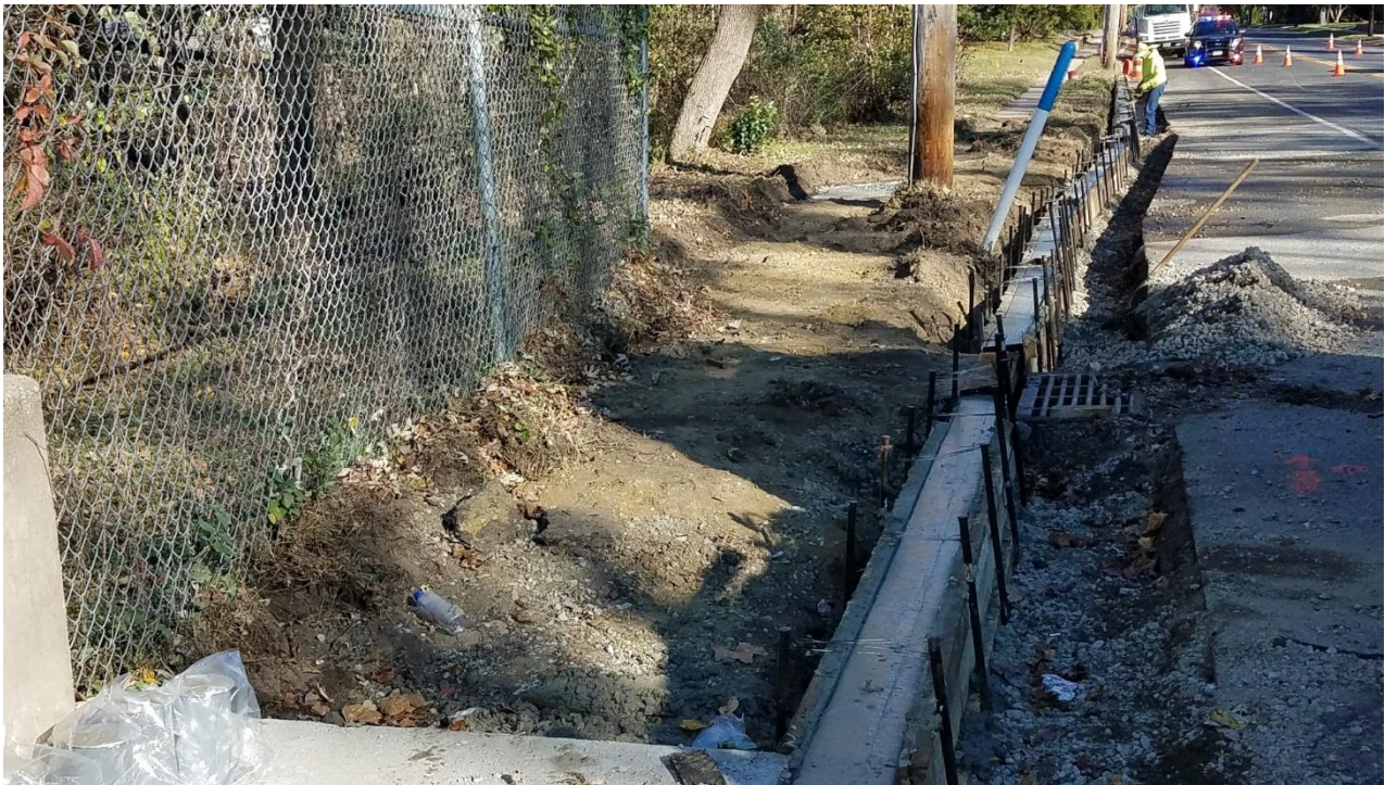
Figure 3. Lexa removing sidewalk at Location #5 westbound. Note the utility pole will need to be relocated.
