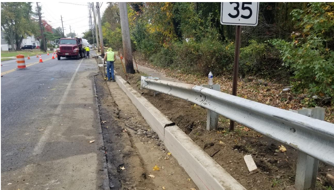
Figure 2. New curb at Location #3 westbound. Guiderail to be removed in this location.
