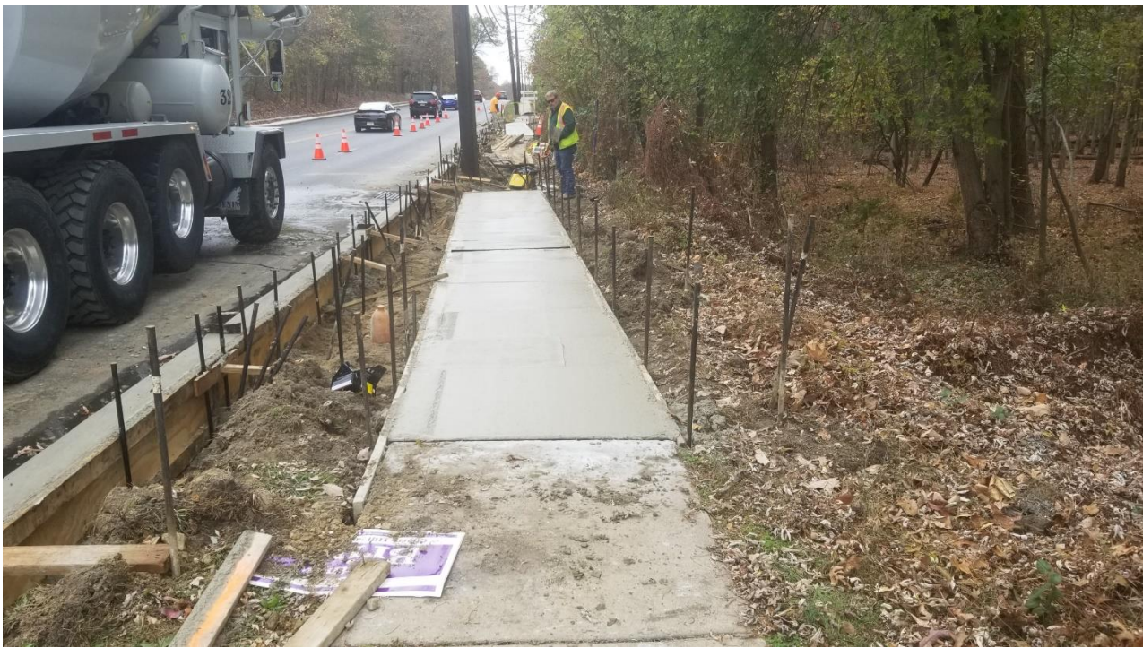
Figure 3. New sidewalk at Location 6 westbound. Note the utility pole will need to be relocated.
