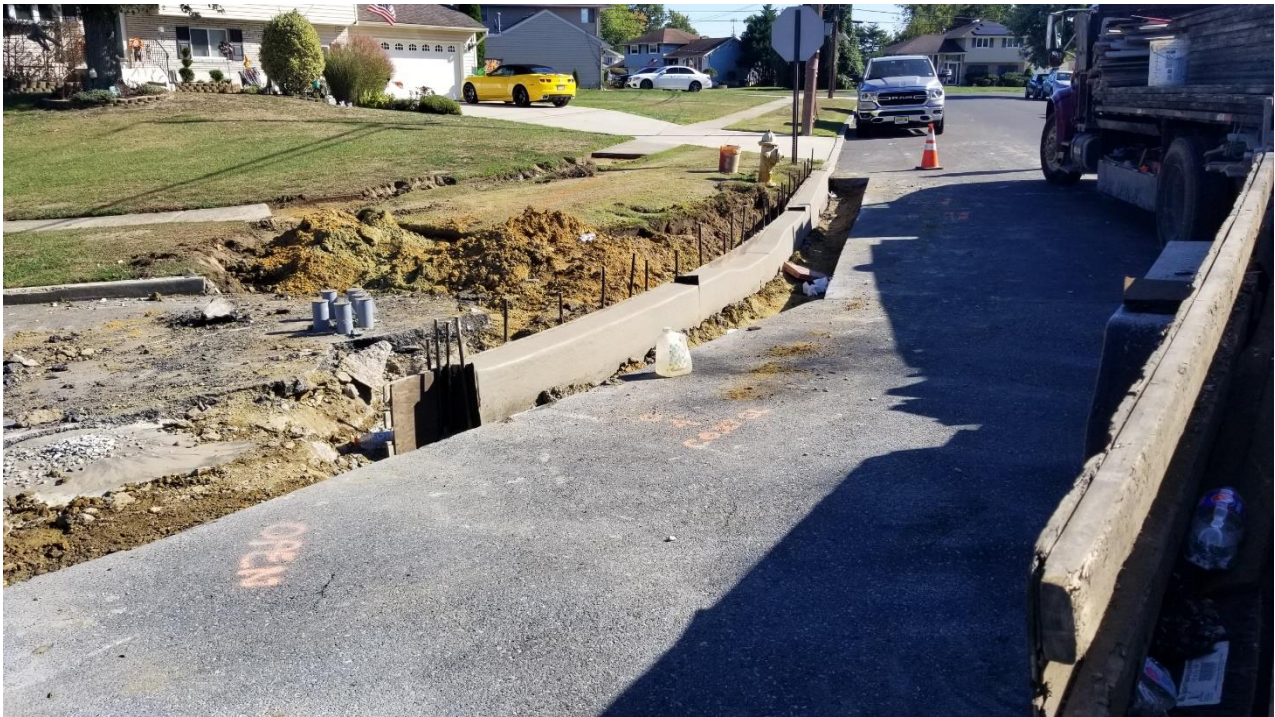
Figure 4. Lexa placed concrete curb at the intersection of Albert Road and Evesham Road.
