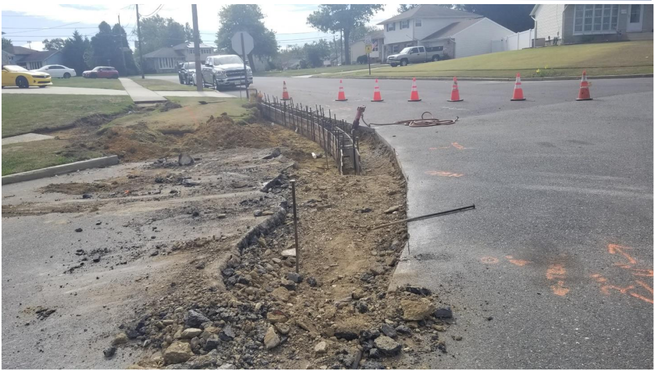
Figure 3. Lexa removed asphalt to extend the sidewalk and curb at the intersection of Albert Road and Evesham Road.
