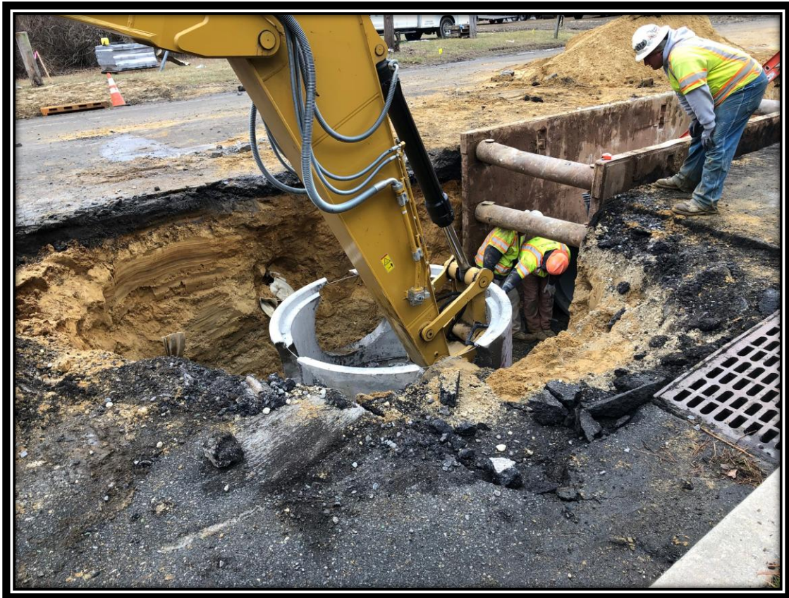
Figure: 1 – Installation of 6' diameter storm sewer manhole along the northbound lane of Watsonstown-New Freedom Road (CR 691) in the Borough of Berlin
