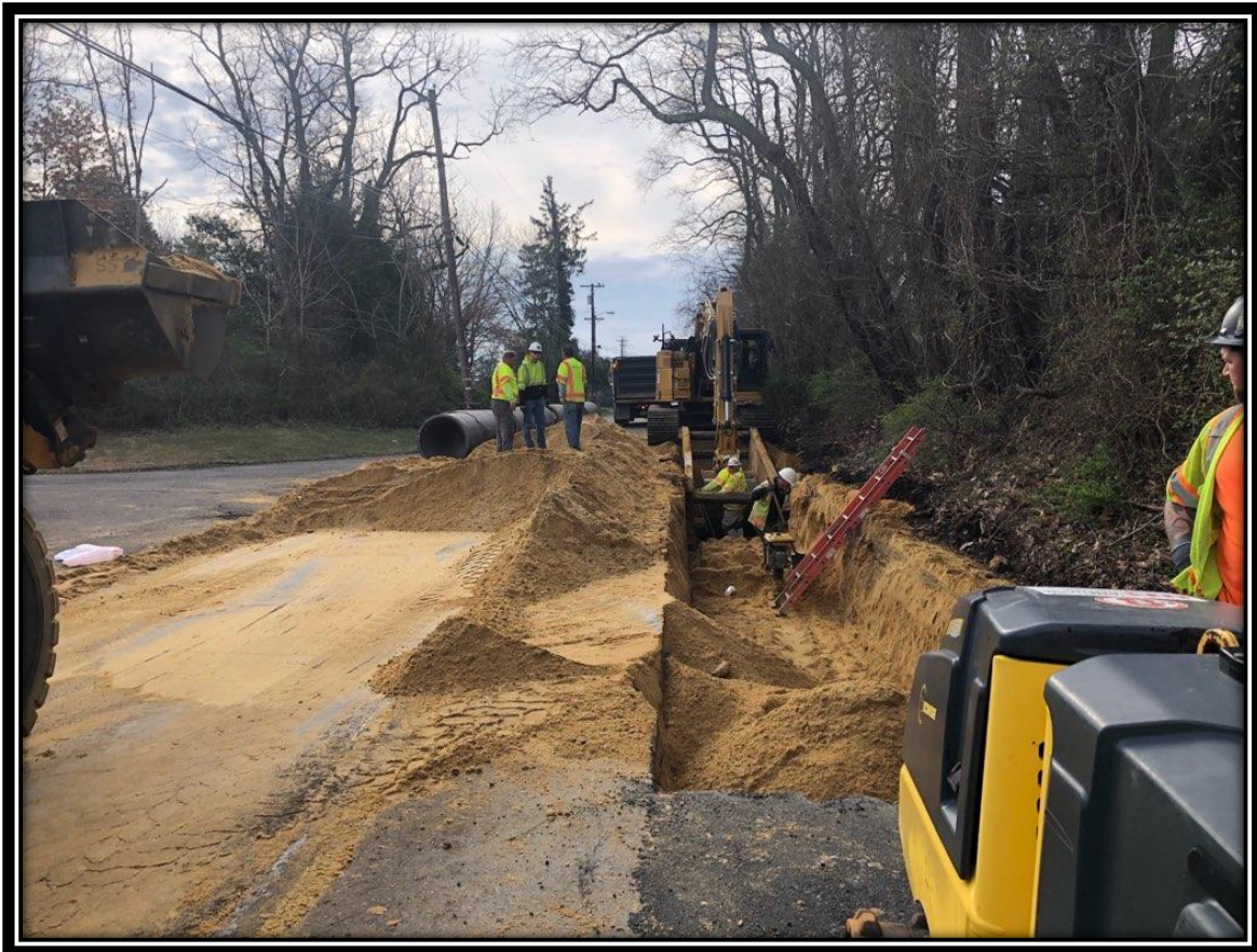
Figure: 1 – Installation of 36” RCP along the southbound lane of Watsonstown-New Freedom Road (CR 691) in the Borough of Pine Hill
