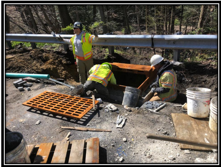
Figure: 3 – Installation of type 'B' inlet in the southbound lane of Watsontown-New Freedom Road (CR 691) in the Borough of Pine Hill
