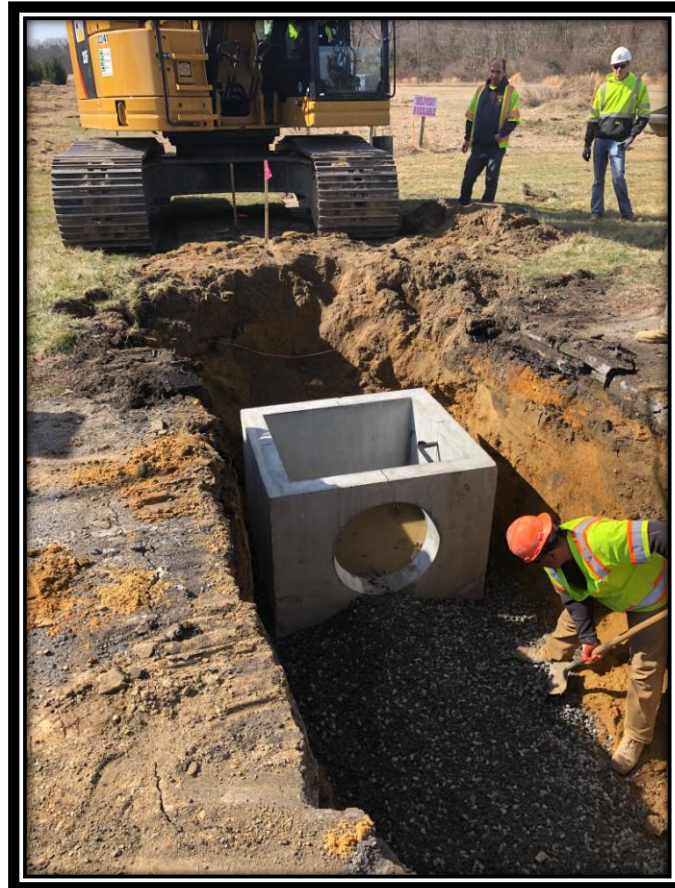
Figure: 1 – Installation of type B inlet along the southbound lane of Watsonstown-New Freedom Road (CR 691) in the Borough of Pine Hill
