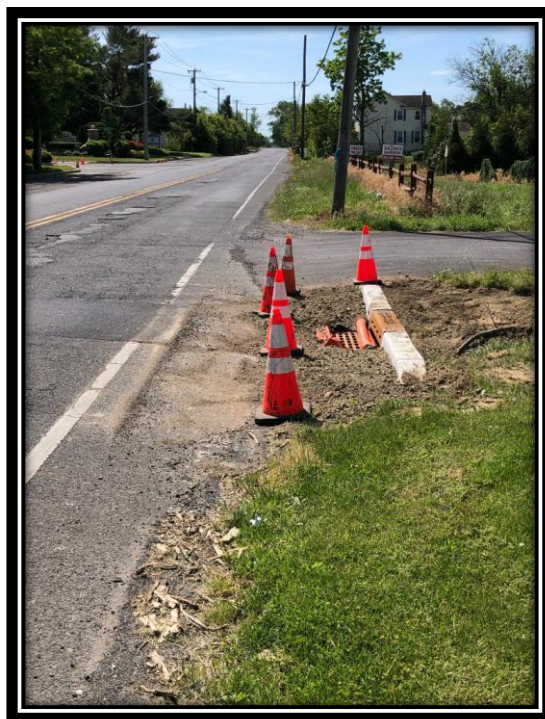
Figure: 3 – Installation of concrete curb along the southbound lane between Carriage Stop Drive and Westbury Drive in the Borough of Pine Hill
