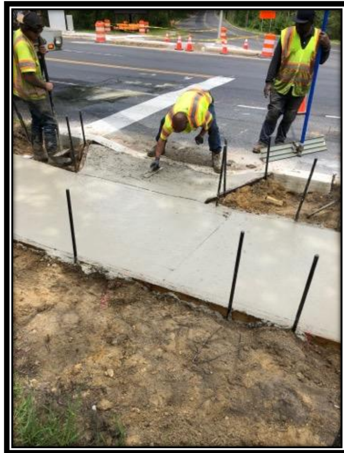
Figure: 1 – Installation of ADA ramp at the southwest corner of the intersection Watsonstown-New Freedom Road (CR 691) and Berlin-Clementon Road in the Borough of Clementon
