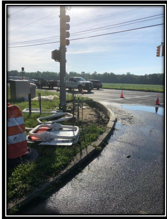
Figure: 2 – Installation of concrete curb for the proposed ADA ramp at the northeast corner of the intersection with Berlin-Cross Keys Road in the Borough of Berlin
