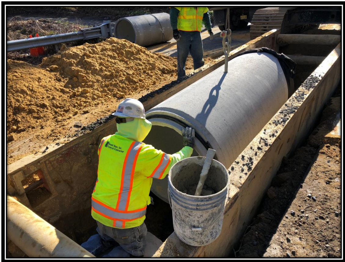
Figure: 1 – Installation of 36” RCP along the southbound lane of Watsonstown-New Freedom Road (CR 691) in the Borough of Pine Hill
