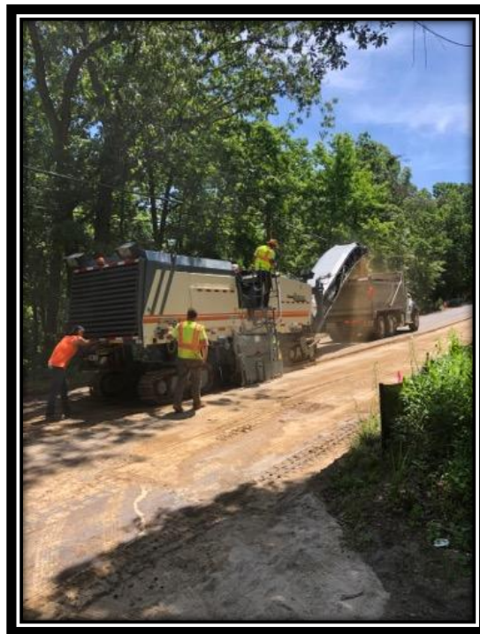
Figure: 3 – Final grading of the newly reclaimed roadway subbase using the milling machine between the White Horse Pike and Berlin-Clementon Road in the Borough of Clementon
