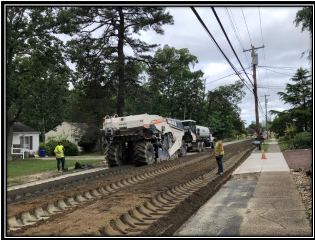
Figure: 1 – Full depth reclamation with cement between the White Horse Pike and Berlin Clementon Road in the Borough of Clementon
