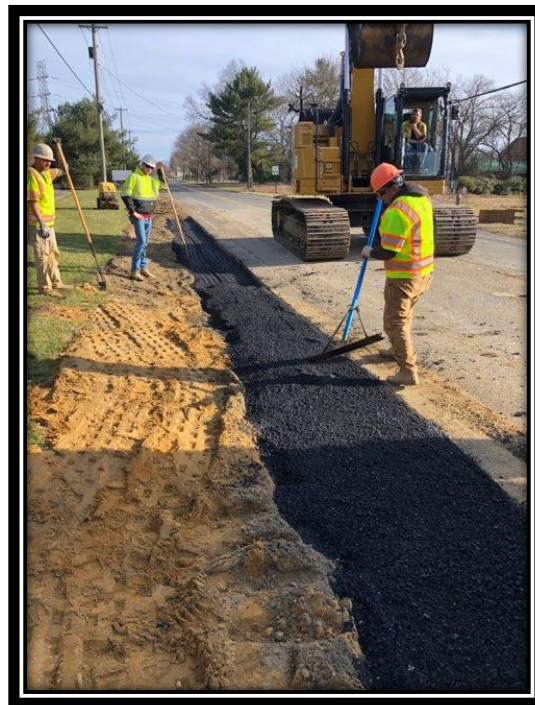
Figure: 3 – HMA restoration of the 24” RCP trench along the northbound lane of Watsontown-New Freedom Road (CR 691) in the Borough of Berlin
