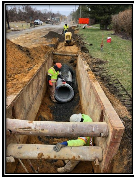
Figure: 2 – Installation of 24” RCP along the northbound lane of Watsontown-New Freedom Road (CR 691) in the Borough of Berlin
