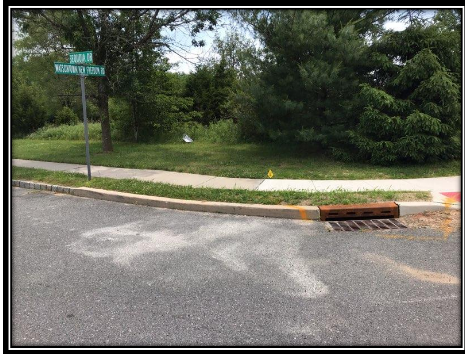
Figure: 2 – Installation of type ‘N’ eco inlet curb piece along the northbound lane at the intersection with Sequoia Drive in the Borough of Berlin
