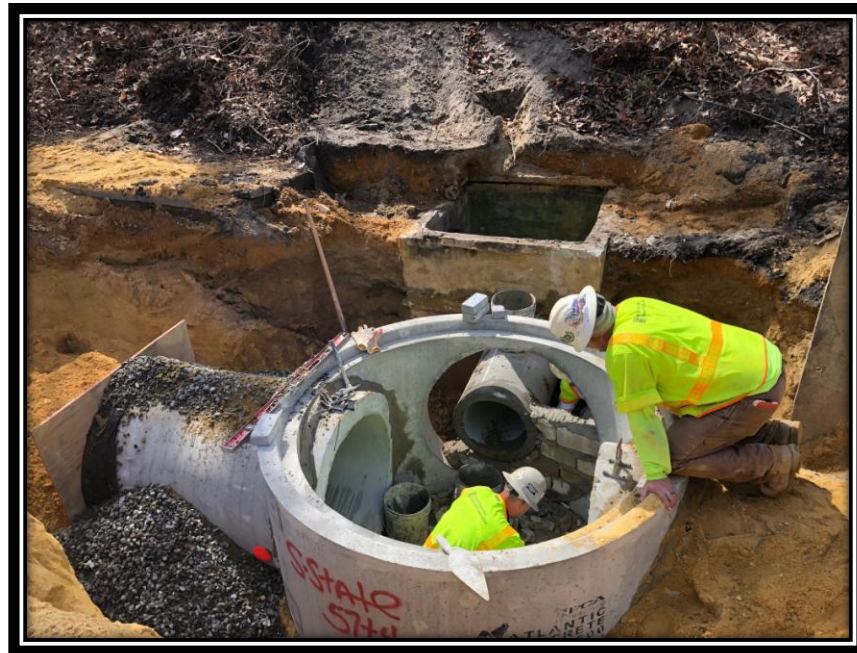
Figure: 2 – Installation of 6' diameter storm sewer manhole on Watsontown-New Freedom Road (CR 691) between Berlin-Clementon Road and Carriage Stop Drive in the Borough of Pine Hill
