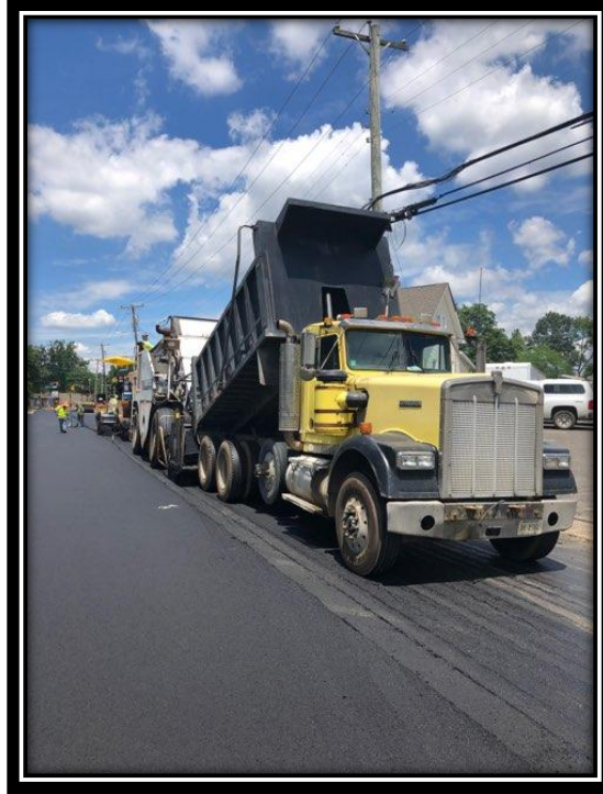
Figure: 2 – Installation of HMA 9.5M64 surface course in the southbound lane between the White Horse Pike and Berlin-Clementon Road in the Borough of Clementon
