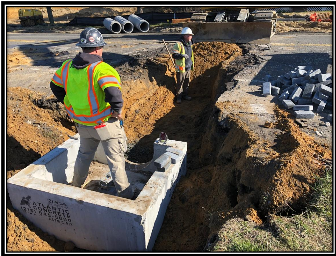
Figure: 1 – Installation of type B inlet along the southbound lane of Watsonstown-New Freedom Road (CR 691) in the Borough of Pine Hill
