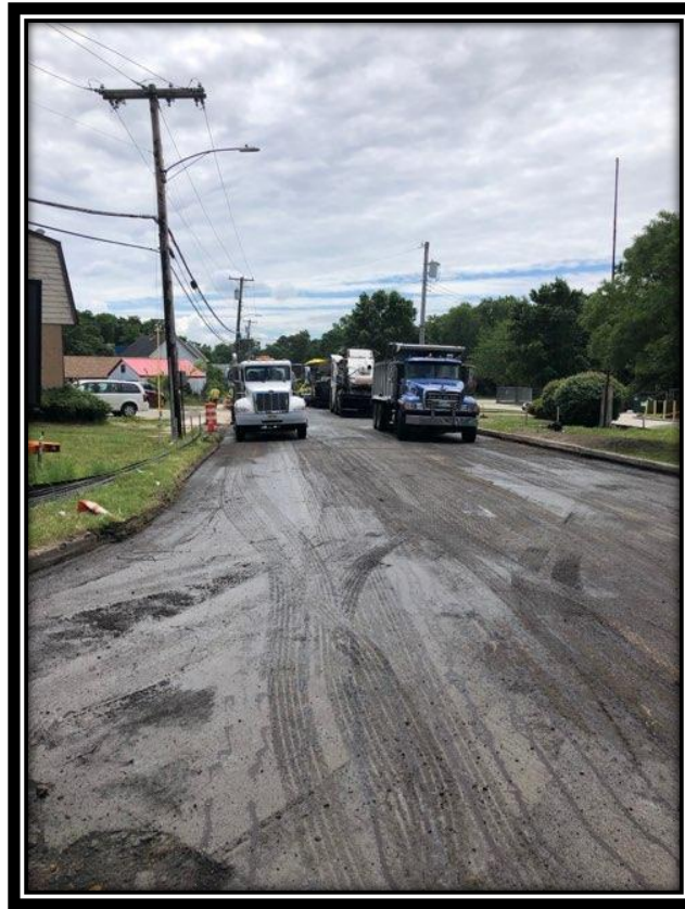
Figure: 1 – Installation of HMA 19M64 base course in the northbound lane between Smith Terrace and the White Horse Pike in the Borough of Clementon
