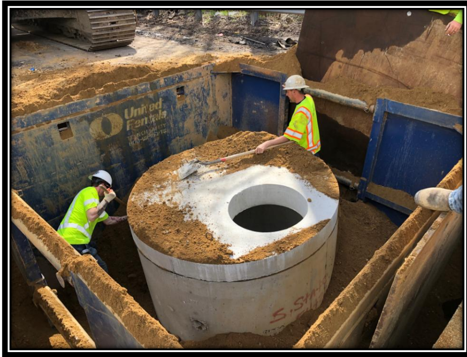
Figure: 2 – Installation of 6' diameter storm sewer manhole on Watsontown-New Freedom Road (CR 691) between Berlin-Clementon Road and Carriage Stop Drive in the Borough of Pine Hill
