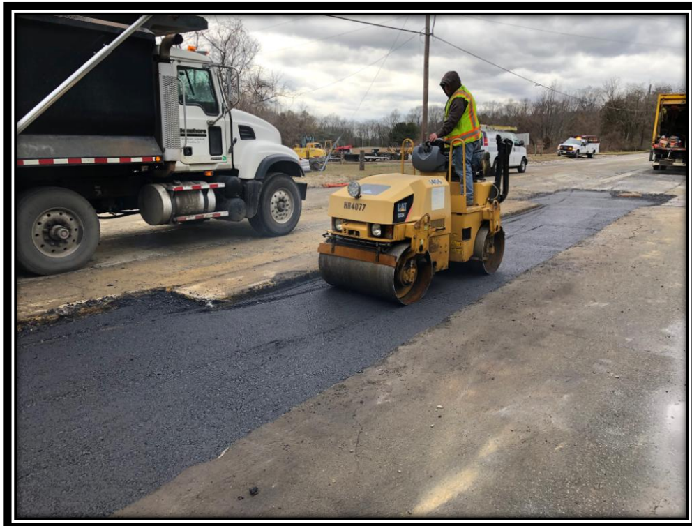
Figure: 3 – HMA restoration of the 36” RCP trench along the northbound lane of Watsontown-New Freedom Road (CR 691) in the Borough of Berlin
