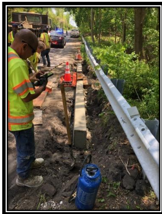
Figure: 3 – Installation of concrete curb adjacent to the newly reconstructed type 'B' inlet in the southbound lane between Berlin-Clementon Road and Berlin-Cross Keys Road
