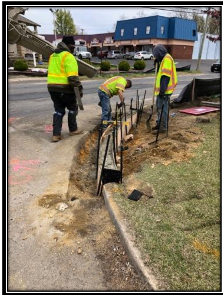
Figure: 1 – Installation of concrete curb along the southbound lane of Watsonstown-New Freedom Road (CR 691) at the intersection with Smith Terrace in the Borough of Clementon
