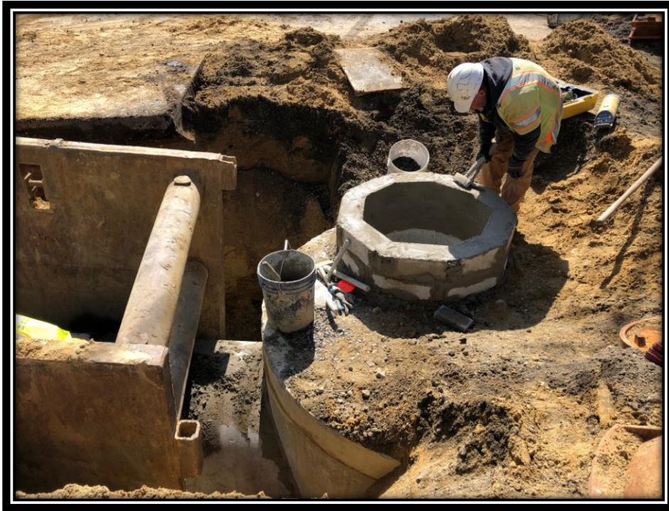
Figure: 2 – Installation of a 6' diameter storm manhole in the southbound lane of Watsontown-New Freedom Road (CR 691) in the Borough of Pine Hill
