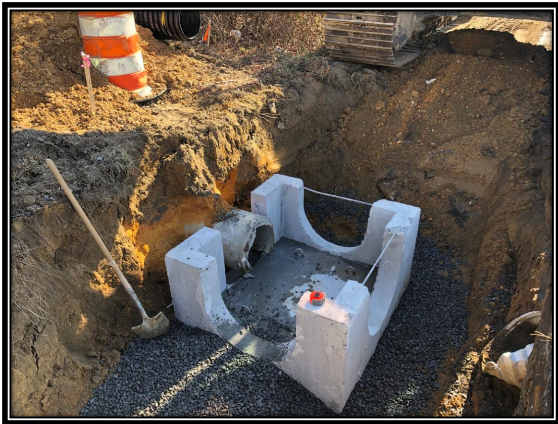
Figure: 1 – Installation of type B inlet along the southbound lane of Watsonstown-New Freedom Road (CR 691) in the Borough of Pine Hill
