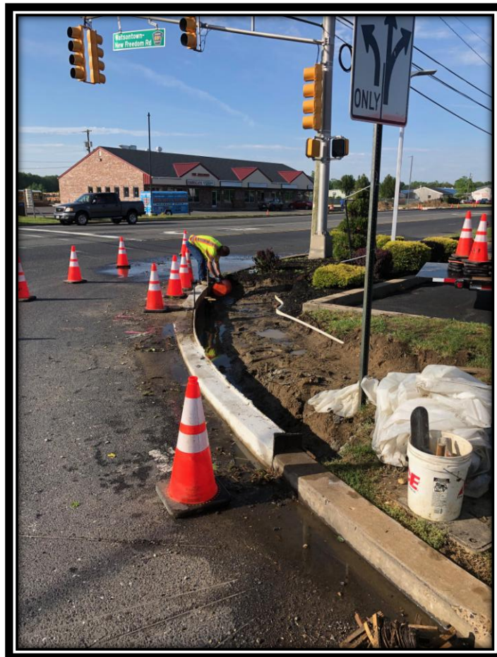
Figure: 1 – Installation of concrete curb for the proposed ADA ramp at the northwest corner of the intersection with Berlin-Cross Keys Road in the Borough of Berlin
