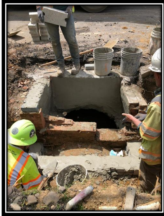
Figure: 2 – Reconstruction of existing inlet in the northbound lane of Watsontown-New Freedom Road (CR 691) between the White Horse Pike and Berlin-Clementon Road in the Borough of Clementon
