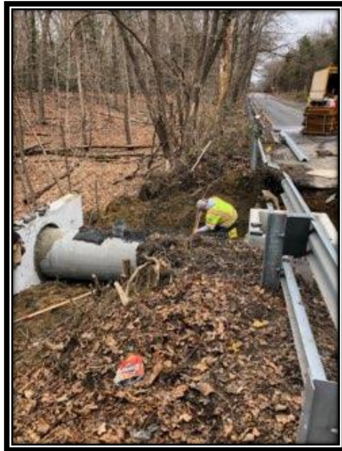
Figure: 1 – Installation of 30” concrete headwall, type B inlet and 30” RCP along the southbound lane of Watsonstown-New Freedom Road (CR 691) in the Borough of Pine Hill
