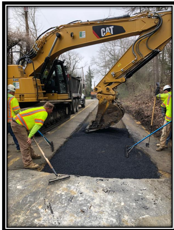
Figure: 3 – Asphalt restoration of the 36" RCP trench along the southbound lane of Watsontown-New Freedom Road (CR 691) in the Borough of Pine Hill
