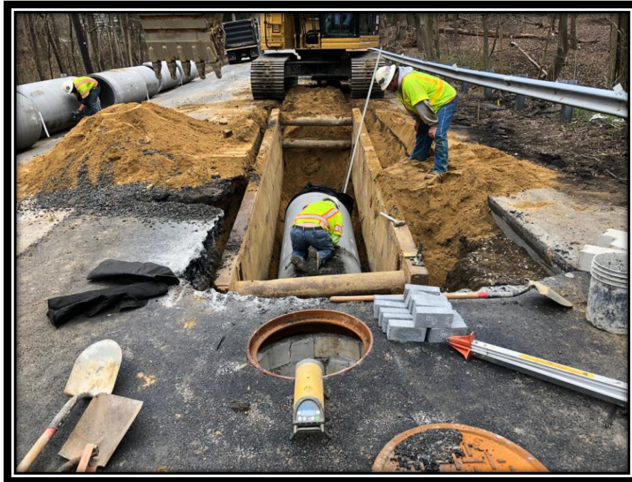
Figure: 3 – Installation of 36" RCP along the southbound lane of Watsontown-New Freedom Road (CR 691) between Berlin-Clementon Road and Carriage Stop Drive in the Borough of Pine Hill
