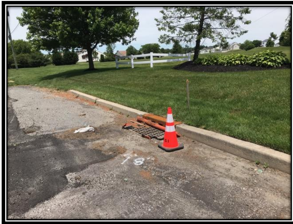
Figure: 3 – Installation of type ‘N’ eco inlet curb piece along the northbound lane between Westbury Drive and Carriage Stop Drive in the Borough of Berlin
