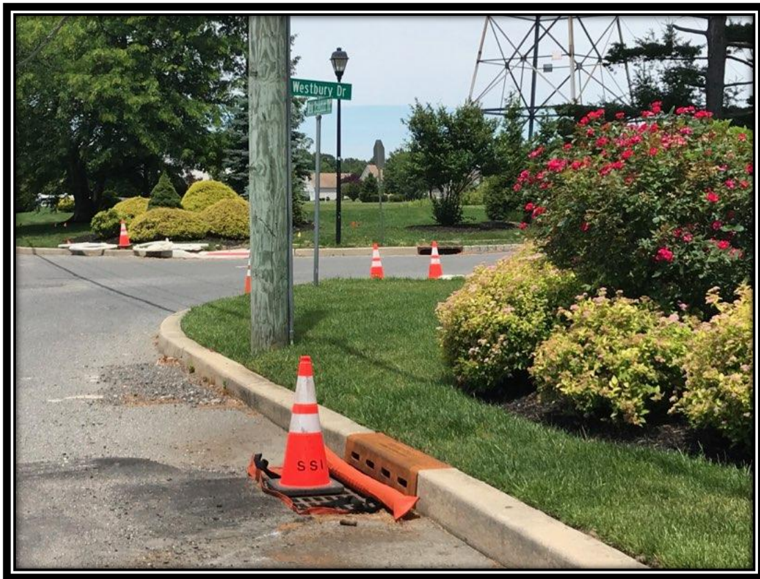
Figure: 1 – Installation of type 'N' eco inlet curb piece along the northbound lane approaching the intersection with Westbury Drive in the Borough of Berlin
