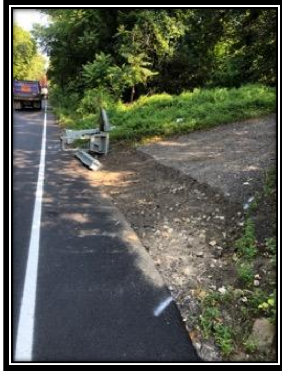
Figure: 2 – Preparation of subbase before installation of HMA driveway along the northbound lane between Carriage Stop Drive and Berlin-Clementon Road in the Borough of Berlin
