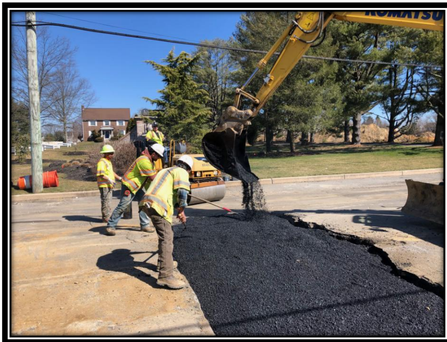
Figure: 3 – Asphalt restoration of the 36” RCP trench along the southbound lane of Watstown-New Freedom Road (CR 691) in the Borough of Pine Hill
