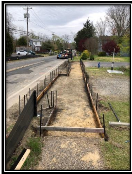
Figure: 2 – Installation of concrete driveway and sidewalk along the southbound lane of Watsontown-New Freedom Road (CR 691) between the White Horse Pike and Berlin-Clementon Road in the Borough of Clementon
