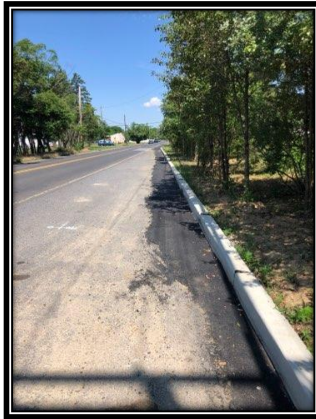
Figure: 1 – Base course trench restoration in front of the newly installed concrete curb along the northbound lane between Sequoia Drive and Wyndam Road in the Borough of Berlin
