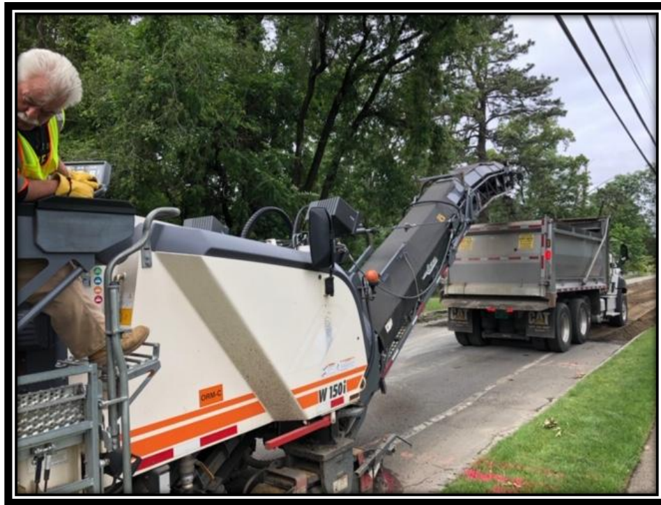
Figure: 2 – Removal of existing asphalt along gutters prior to full depth reclamation with cement between the White Horse Pike and Berlin Clementon Road in the Borough of Clementon
