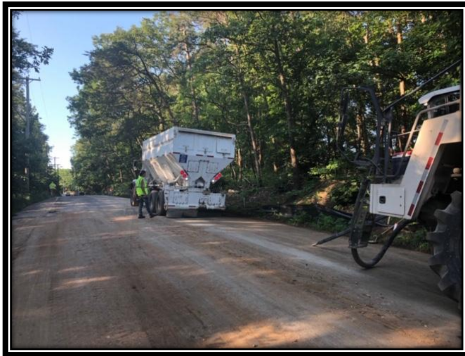
Figure: 3 – Full depth reclamation with cement between the White Horse Pike and Berlin Clementon Road in the Borough of Clementon
