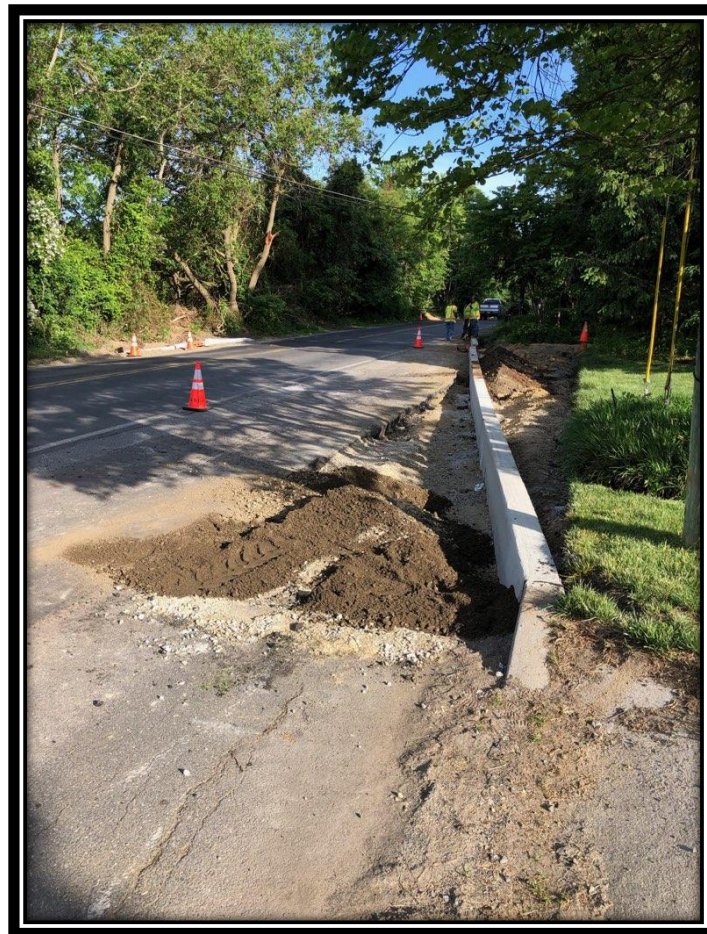
Figure: 1 – Installation of concrete curb in the northbound acceleration lane just past the intersection with Carriage Stop Drive in the Borough of Berlin
