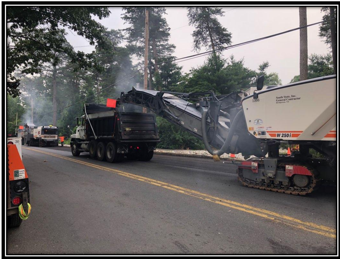
Figure: 1 – HMA milling in the southbound lane between Berlin-Clementon Road and Berlin-Cross Keys Road in the Borough of Pine Hill
