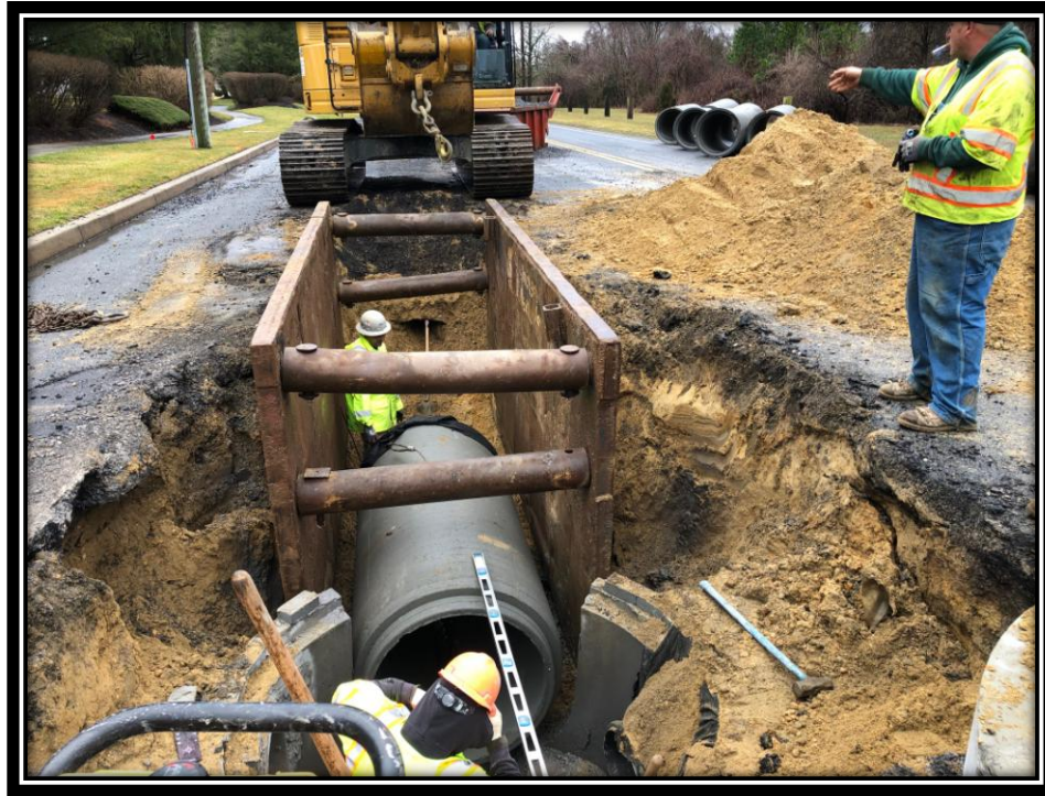
Figure: 2 – Installation of 36” RCP along the northbound lane of Watsontown-New Freedom Road (CR 691) in the Borough of Berlin
