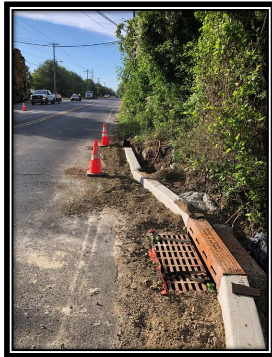
Figure: 2 – Installation of concrete curb along the southbound lane between Berlin-Clementon Road and Carriage Stop Drive in the Borough of Pine Hill
