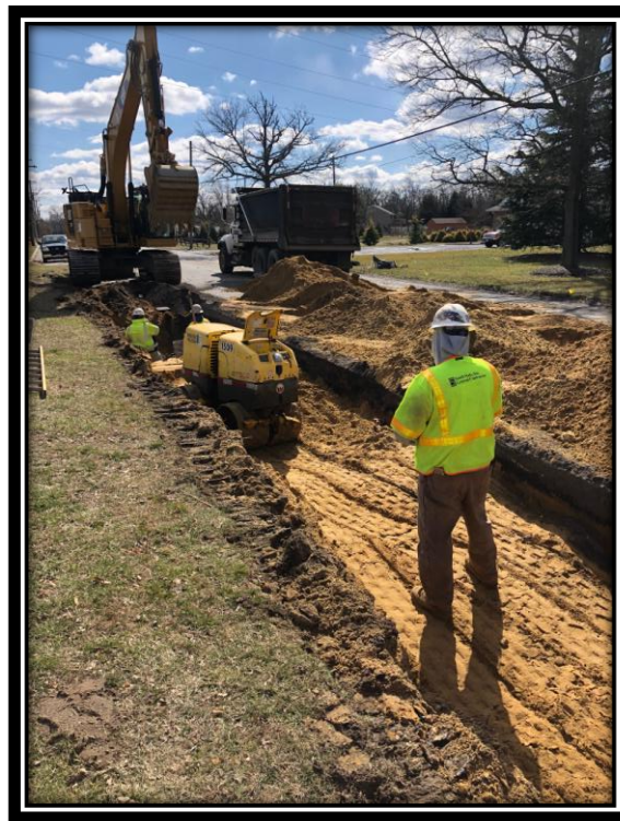
Figure: 3 – Backfill and compaction of the 24” RCP trench along the northbound lane of Watsontown-New Freedom Road (CR 691) in the Borough of Berlin
