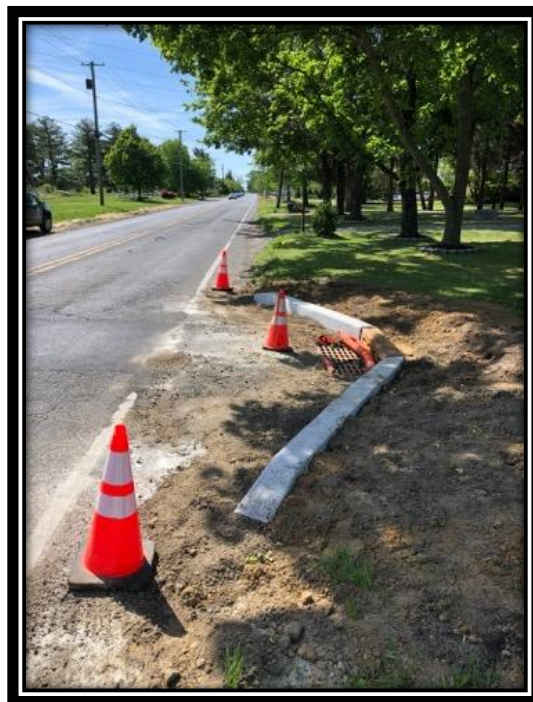
Figure: 3 – Installation of concrete curb along the northbound lane between Wyndam Road and Westbury Drive in the Borough of Berlin
