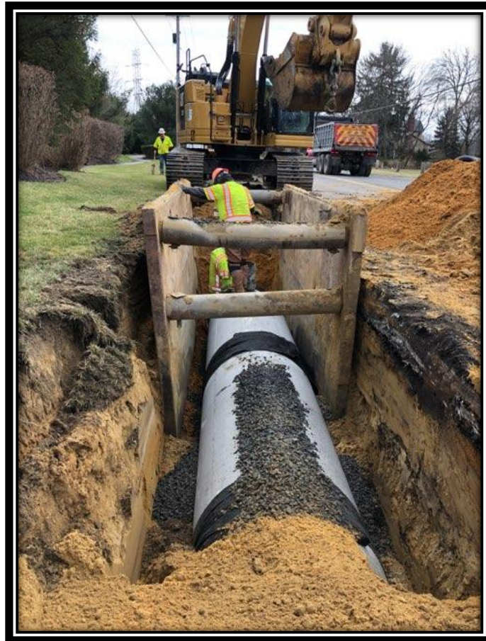
Figure: 1 – Installation of 36” RCP along the northbound lane of Watsonstown-New Freedom Road (CR 691) in the Borough of Berlin
