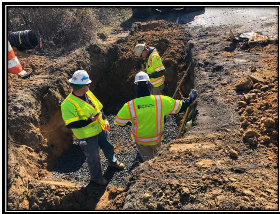
Figure: 3 – Backfill and compaction of the 18” RCP trench along the northbound lane of Watsontown-New Freedom Road (CR 691) in the Borough of Berlin
