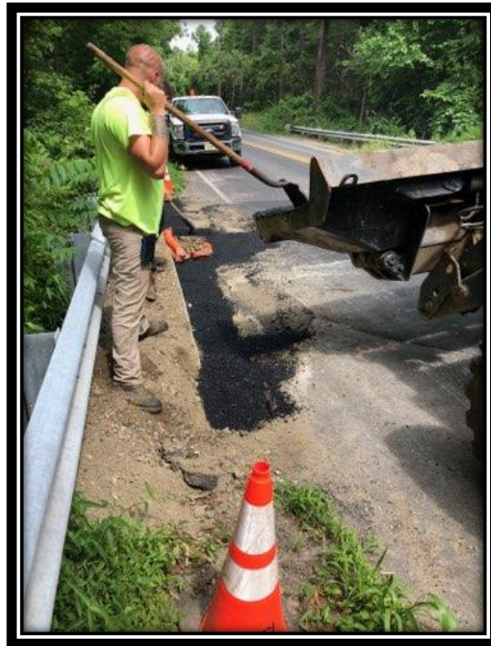
Figure: 3 – Road restoration at the newly installed storm sewer improvements along the southbound lane between Berlin-Clementon Road and Berlin-Cross Keys Road in the Borough of Pine Hill
