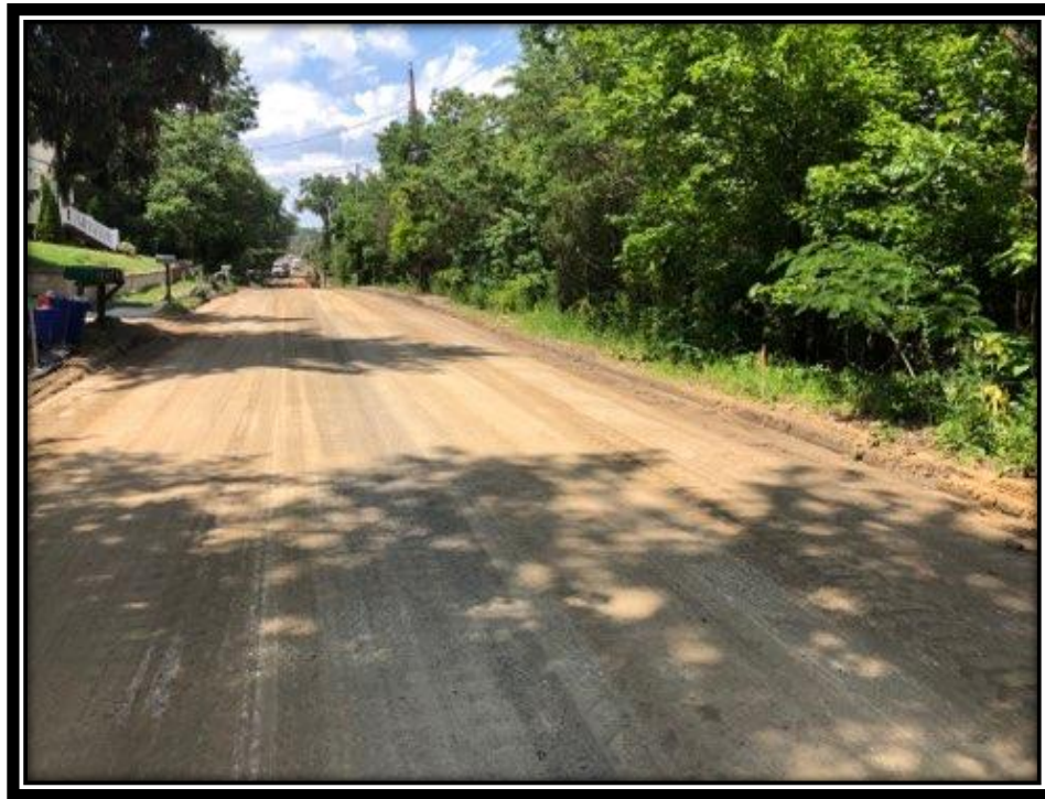
Figure: 2 – Final grading of the newly reclaimed roadway subbase between the White Horse Pike and Berlin-Clementon Road in the Borough of Clementon
