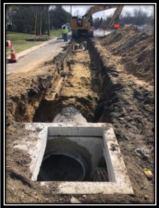
Figure: 3 – Installation of 36” RCP along the northbound lane of Watstown-New Freedom Road (CR 691) in the Borough of Berlin approaching Carriage Stop Drive
