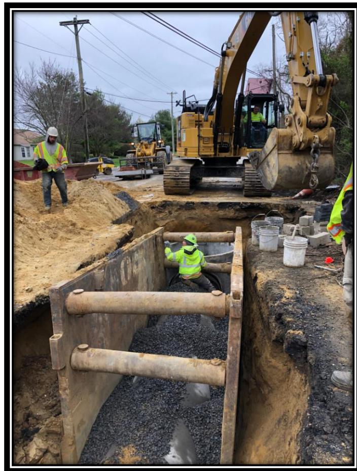
Figure: 1 – Installation of 36” RCP along the southbound lane of Watsonstown-New Freedom Road (CR 691) in the Borough of Pine Hill
