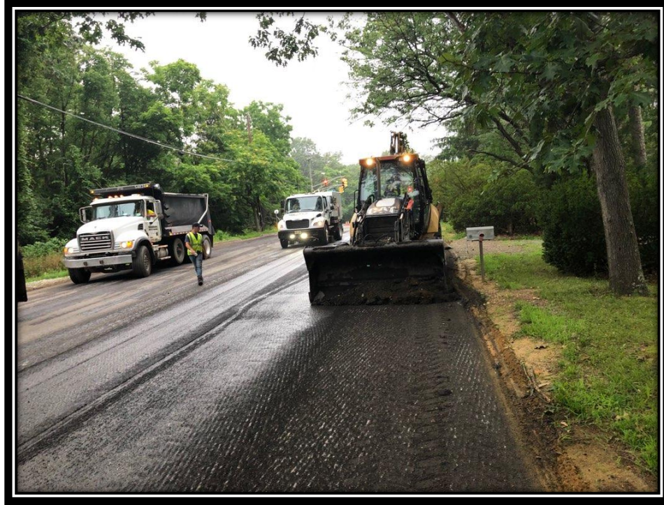
Figure: 2 – Clearing of edge of paving after completion of milling in the northbound lane Berlin-Clementon Road and Berlin-Cross Keys Road in the Borough of Berlin
