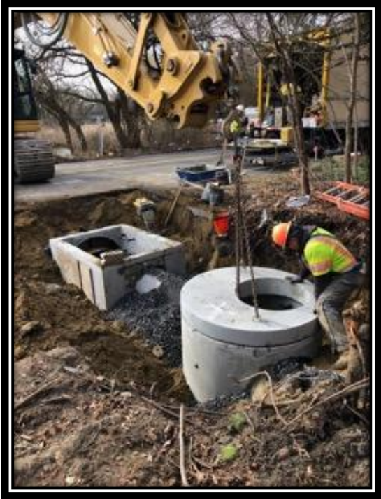
Figure: 2 – Installation of 4’ diameter storm sewer manhole, type B inlet and 18” RCP along the northbound lane of Watstown-New Freedom Road (CR 691) in the Borough of Berlin
