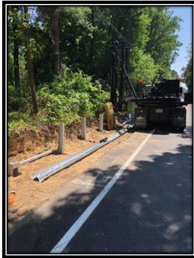
Figure: 1 – Installation of beam guide rail along the southbound lane between Berlin-Clementon Road and Carriage Stop Drive in the Borough of Pine Hill
