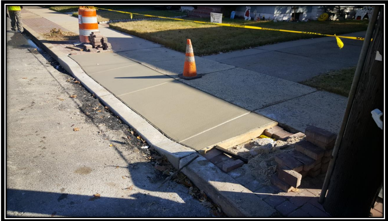
Figure: 2 – Installation of concrete driveway apron between 45 th Street and 46 th Street along the eastbound lane
