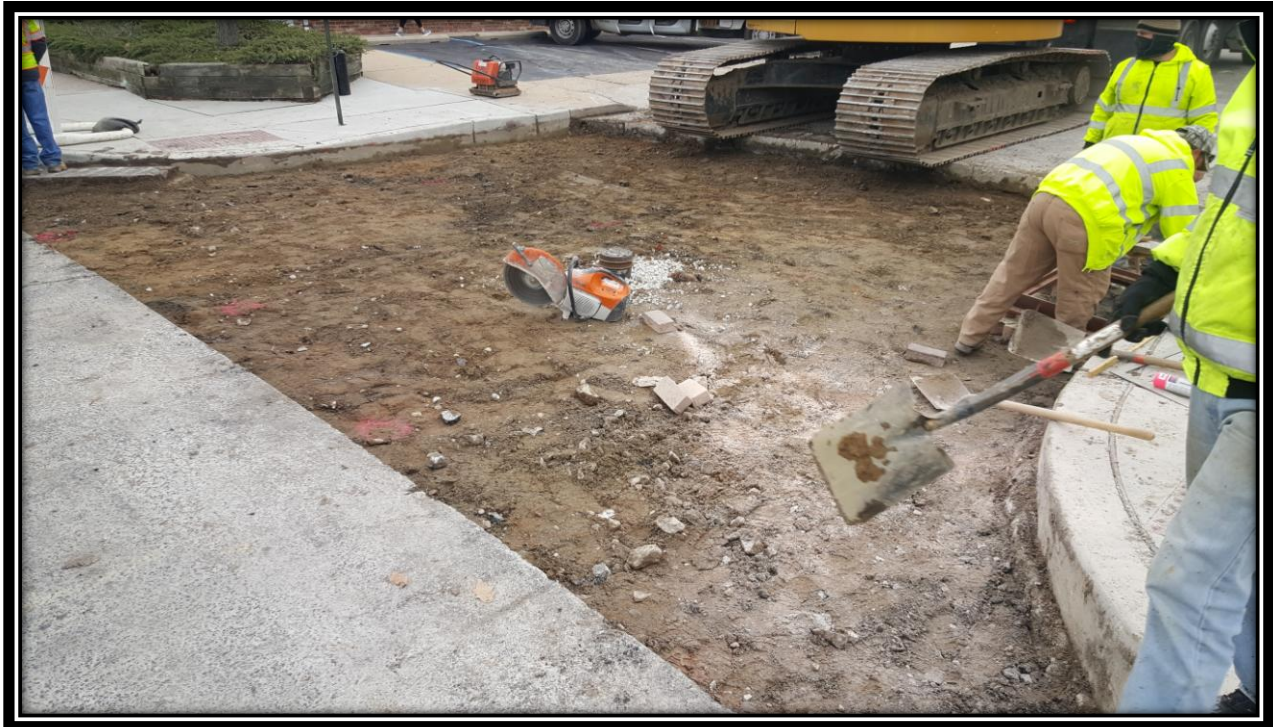
Figure: 2 – Replacement of water valve and inlet grate at the intersection with 46 th Street along the eastbound lane
