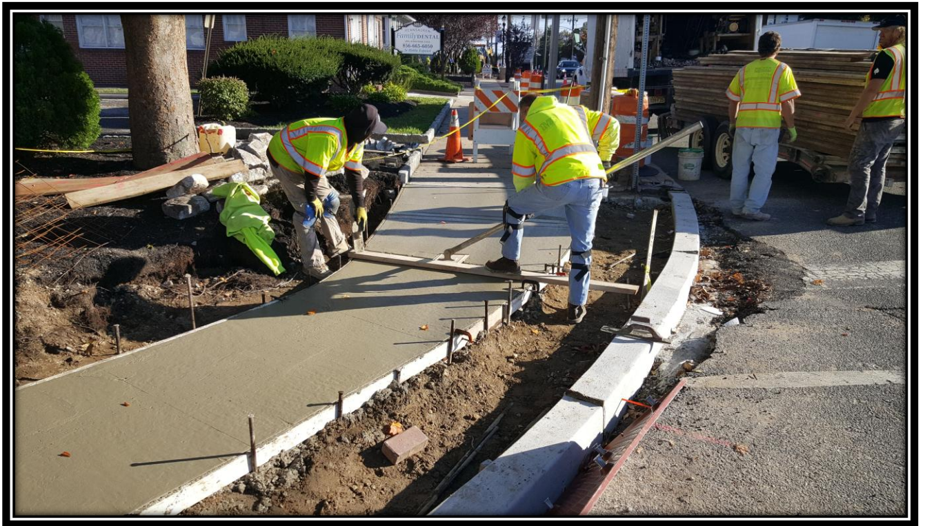
Figure: 1 – Installation of a concrete sidewalk at the northeast corner of the intersection with Browning Road along the westbound lane
