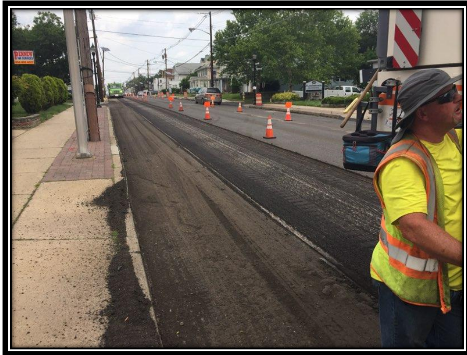
Figure: 2 – HMA milling of the eastbound lane between 42 nd Street and Browning Road
