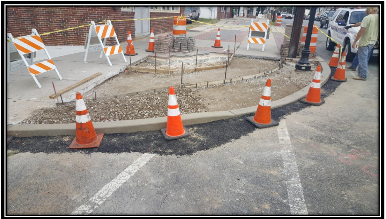
Figure: 3 – Installation of concrete curb at the northeast corner of the intersection with 48 th Street along the westbound lane
