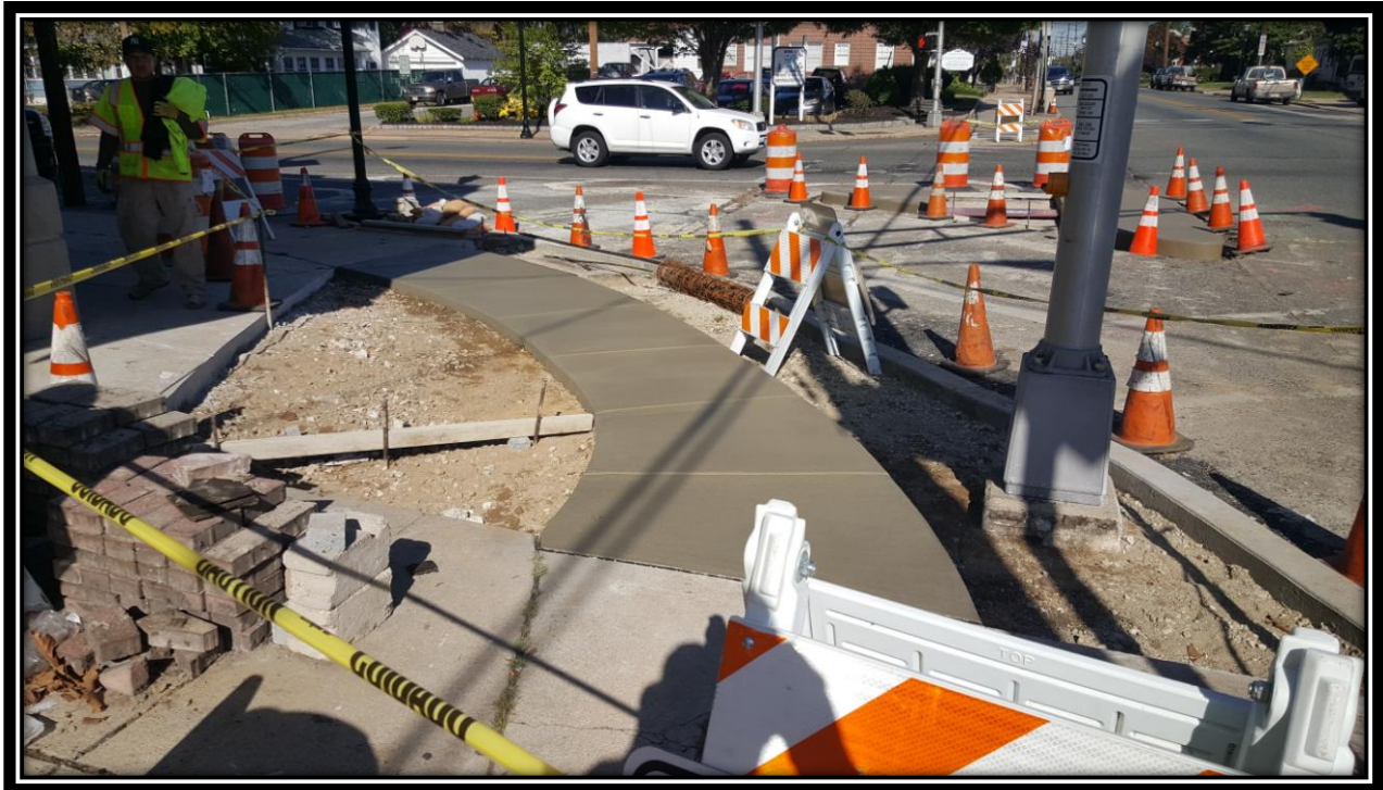
Figure: 2 – Installation of concrete sidewalk at the northwest corner of the intersection with Browning Road along the westbound lane
