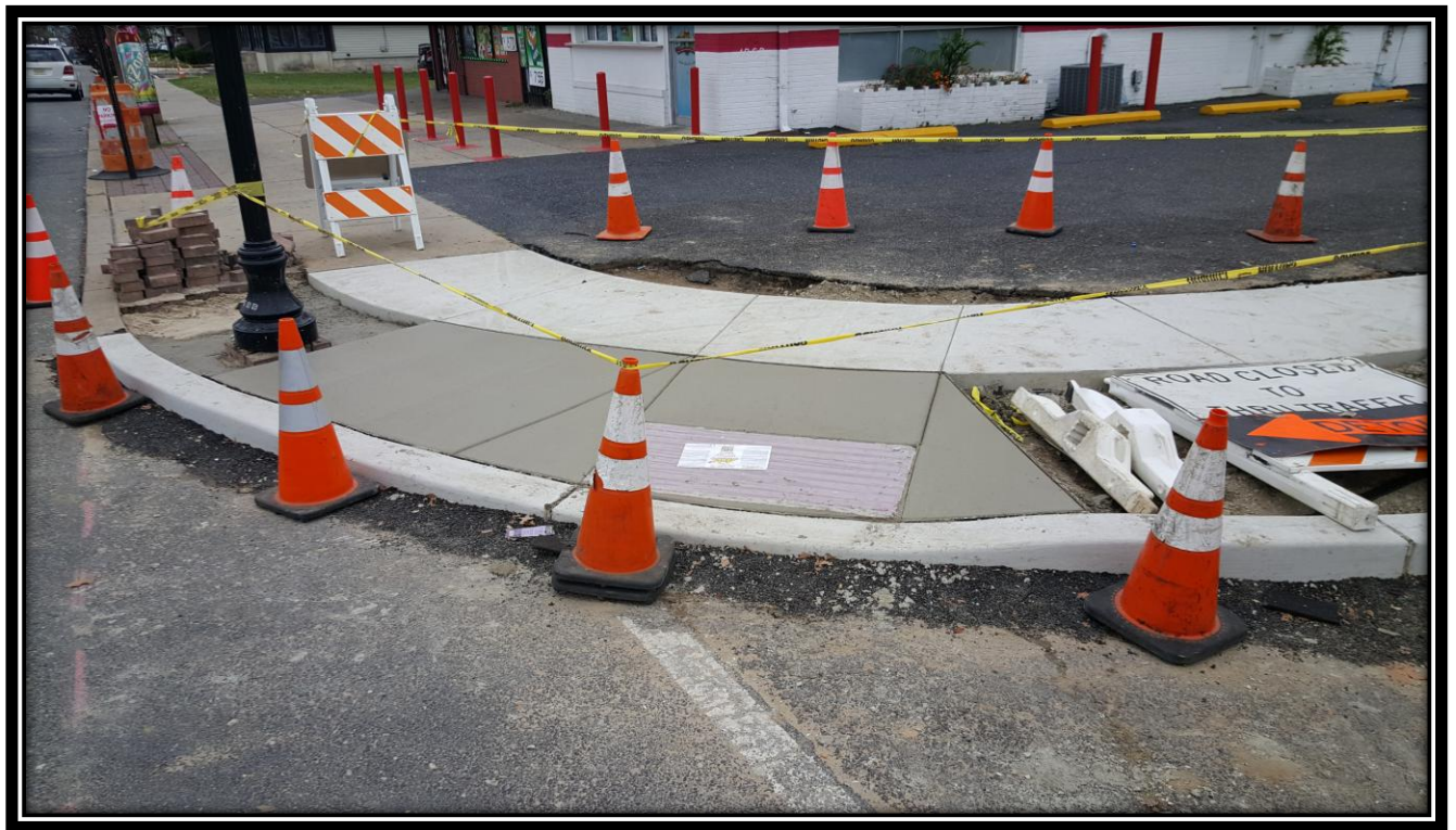
Figure: 1 – Installation of a concrete ADA ramp at the northwest corner of the intersection with 48 th Street along the westbound lane
