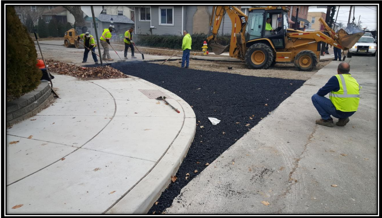
Figure: 2 – Installation of HMA 19M64 base course at the intersection with Tinsman Avenue along the westbound lane
