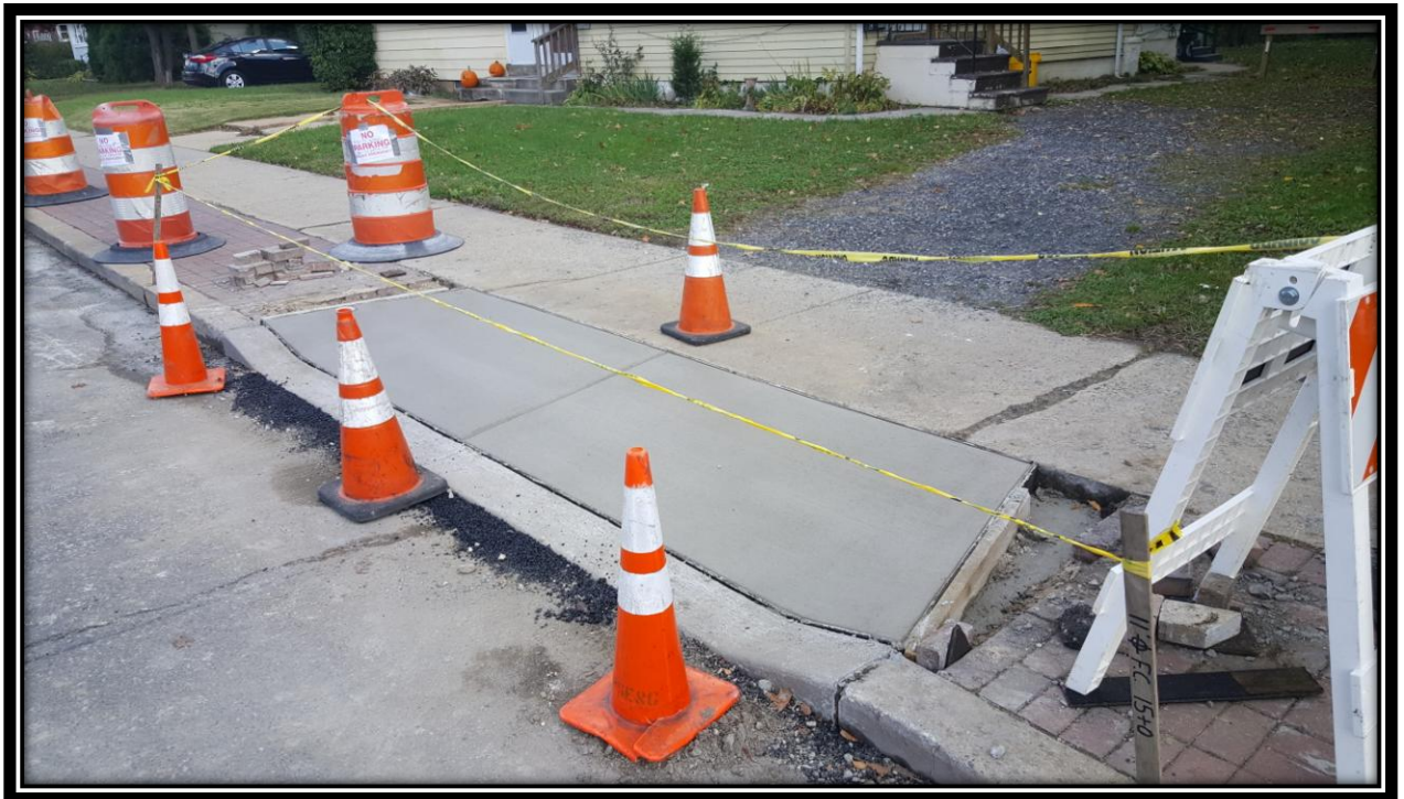
Figure: 3 – Installation of concrete driveway apron between Tinsman Avenue and Browning Road along the eastbound lane
