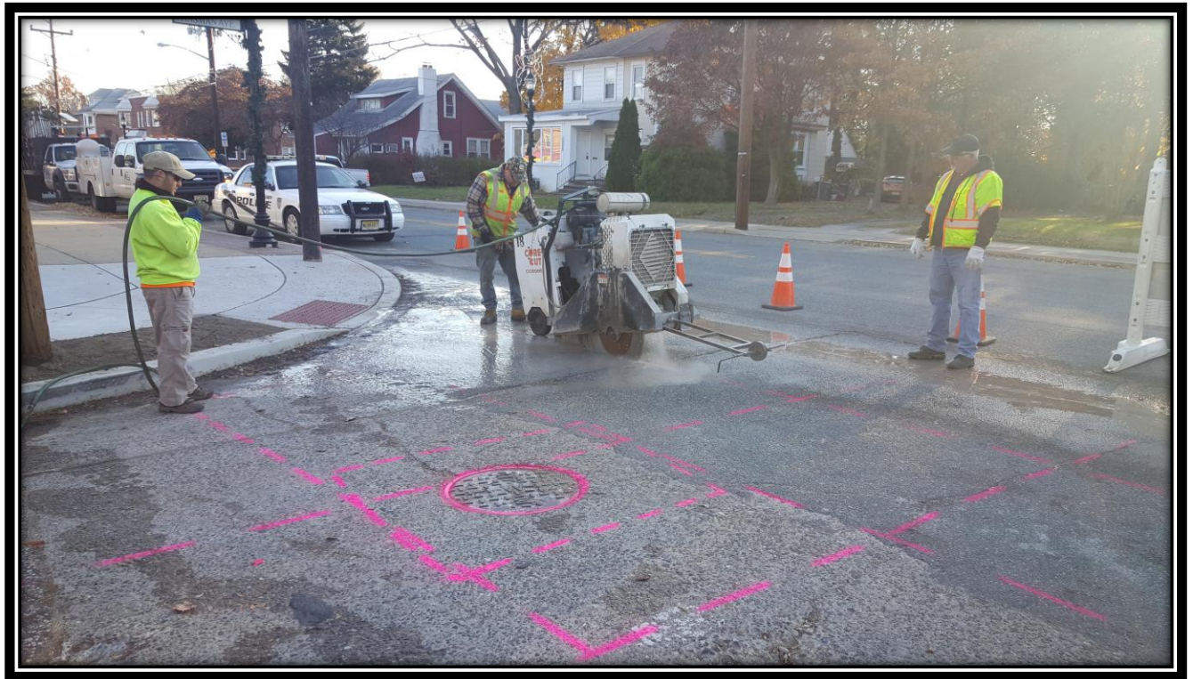
Figure: 1 – Sawcutting of existing concrete roadway to be removed at the intersection with Tinsman Avenue along the westbound lane
