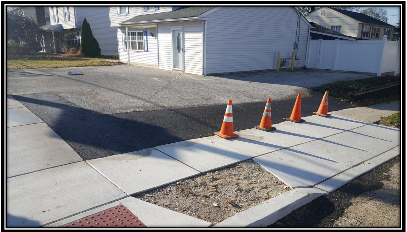
Figure: 1 – Installation of HMA driveway at the northwest corner of the intersection with 45 th Street along the westbound lane
