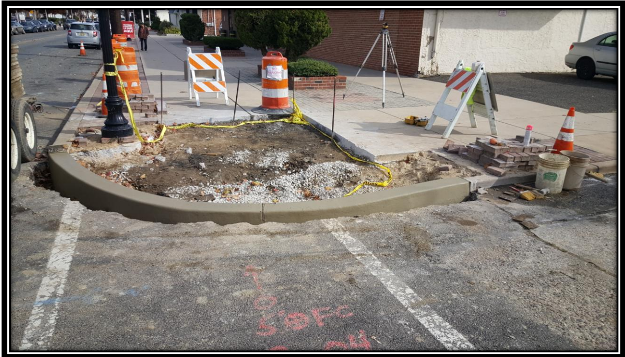
Figure: 2 – Installation of concrete curb at the southeast corner of the intersection with 49 th Street along the eastbound lane
