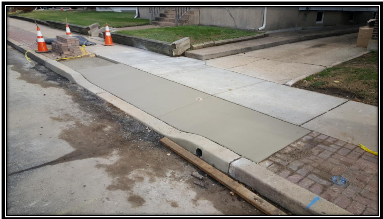
Figure: 3 – Installation of reinforced concrete driveway apron between 46 th Street and 47 th Street along the eastbound lane
