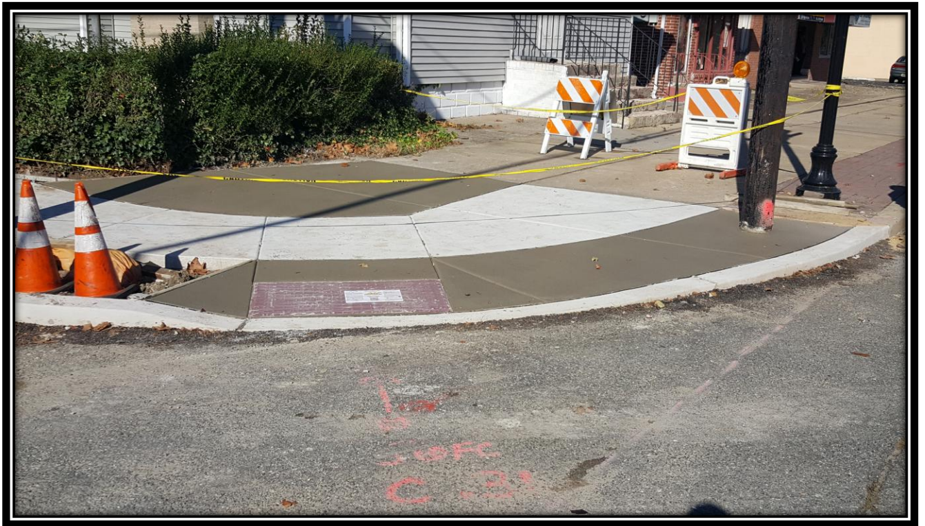
Figure: 1 – Installation of a concrete ADA ramp at the northeast corner of the intersection with Tinsman Avenue along the westbound lane
