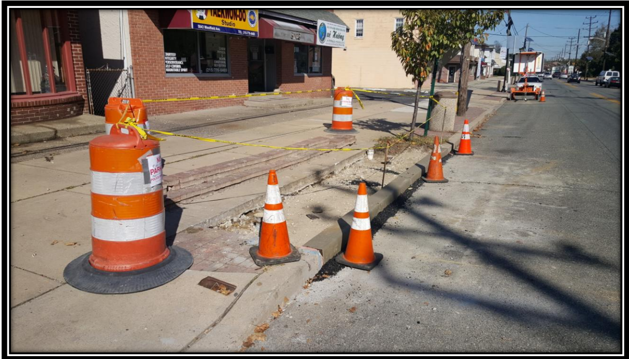
Figure: 2 – Installation of concrete curb at between Tinsman Avenue and Lexington Avenue along the westbound lane
