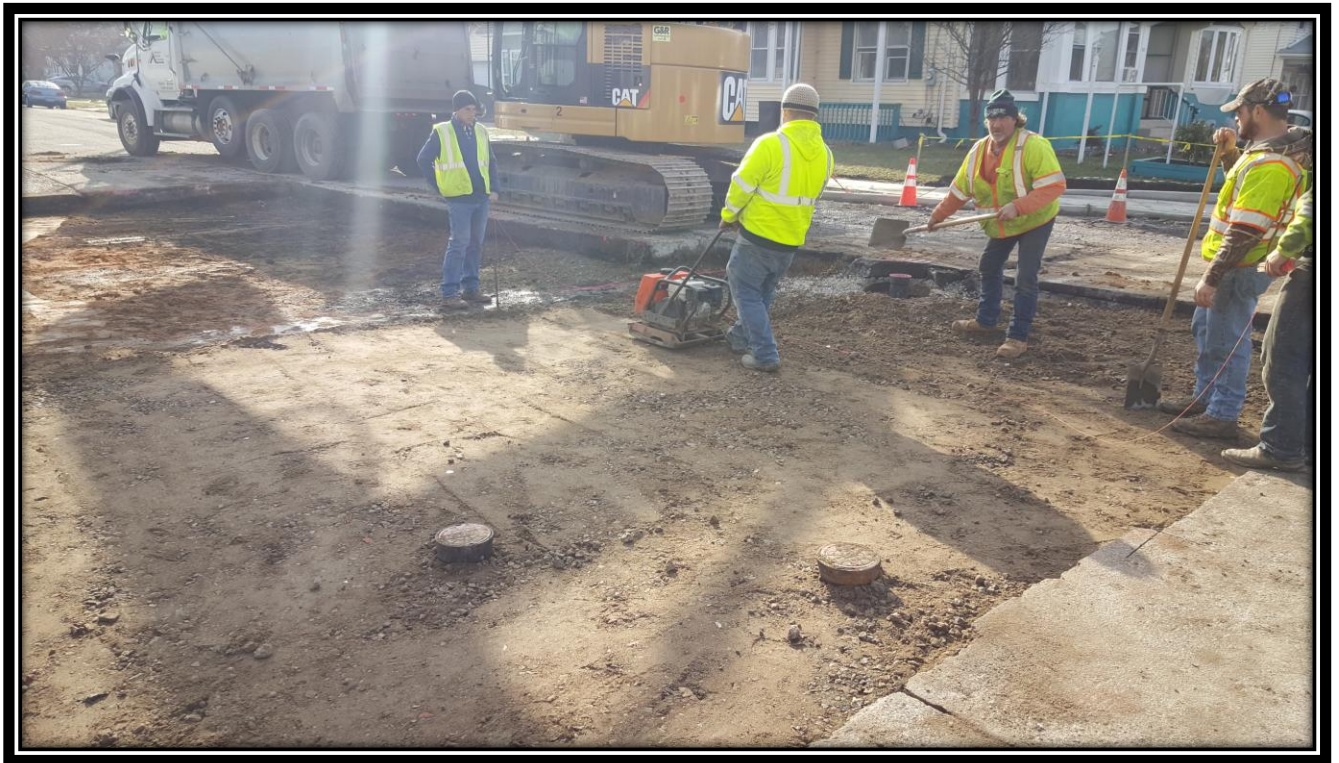
Figure: 1 – Installation of dense graded aggregate base course at the intersection with 44 th Street along the eastbound lane
