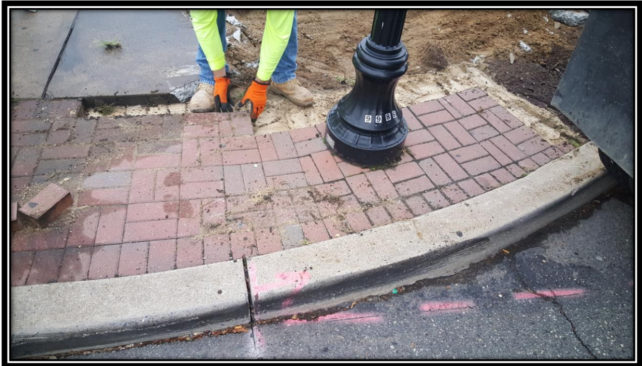
Figure: 2 – Resetting of brick pavers at northwest corner of the intersection with 46th Street along the westbound lane
