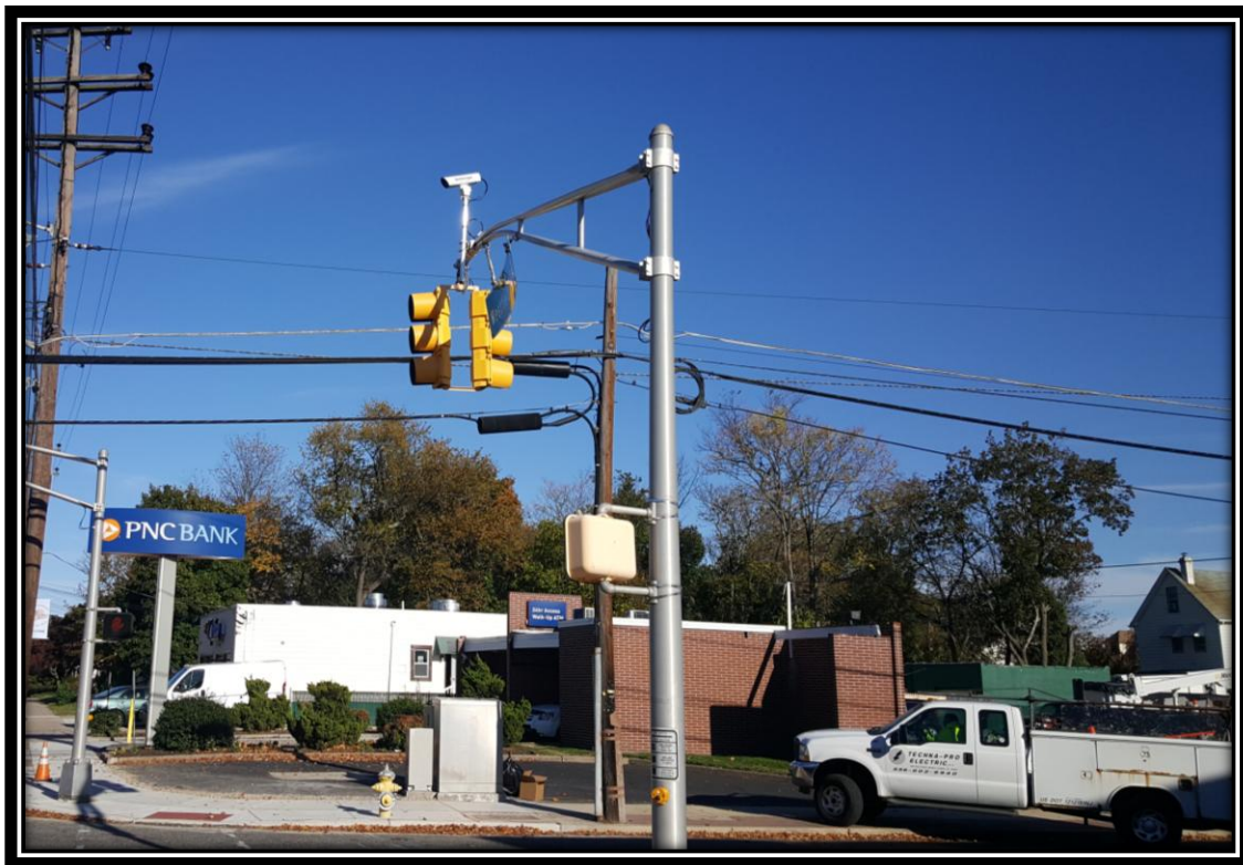
Figure: 3 – Installation of traffic image detector cameras at the intersection with Browning Road
