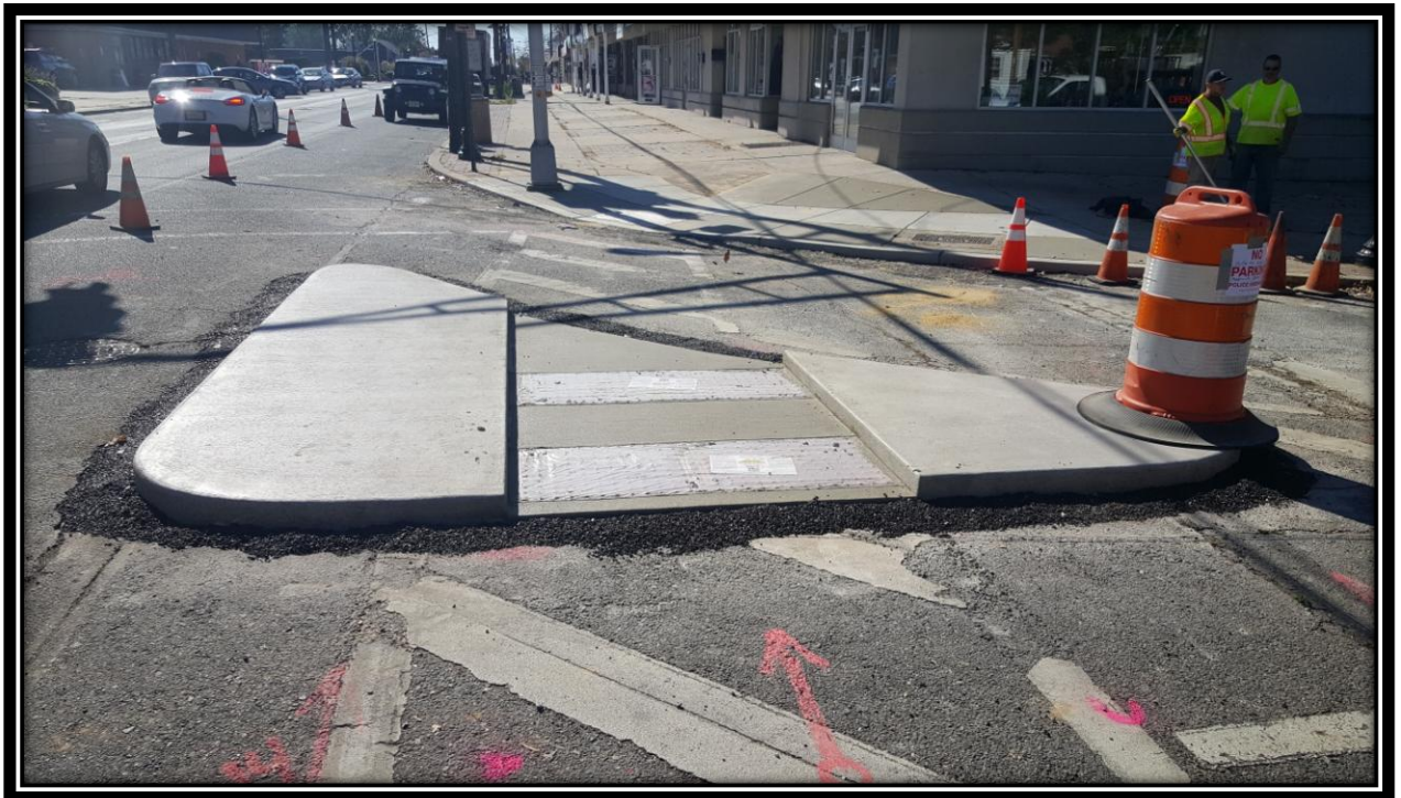
Figure: 3 –Installation of concrete island and ADA ramp at the intersection with Browning Road along the westbound lane
