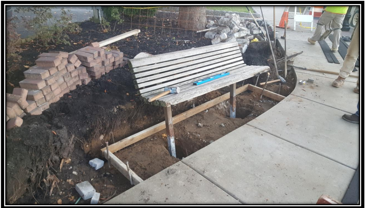
Figure: 3 – Resetting of an existing bench at the northeast corner of the intersection with Browning Road along the westbound lane
