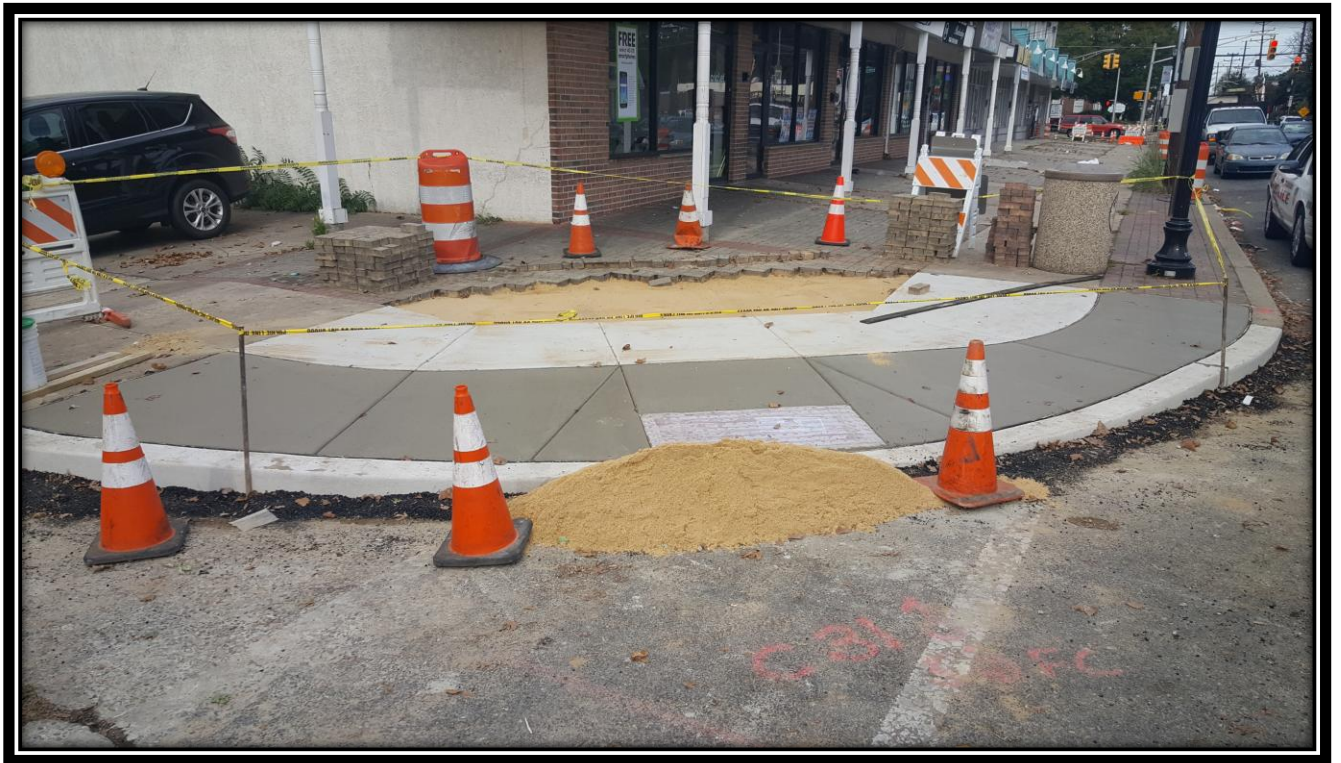
Figure: 1 – Installation of a concrete ADA ramp at the northeast corner of the intersection with 49 th Street along the westbound lane
