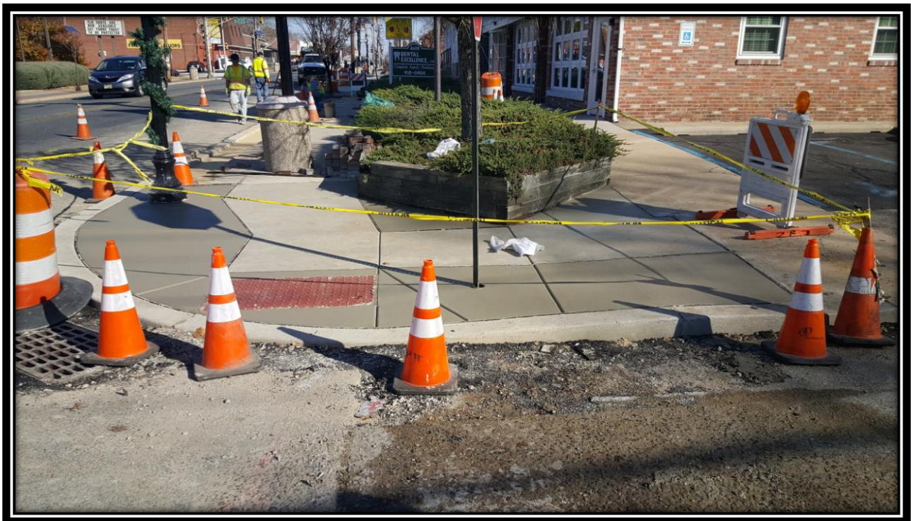
Figure: 3 – Installation of ADA ramp at the southeast corner of the intersection with 46 th Street along the eastbound lane
