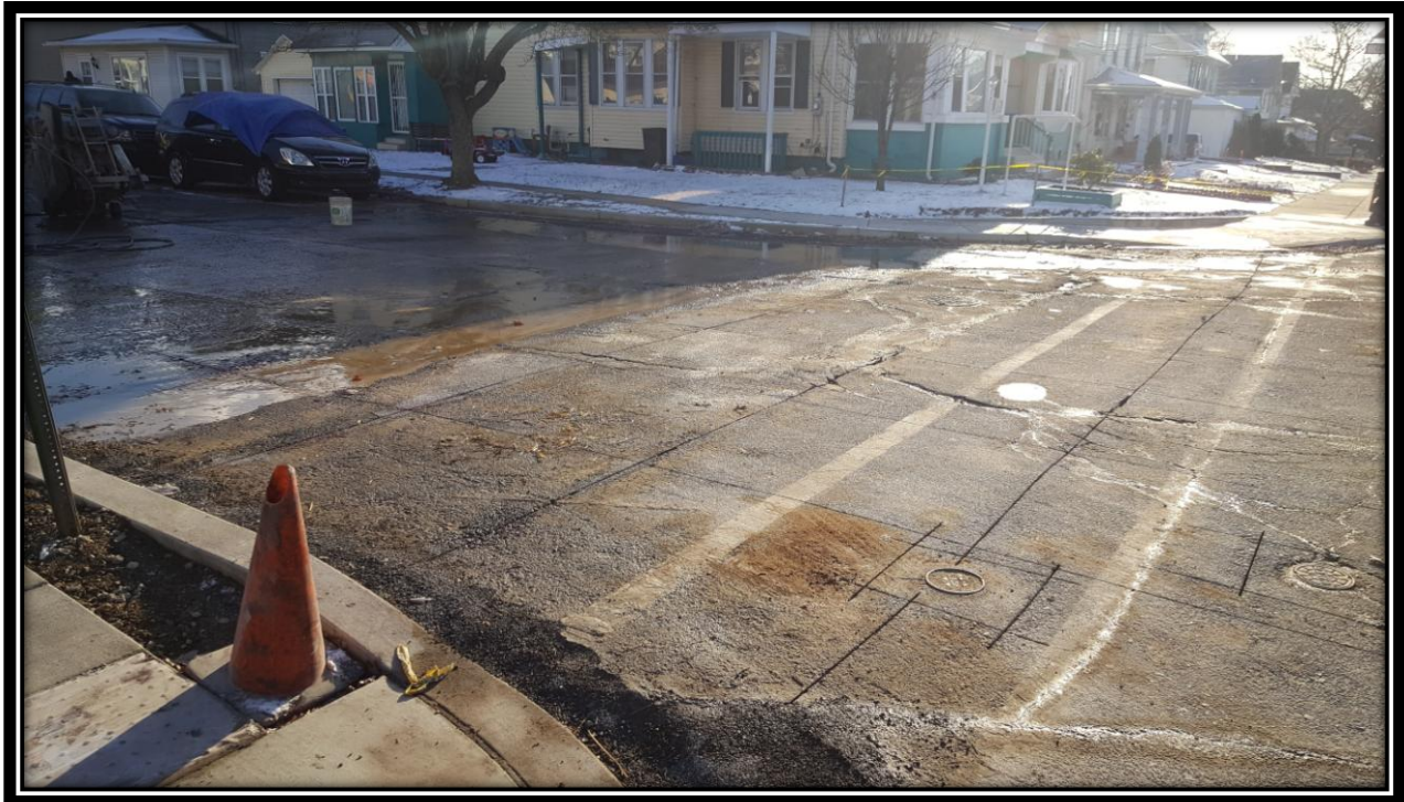
Figure: 2 – Saw cutting of the existing roadway at the intersection with 44 th Street along the eastbound lane
