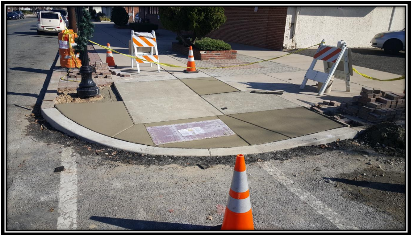
Figure: 1 – Installation of ADA ramp at the southeast corner of the intersection with 49 th Street along the eastbound lane
