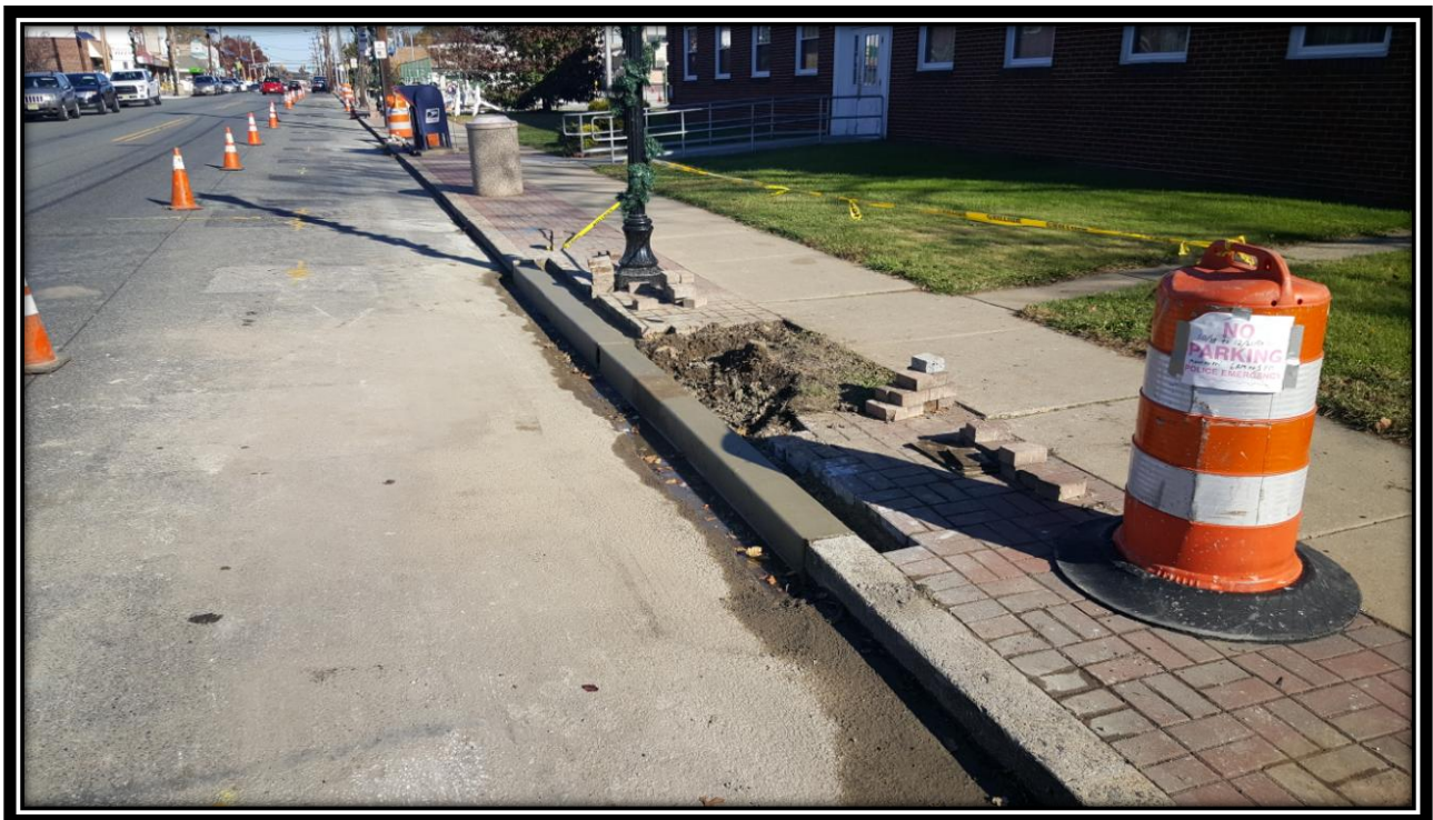
Figure: 3 – Installation of concrete curb between 47 th Street and 48 th Street along the eastbound lane
