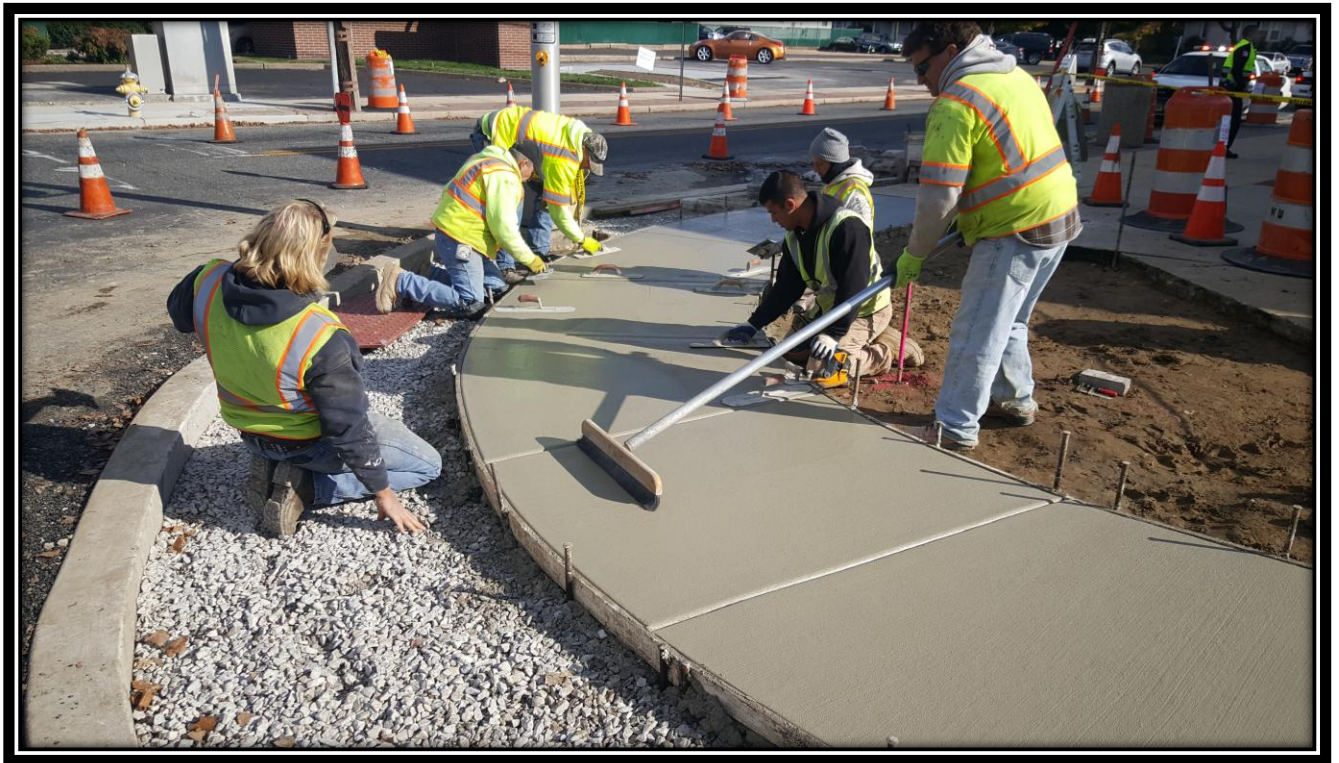
Figure: 1 – Installation of a concrete sidewalk at the southwest corner of the intersection with Browning Road along the eastbound lane
