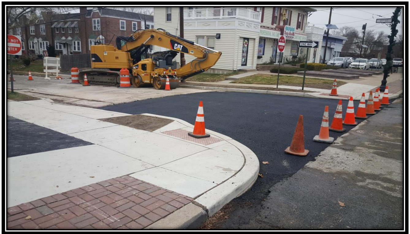
Figure: 1 – Installation of HMA 19M64 base course at the intersection with 45 th Street along the westbound lane
