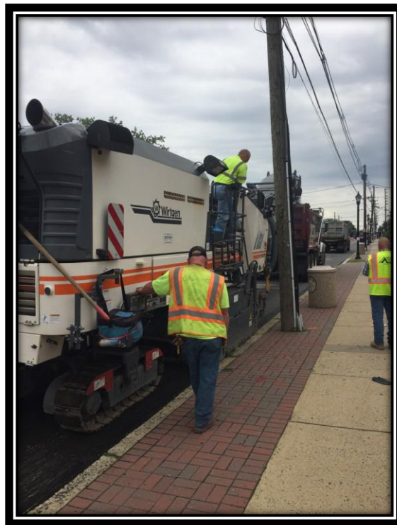
Figure: 3 – HMA milling of the westbound lane between 42 nd Street and Browning Road
