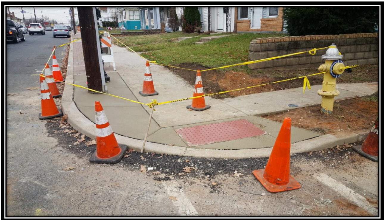
Figure: 3 – Installation of ADA ramp at the southeast corner of the intersection with 43 rd Street along the eastbound lane
