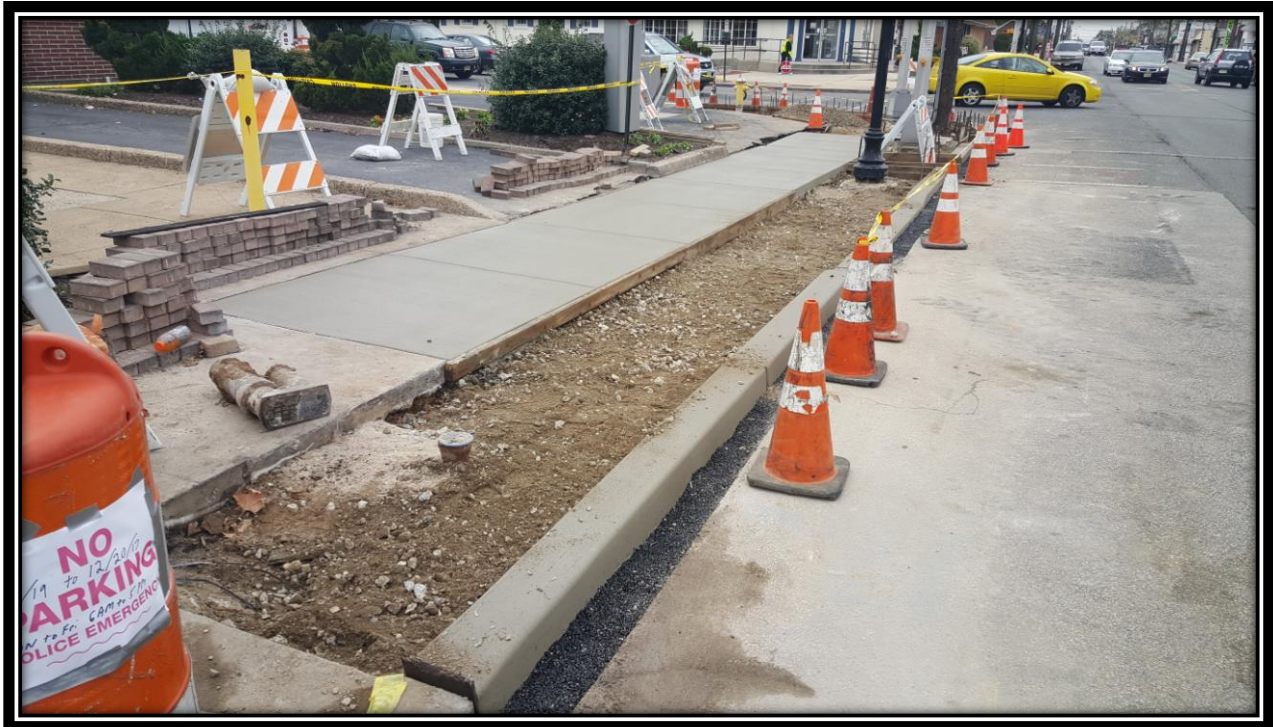
Figure: 2 – Installation of concrete sidewalk the northeast corner of the intersection with Browning Road along the eastbound lane
