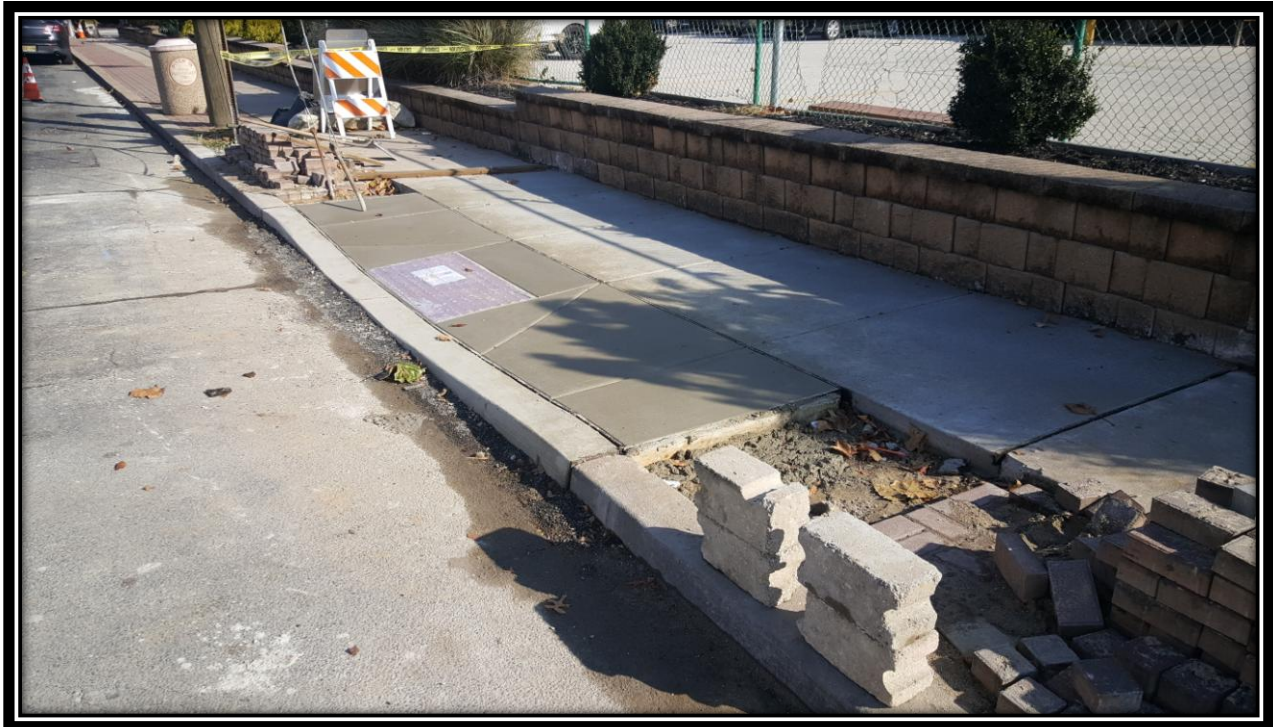
Figure: 2 – Installation of midblock ADA ramp between 48 th Street and 49 th Street along the eastbound lane
