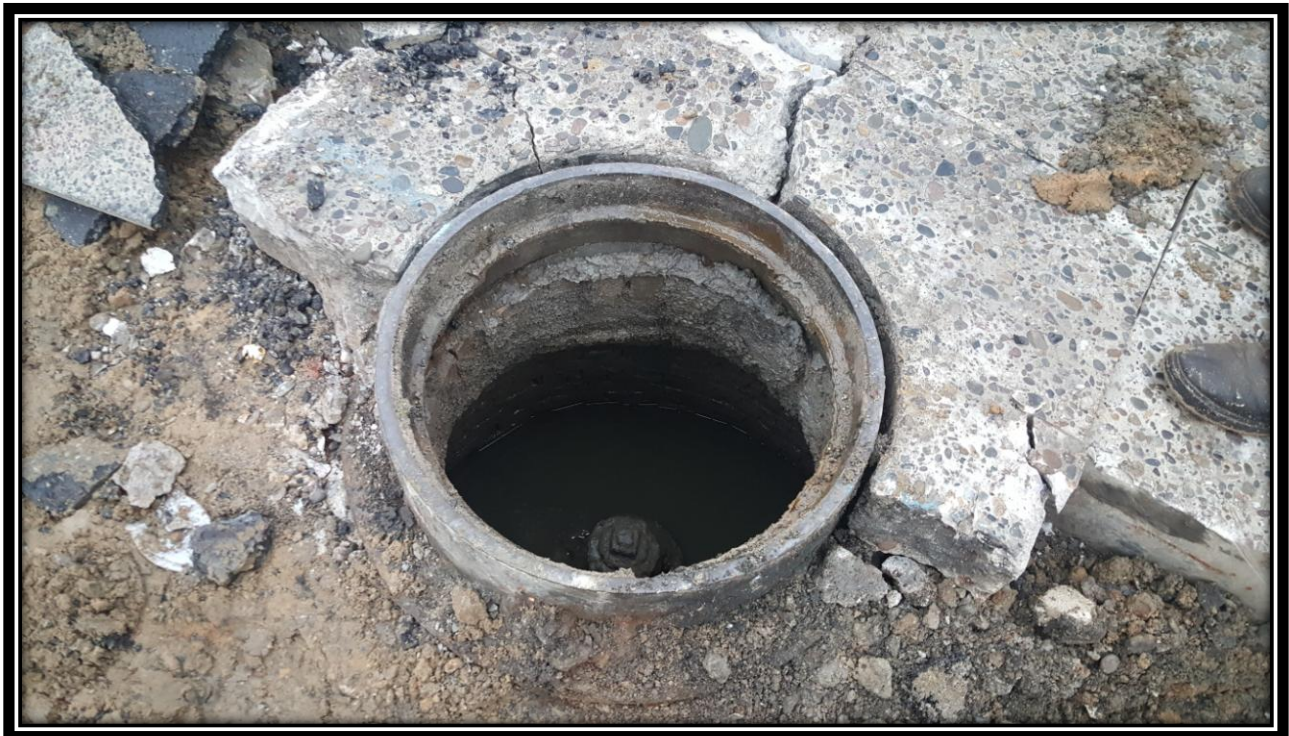
Figure: 3 – Resetting of the existing water manhole in the intersection with 47 th Street along the eastbound lane
