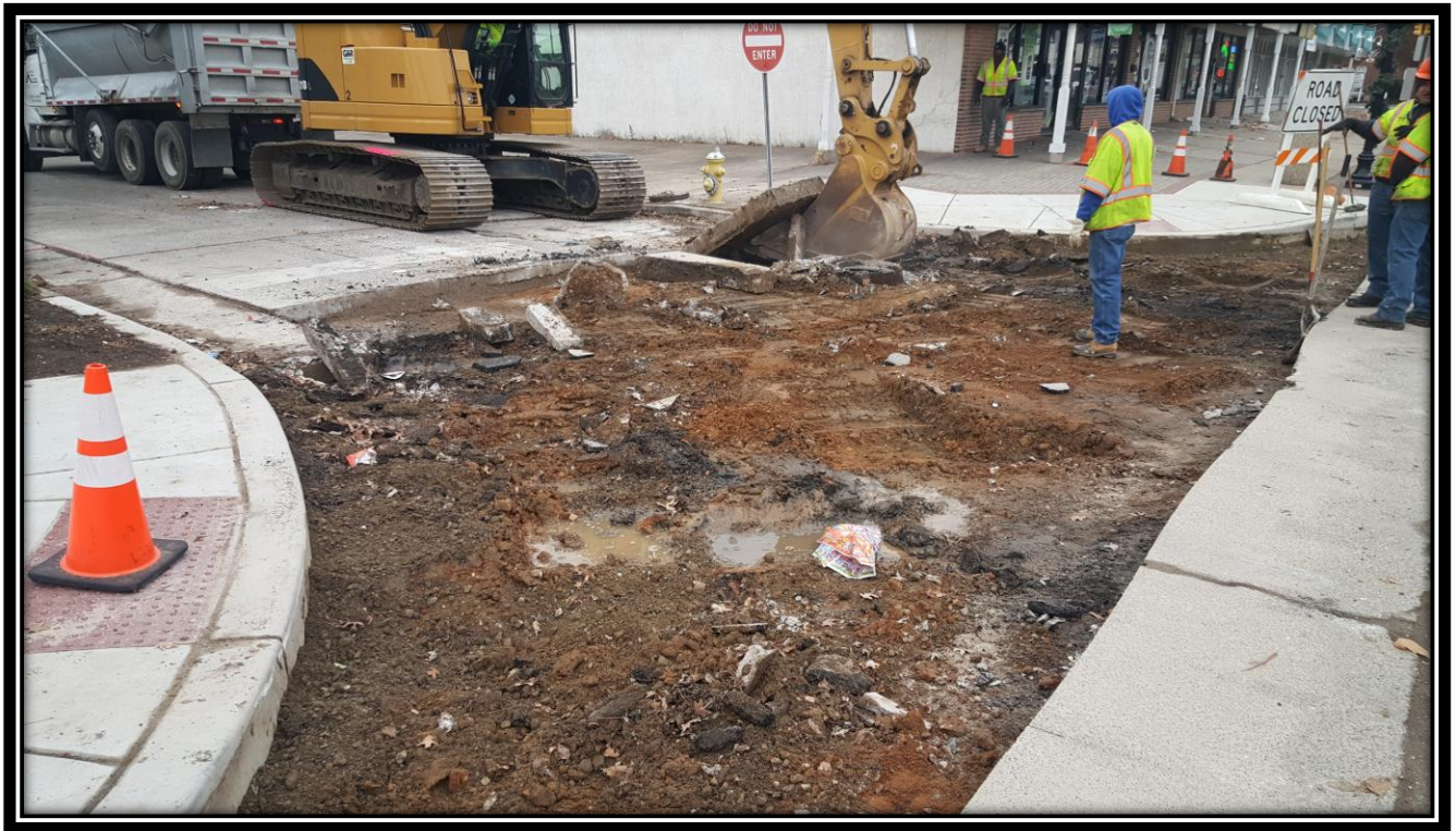
Figure: 1 – Removal of existing concrete roadway at the intersection with 49 th Street along the westbound lane
