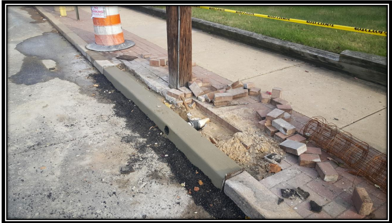
Figure: 2 – Installation of concrete curb between 46 th Street and 47 th Street along the eastbound lane
