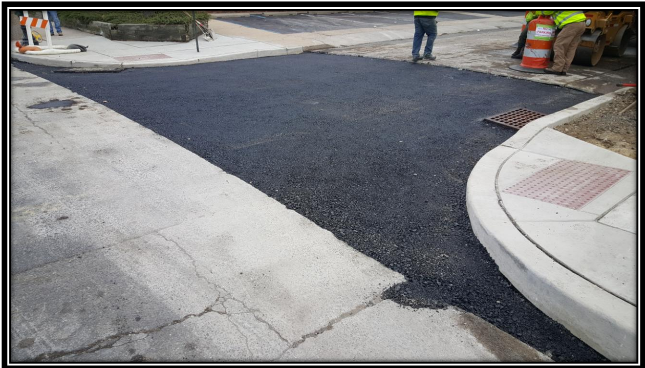
Figure: 3 – Installation of HMA 19M64 base course at the intersection with 46 th Street along the eastbound lane
