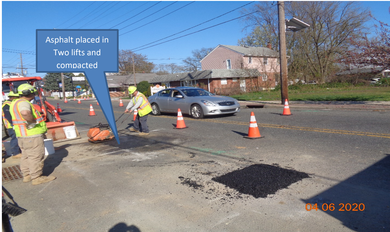
Figure 3: PSE&G Gas- Asphalt placement for excavated area along Westfield Avenue at Hillcrest Avenue
