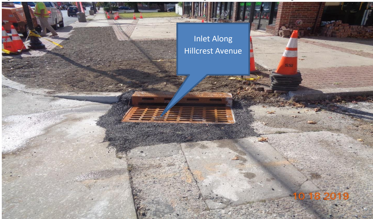
Figure 10: Inlet along Hillcrest Avenue – Reconstructed Inlet Type B using new casting and set curb piece Type N ECO
