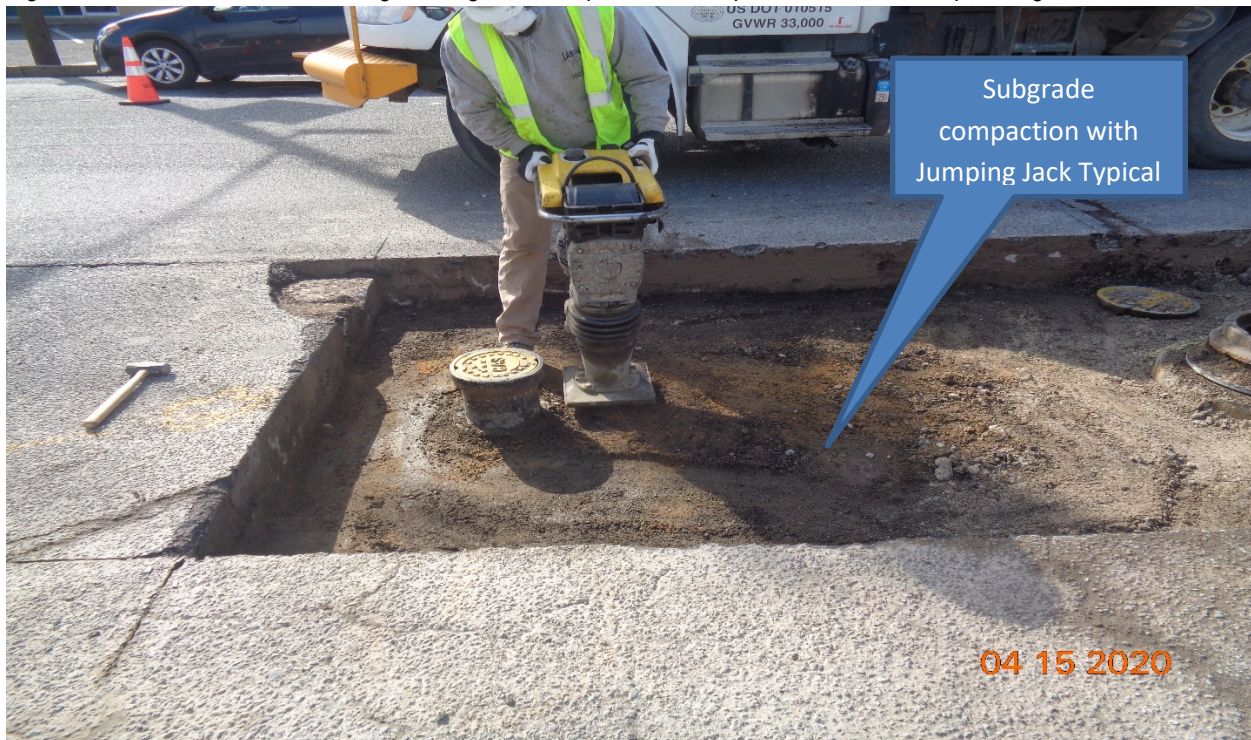
Figure 6: PSE&G Gas – Compaction of subgrade with jumping jack. – Typical at Each location
