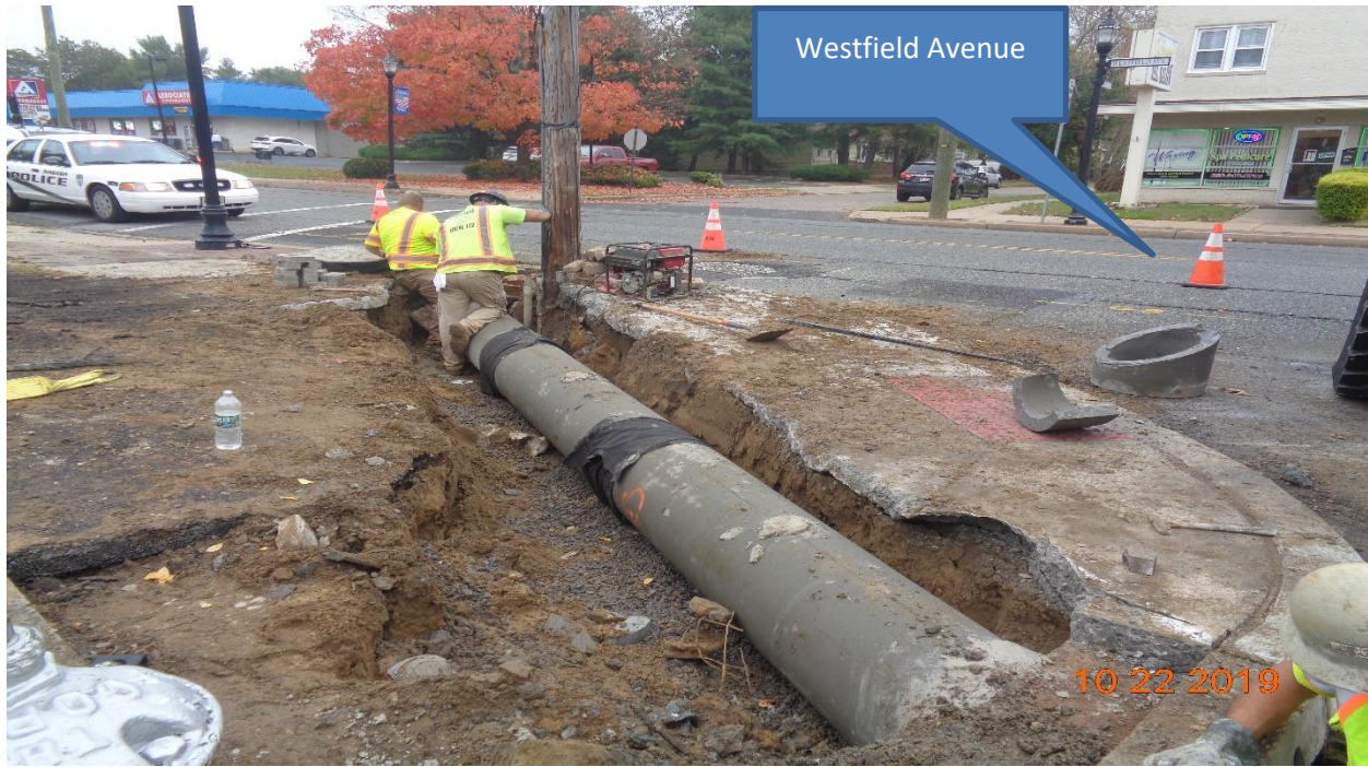
Figure 5: 15" Reinforced Concrete Pipe was installed from inlet along Westfield Avenue to East Inlet along Horner Avenue, LT.
