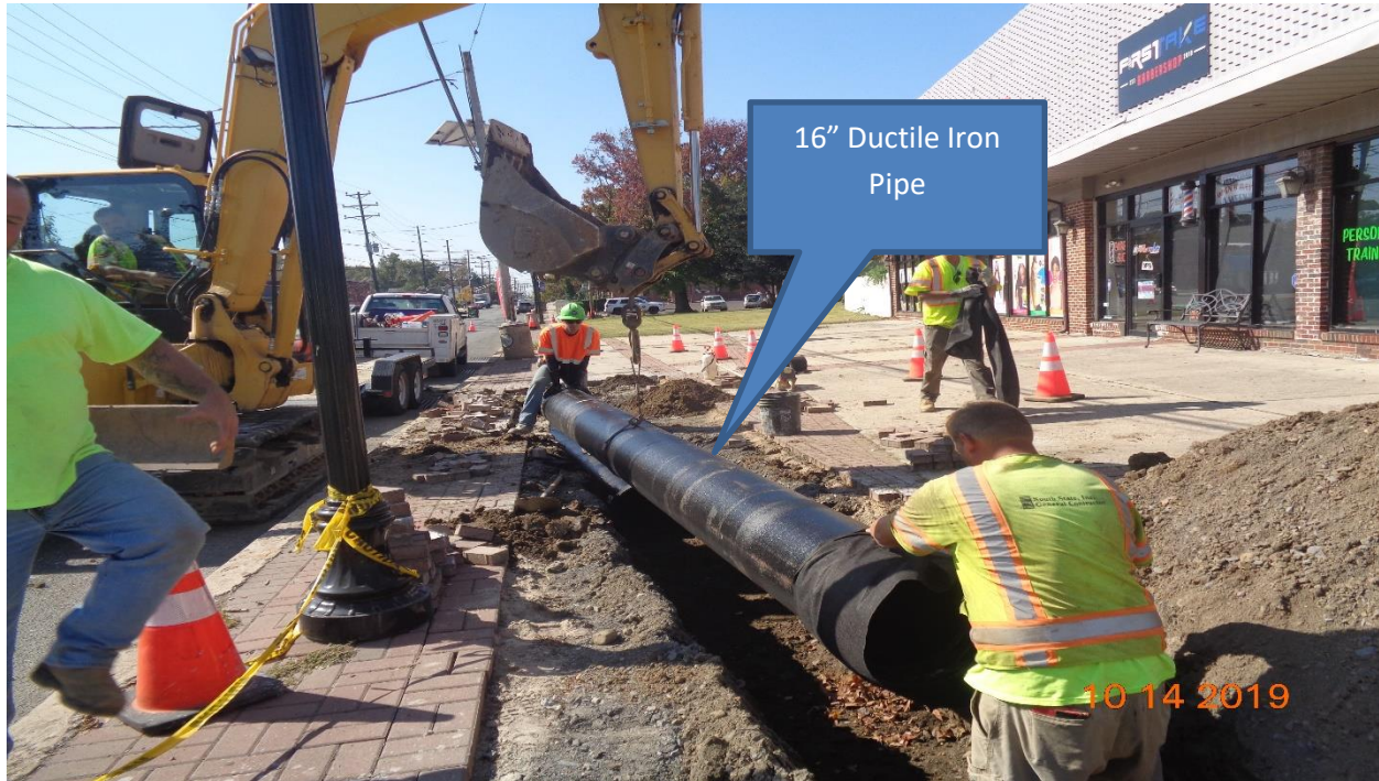
Figure 1: Installation of 16" Ductile Iron Pipe from Inlet on Hillcrest Avenue to Inlet along Westfield Avenue, LT
