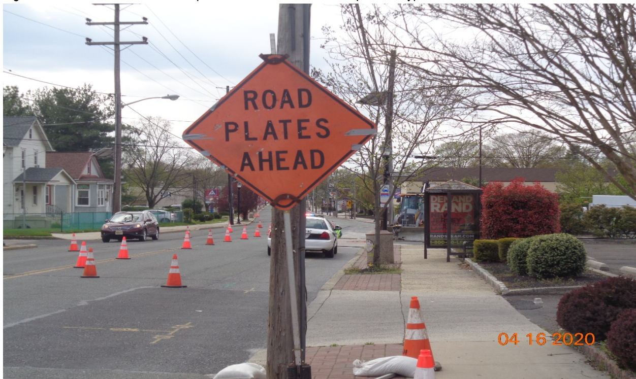
Figure 10: PSE&G Gas – Warning sign for steel plates on the road at each location in both directions for safety.
