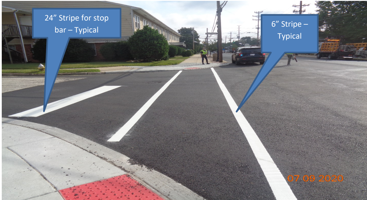
Figure 11: Thermoplastic striping along side streets from Lexington Avenue to Sherman Avenue, RT, and LT
