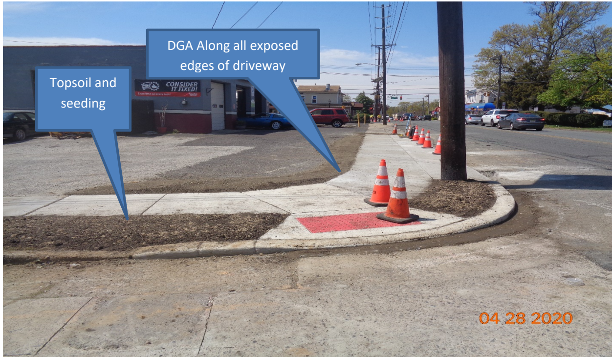
Figure 9: Topsoil and seeding along West sidewalk at Marlon Avenue, RT, And DGA along edges of driveway
