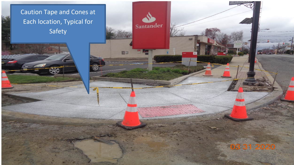
Figure 3: West Concrete curb, sidewalk and HC Ramp at Gross Avenue along Westfield Avenue, RT.
