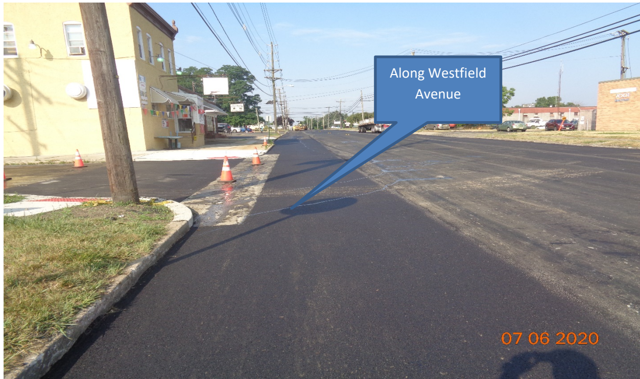
Figure 1: Hot Mix Asphalt 9.5 M surface Course was placed along Westfield Avenue from Sherman Avenue STA 109+50 – Tinsman Avenue 64+00
