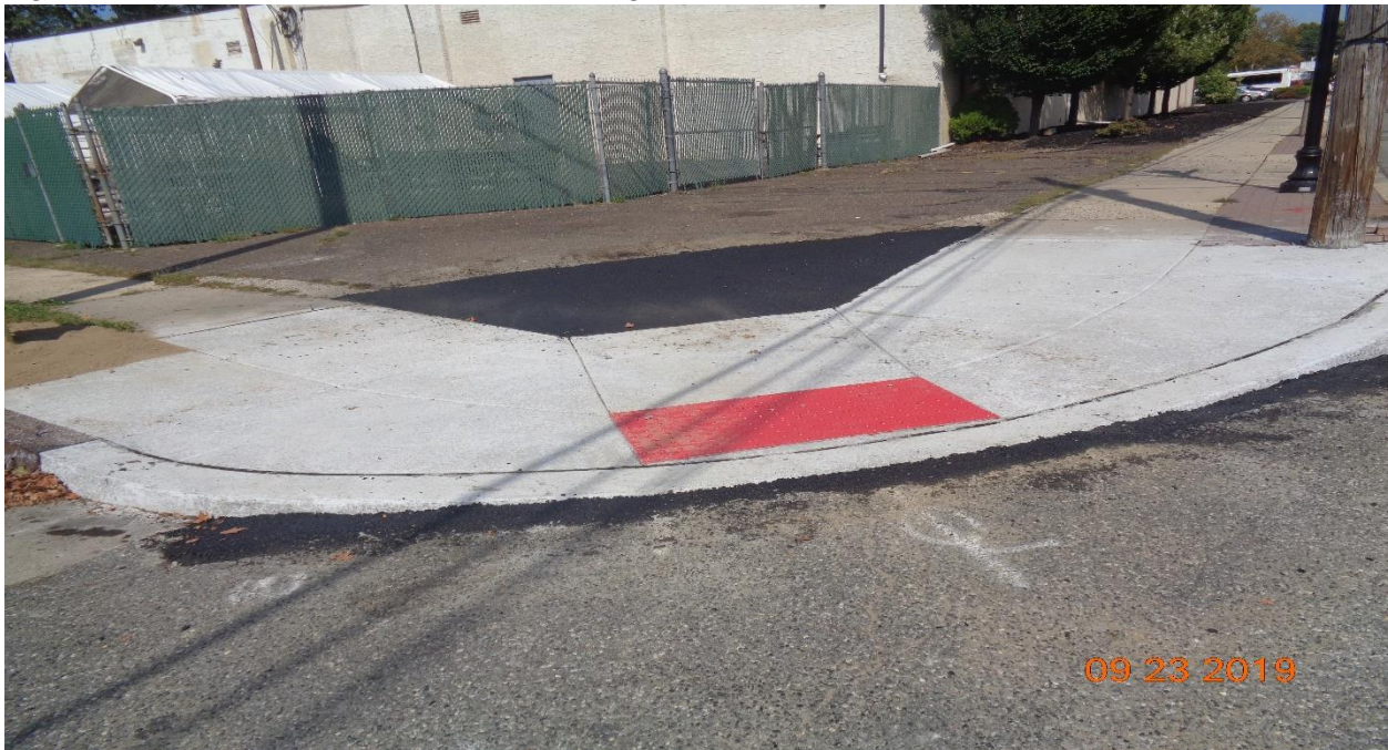
Figure 9: Asphalt around Sidewalk along Horner Avenue, East
