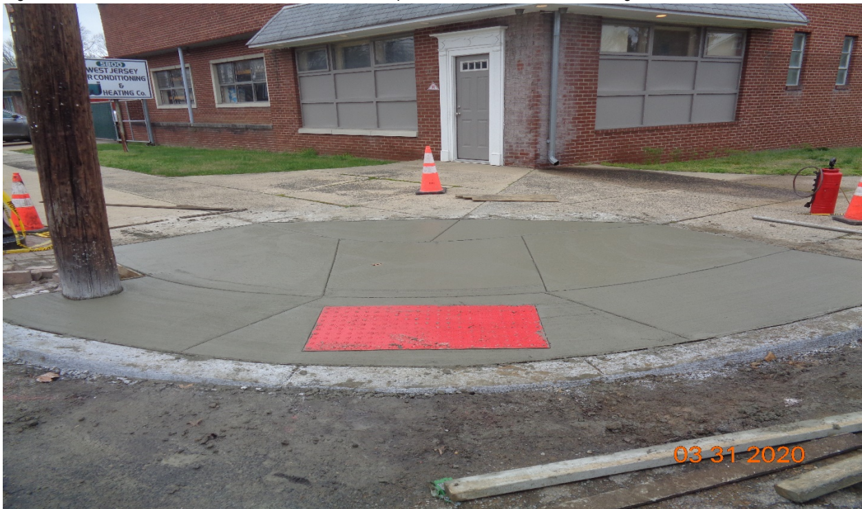
Figure 2: East Concrete curb, sidewalk and HC Ramp at Gross Avenue along Westfield Avenue, RT.
