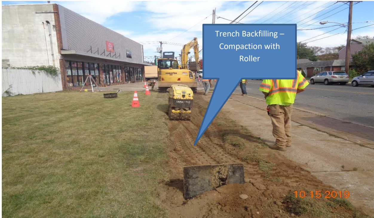
Figure 5: Installation of 16" DIP Along Westfield Avenue from Proposed Manhole to Proposed Manhole at Hollinshead Avenue.
