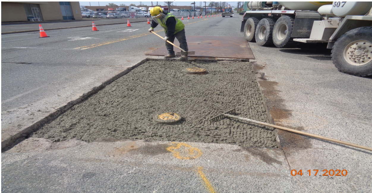
Figure: 8 - PSE&G Gas – NJDOT Class V Concrete placed – Typical at all locations.
