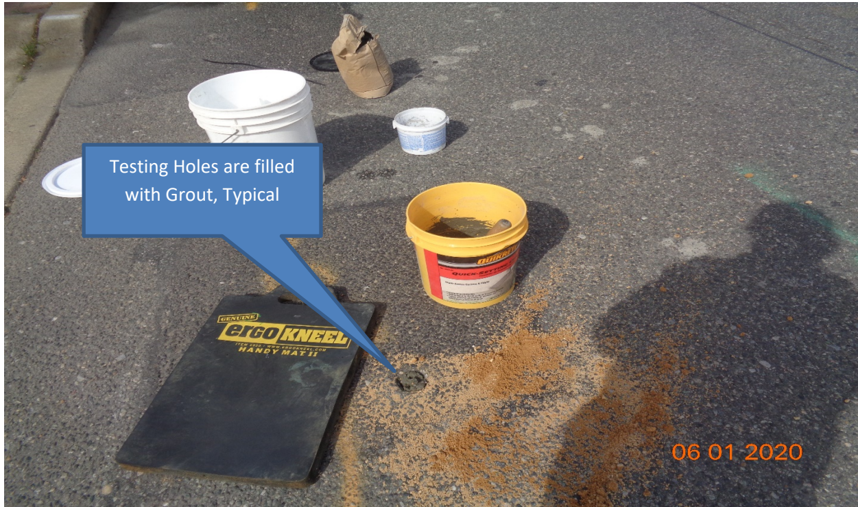
Figure 1: Gas Leak testing holes were filled with grout along Westfield Avenue at Merchantville Avenue.
