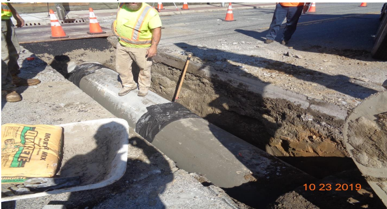
Figure 8: 24" Reinforced Concrete Pipe, Class IV was installed across Westfield Avenue at Hillcrest Avenue.
