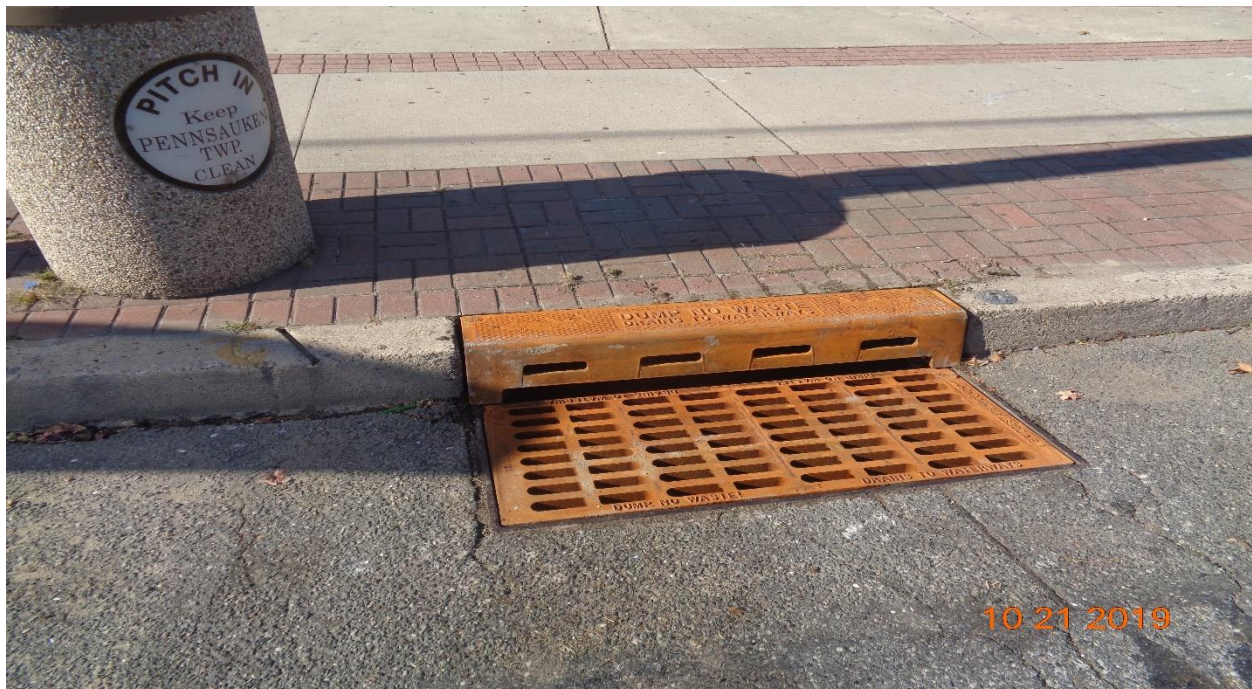
Figure 2: Curb piece, Type N ECO were installed for three inlets along Westfield Avenue, LT between Hillcrest Avenue and Hollinshead Avenue.
