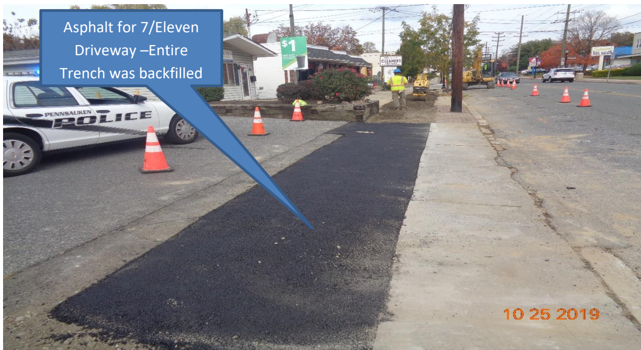
Figure 11: 18" Reinforced Concrete Pipe was installed along Westfield Avenue, LT Between Hillcrest Avenue and Horner Avenue
