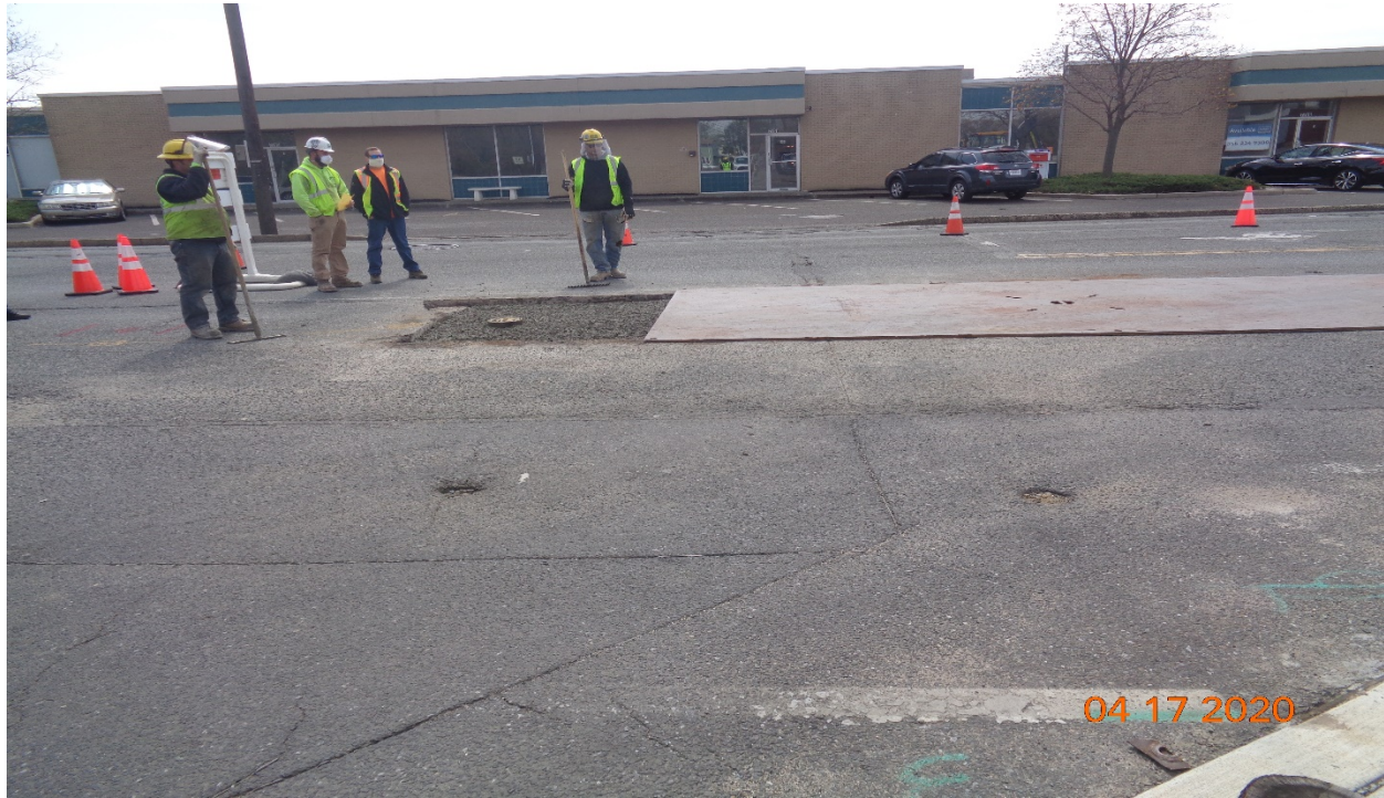
Figure 9 - PSE&G Gas – Concrete patch was covered with steel plate. – Typical at all locations.
