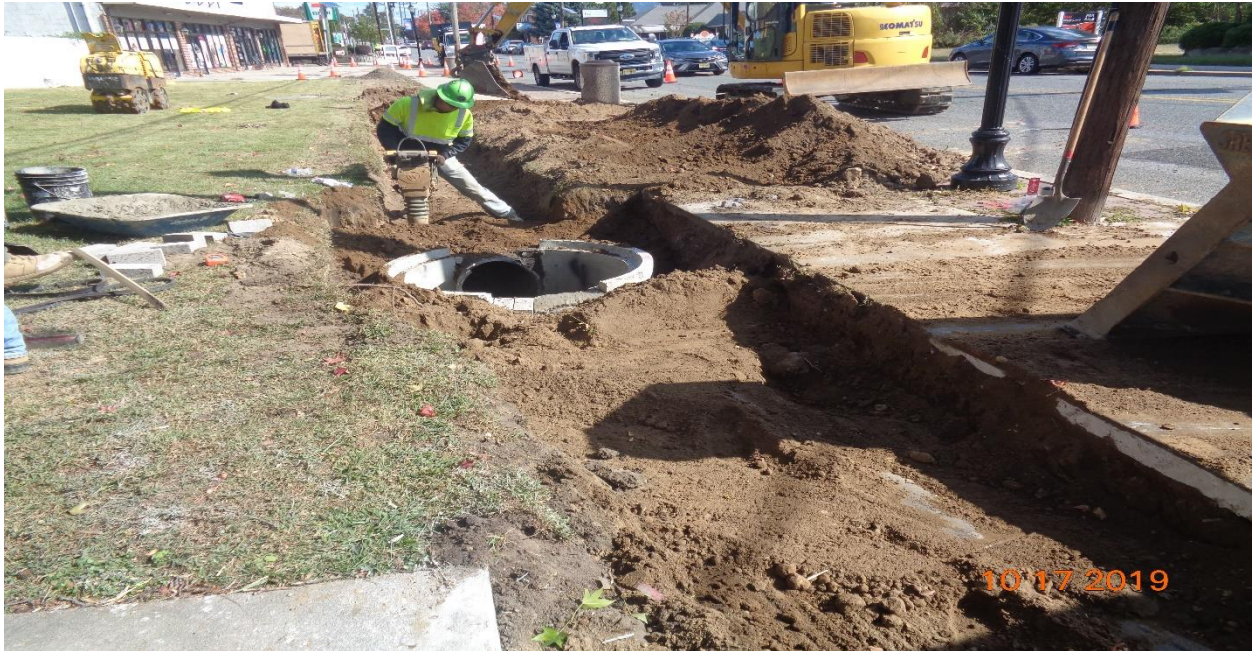
Figure 7: Installation of 16" DIP from Proposed Manhole at Hollingshead Avenue to Inlet Along Hollinshead Avenue
