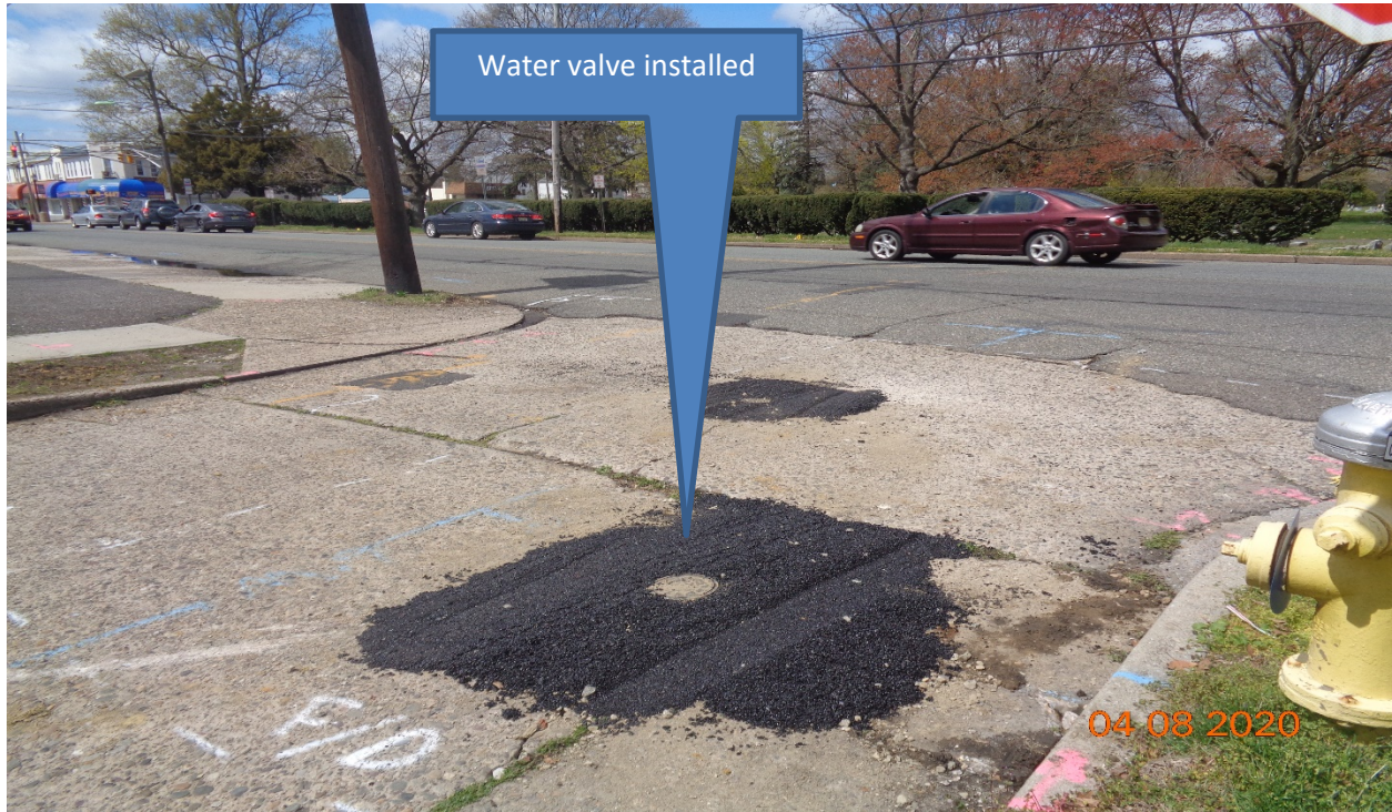
Figure7: MPWC – Water valve installed along Marlon Avenue, RT
