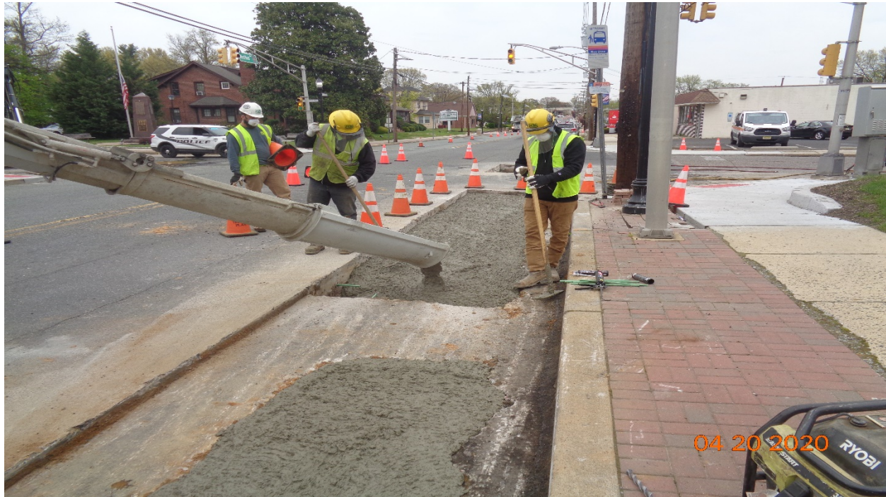
Figure 15: PSE&G Gas – NJDOT Class V Concrete placement with dowels, Typical at each location.
