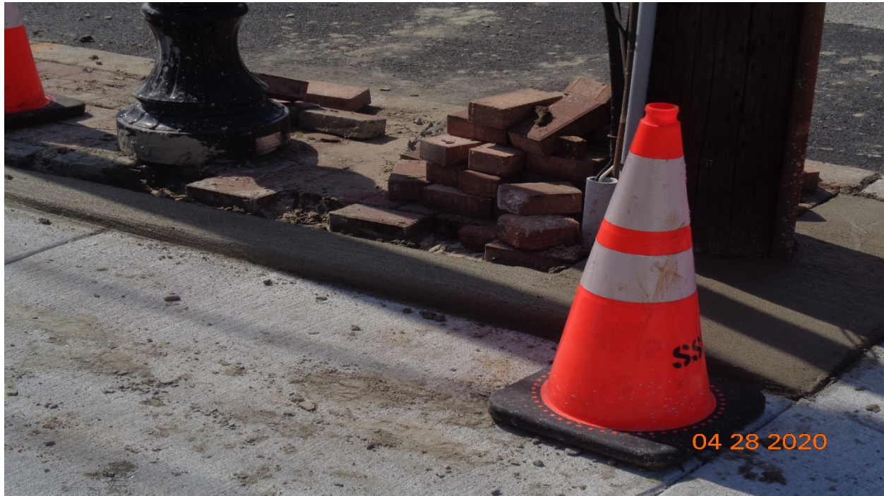
Figure 7: Hader Curb along Horner Avenue East, RT
