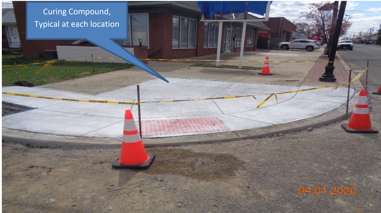
Figure 5: West Concrete curb, sidewalk and HC Ramp at Hollinshead Avenue along Westfield Avenue, RT.
