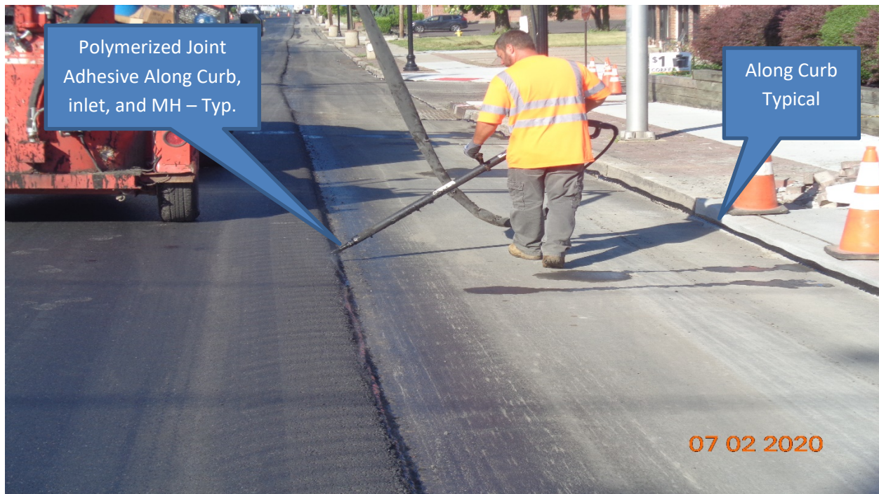
Figure 14: Hot Mix Asphalt 9.5 M surface Course was placed along Westfield Avenue from Sherman Avenue STA 109+50 – Tinsman Avenue 64+00
