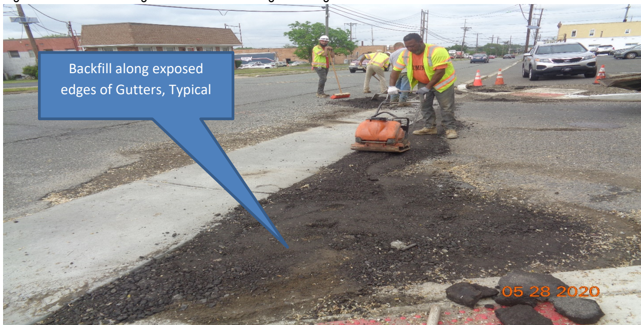
Figure 2: Exposed edges of concrete gutters were filled with DGA Along Westfield Avenue, RT, at Sherman Avenue, Bethel Avenue, and Clement Avenue, Typical
