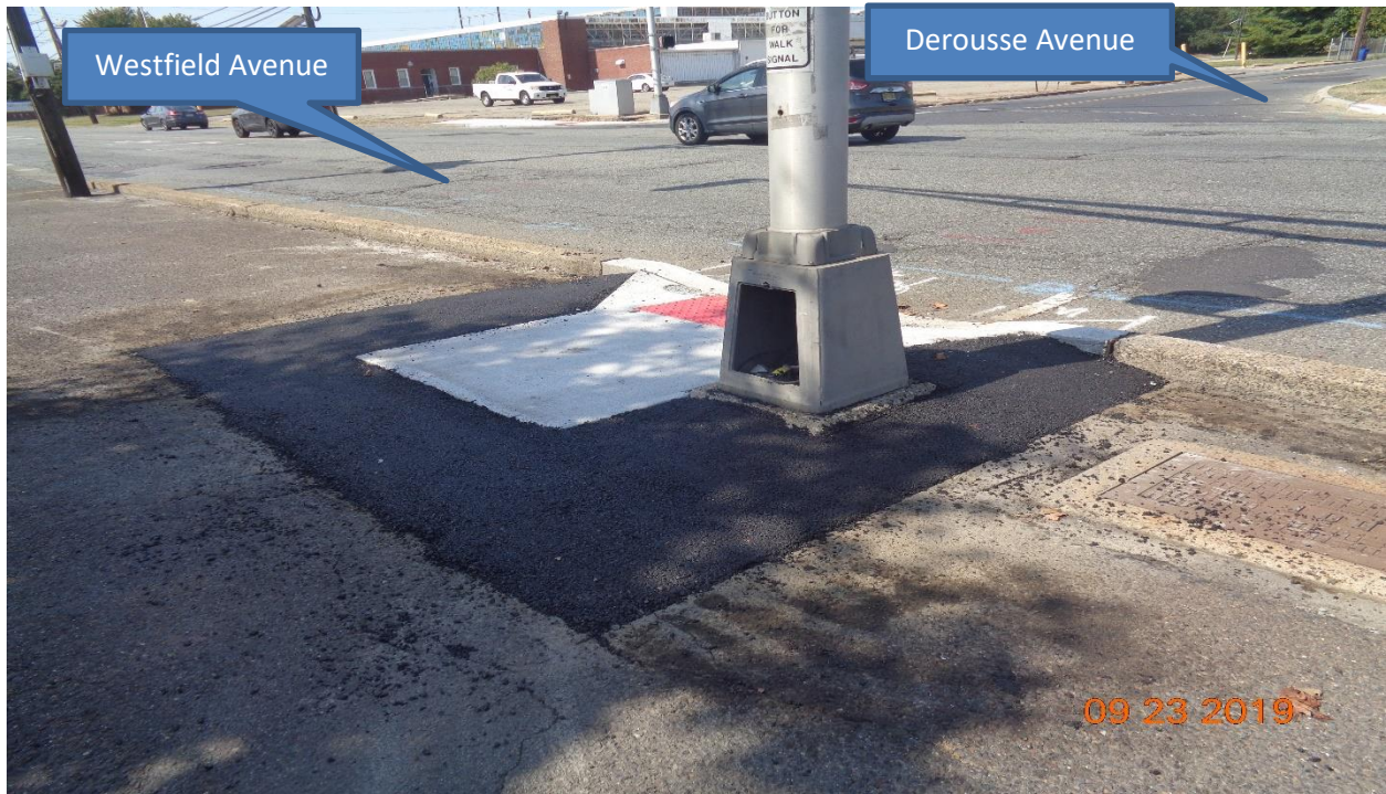
Figure 3: Asphalt at Sidewalk along Westfield Avenue, RT STA 124+75
