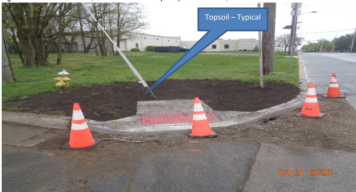
Figure 12: Topsoil placement at West concrete sidewalk and HC Ramp at Bethel Avenue – Typical for all locations
