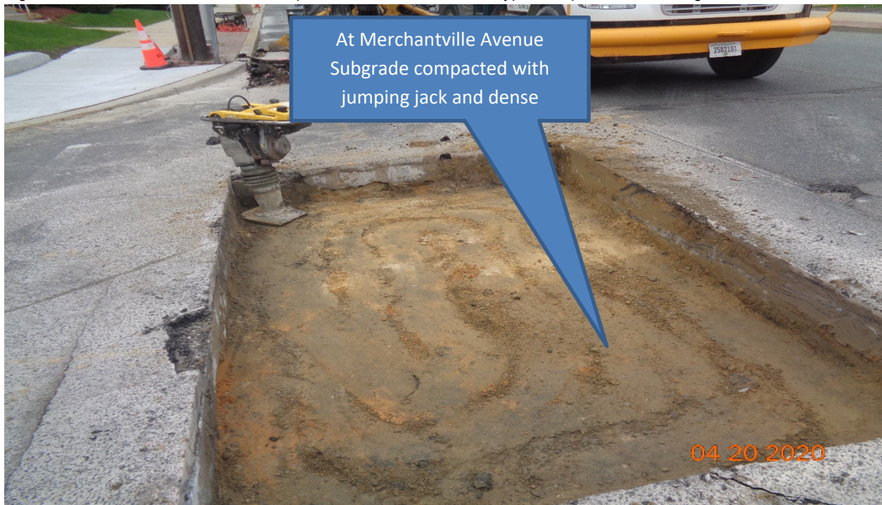
Figure 14: PSE&G Gas – Permanent Concrete pavement Patch – Subgrade Preparation – Typical at all locations.
