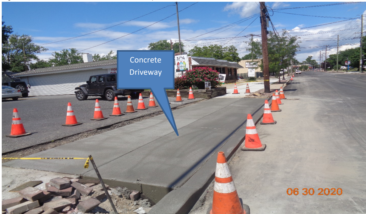
Figure 2: Concrete driveway at Seven Eleven Store, LT
