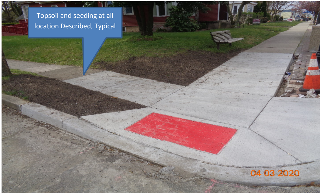
Figure 10: Topsoil and seeding were performed along all constructed sidewalks along Westfield Avenue, RT Between Lexington Avenue to Hillcrest Avenue.
