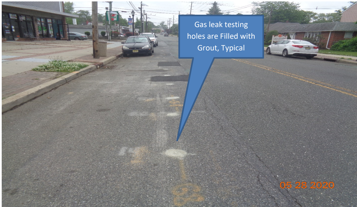
Figure 1: Gas Leak testing holes were filled with grout along Westfield Avenue at Hillcrest Avenue.
