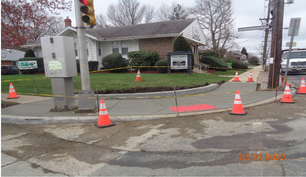
Figure 1: West Concrete curb, sidewalk and HC Ramp at Merchantville Avenue along Westfield Avenue, RT
