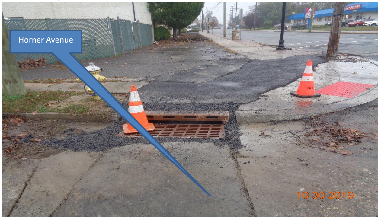
Figure 8: Existing three (3) Type B inlets along Horner Avenue East and West were Reconstructed using new casting, And Curb piece, Type N ECO was installed.
