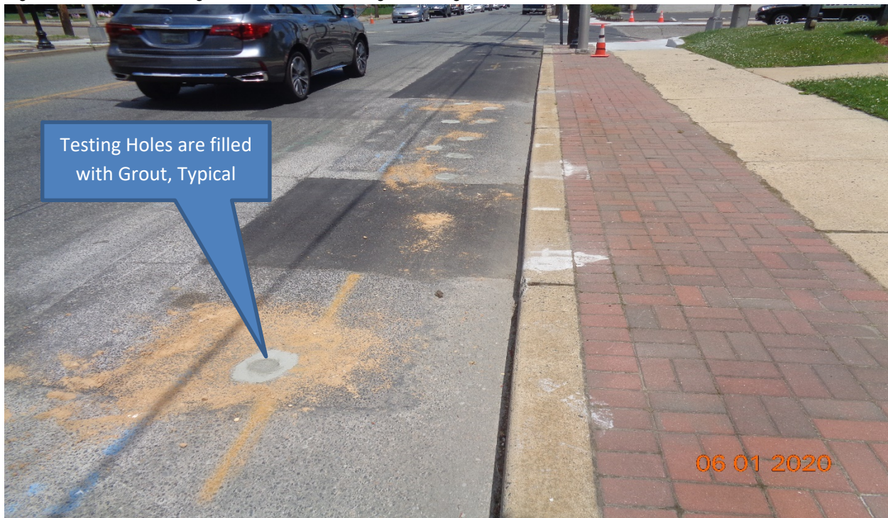
Figure 2: Gas Leak testing holes were filled with grout along Westfield Avenue at Merchantville Avenue.
