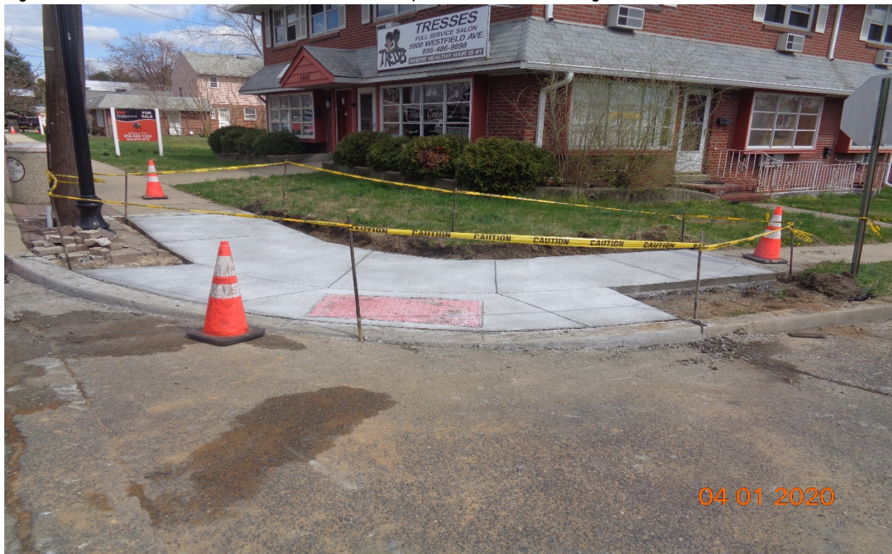
Figure 4: East Concrete curb, sidewalk and HC Ramp at Hollinshead Avenue along Westfield Avenue, RT.
