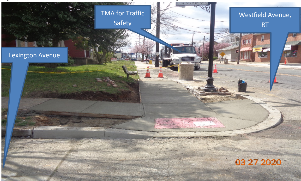
Figure 4: West concrete curb and sidewalk at Lexington Avenue along Westfield Avenue, RT
