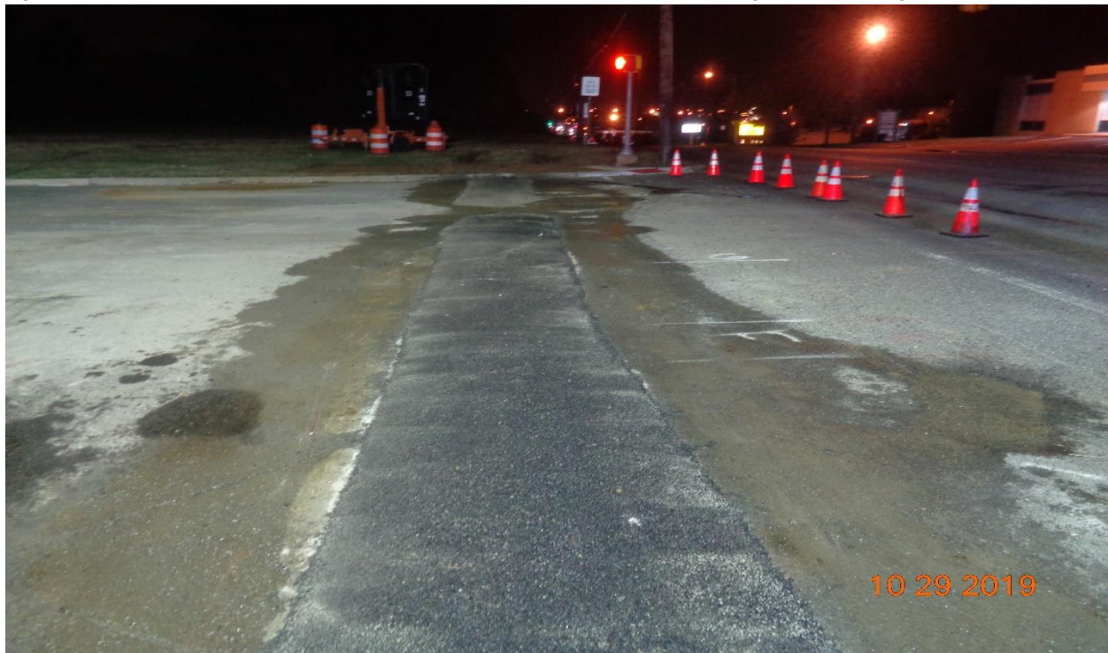
Figure 6: Installation of 12" ductile iron pipe across Derosse Avenue form existing inlet to existing manhole – Asphalt placed for Trench.
