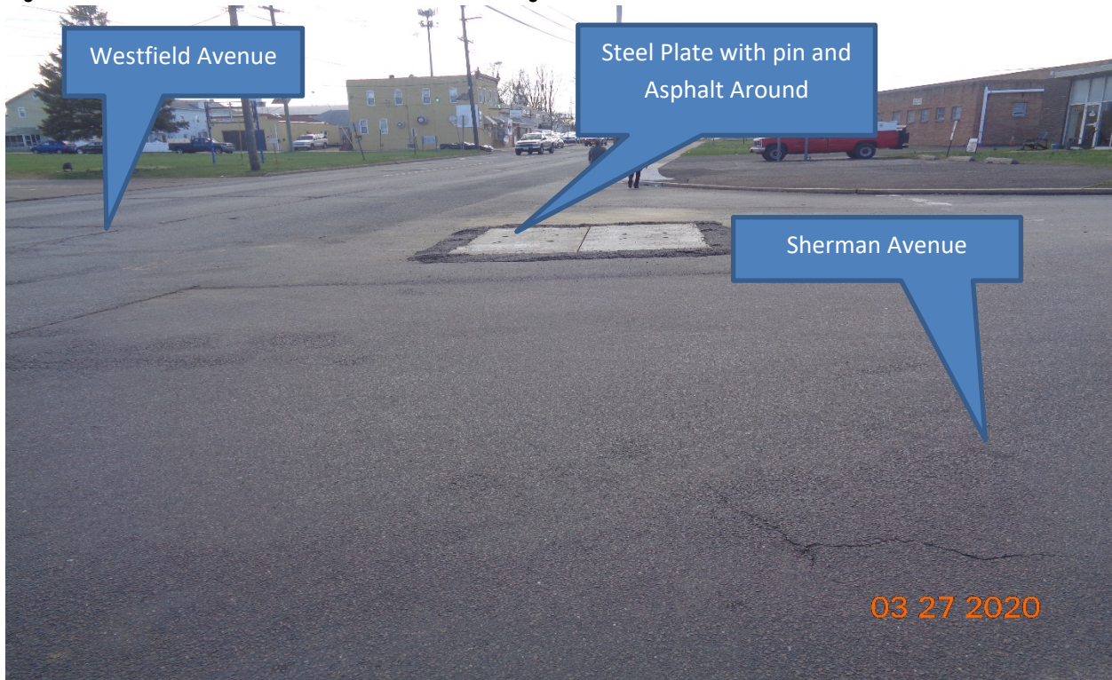
Figure 6: PSE&G Gas leak fix at Sherman Avenue along Westfield Avenue,
