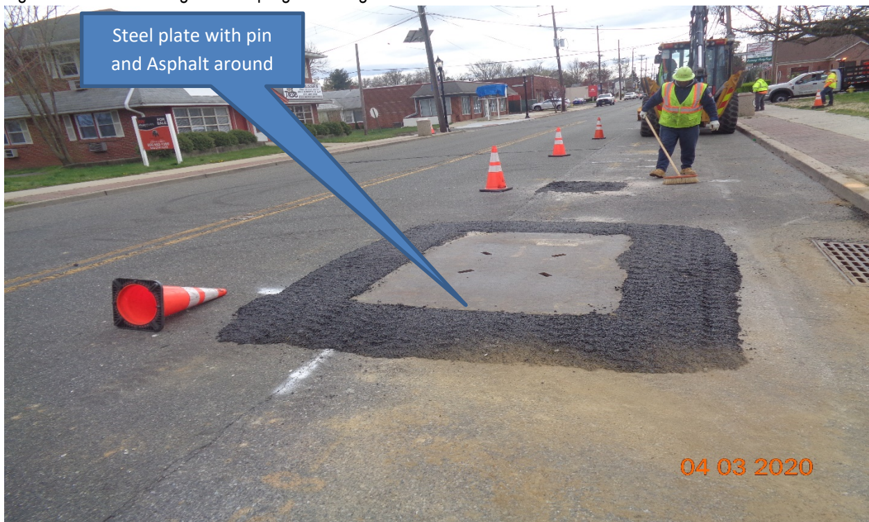
Figure 14: Gas leak detection is under progress along Westfield Avenue at Hillcrest Avenue
