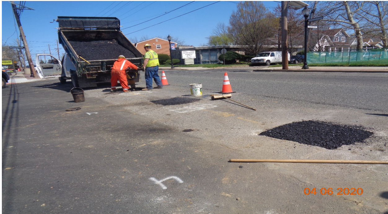
Figure 1: Asphalt placement for PSE&G Gas fixed locations along Westfield Avenue at Scovel Avenue.
