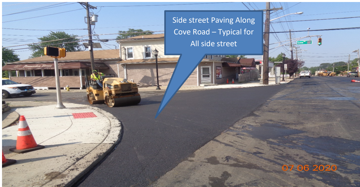
Figure 2: Hot Mix Asphalt 9.5M Surface course was place at all side street along Westfield Avenue from Lexington Avenue – Sherman Avenue, LT, and RT.
