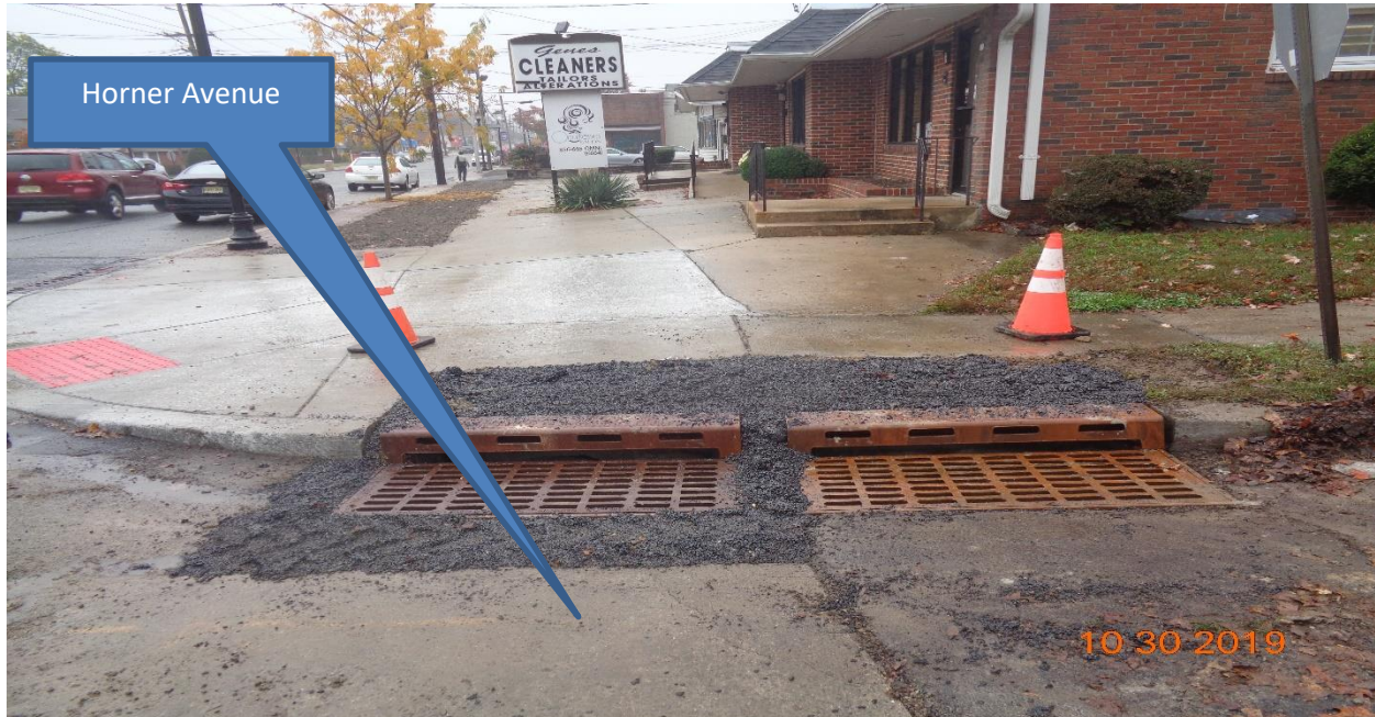
Figure 7: Existing three (3) Type B inlets along Horner Avenue East and West were Reconstructed using new casting, And Curb piece, Type N ECO was installed.
