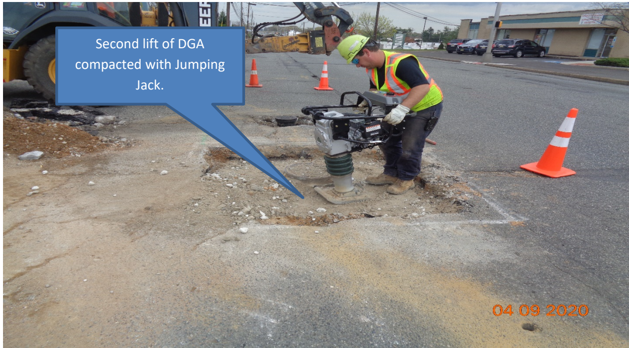
Figure 5: PSE&G Gas – Along Westfield Avenue at Derausse Avenue – DGA Placement in lifts
