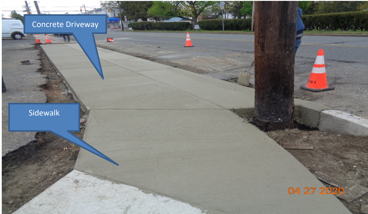
Figure 1: Concrete driveway 6" thick along Westfield Avenue STA 93+00-93+50, RT, and West sidewalk at Marlon Avenue, RT
