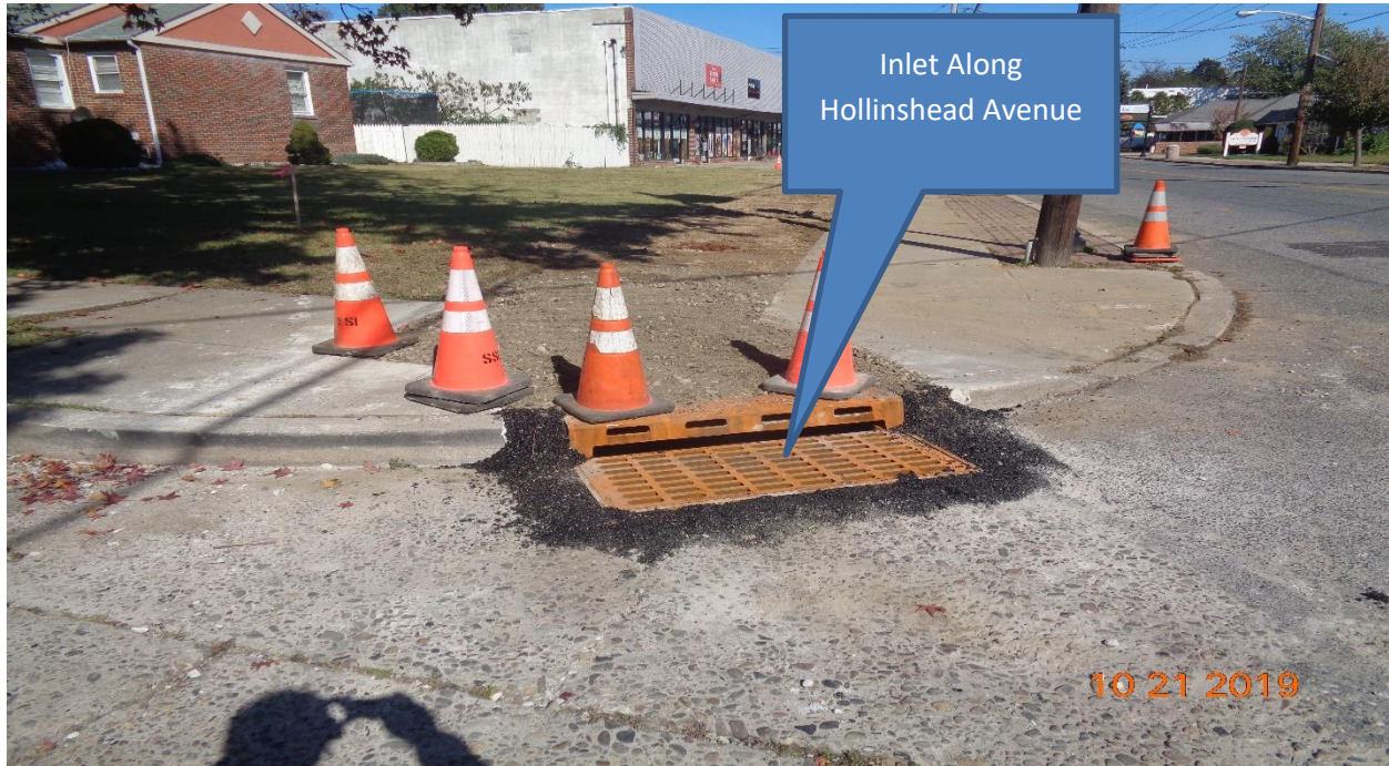
Figure 1: Existing Type B inlet along Hollinshead Avenue West was Reconstructed using new casting, And Curb piece, Type N ECO was installed.
