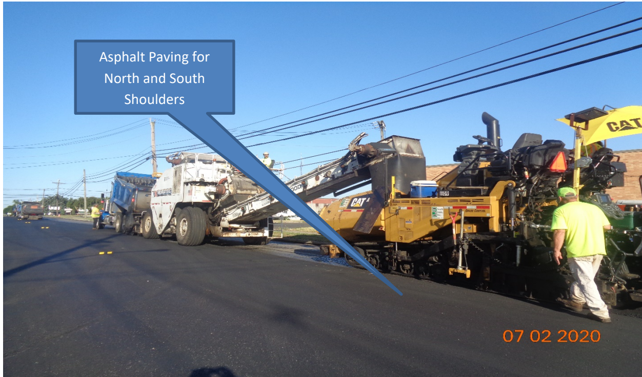
Figure 15: Hot Mix Asphalt 9.5 M surface Course was placed along Westfield Avenue from Sherman Avenue STA 109+50 – Tinsman Avenue 64+00
