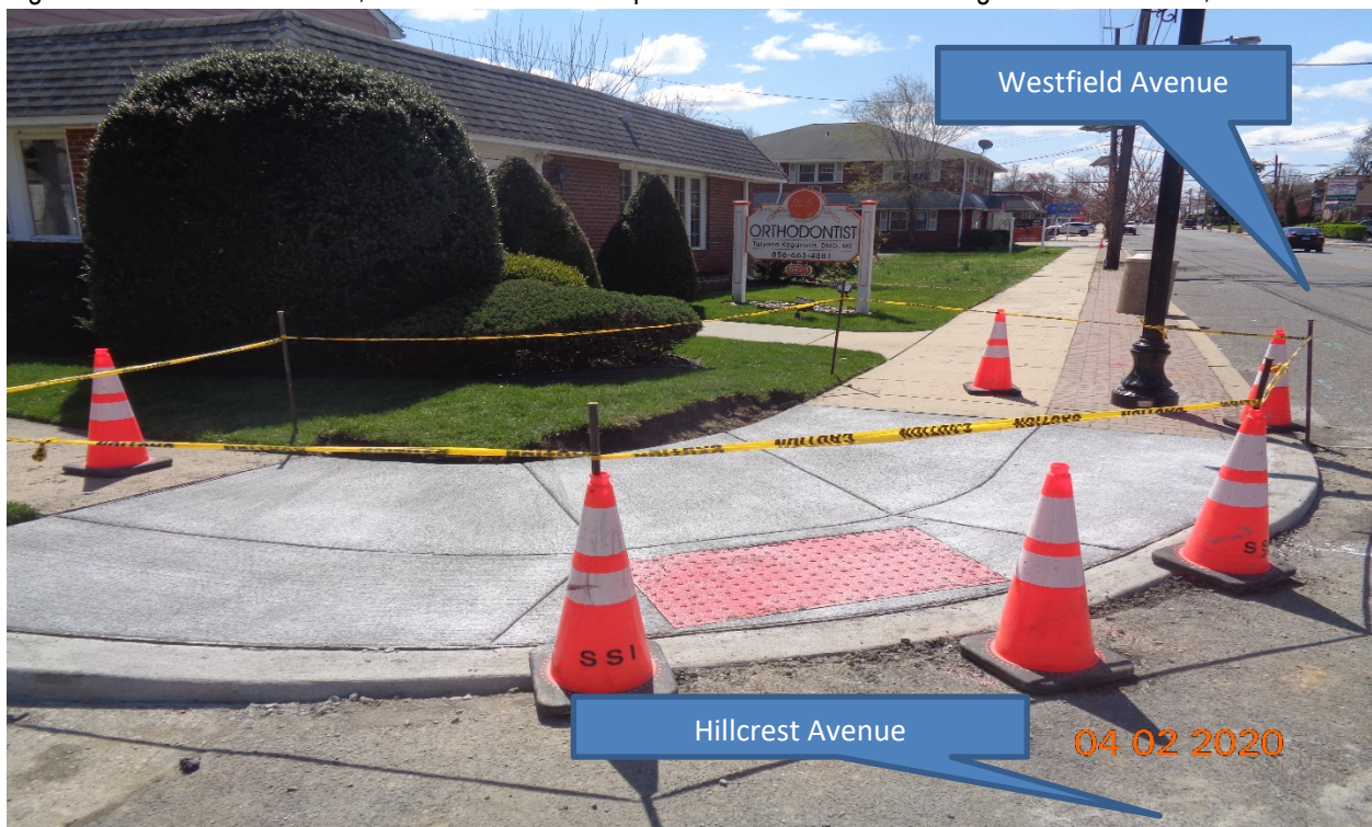
Figure 6: West Concrete curb, sidewalk and HC Ramp at Hillcrest Avenue along Westfield Avenue, RT.
