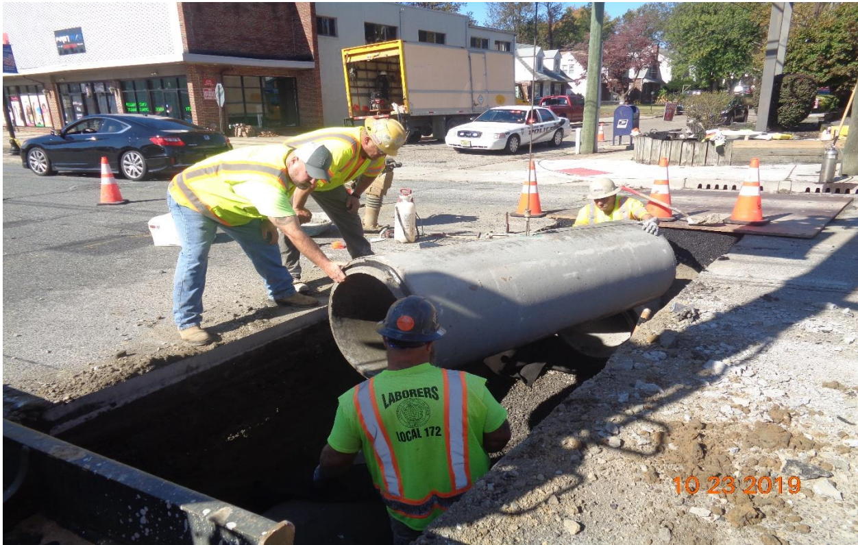
Figure 7: 24" Reinforced Concrete Pipe, Class IV was installed across Westfield Avenue at Hillcrest Avenue.
