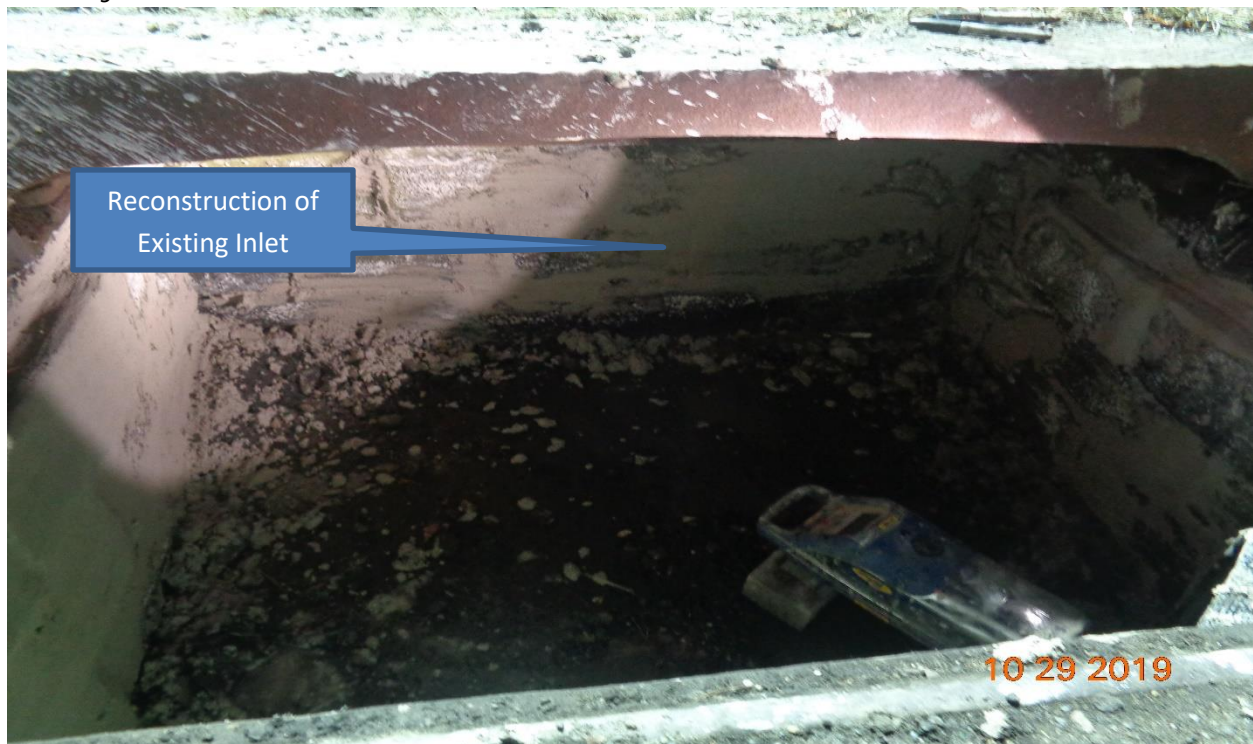
Figure 4: Installation of 12" ductile iron pipe across Derausse Avenue from existing inlet to existing manhole- Inlet reconstruction.
