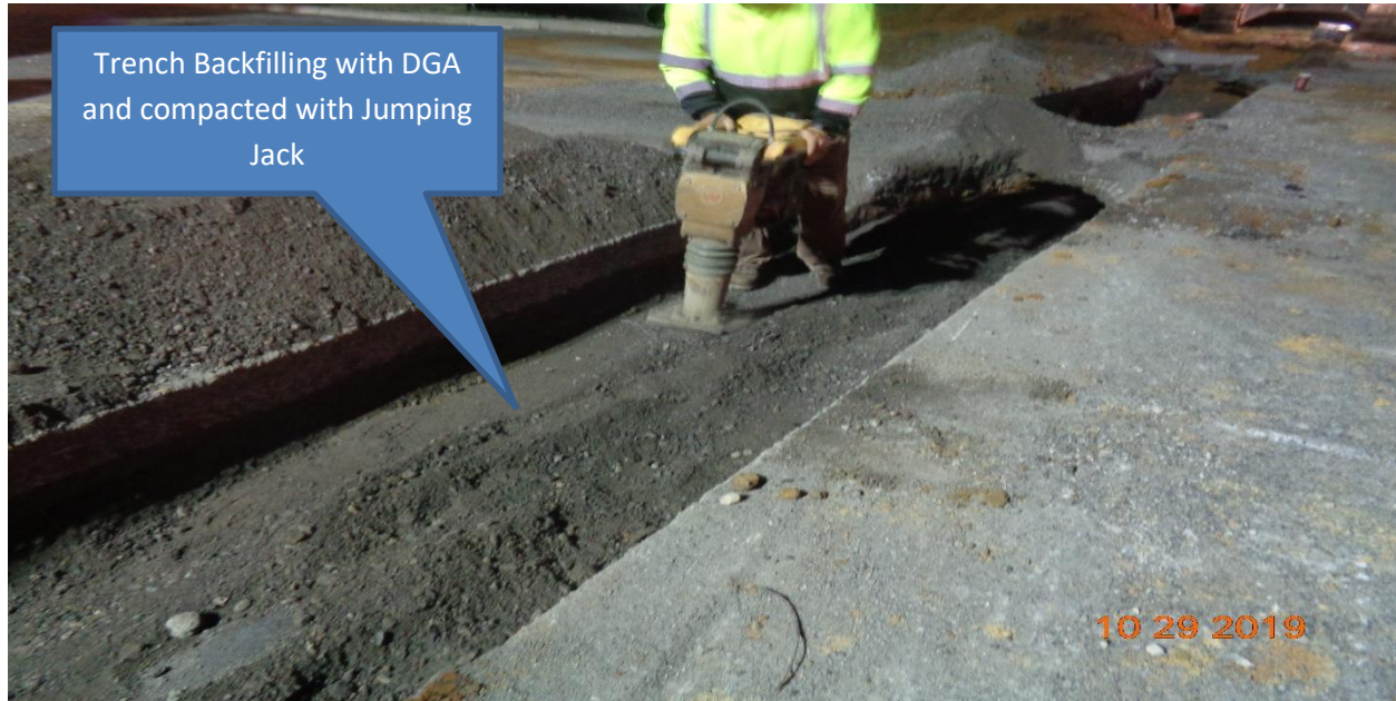
Figure 3: Installation of 12" ductile iron pipe across Derausse Avenue from existing inlet to existing manhole – Trench Backfilling.
