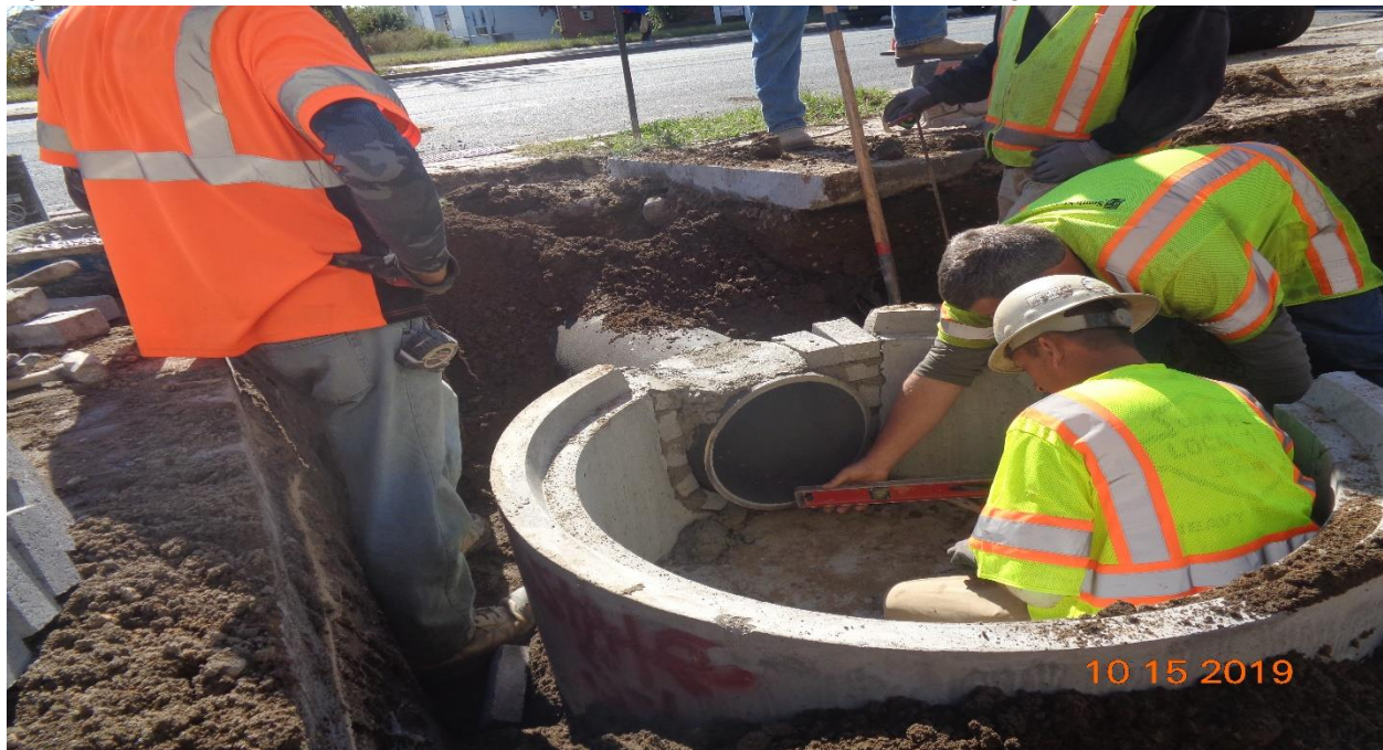
Figure 4: Installation of 16" DIP from Inlet along Westfield Avenue to Proposed 4' Diameter Manhole
