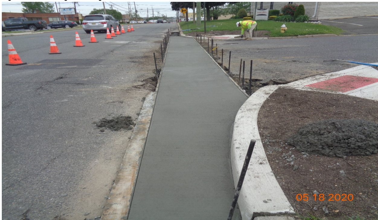
Figure 1: Concrete gutter along Westfield Avenue, RT at Clement Avenue
