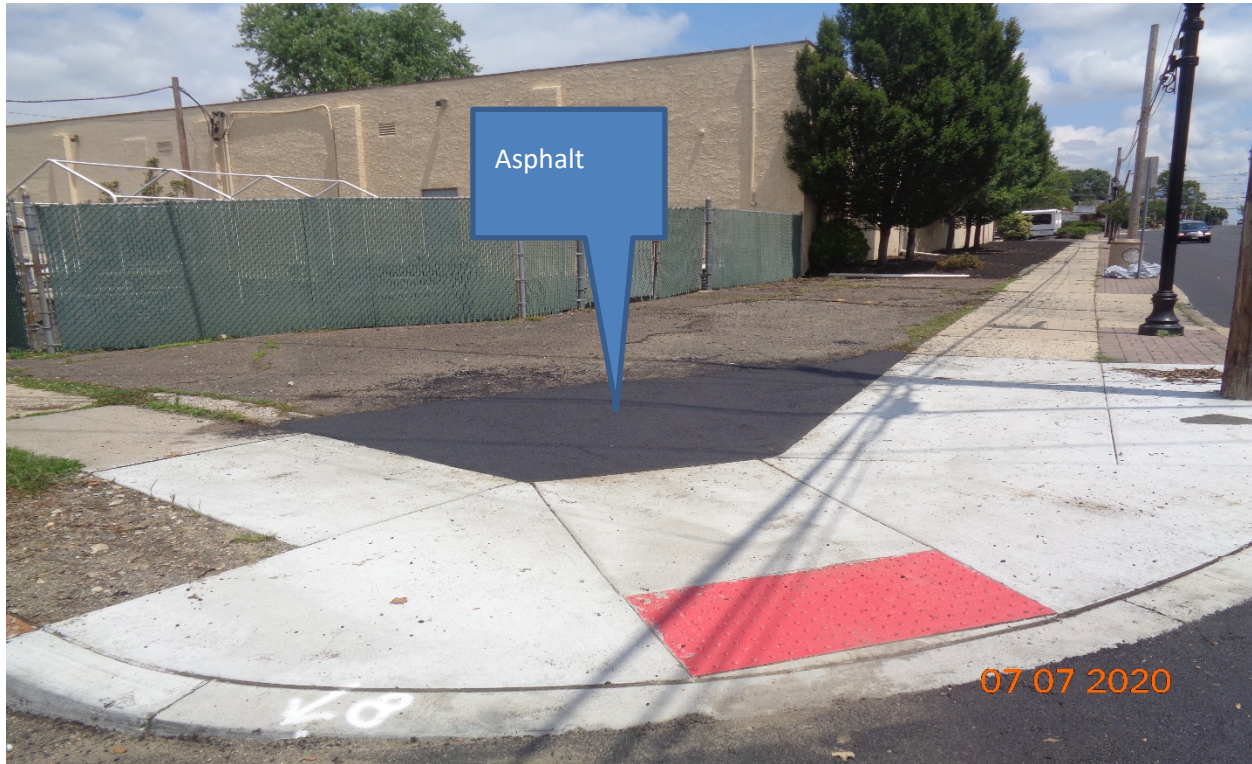
Figure 3: Horner Avenue, LT – Asphalt along sidewalk
