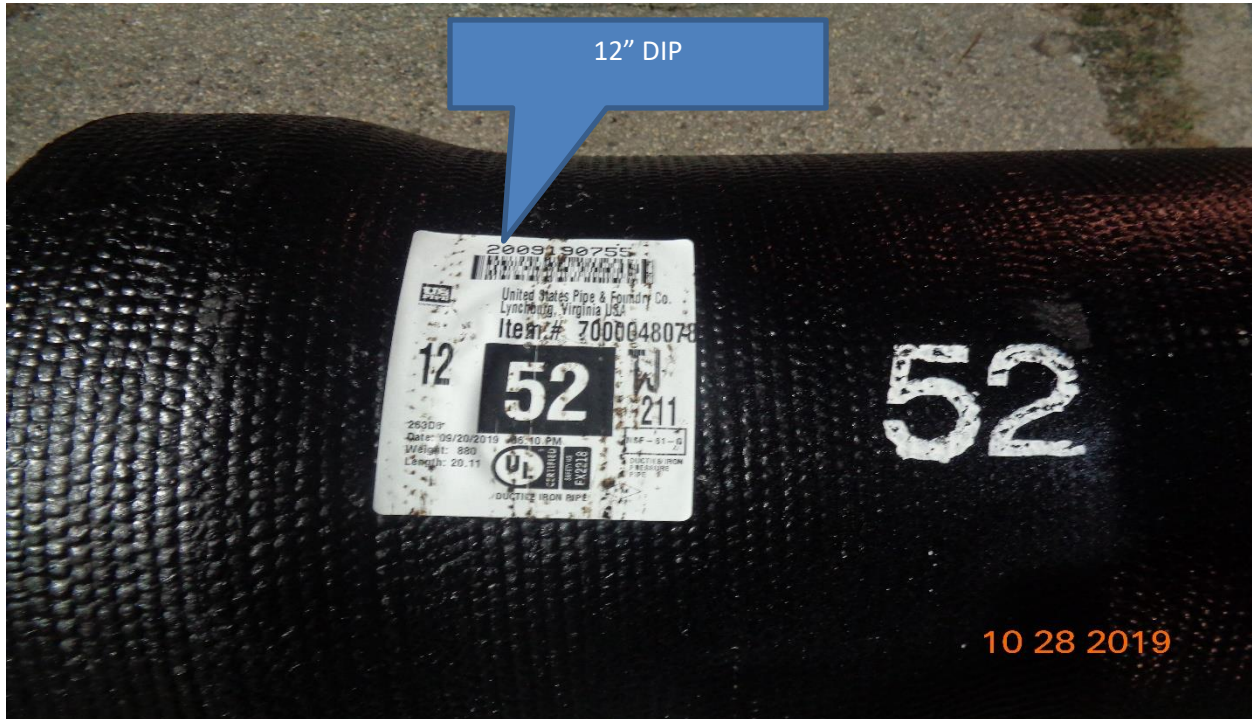
Figure 1: Installation of 12" ductile iron pipe across Derrusse Avenue from existing inlet to existing manhole.
