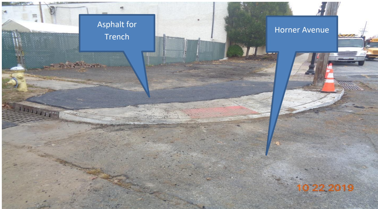
Figure 6: 15" Reinforced Concrete Pipe was installed from inlet along Westfield Avenue to East Inlet along Horner Avenue, LT.
