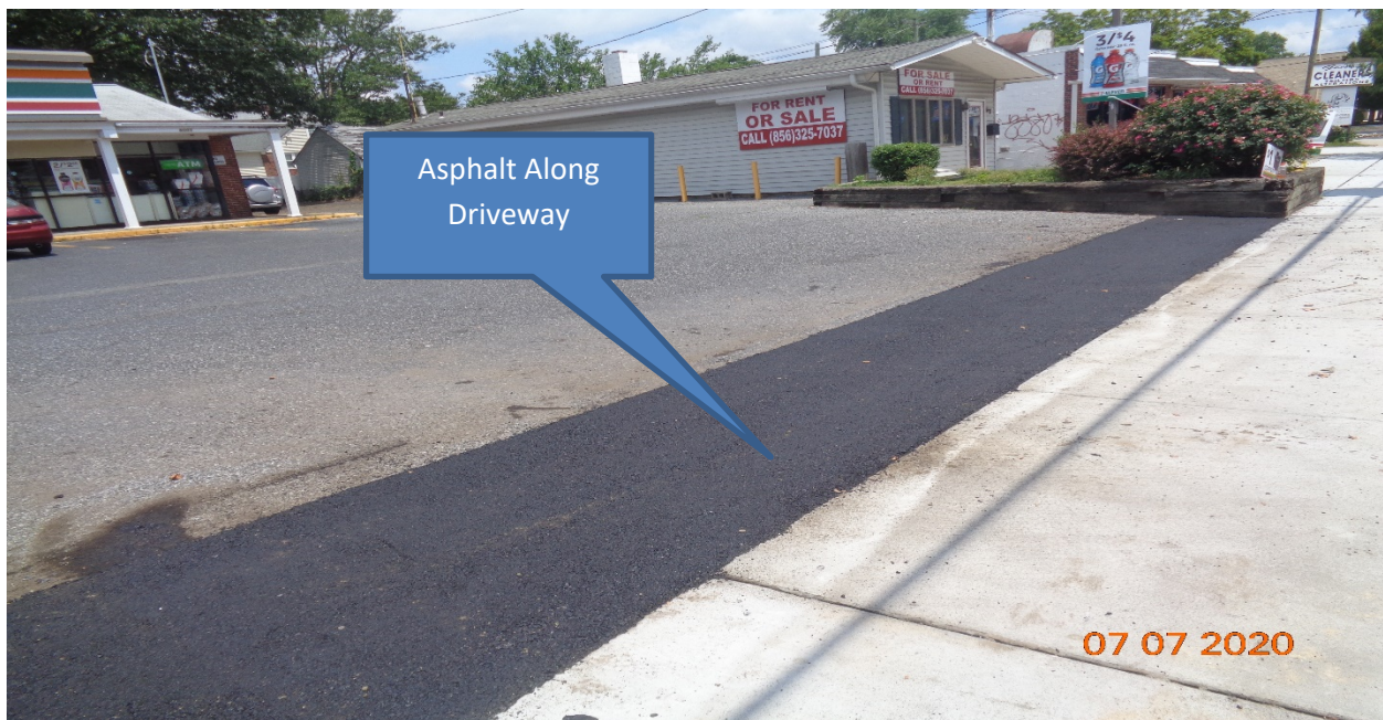
Figure 4: Concrete Driveway at Seven Eleven – Asphalt along Driveway
