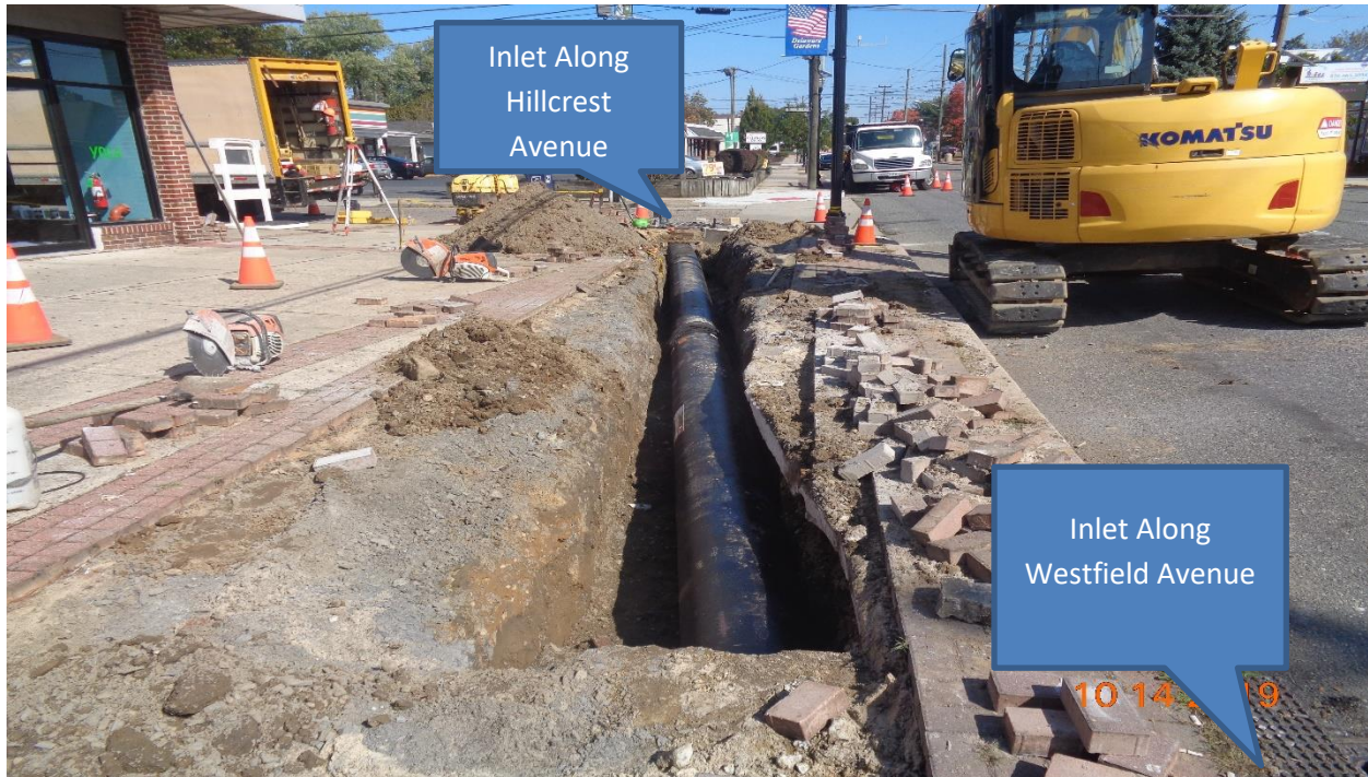
Figure 2: Installation of 16" Ductile Iron Pipe from Inlet on Hillcrest Avenue to Inlet along Westfield Avenue, LT
