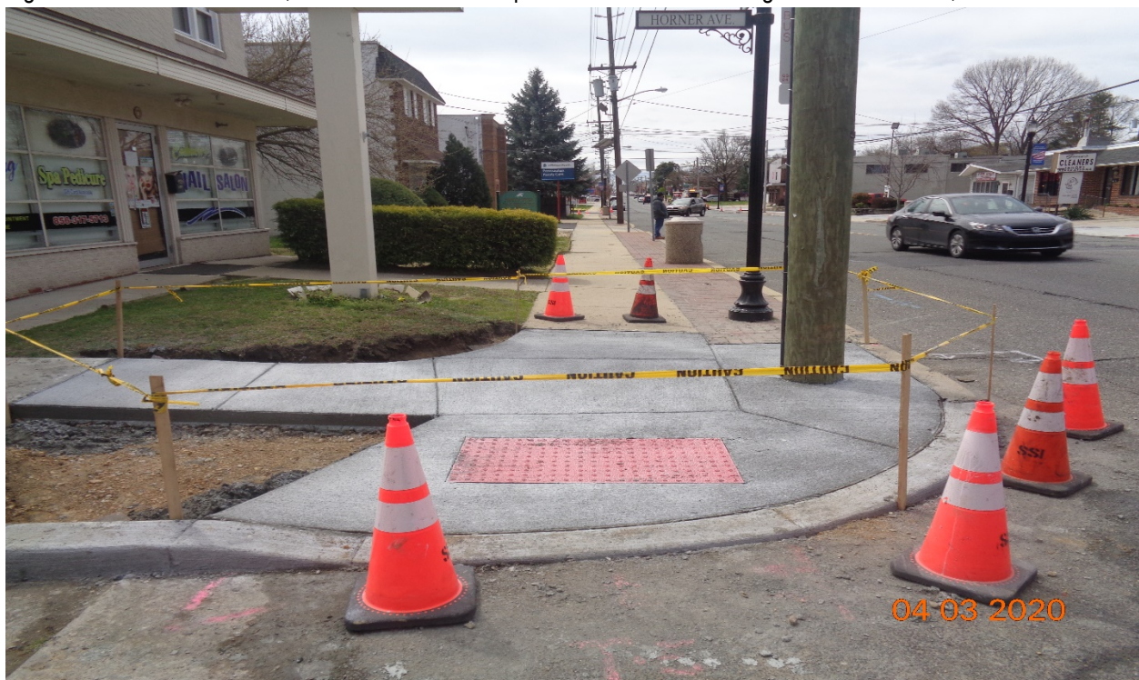
Figure 8: West Concrete curb, sidewalk and HC Ramp at Horner Avenue along Westfield Avenue, RT.
