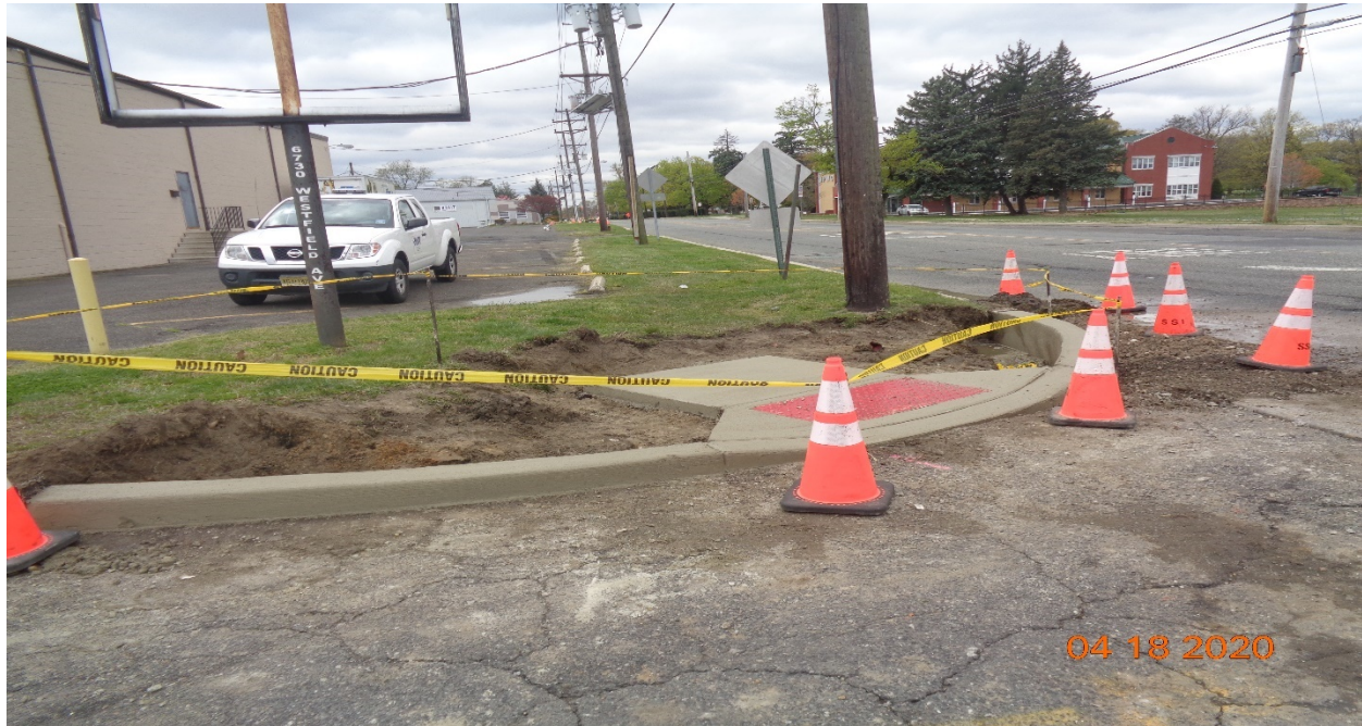
Figure 3: West concrete curb, sidewalk and HC Ramp at Clements Avenue, RT
