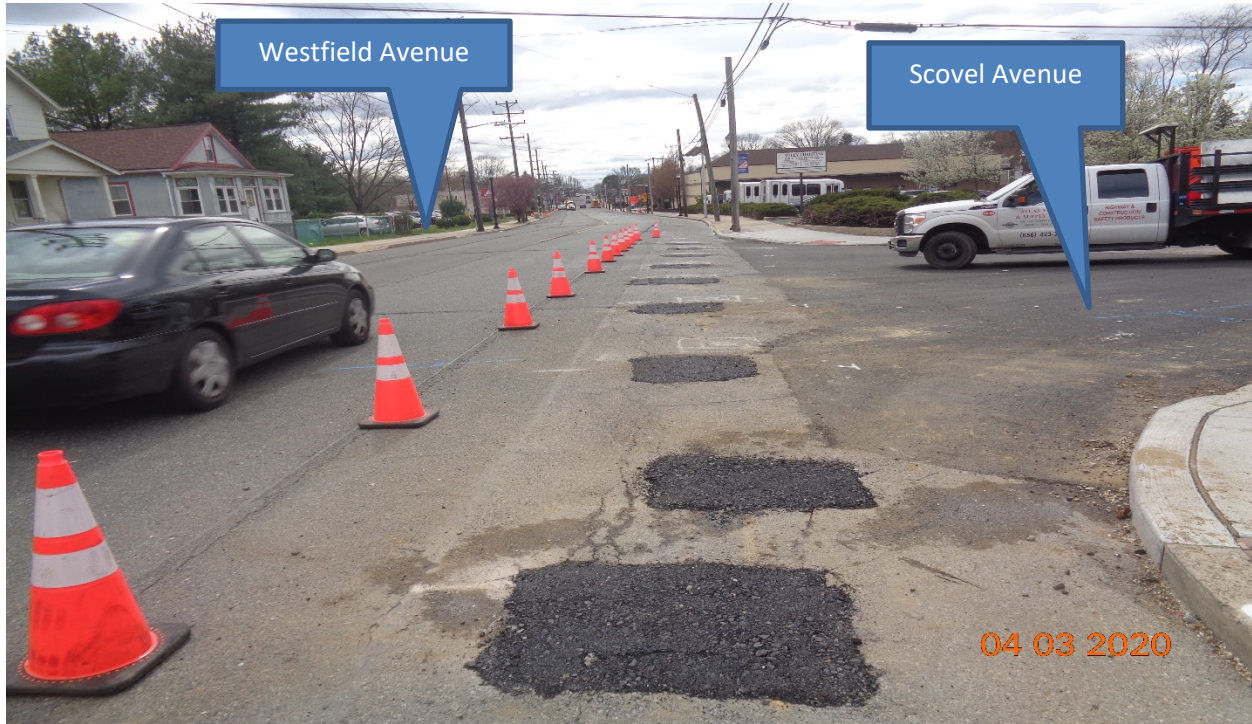
Figure13: Gas leak fixing is under progress along Westfield Avenue at Scovel Avenue
