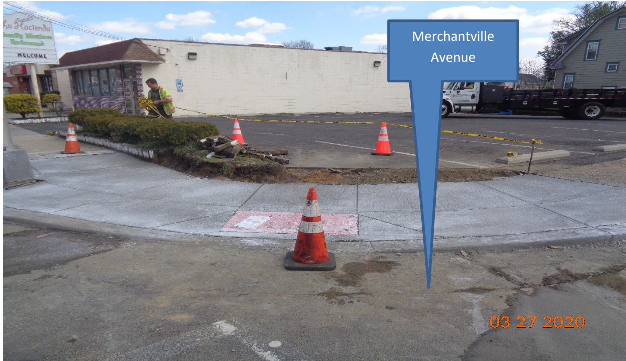
Figure 1: East concrete curb and sidewalk at Merchantville Avenue along Westfield Avenue, RT
