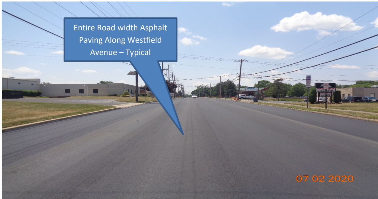
Figure 16: Hot Mix Asphalt 9.5 M surface Course was placed along Westfield Avenue from Sherman Avenue STA 109+50 – Tinsman Avenue 64+00
