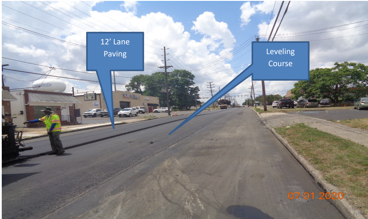
Figure 9: Hot Mix Asphalt 9.5 M surface Course was placed along Westfield Avenue from Sherman Avenue STA 109+50 – Tinsman Avenue 64+00
