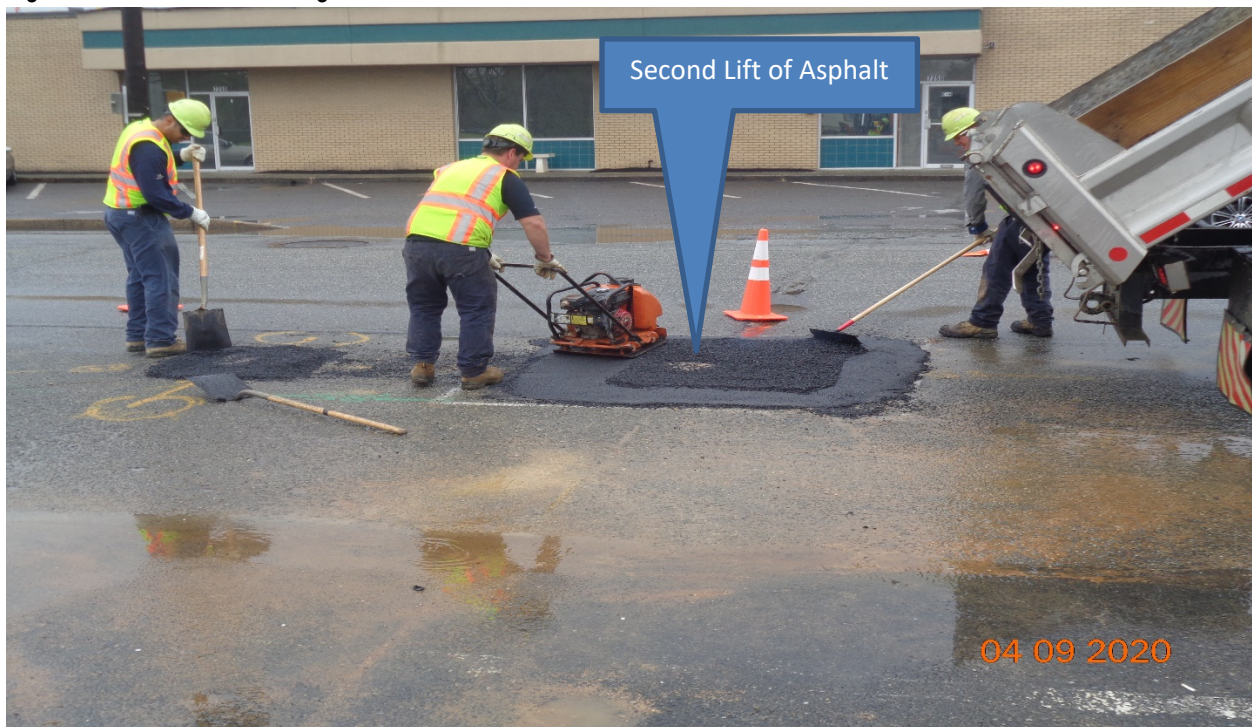
Figure6: PSE&G Gas – Along Westfield Avenue at Derausse Avenue – Asphalt Placement in lift.
