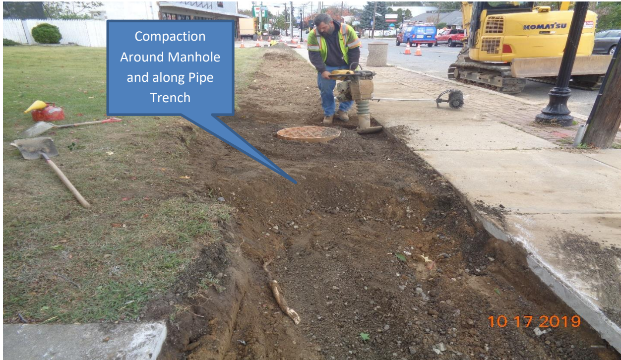
Figure 9: Installation of 16" DIP from Proposed Manhole at Hollingshead Avenue to Inlet Along Hollinshead Avenue
