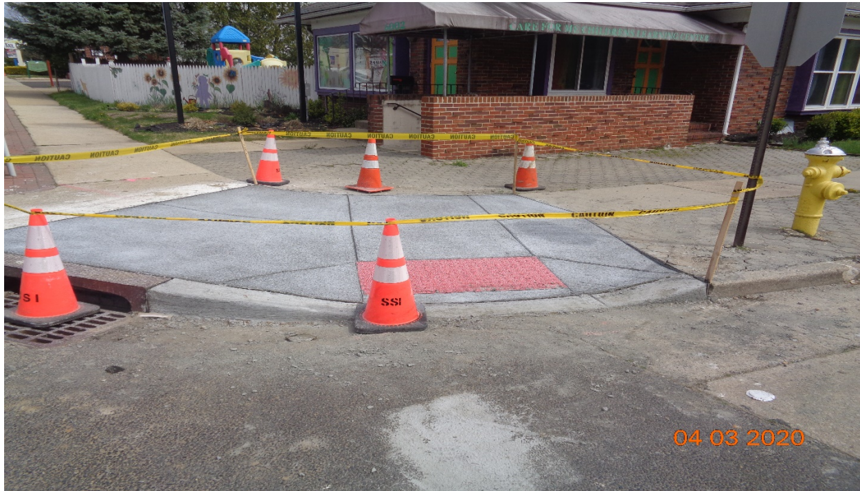
Figure 7: East Concrete curb, sidewalk and HC Ramp at Hillcrest Avenue along Westfield Avenue, RT.
