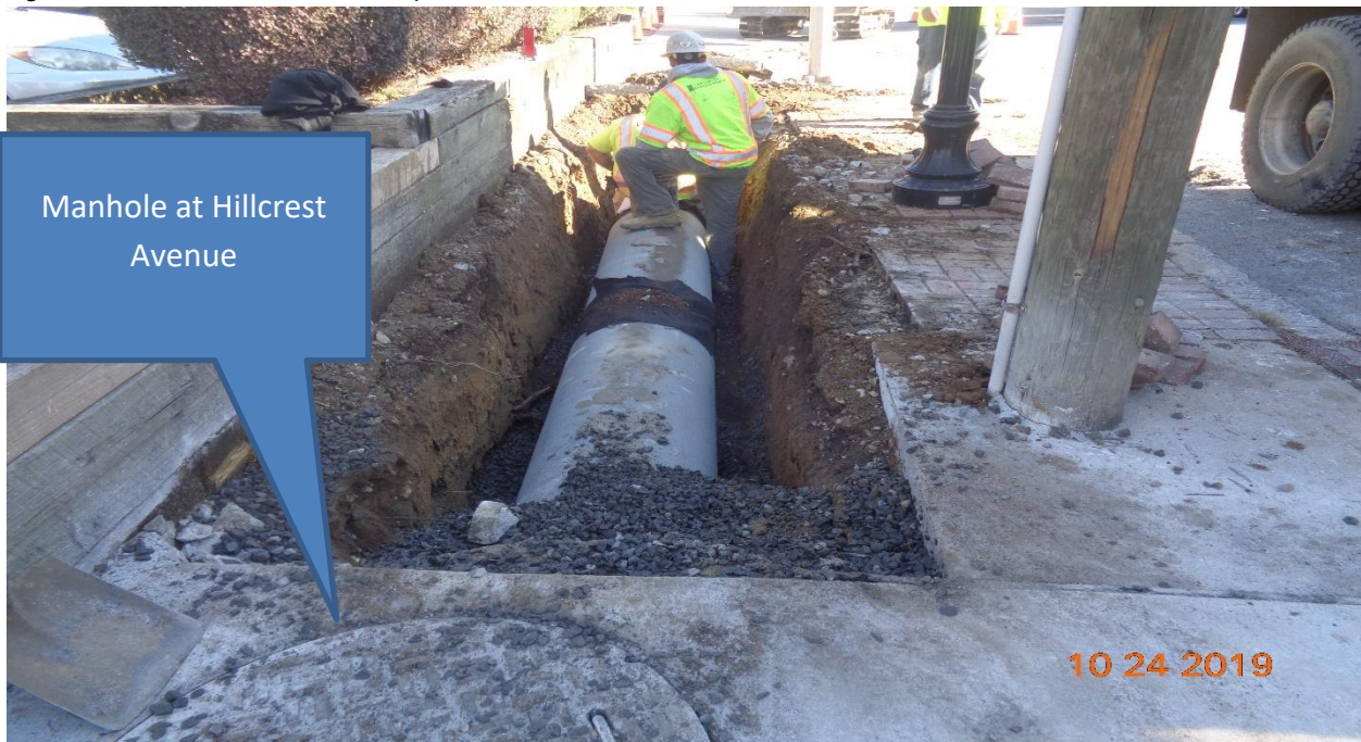
Figure 10: 18" Reinforced Concrete Pipe was installed along Westfield Avenue, LT Between Hillcrest Avenue and Horner Avenue
