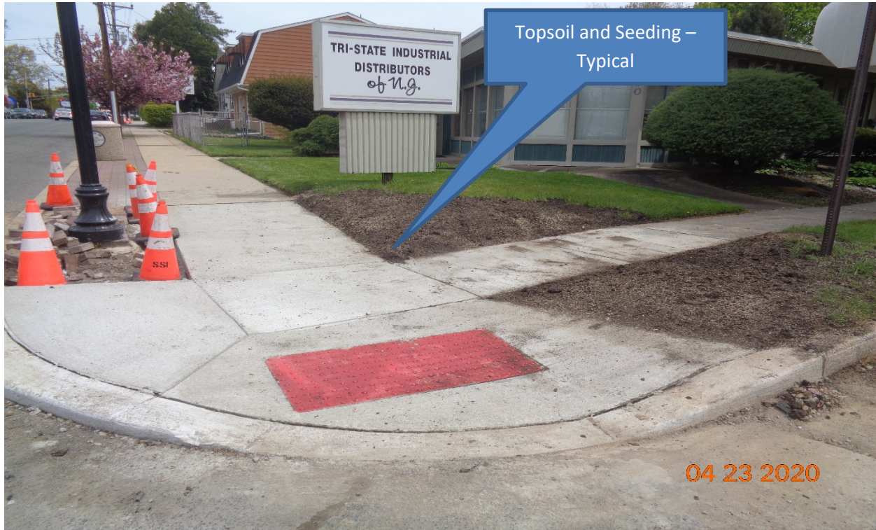
Figure 13: West sidewalk and HC Ramp at Scovel Avenue, RT – Typical Topsoil and seeding at all locations.
