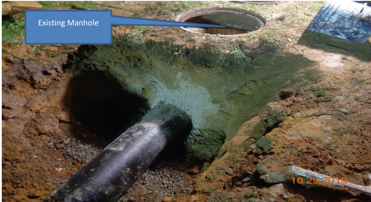
Figure 5: Installation of 12" ductile iron pipe across Derosse Avenue form existing inlet to existing manhole.
