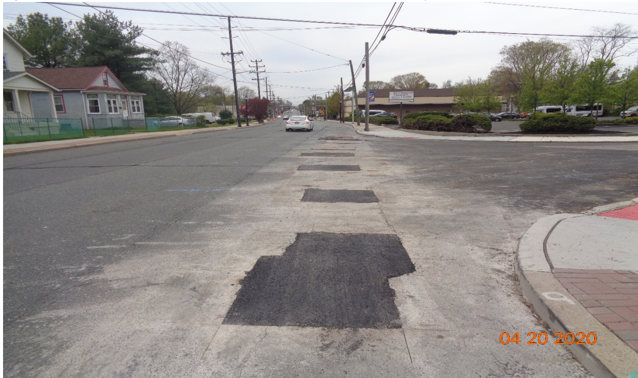
Figure 16: Asphalt was placed for previously placed concrete patch area, Typical at all locations.
