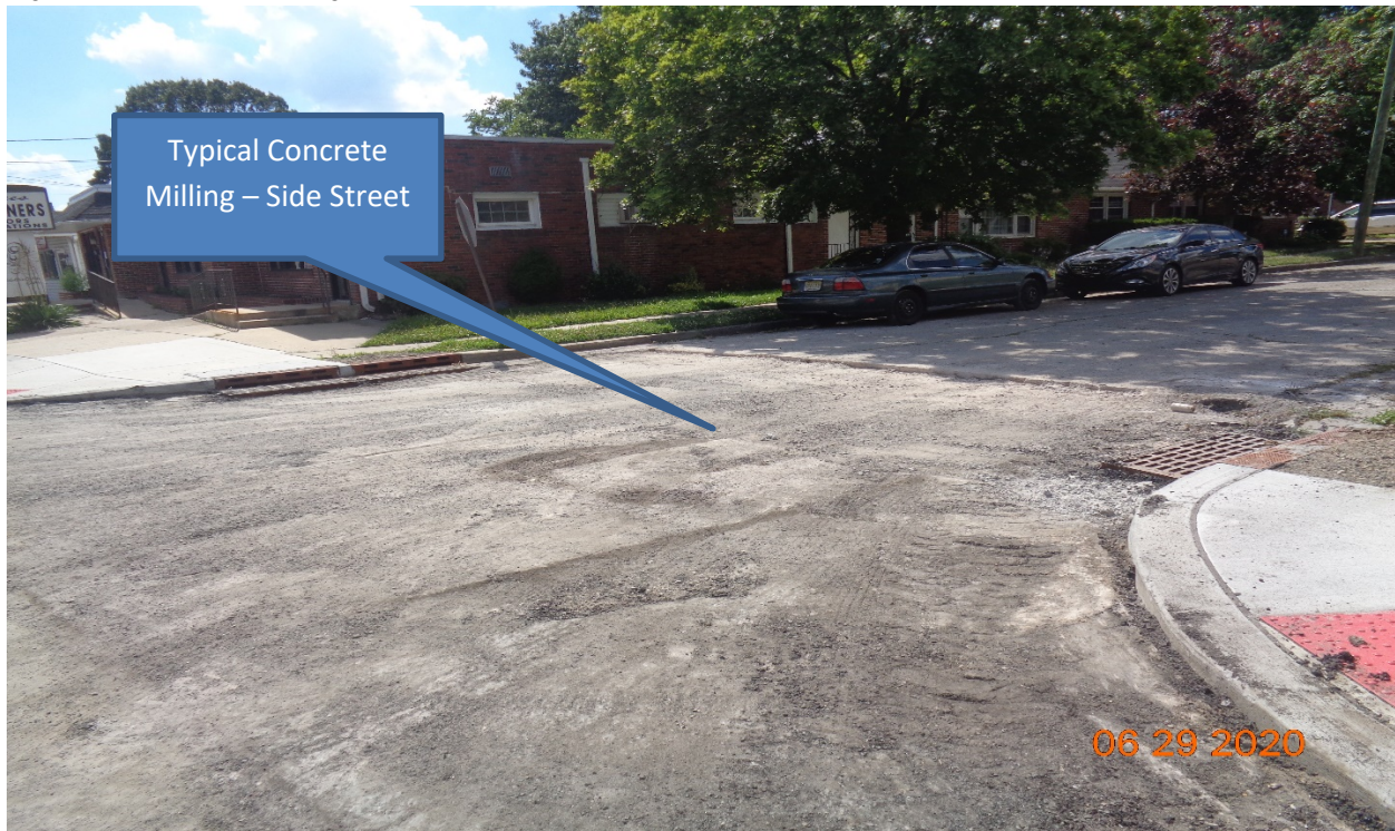
Figure 4: Concrete Milling along Horner Avenue, LT – Typical all side street Concrete Milling.
