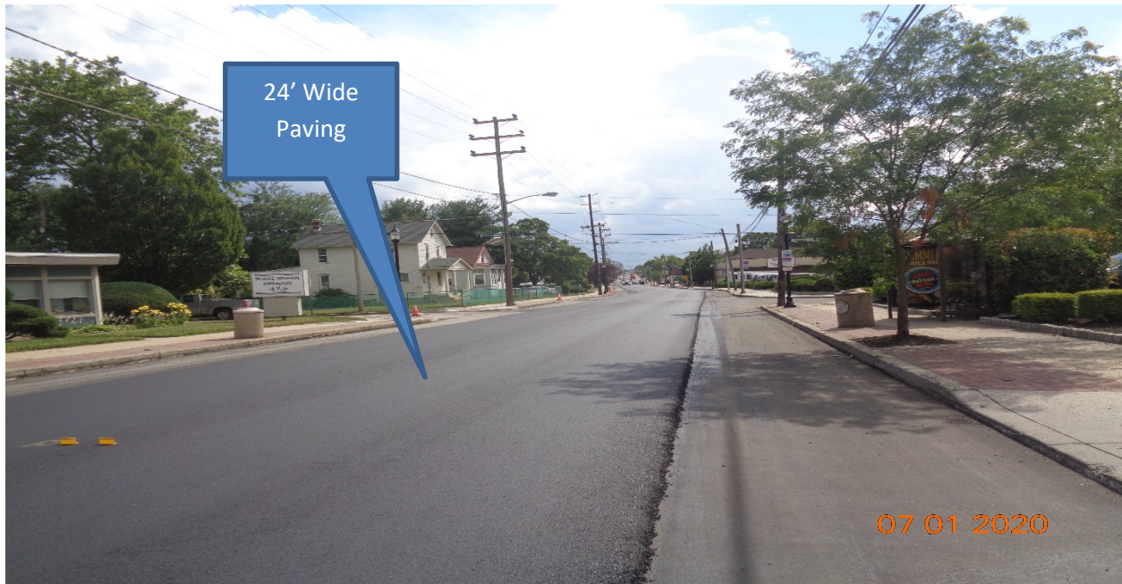
Figure 10: Hot Mix Asphalt 9.5 M surface Course was placed along Westfield Avenue from Sherman Avenue STA 109+50 – Tinsman Avenue 64+00
