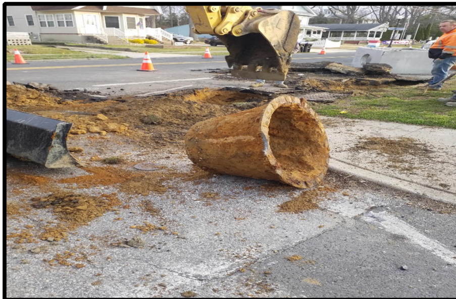
Photograph 3 – Old Manhole casting found in roadway – Buried Treasury!
