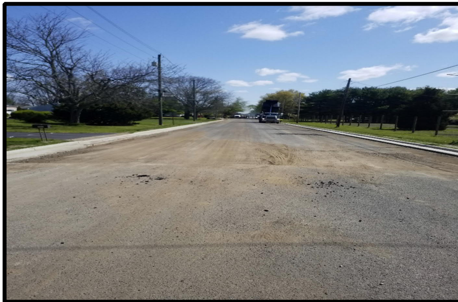
Photograph 3 – Full Depth Reclamation (FDR) milled to grade from Forth to Jackson Road.
