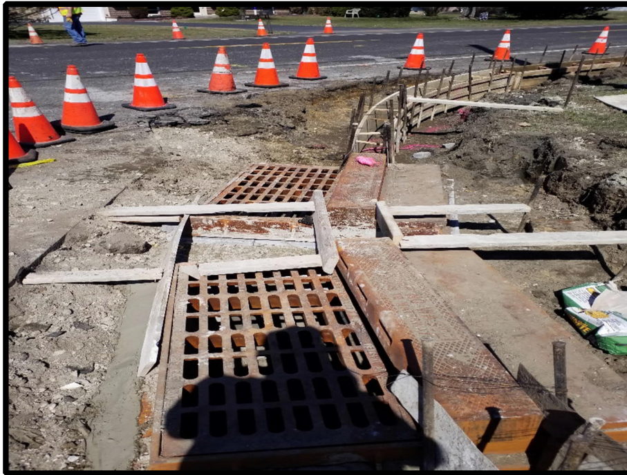
Photograph 2 – New “B” Inlet and casting set on both new and old at 4 th Street.
