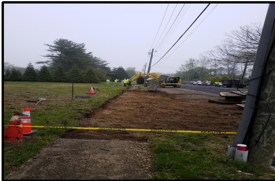
Photograph 3 – Trees removed that caused curb, sidewalk displacement and safety concerns.
