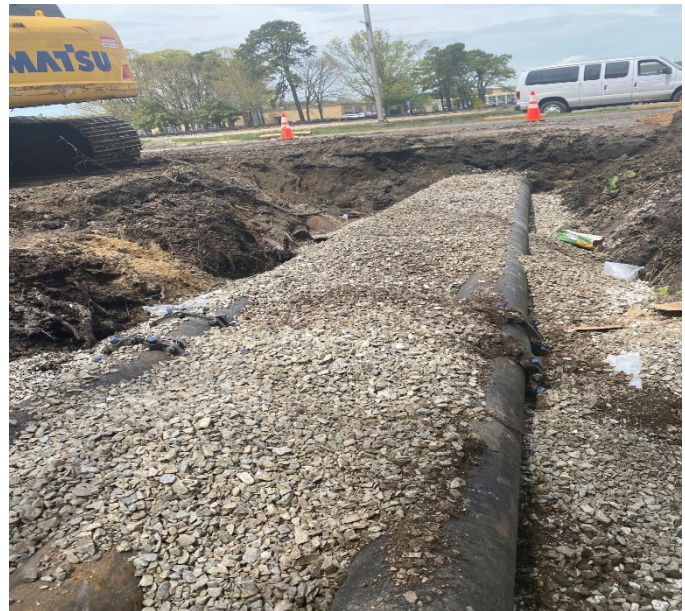
Figure 2: (3) Ductile Iron Pipe Crossing at CCTS
