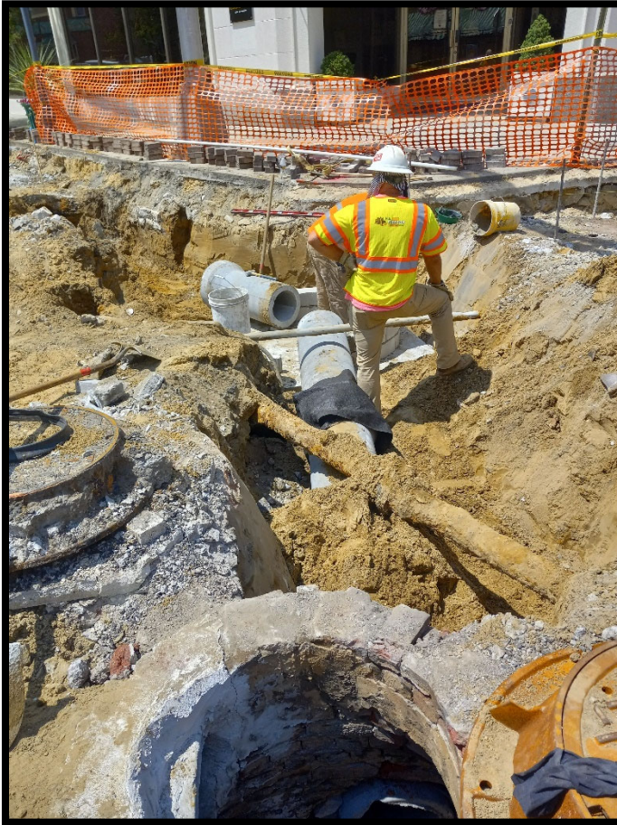
Photograph 2 – Storm improvements being installed in the Centre Street and Park Avenue intersection.
