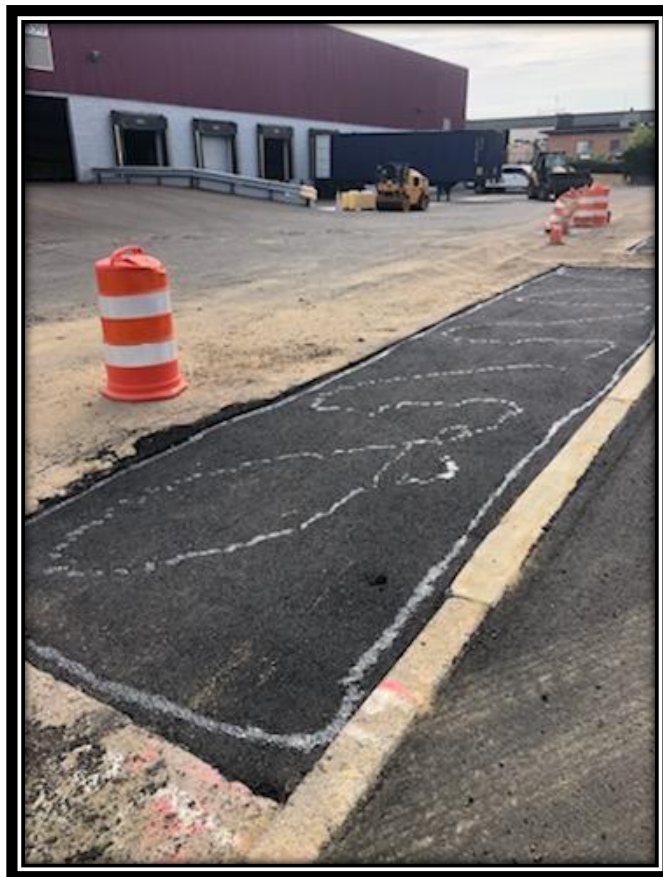
Figure: 1 – Installation of 2” thick HMA base course lift prior to installation of 2” thick HMA surface course lift for 4” thick HMA driveway along the westbound lane between the railroad tracks and Sherman Lane
