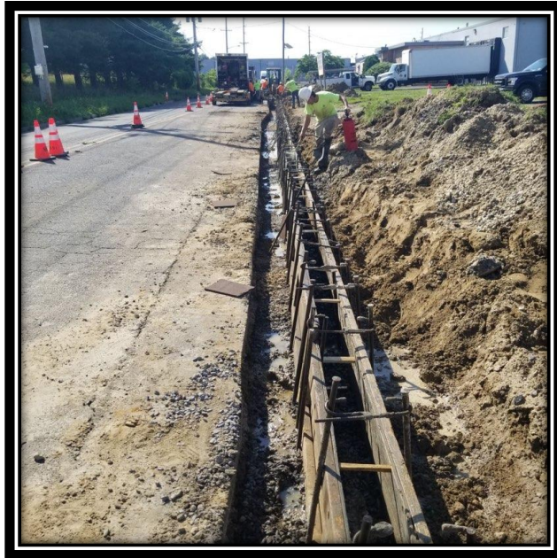
Figure: 2 – Installation of formwork for 9” x 18” Concrete Vertical Curb along the eastbound lane between River Road and Sherman Lane
