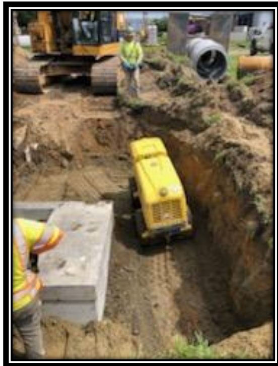
Figure: 3 – Compaction of newly installed 36” RCP storm sewer trench along the eastbound lane of Sherman Avenue between River Road and Sherman Lane
