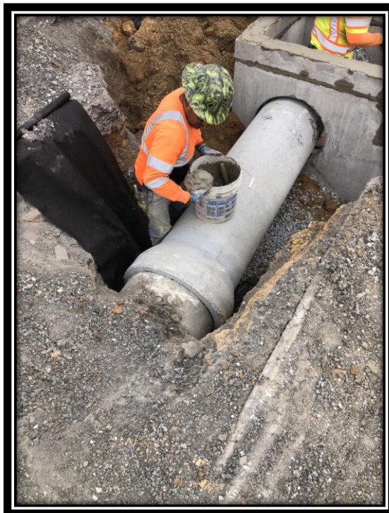
Figure: 3 – Installation of 24” RCP storm sewer along the eastbound lane of Sherman Avenue between Sherman Lane and the Railroad Tracks
