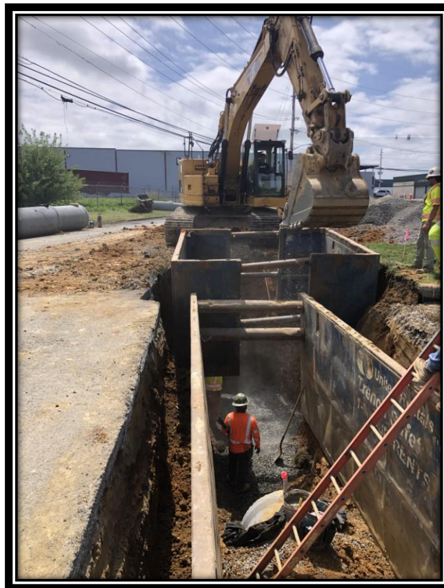
Figure: 1 – Installation of 36” RCP storm sewer along the eastbound lane of Sherman Avenue between River Road and Sherman Lane
