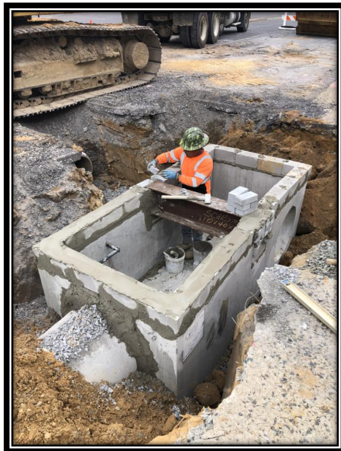
Figure: 1 – Installation of Type Double 'B' Inlet along the eastbound lane between Sherman Lane and the Railroad Tracks
