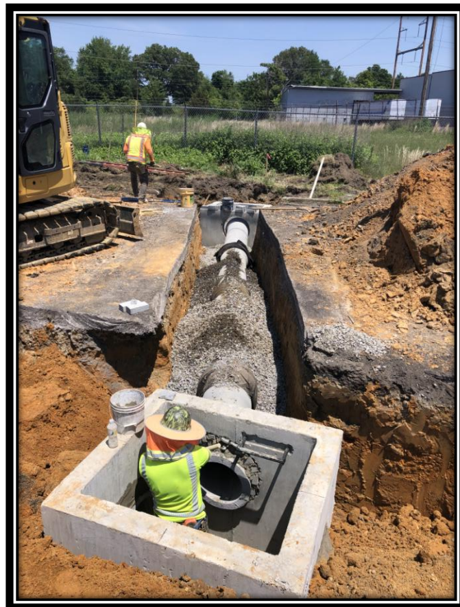
Figure: 1 – Installation of 15” RCP storm sewer and Type B Inlet between River Road and Sherman Lane
