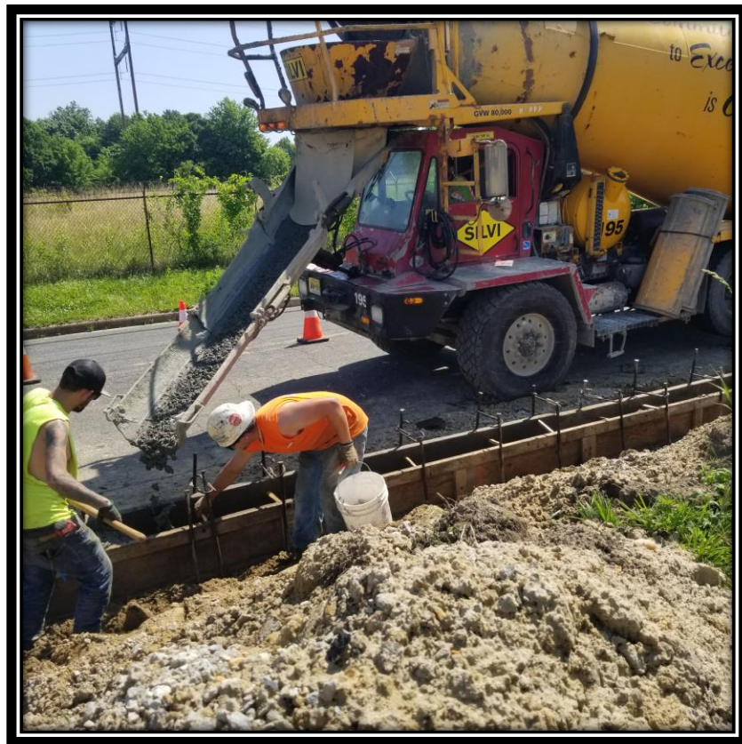
Figure: 1 – Installation of 9” x 18” Concrete Vertical Curb along the eastbound lane between River Road and Sherman Lane
