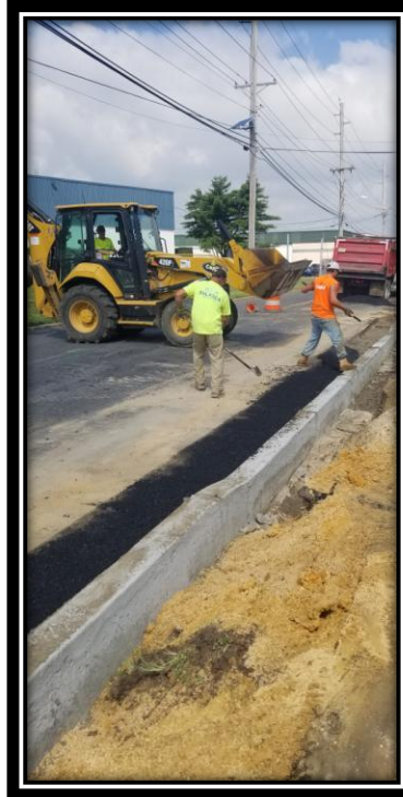
Figure: 3 – Installation of 9M64 base course in front of 9" x 18" Concrete Vertical Curb along the eastbound lane between River Road and Sherman Lane
