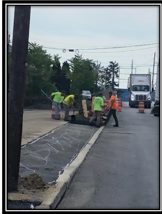
Figure: 2 – Installation of 2” thick HMA surface course lift for 4” thick HMA driveway along the westbound lane between the railroad tracks and Sherman Lane
