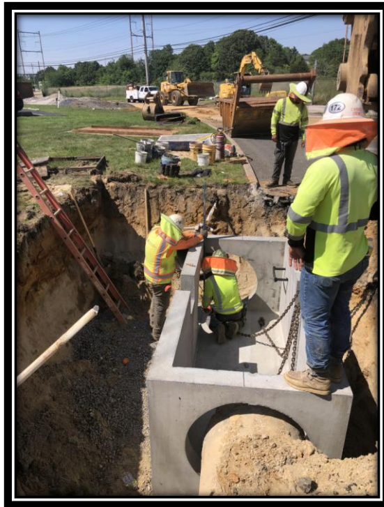
Figure: 2 – Installation of Type Double ‘B’ Inlet along the eastbound lane approaching the intersection with Sherman Lane
