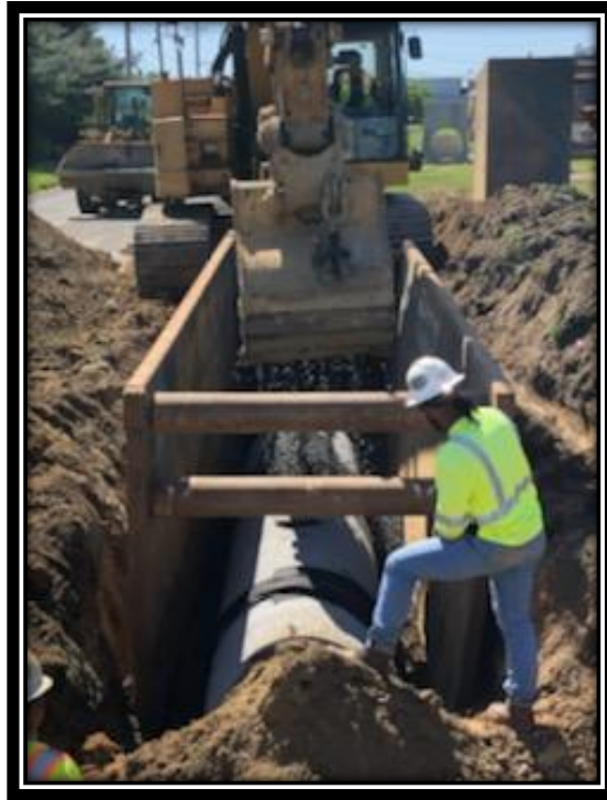
Figure: 2 – Installation of 36” RCP storm sewer along the eastbound lane of Sherman Avenue between River Road and Sherman Lane
