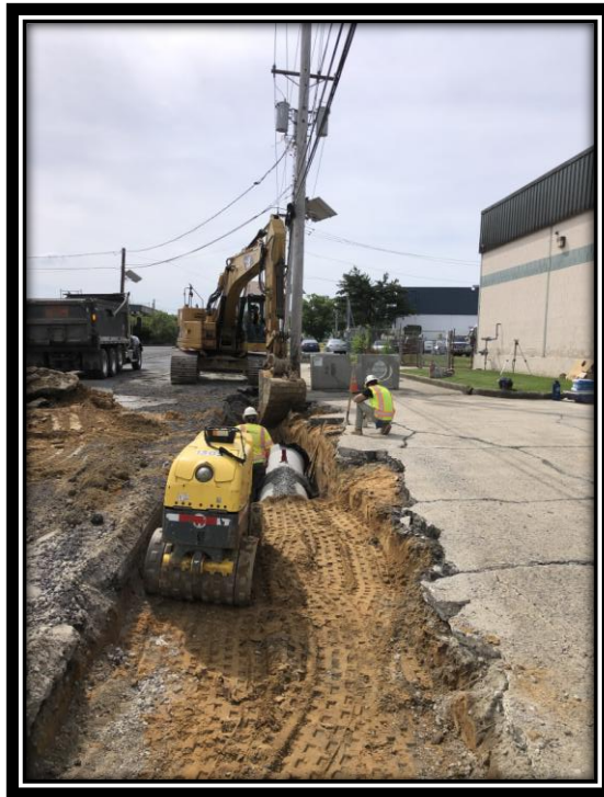
Figure: 2 – Compaction of the 24” RCP storm sewer along the eastbound lane between Sherman Lane and the Railroad Tracks
