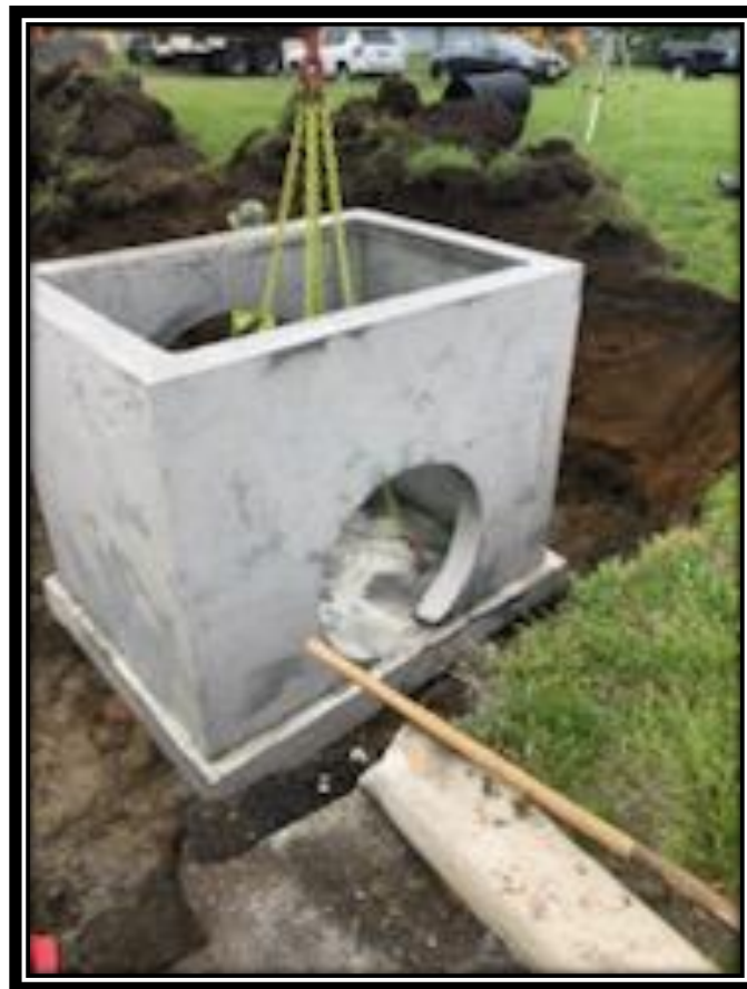
Figure: 1 – Installation of type B-1 inlet along the eastbound lane of Sherman Avenue between River Road and Sherman Lane
