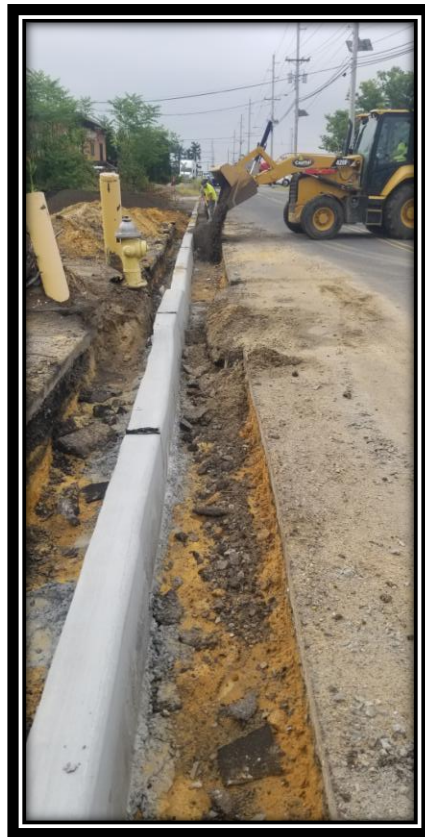
Figure: 1 – Backfill in front of 9” x 18” Concrete Vertical Curb along the westbound lane between the Railroad Tracks and Sherman Lane
