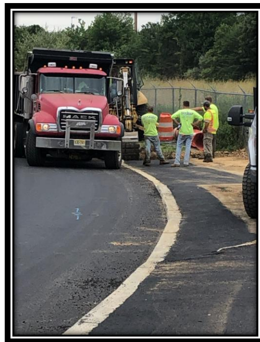
Figure: 3 – Installation of 4” thick HMA driveway along the westbound lane between Sherman Lane and River Road
