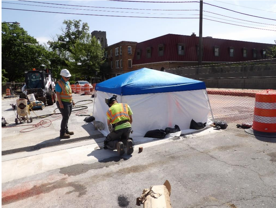
Figure 6 – Enclosure set up for sandblasting operation for the deck end PPC joint
