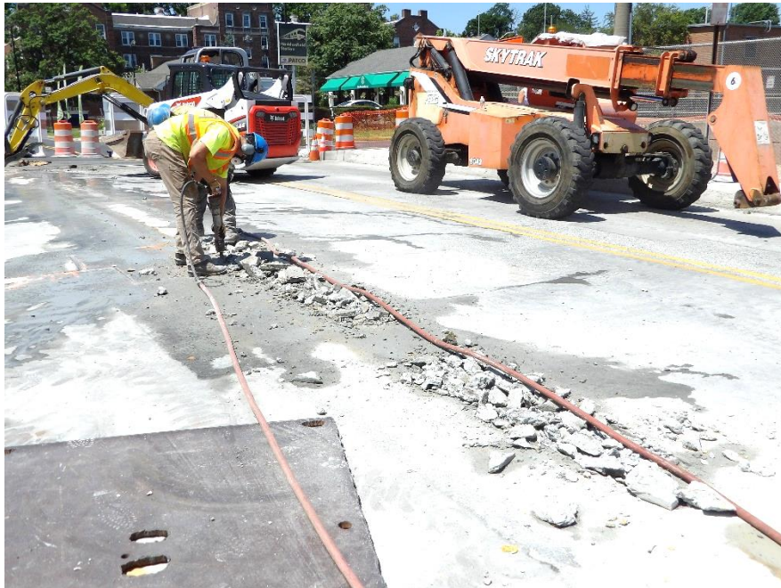
Figure 3 – Workers removed the deteriorated concrete from the top of the bridge deck
