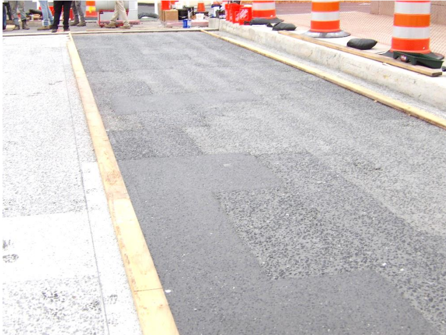
Figure 3 – PPC primer was mixed and applied to the top of deck in each lane
