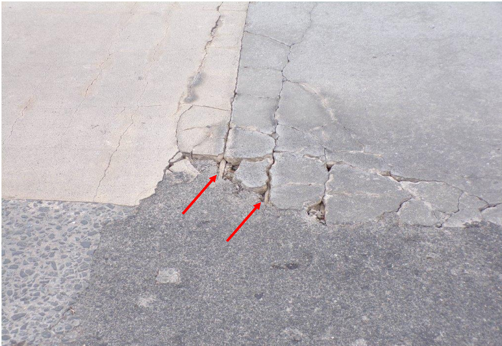
BEFORE: Exposed deck reinforcement within deteriorated patch in the southbound lane, looking east.
