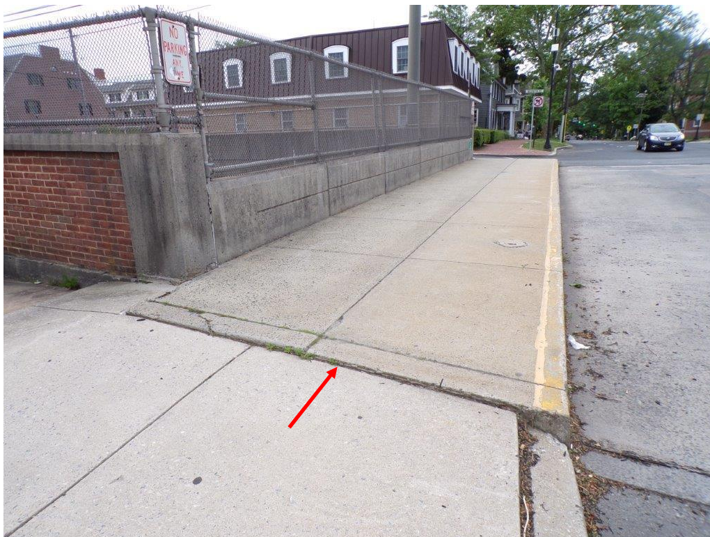
BEFORE: Settlement of the approach sidewalk at the northeast corner, looking south. Approach curb settled.
