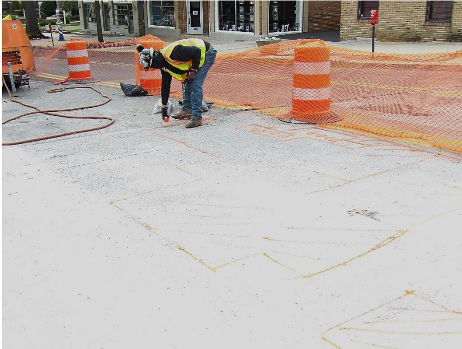
Figure 1 – Top of deck, Stage 1, was sounded for deteriorated concrete areas
