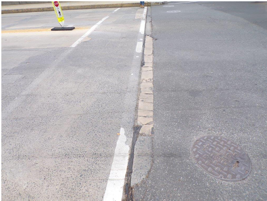
BEFORE: Compression seal at south deck joint torn full-length, looking east. Deck header is spalled and cracked.
