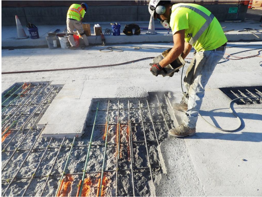
Figure 4 – After cleaning, the patch areas were sprayed with a concrete bonding agent
