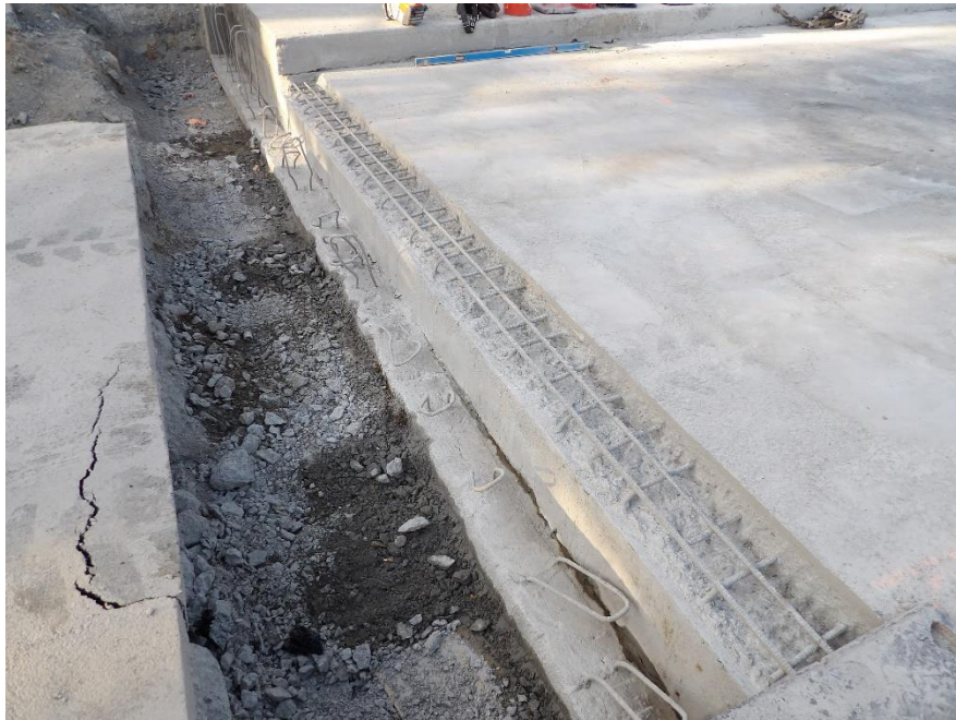
Figure 3 – Workers completed removal of the headers and deck concrete for the PPC joint
