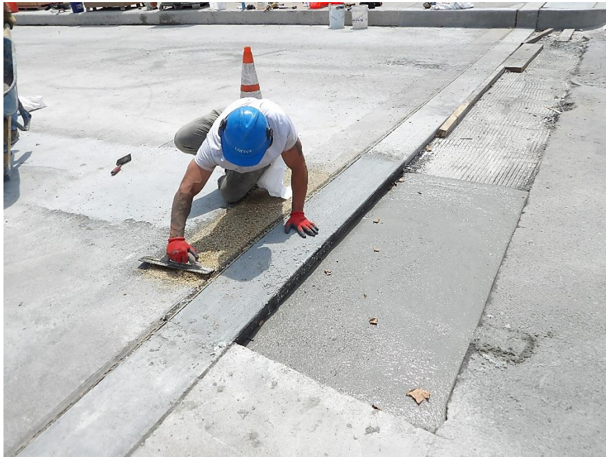
Figure 3 – Workers poured and finished the PPC header joints at each deck end
