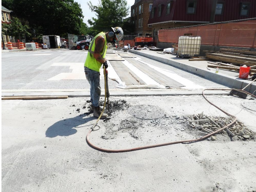
Figure 6 – Chipping around approach utility covers that were inaccessible to the milling machine
