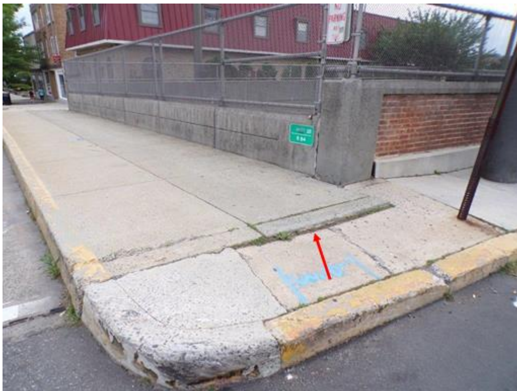
BEFORE: Settlement of the approach sidewalk at the southeast corner, looking northeast.
