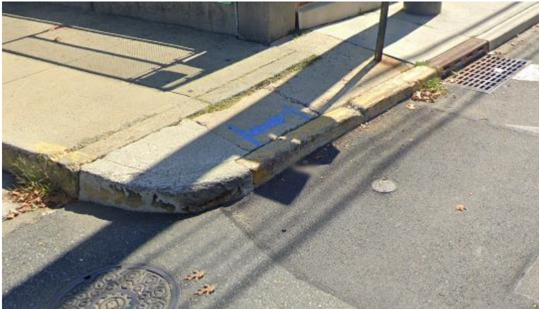
BEFORE: Southeast Corner Condition
