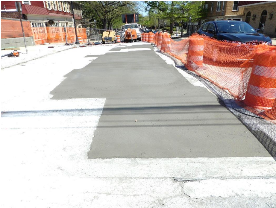
Figure 9 – Concrete was sprayed with a liquid curing compound and left to set
