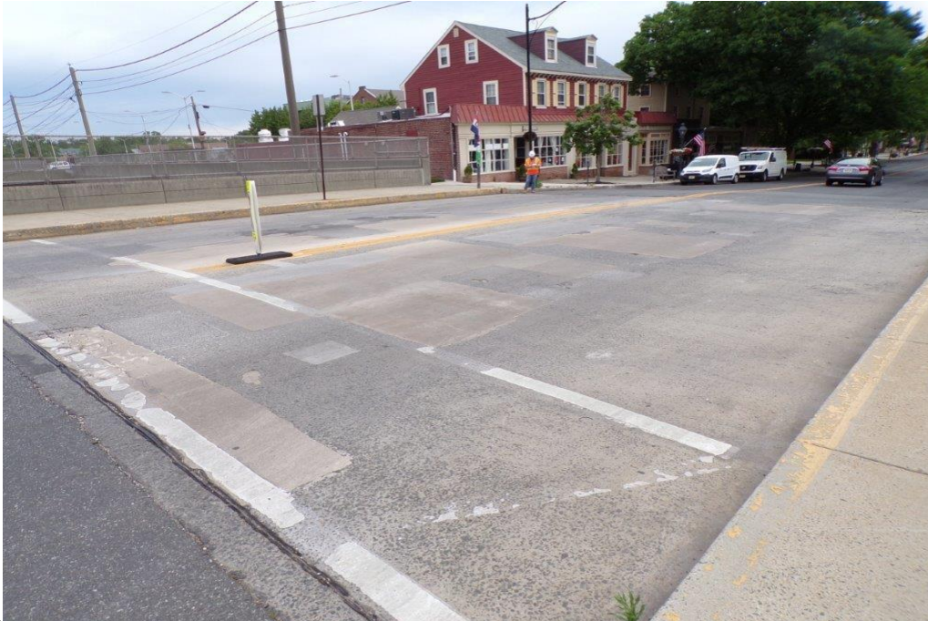
BEFORE: – General view of deck Patches typical throughout.
