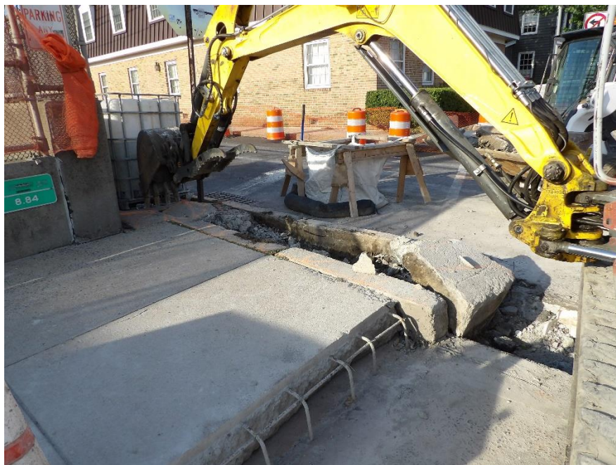
Figure 1 – Workers continued to excavate behind the abutments for header demolition and removal
