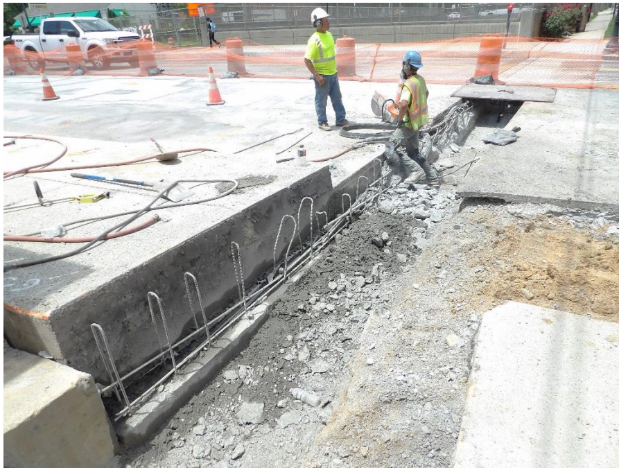
Figure 11 – Workers continue to remove the east abutment header, work is in progress
