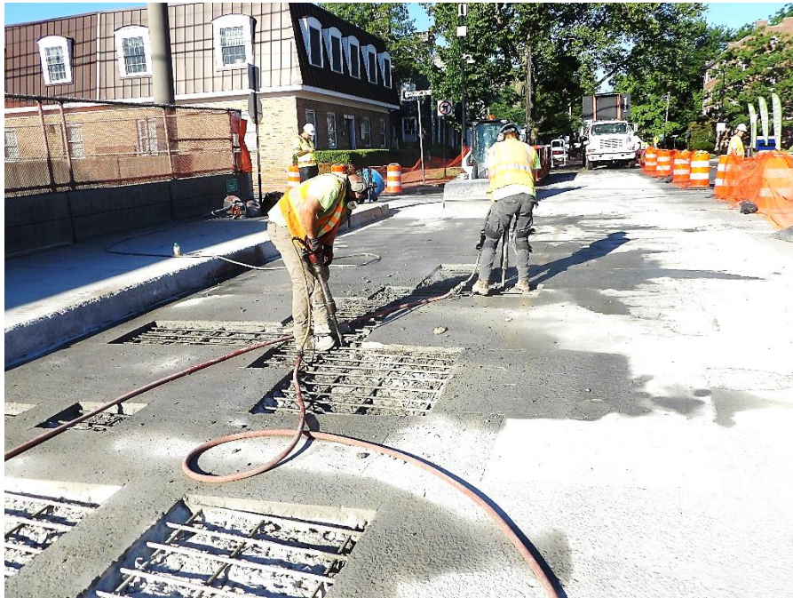
Figure 1 – Workers began to remove deteriorated concrete from the top of deck in Stage 2
