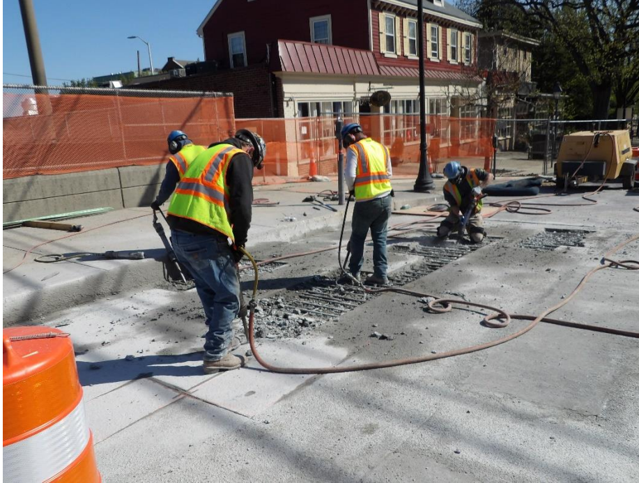
Figure 10 – Workers resume removal of deteriorated concrete from Stage 1 for the next pour
