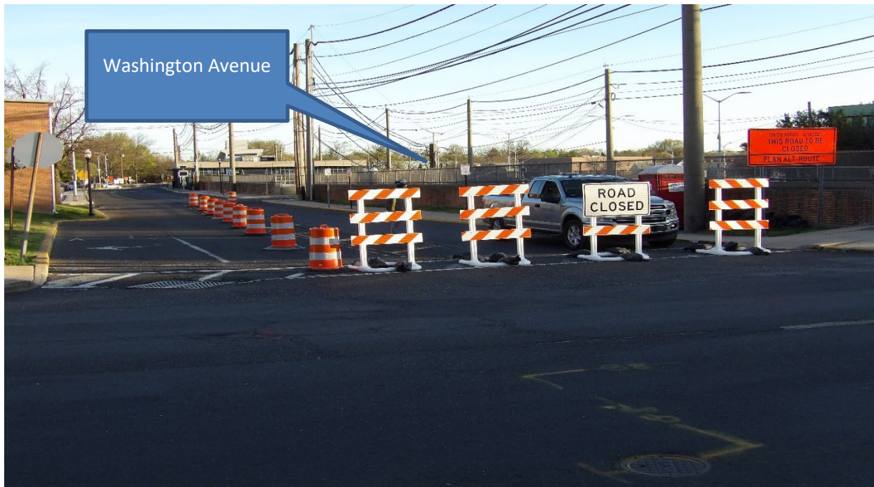
Figure 7: Washing Avenue Closed along West Side
