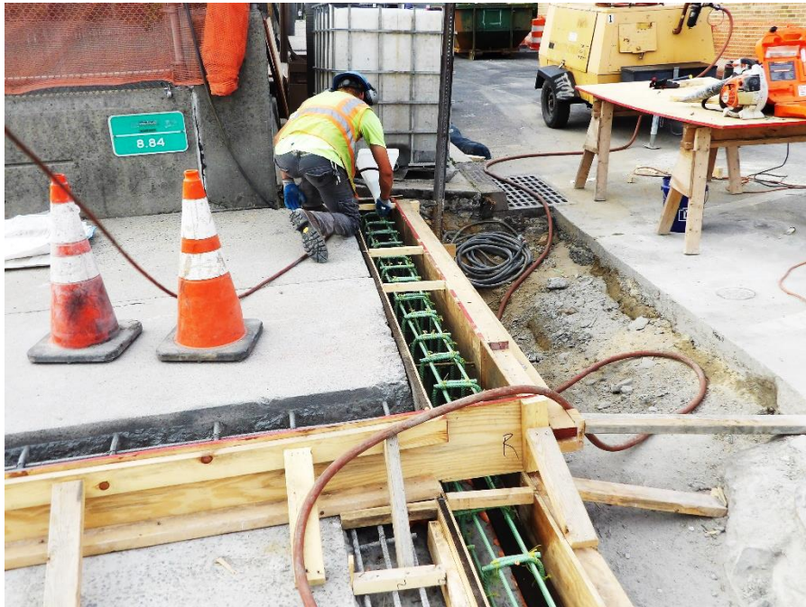
Figure 1 – Workers completed excavations and formed for the new headers at each abutment
