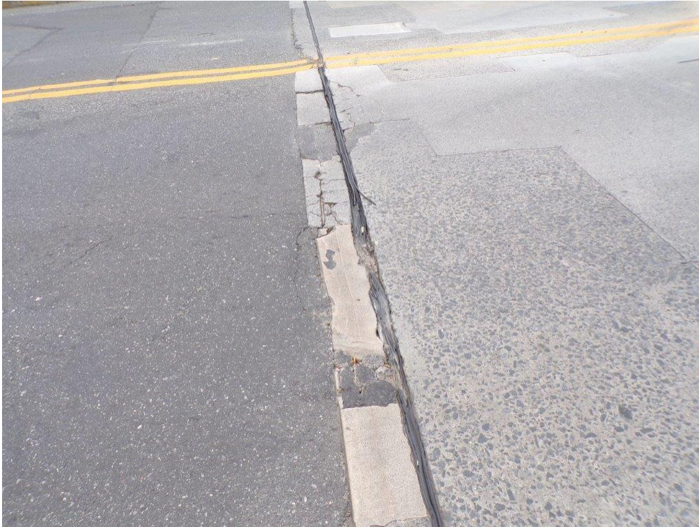
BEFORE: Crushed and torn compression seal at north deck joint in southbound lane, looking east. Deck header is spalled with exposed reinforcement.
