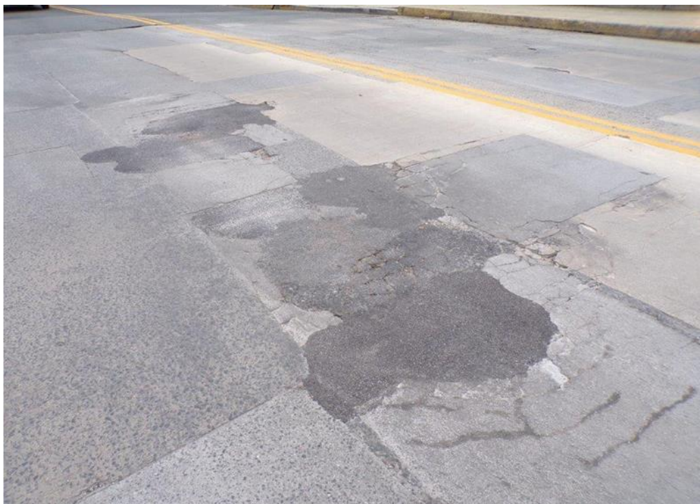
BEFORE: Large area of uneven asphalt patched spalls, cracked and broken patches with exposed reinforcement in southbound lane, looking southeast.
