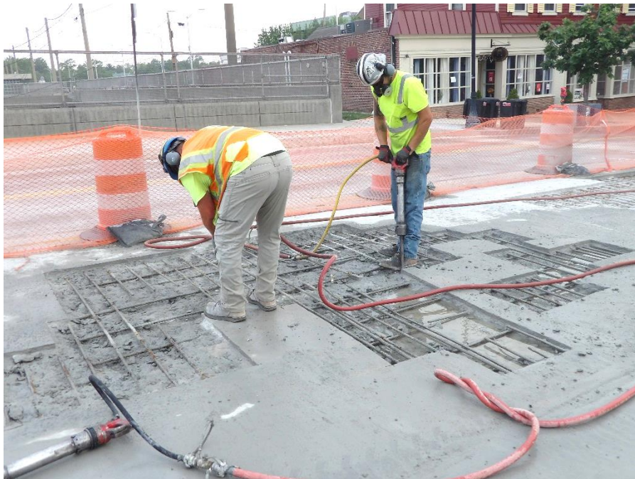
Figure 1 – Workers continued to remove deteriorated concrete from the top of deck in Stage 2
