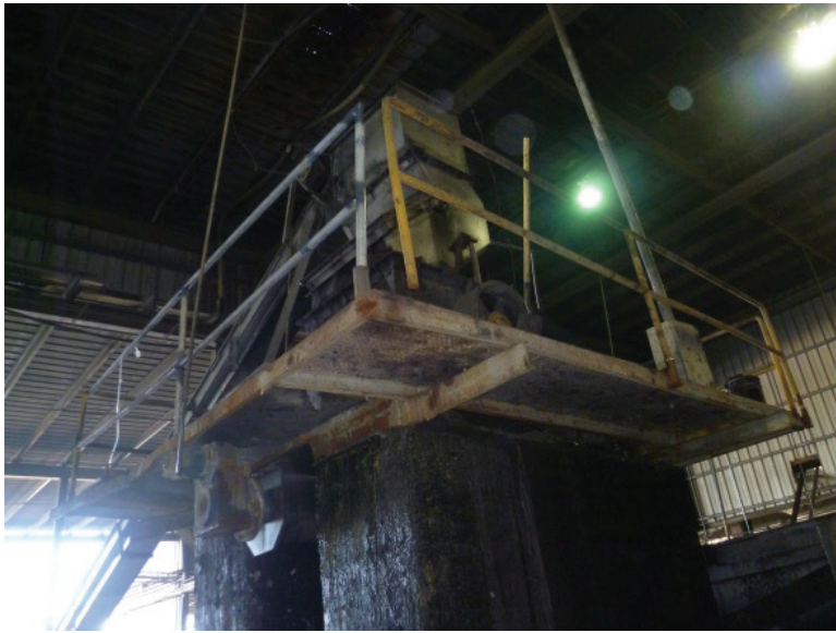
Figure 10. Unsecured guardrail on battery breaker mezzanine. Photo by NIOSH.
