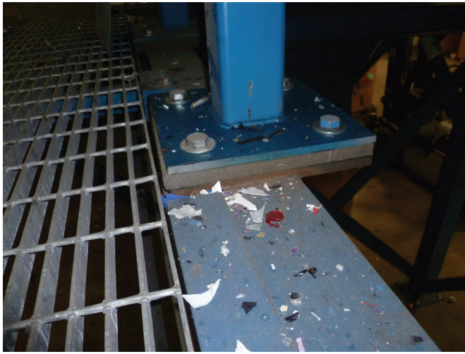
Figure 7. Eddy current separator bolted to support frame with vibration isolation felt at the point of attachment. Photo by NIOSH.
