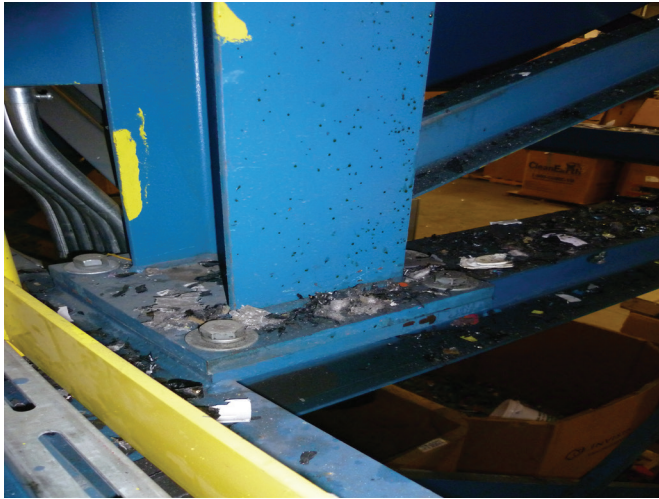
Figure 8. Eddy current separator bolted directly to support frame. Photo by NIOSH.
