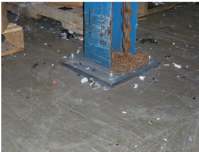
Figure 9. Support frame below eddy current separator bolted directly to concrete floor. Photo by NIOSH.
