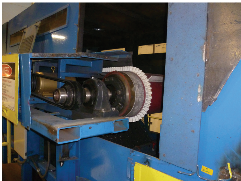
Figure 11. Unguarded belt drive on eddy current conveyor. Photo by NIOSH.
