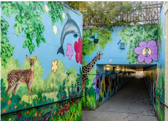
New lighting in the East Washington Avenue pedestrian tunnel at Wright Street
