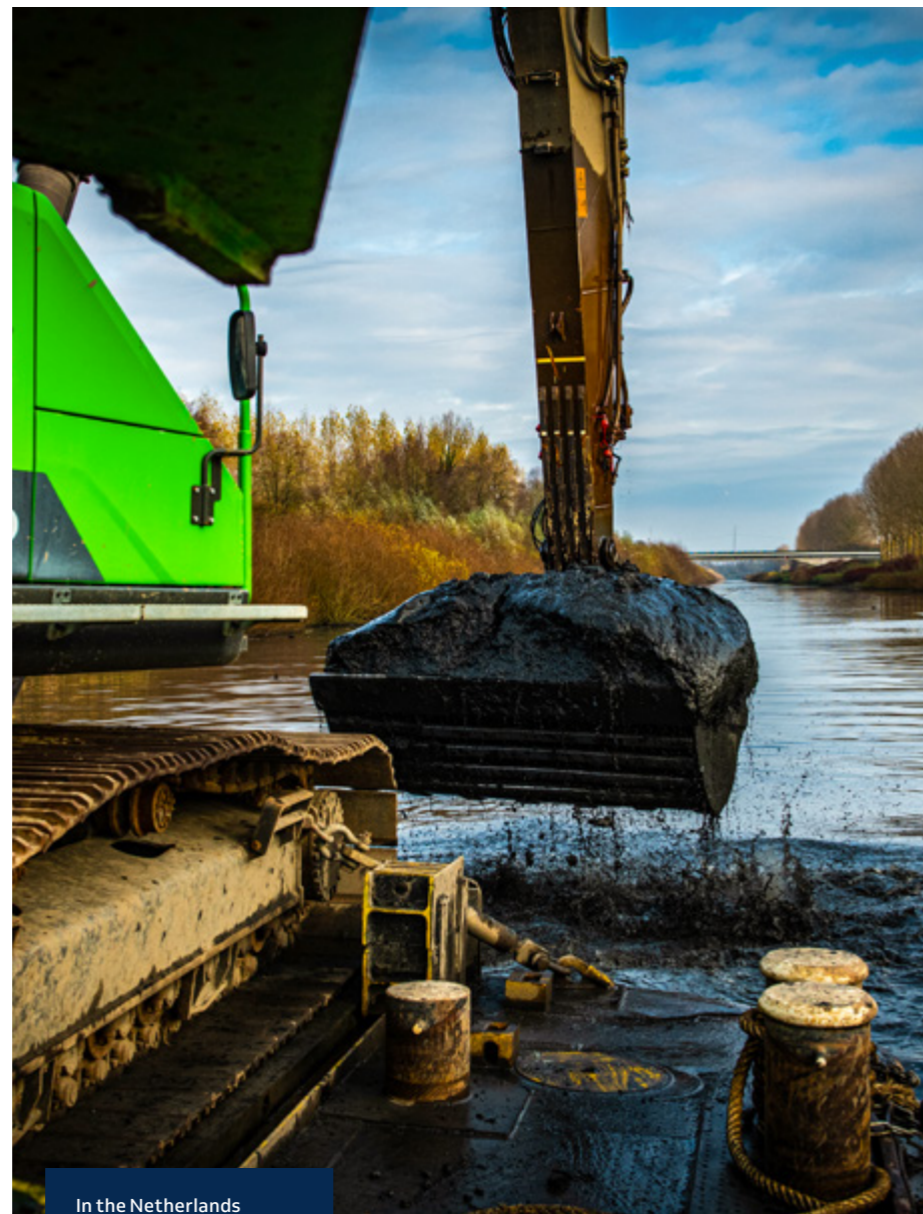
In the Netherlands we participate in a partnership to accelerate the energy transition in the infrastructure sector.
