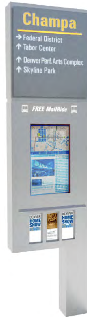
Way-finding sign pylon: near-term strategy – remove top decorative metal apparatus, repaint in silver metallic color. Long term strategy – replace with simpler, more weather resistant unit.
