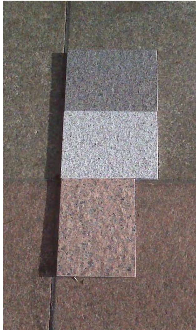
Mall granite paving: renovate per the Phase I Technical Assessment and Rehabilitation Study recommendations; new pavers at curb extensions to match color, paver size and pattern of existing; colors – Radiant Red, Charcoal Black and Sierra White from Cold Spring Granite.
