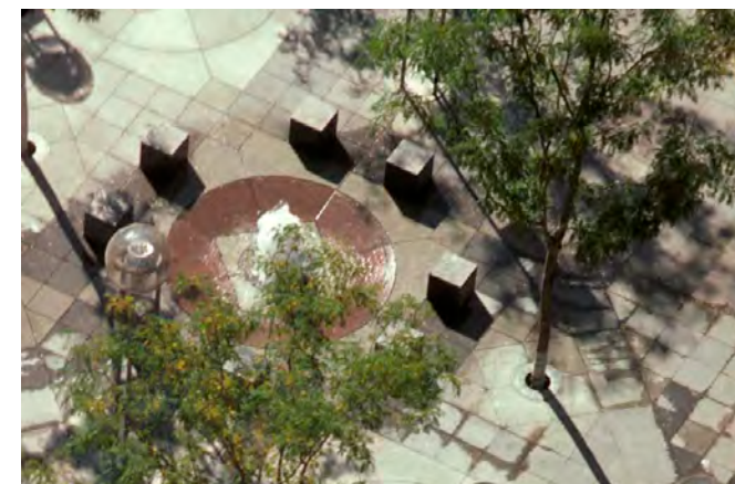
Original fountain basins are to be renovated and have out-board stone pedestal seats removed to allow pedestrian and ADA access along the median.
