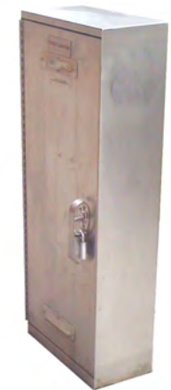
Electrical service cabinet: replace existing painted metal enclosures with smaller, manufactured stainless steel cabinet as electrical infrastructure is replaced with overall Mall renovation.
