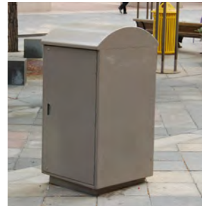
Electrical Service Cabinet: circuitry for all electrical components on the Mall; usually at mid-block; painted steel is subject to corrosion from de-icers in winter; bulkier than necessary for modern equipment.
