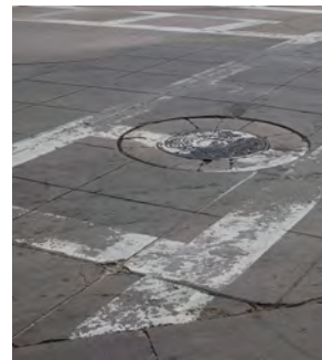
Concrete intersection paving: now 30 years old; has had subsequent utility trenching and is cracked, chipped, spalled and has differential settlement around manholes and former trenches; aesthetically inferior appearance.
