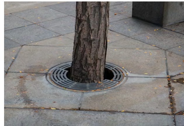
Tree well/grate: maintain current design; ensure accessibility to root vault box with renovation of granite paving; adjust metal grates wider to prevent damage to tree trunk.
