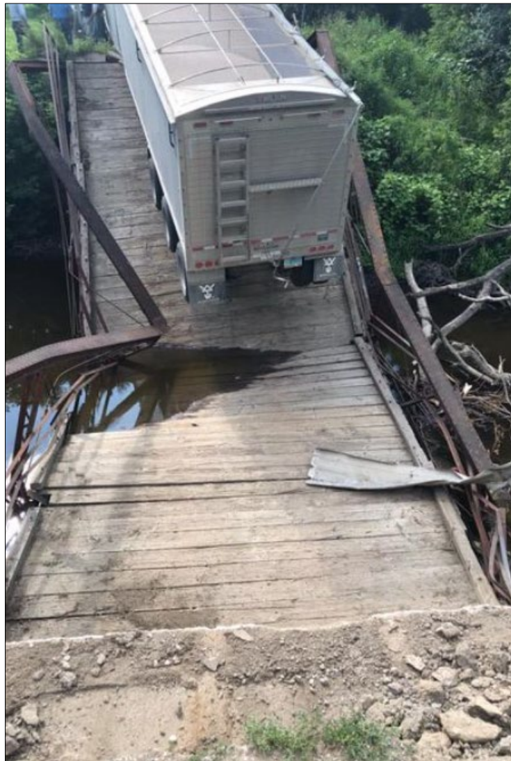
Figure 4.15-4: Northwood historic bridge fails under heavy weight.
