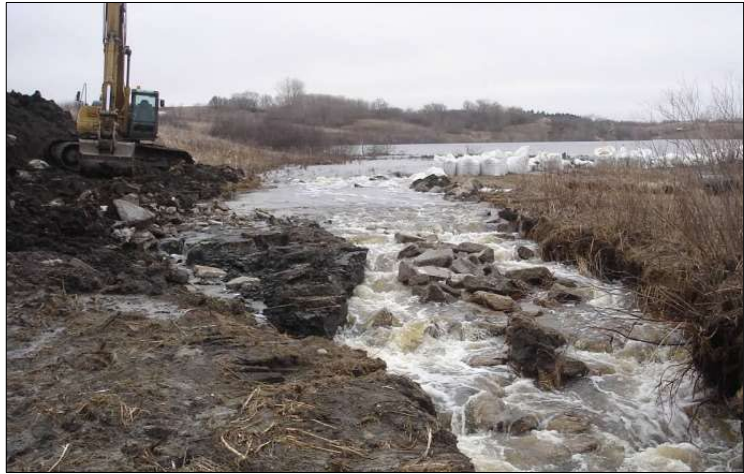
Figure 4.8-7: Erosion at Clausen Springs Dam, 18 April 2009
