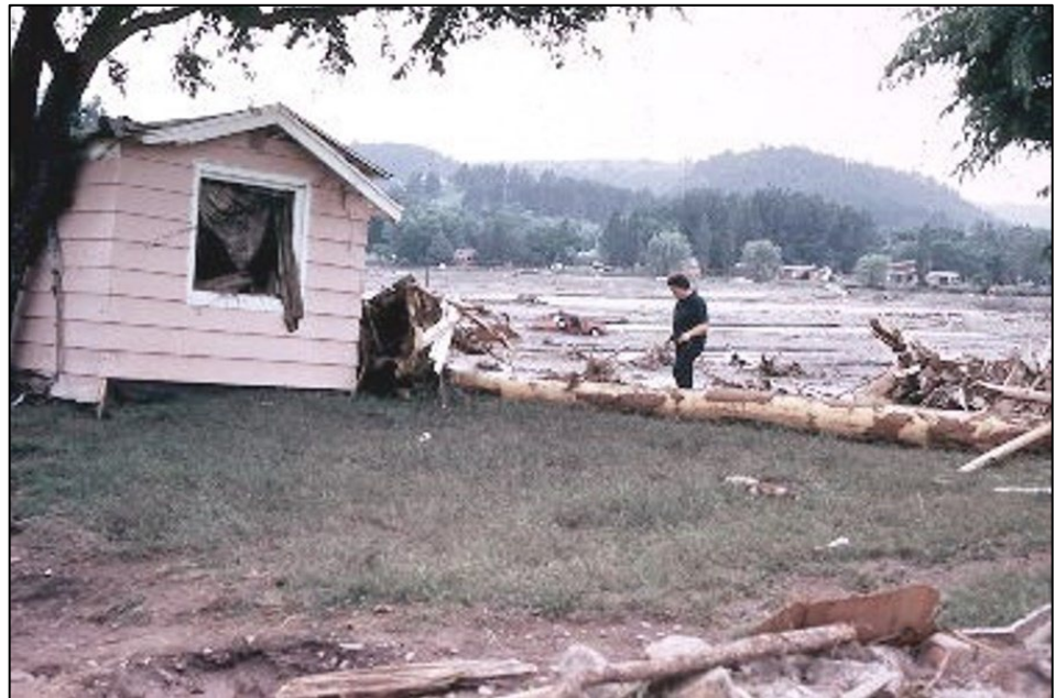
Figure 4.8-14: House Dislodged from Foundation from Canyon Lake Dam Failure, 1972
