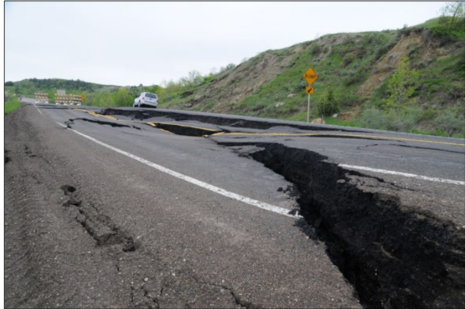
Figure 4.12-9: Highway 22 slumping, near Killdeer
