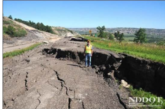
Highway 22 Landslide/North Dakota Department of Transportation
