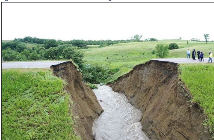
Figure 4.15-51: Road Washout in Standing Rock that Led to Fatalities
