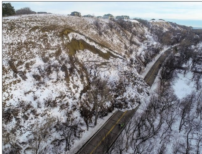
Figure 4.12-30: December 2019 Landslide on River Road, Burleigh County
