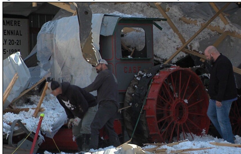
Figure 4.5-43: Sargent County Museum after Roof Collapse
