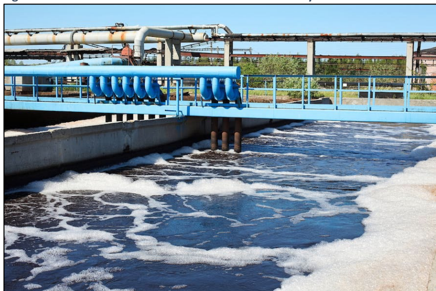
Figure 4.4-9: Oldsmar Florida's water treatment facility was attacked.
