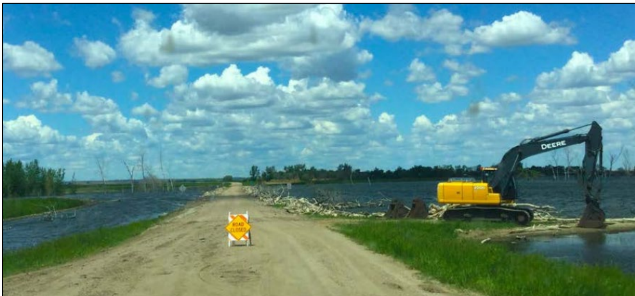
Figure 4.1-7: Rice Lake flooding threatens roads.
