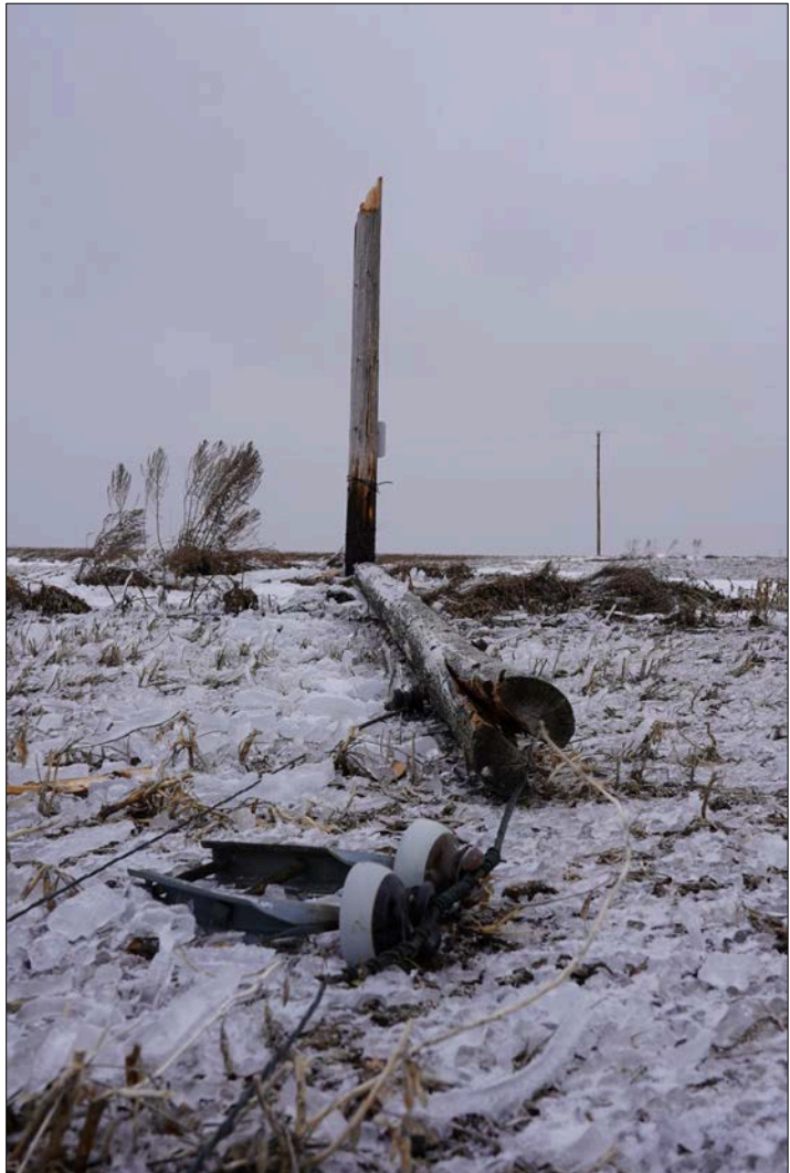
Figure 4.5-9: Shattered Power Poles, end of December 2023
