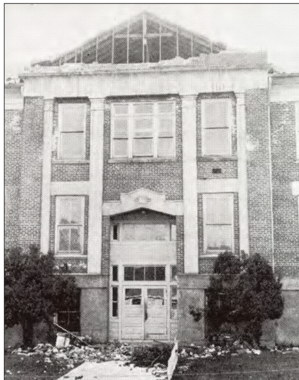
Figure 2. At Castle Rock, a high school student was killed as unanchored gable masonry cascaded to the walk outside the entrance. There could have been more casualties. (From Edwards, 1951.)
