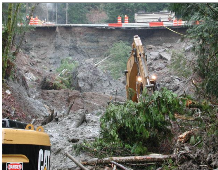
Figure 2. The M6.8 Nisqually earthquake in 2001 caused this landslide at U.S. Highway 101, northwest of Olympia. (Photo: Karl Wegmann/WADNR)
