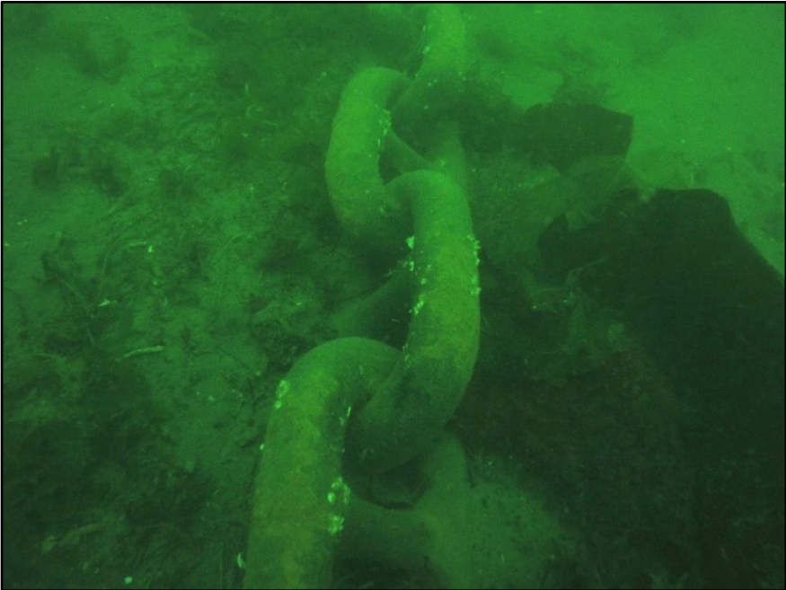
Photograph 16 : Underwater View of the Typical Condition of the Anchor Chain at the Channel Bottom.
