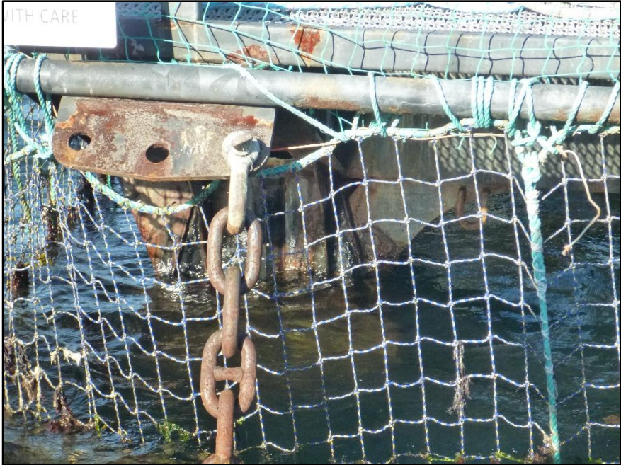
Photograph 9 : View of the Typical Corrosion of the Steel Plate and Shackle.
