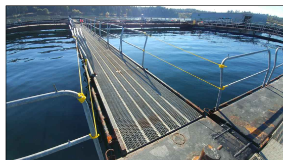
PHOTO 6 PONTON WALKWAY SURFACE
