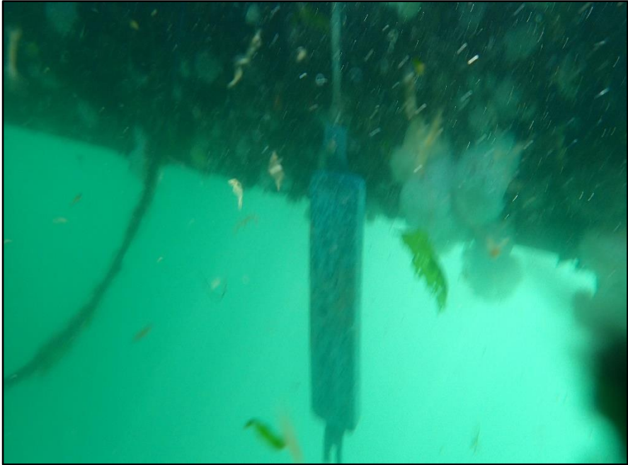
Photograph 5 : Underwater View of the Hanging Style Anode on the pontoons.
