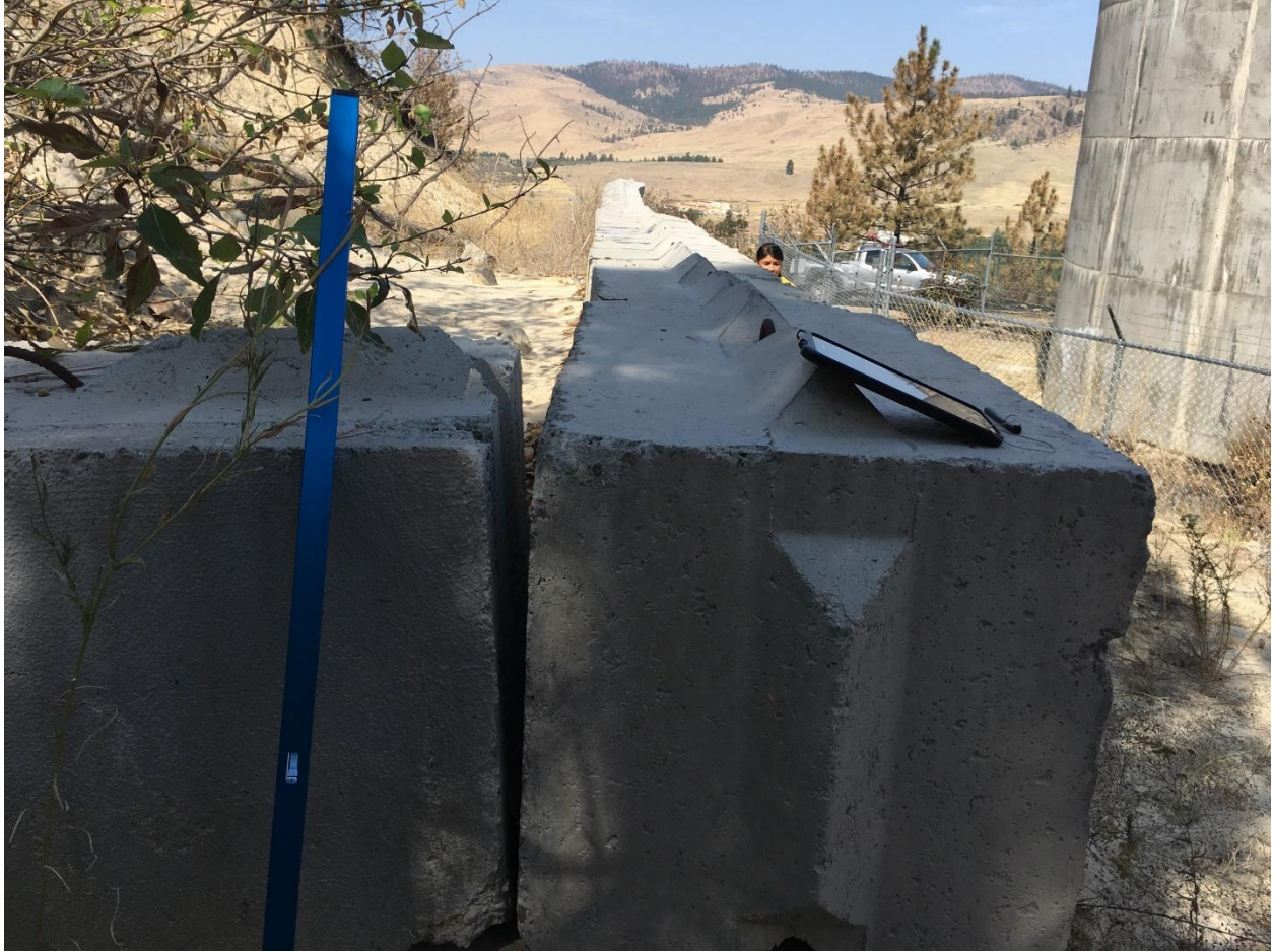
Figure 5. Deformation of 5-year-old retaining wall made of ecology blocks, looking west.
