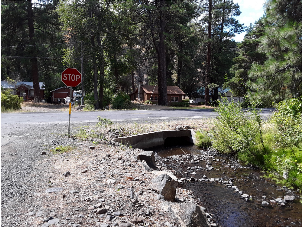
Figure 3. Box culvert at SR410, looking west toward homes 14710 and 14680 WA-410. Site 1 on Figure 2.
