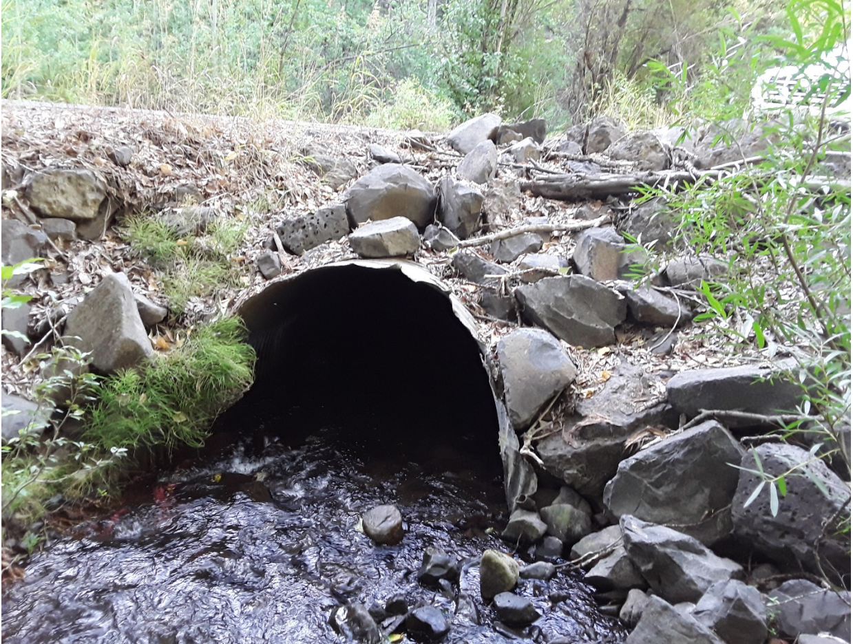
Figure 6. Site 5 on Figure 2, showing culvert under Rock Creek Road. Note bent and torn metal culvert edges from flood-borne rock impacts. Blockage of this culvert could divert the creek, blocking and damaging the road.
