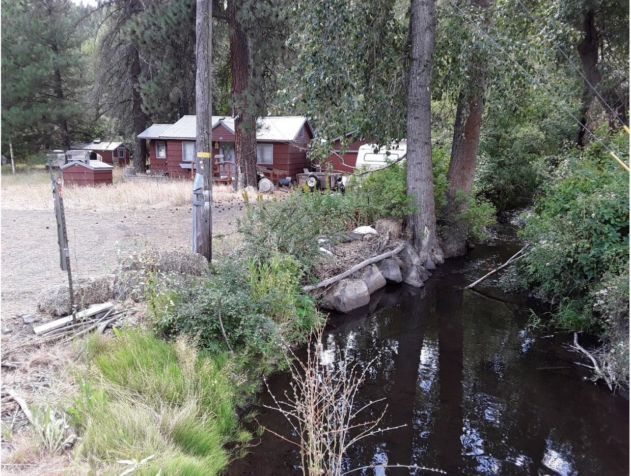
Figure 4. Home at 14680 WA-410, downstream of box culvert along Rock Creek. Note sandbags, boulders, and damage to the base of the tree trunk, second from right, as evidence for previous flooding events. Site 1 on Figure 2.
