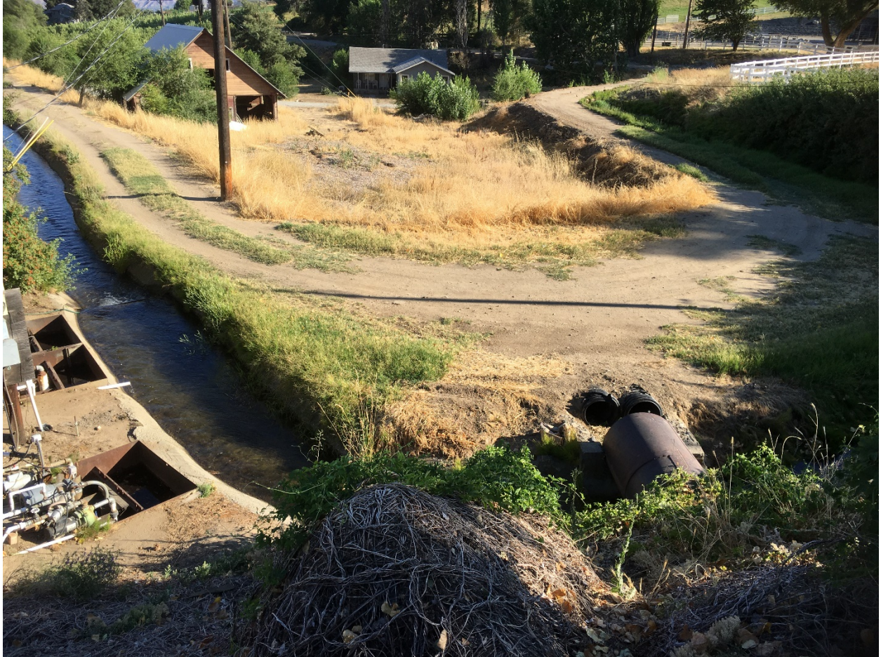
Figure 2. Photo taken downstream of Burch Hollow Lane, near 3510 Burchvale Rd (Location 20 on Plate 1). Depending on the amount of sediment that travels through the larger metal culvert, the smaller corrugated culverts could be clogged resulting in sediment in the canal.
