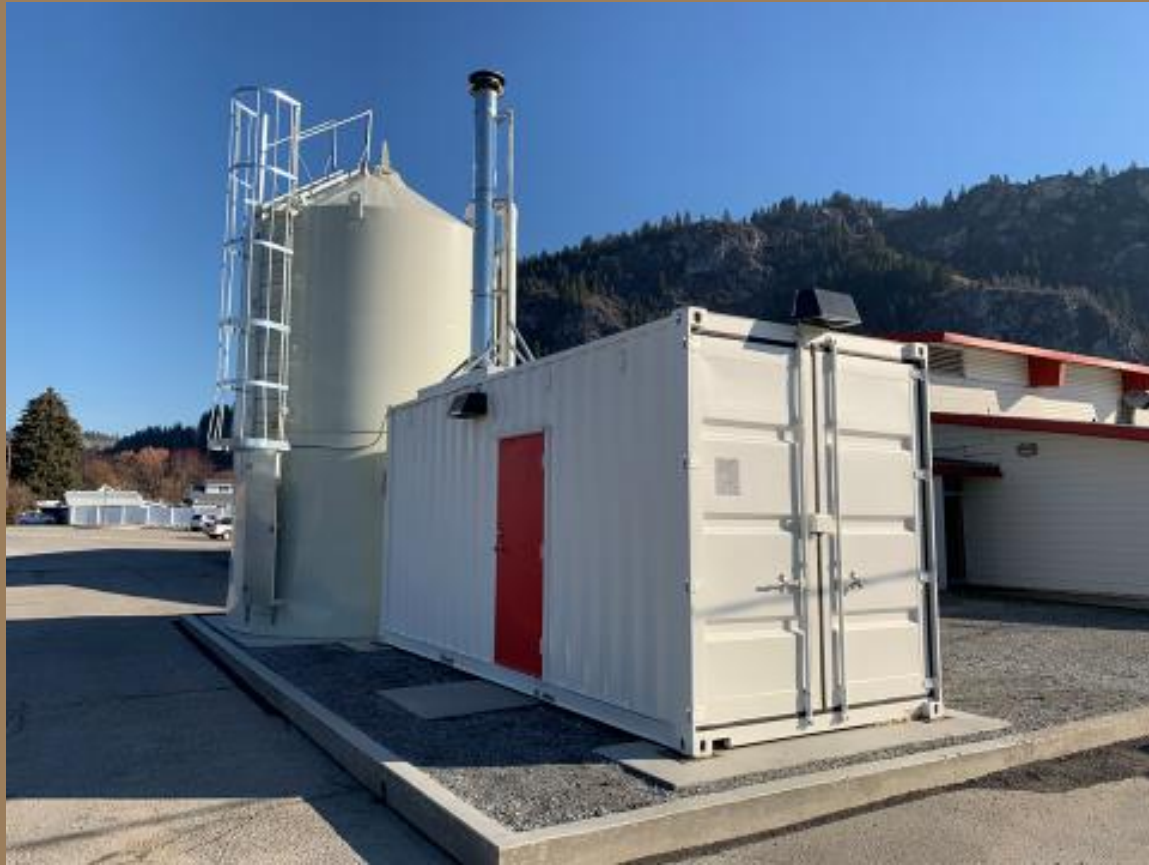
Wood Pellet Boiler (340K BTU), Northport School District Northport, WA, Stevens County
