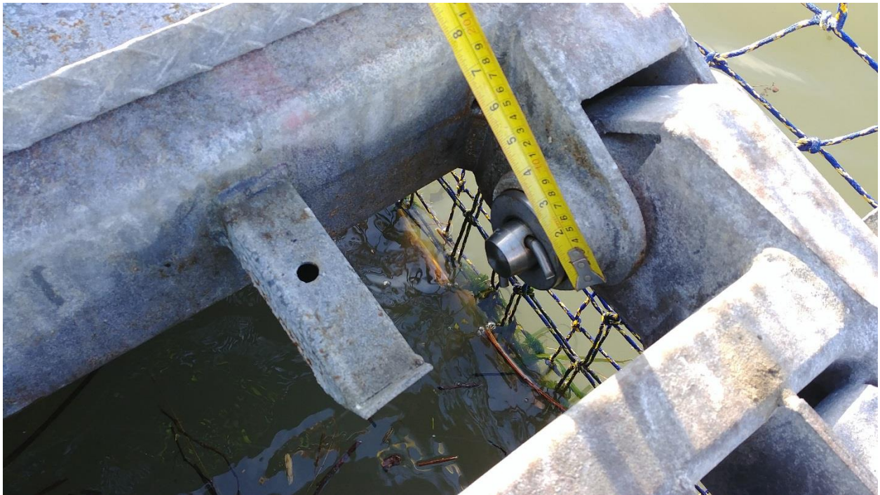
Figure C-97: Pin Connecting Hinged Segments of Main Walkways
