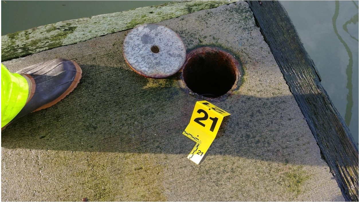
Figure C-62: Anchor #21, NW Corner of the Main Barge. Part of an Anchor Bridle System.
