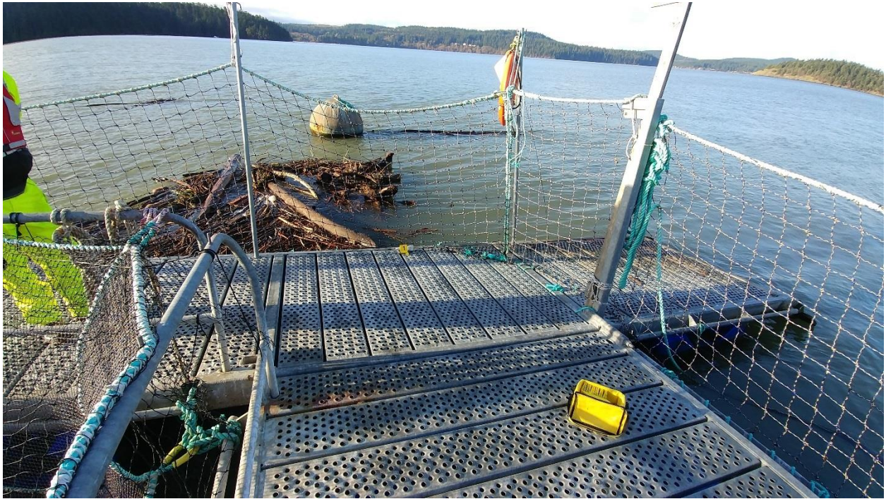
Figure C-10: Hope Island Net Pens - NW Corner, Inadequate Flotation
