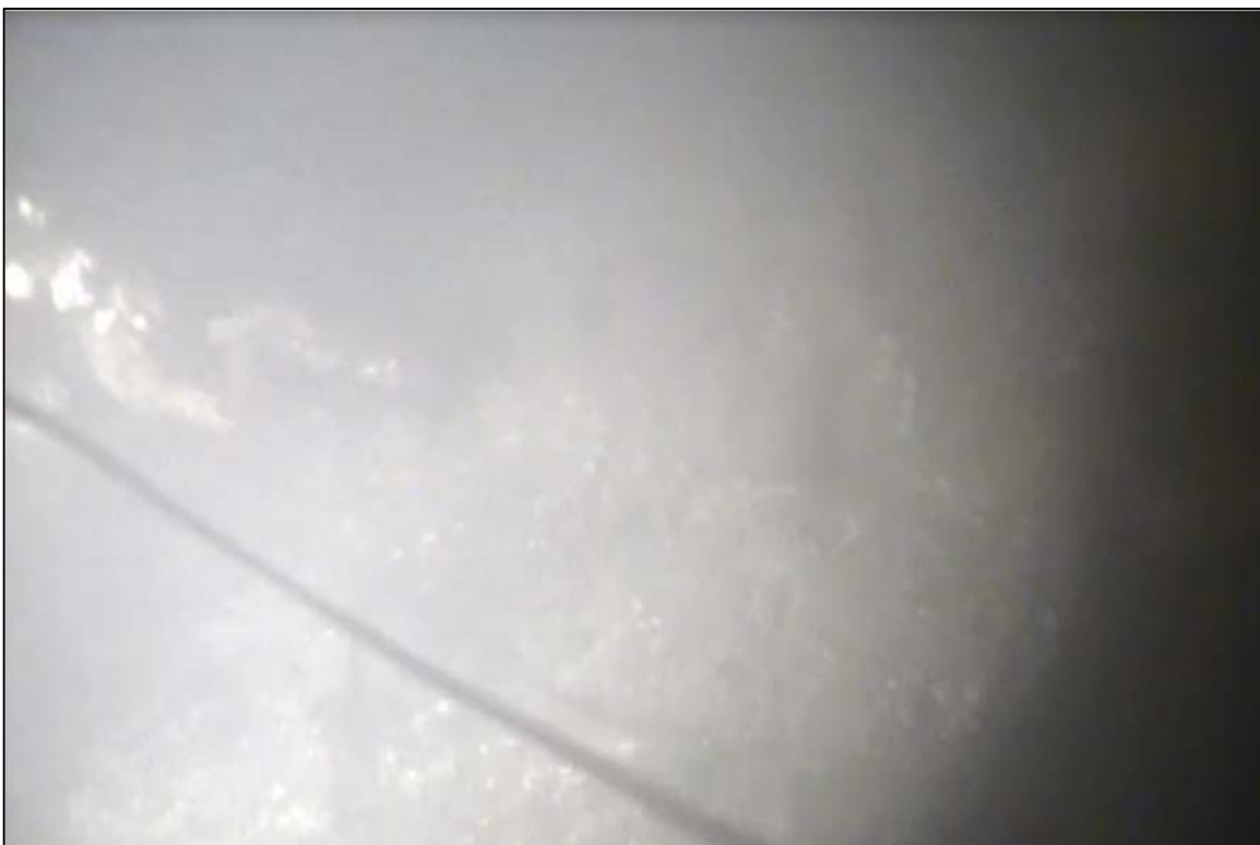
Photograph 40: View of Concrete Anchor Attached to Area of Severe Section Loss in Anchor Chain at Anchor 20, Looking South.
