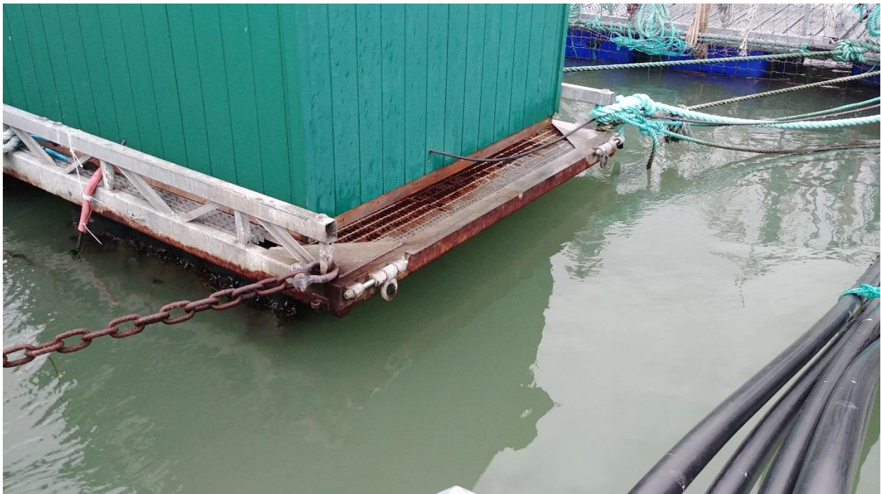
Figure C-75: Rusted chain and Barge Framing Members
