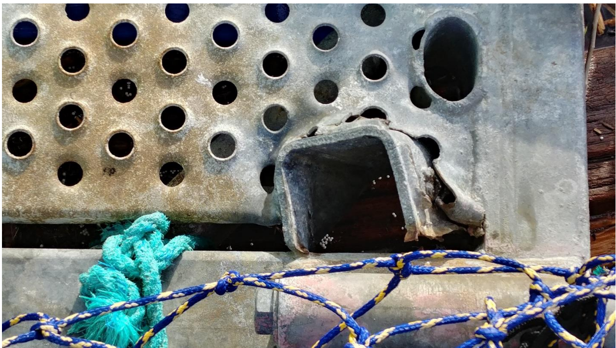
Figure C-109: Damaged Support Post Bracket
