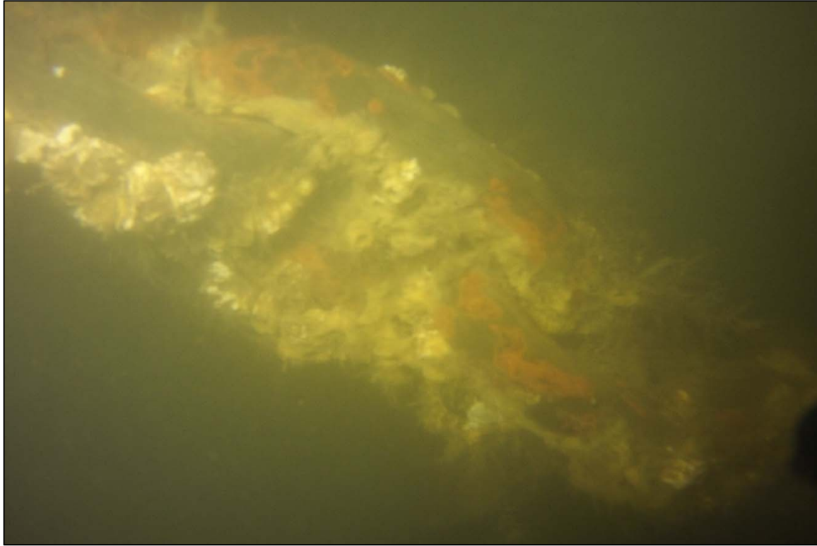
Photograph 25: View of Upper Anchor Chain Below Water at Anchor 21 (Typical), Looking West.
