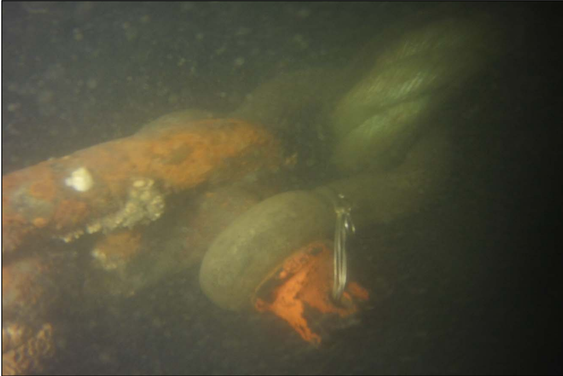
Photograph 27: View of Safety Wire Located on Upper Anchor Chain to Rope Connection (Thimble and Shackle) at Anchor 14 (Typical), Looking Northeast.
