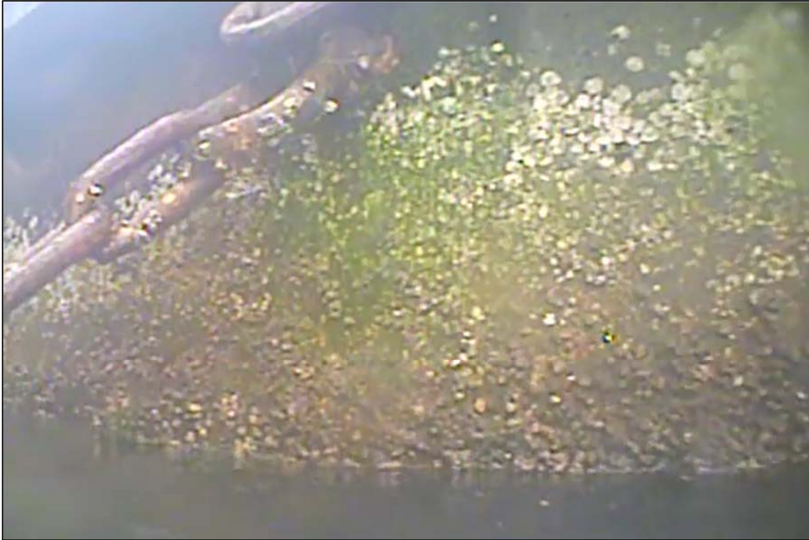
Photograph 21: View of the Typical Concrete Condition at the Waterline at the East Building Support Float, Looking East.
