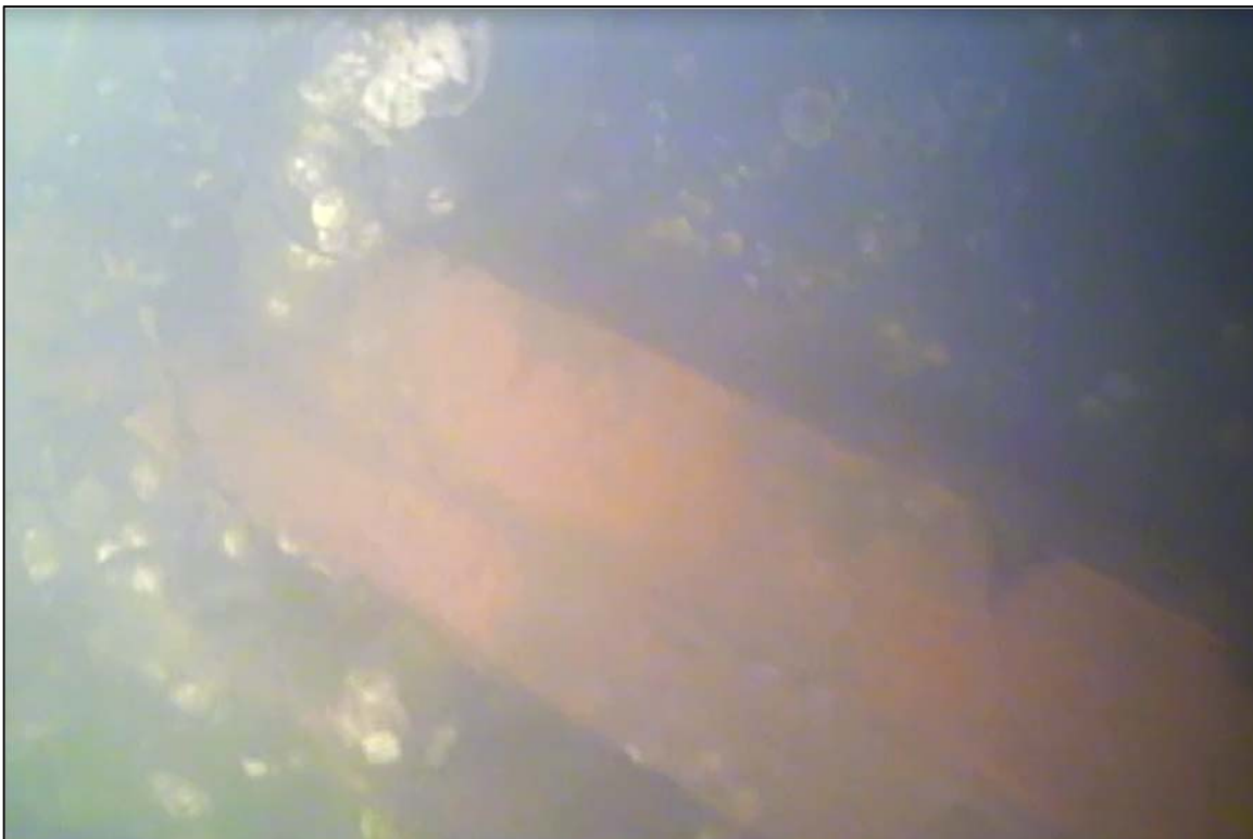
Photograph 16: View of the Southeast Corner Pen Support Float and Bracing Below Water, Looking Southeast.
