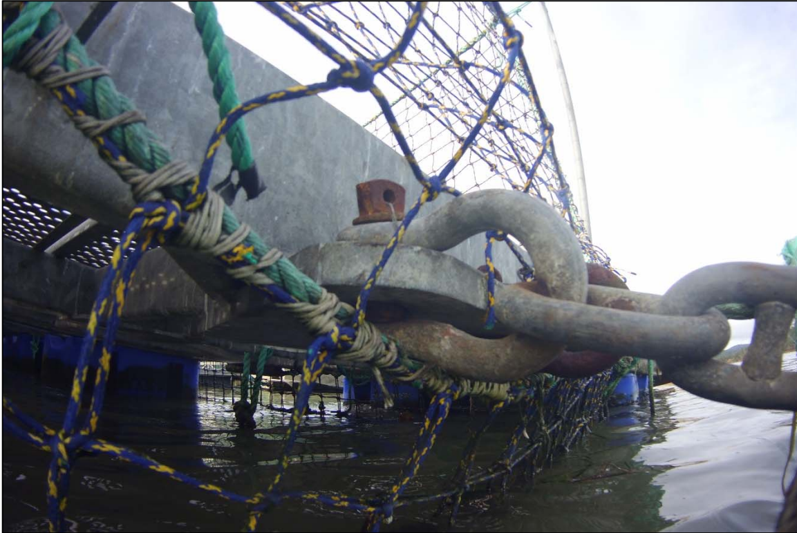
Photograph 23: View of Pen Support Float to Upper Anchor Chain Connection at Anchor 18 (Typical), Looking Northwest.
