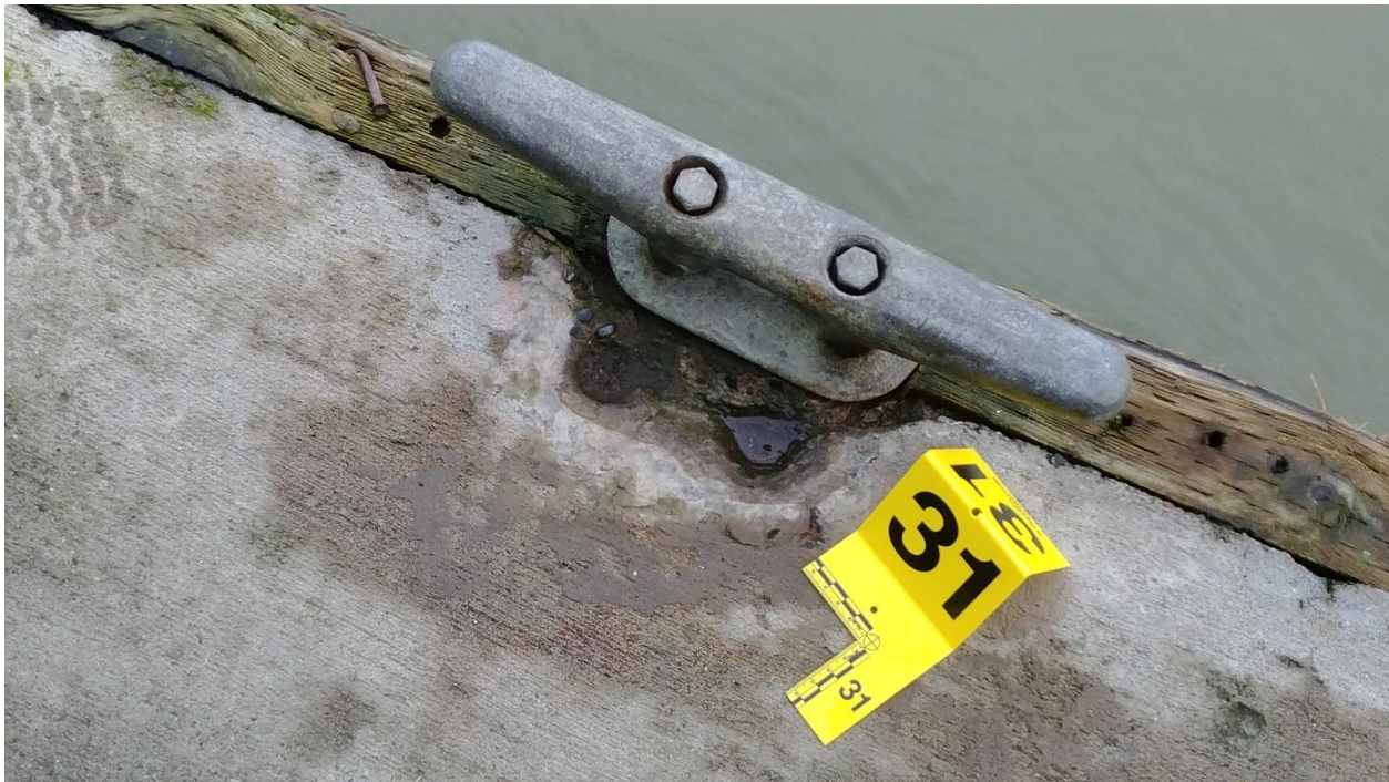
Figure C-77: Mooring Cleat Removed from its Original Location and Reattached into the Timber Waler
