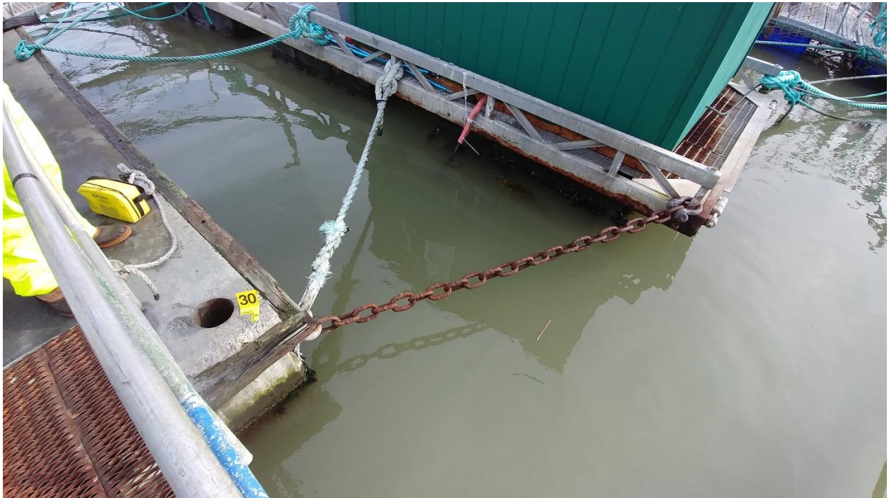
Figure C-74: Rusted chain and Barge Framing Members
