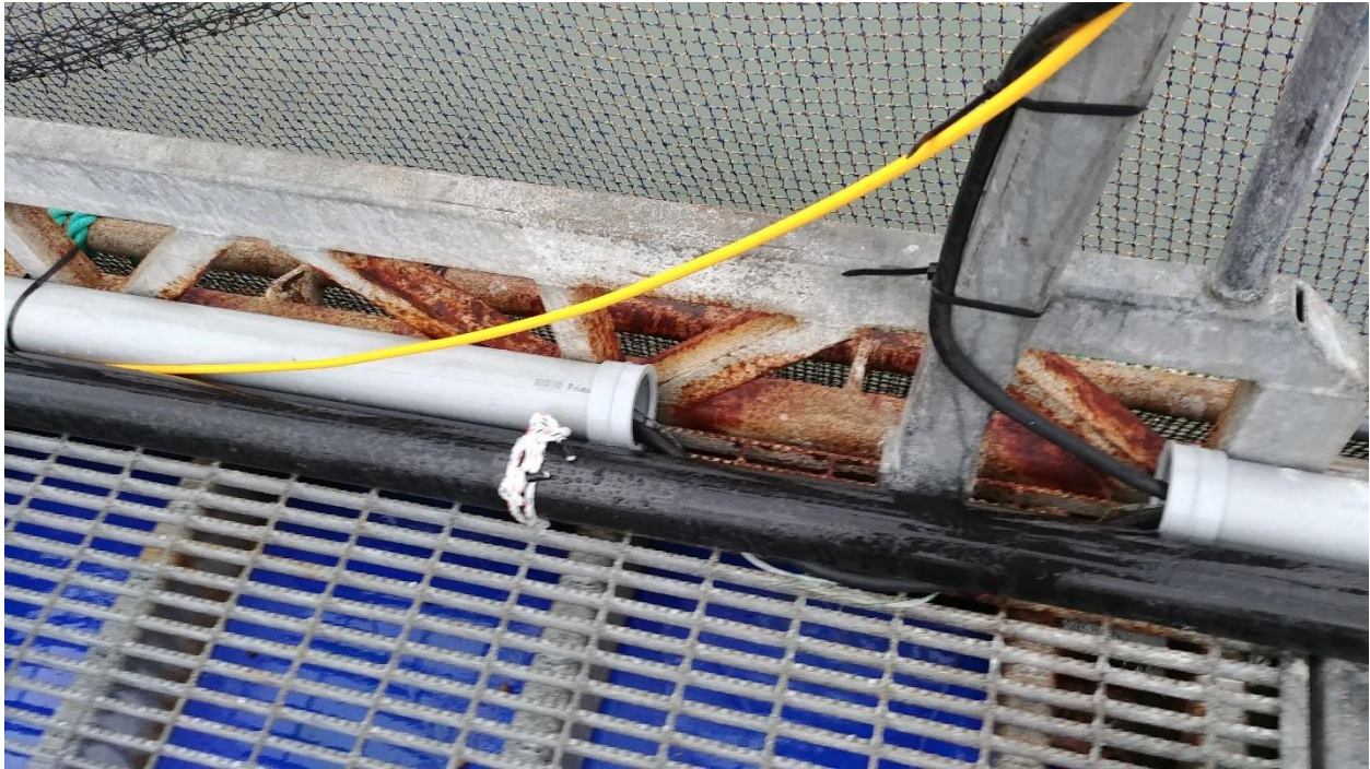
Figure C-110: Moderate Corrosion of Central Walkway Bullrail
