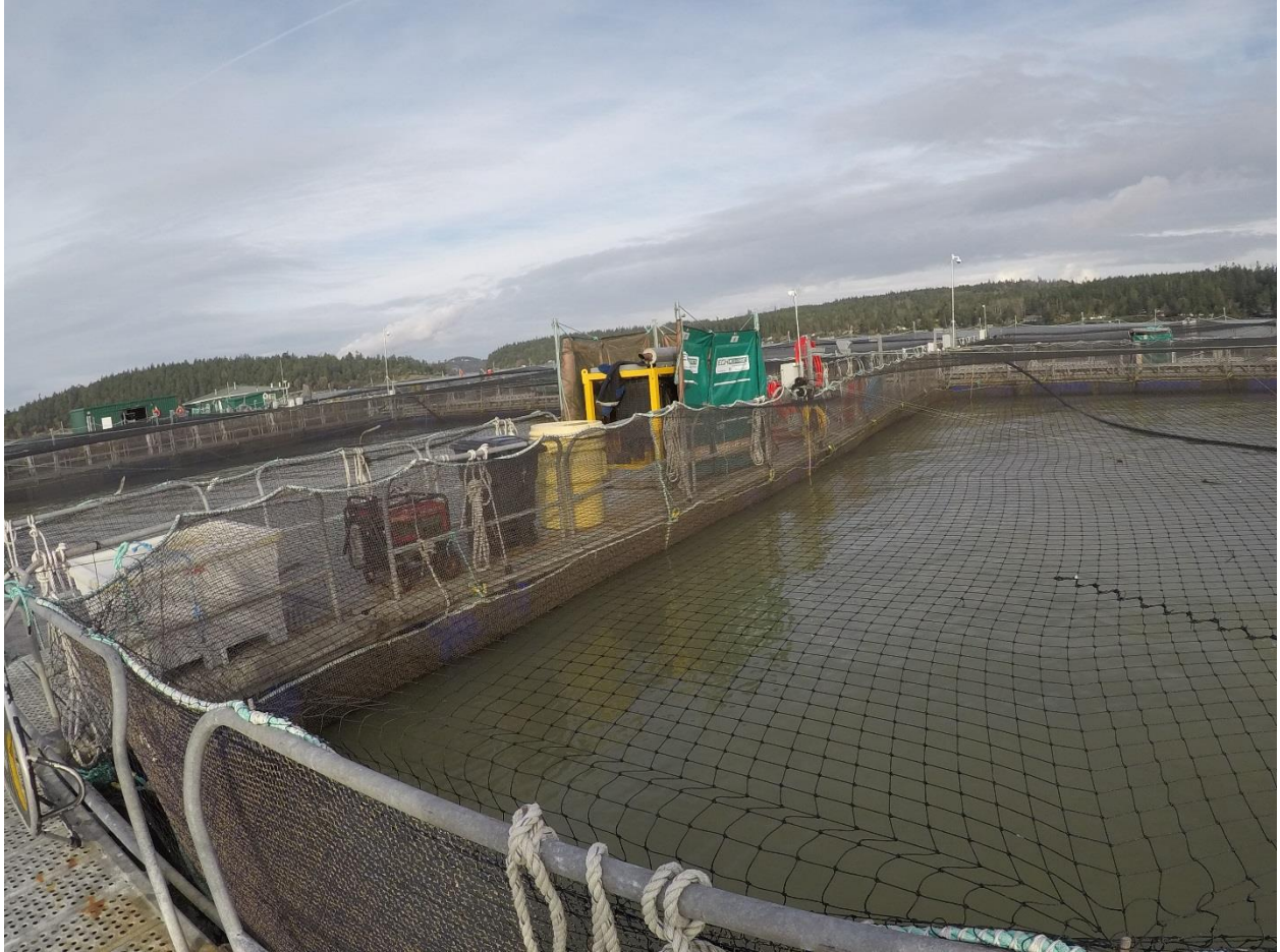
Figure C-116: Assorted Equipment is Causing Connecting Walkway to Deflect
