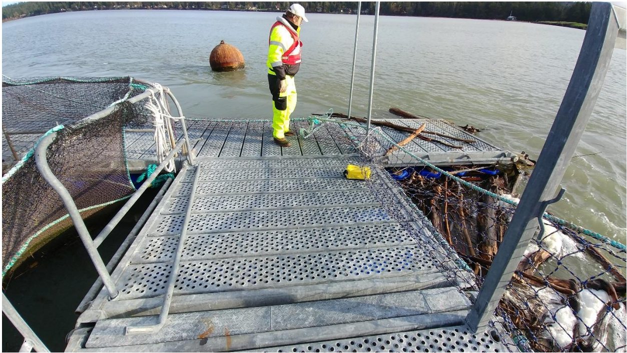
Figure C-12: Hope Island Net Pens - SE Corner, Inadequate Flotation
