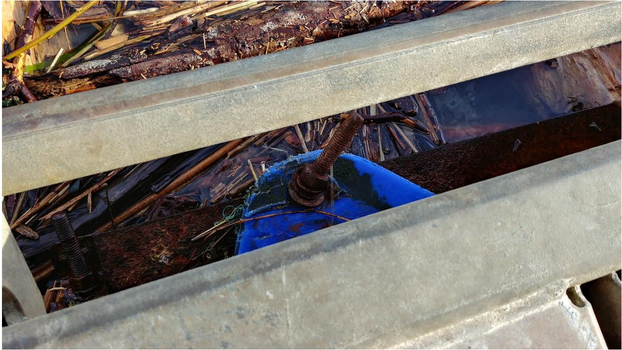
Figure C-108: Majorly Corroded Bolt and Steel Framing Connecting Float Tub
