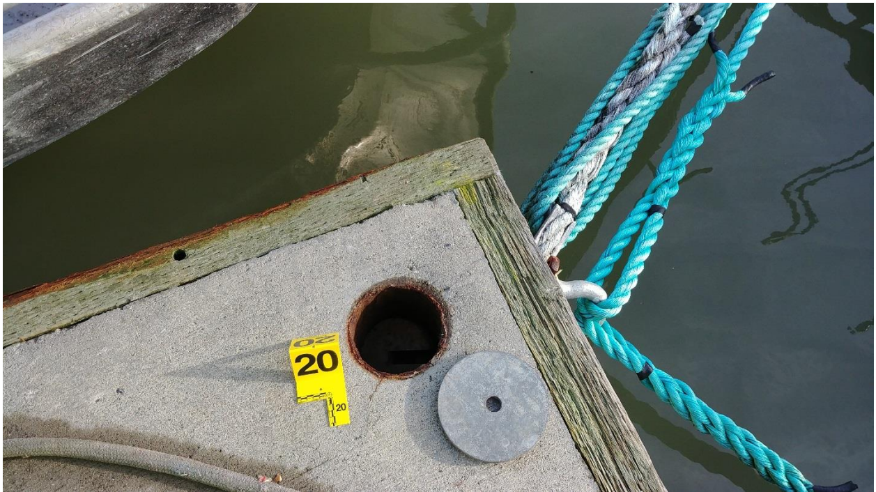
Figure C-57: Anchor #20, SE Corner of the Main Barge. Part of an Anchor Bridle System.
