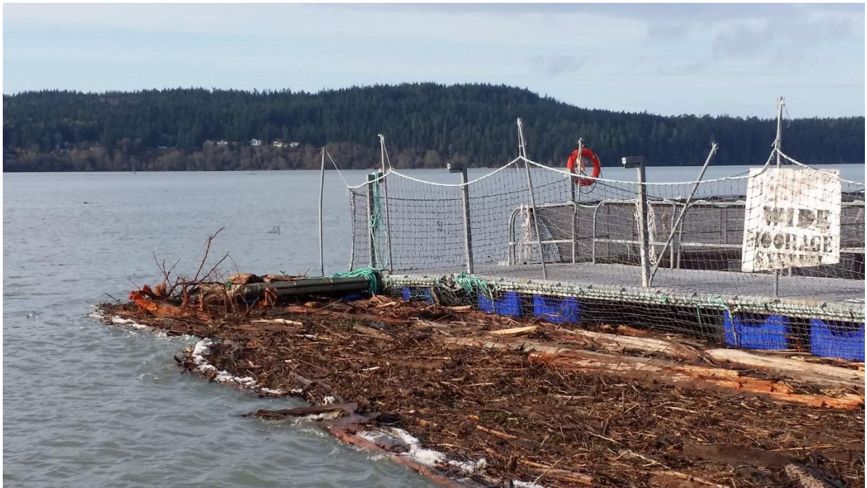
Figure C-15: Hope Island Net Pens - Debris Buildup on South End, Looking West
