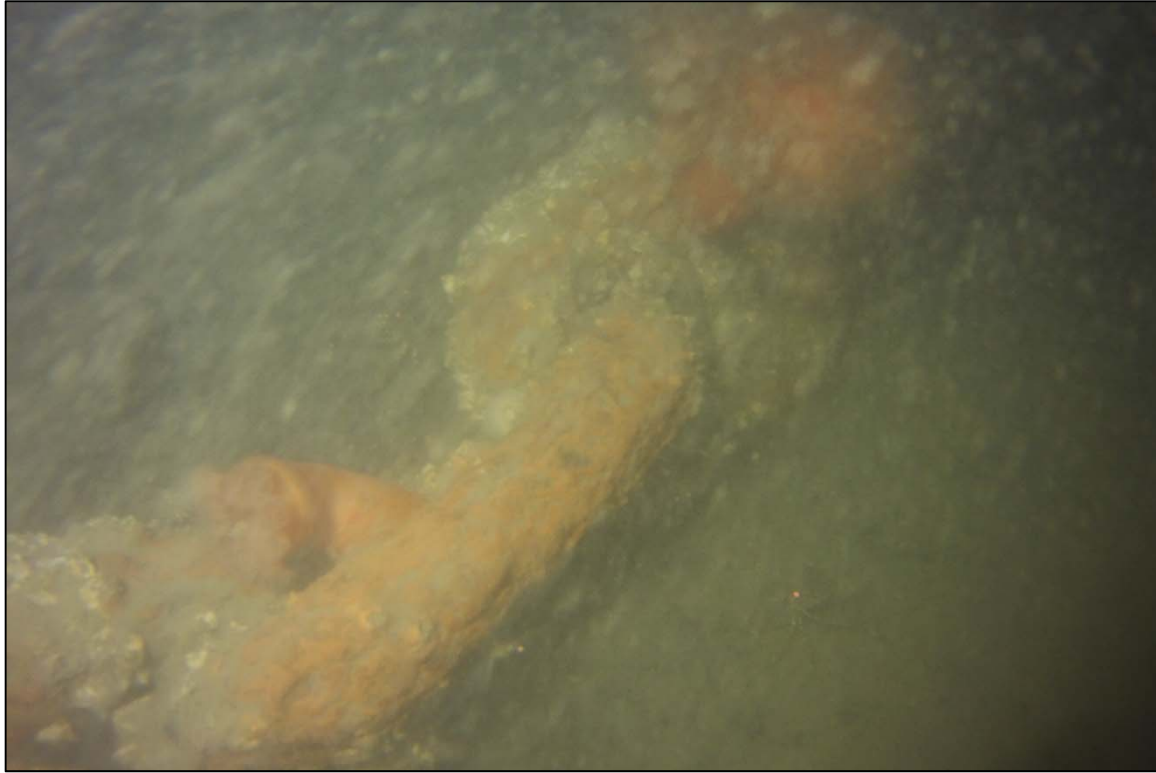
Photograph 41: View of Lower Anchor Chain on Channel Bottom at Anchor 22, Looking Northwest.
