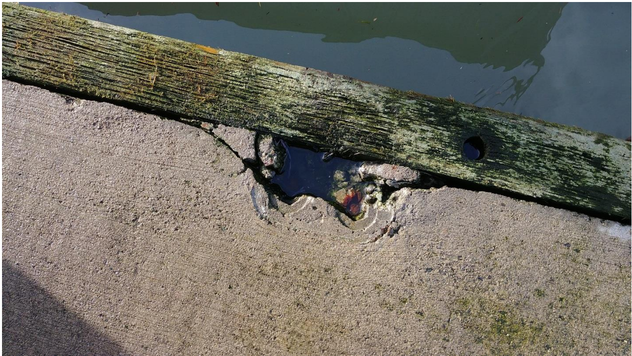
Figure C-79: Mooring Cleat has been Torn Out and is Missing
