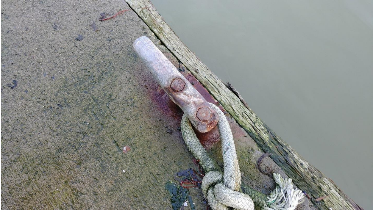
Figure C-78: Horn on Mooring Cleat Has Sheared Off at the Bolt
