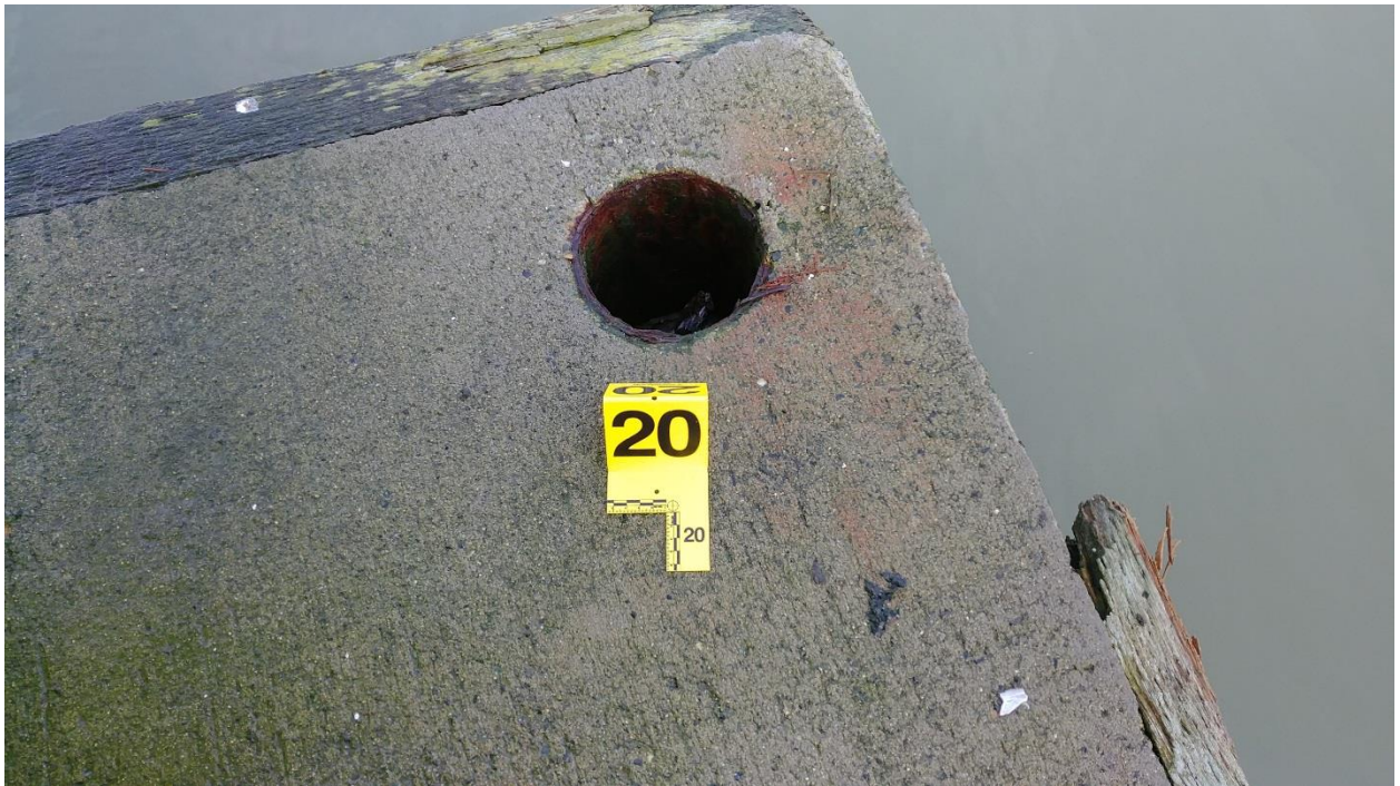
Figure C-59: Anchor #20, NE Corner of the Main Barge. Part of an Anchor Bridle System.
