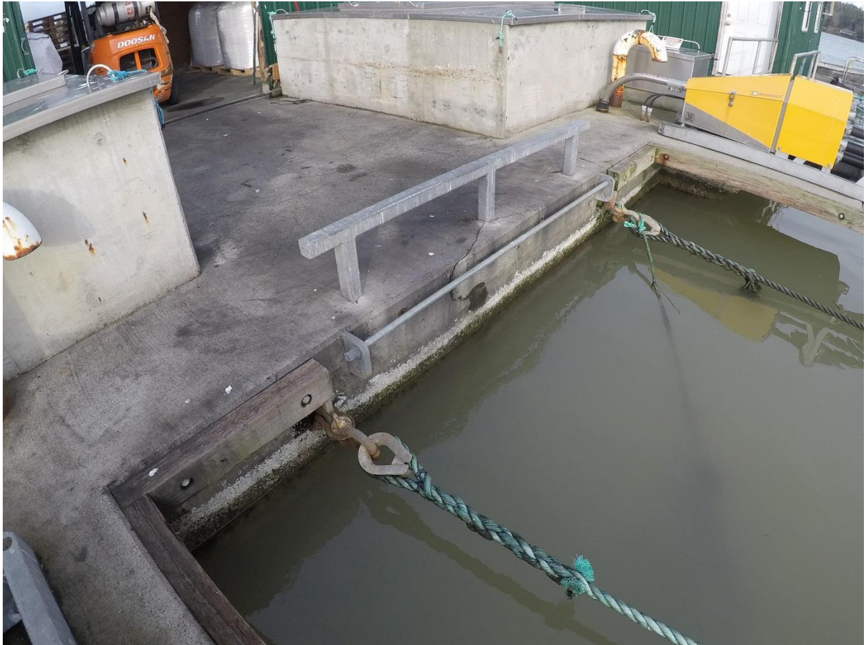
Figure C-82: Concrete on South Side of Feed Barge is Cracked and Nearly Spalling Off
