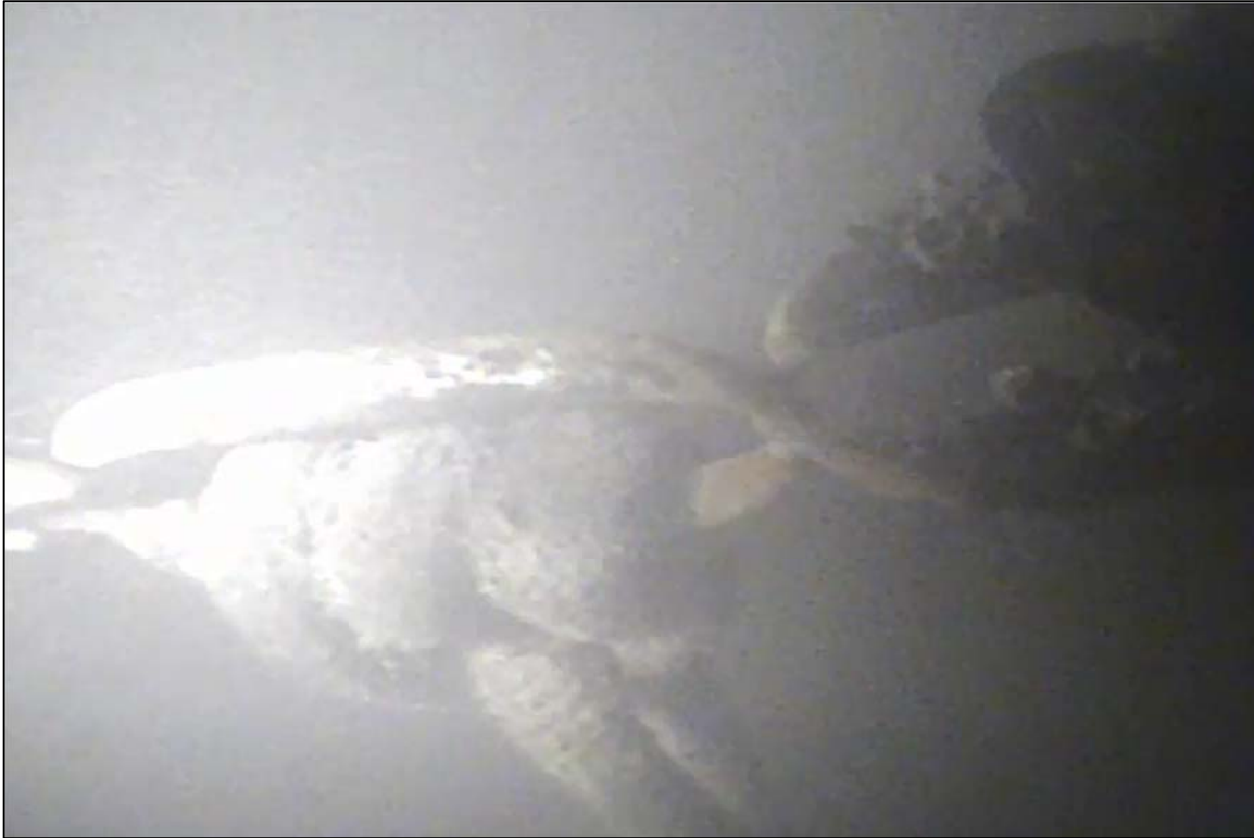
Photograph 39: View of Severe Section Loss in the Anchor Chain at Anchor 20, Looking South.
