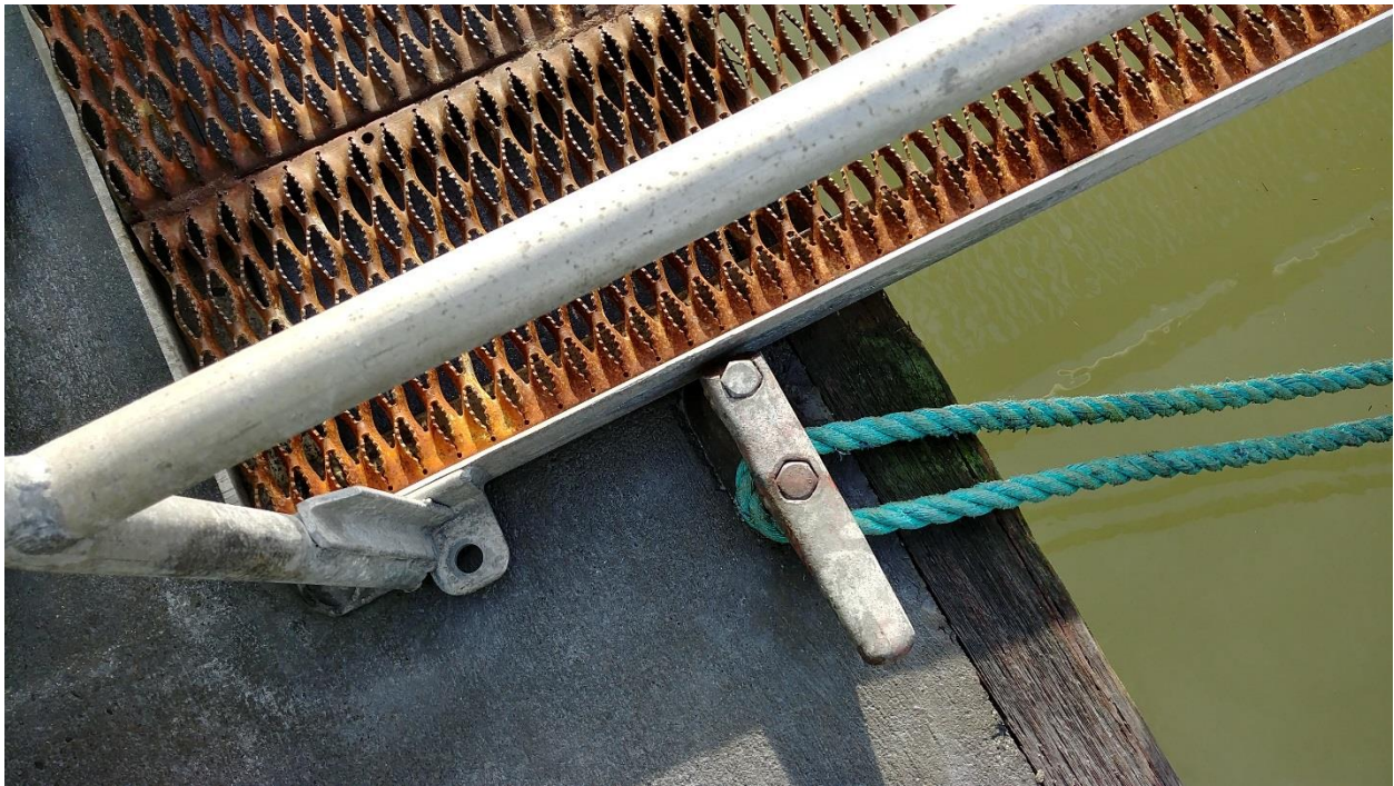
Figure C-80: Horn on Mooring Cleat Has Sheared Off at the Bolt.
