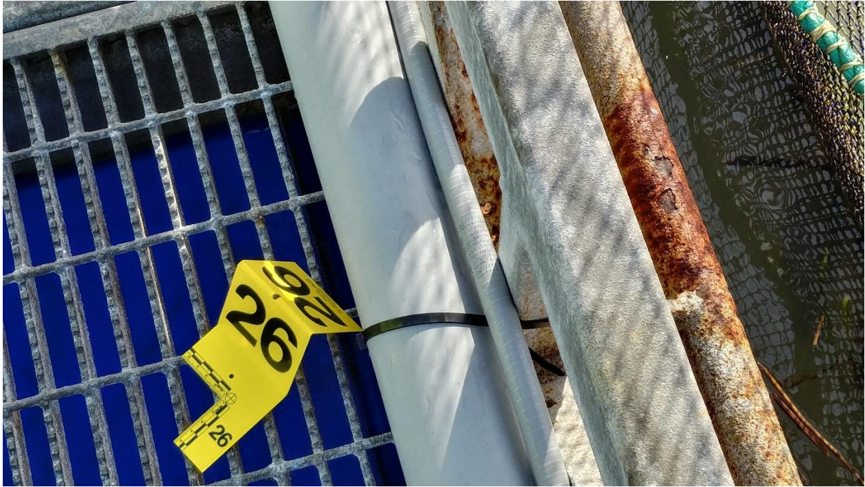
Figure C-70: Moderate Corrosion of
