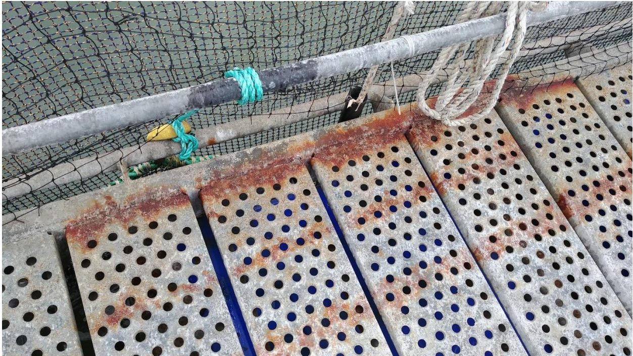
Figure C-112: Minor Corrosion of Steel Walkway Grating, Due to Fish Splash Back
