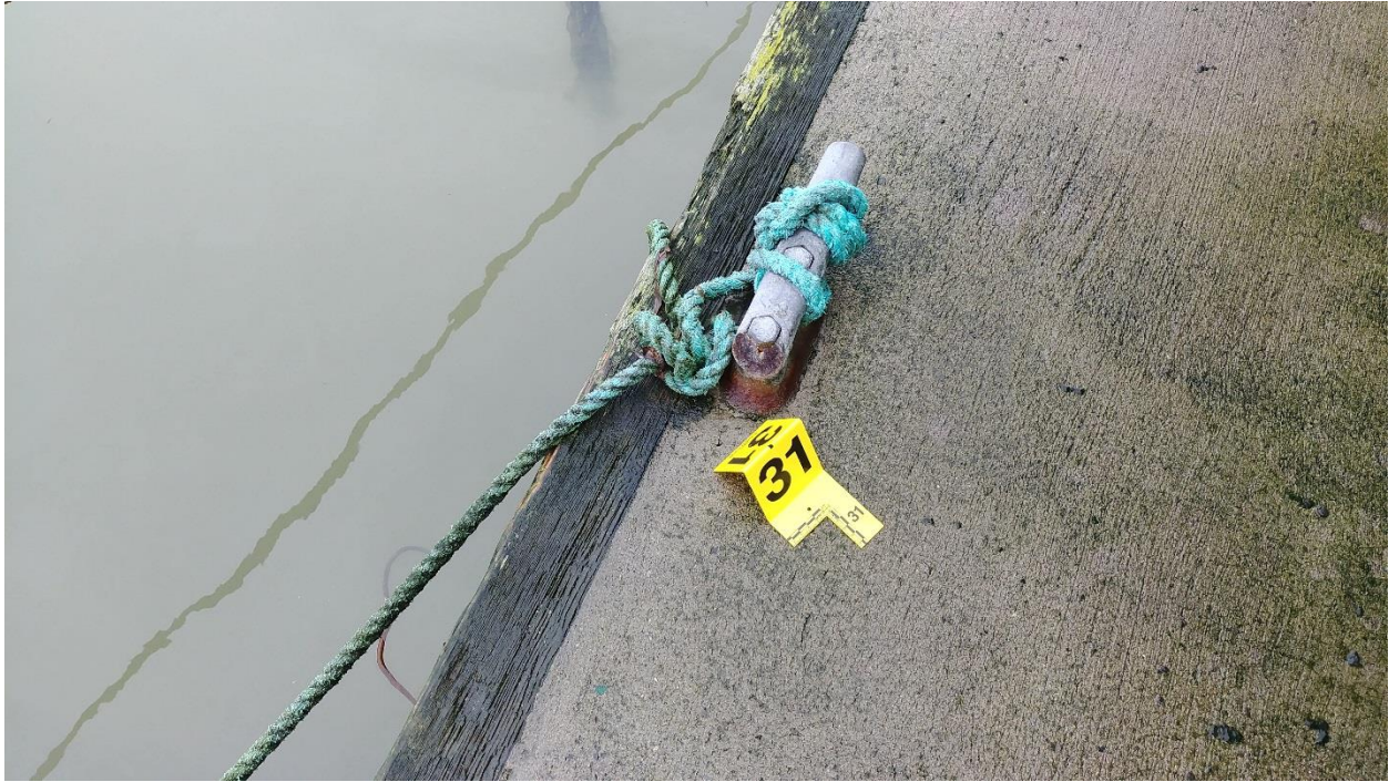
Figure C-76: Horn on Mooring Cleat Has Sheared Off at the Bolt
