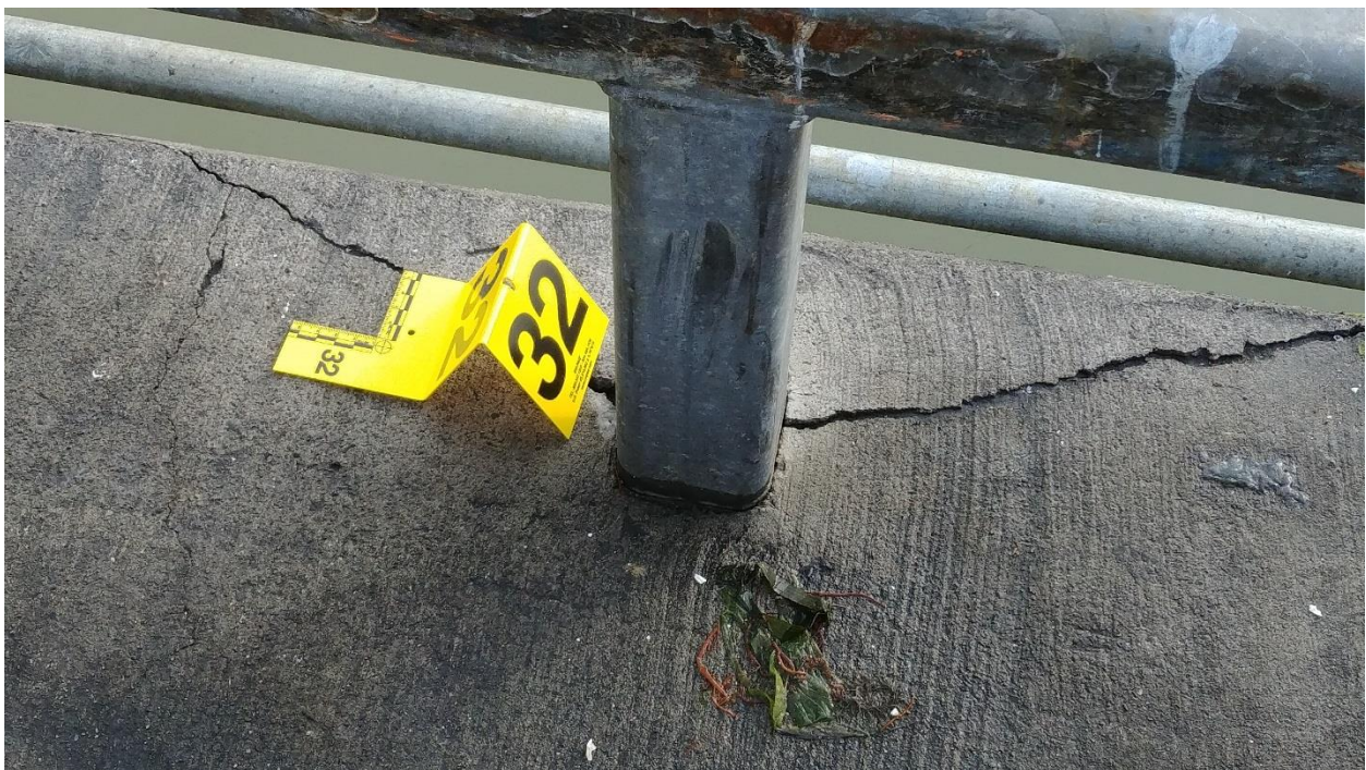
Figure C-81: Concrete on South Side of Feed Barge is Cracked and Nearly Spalling Off
