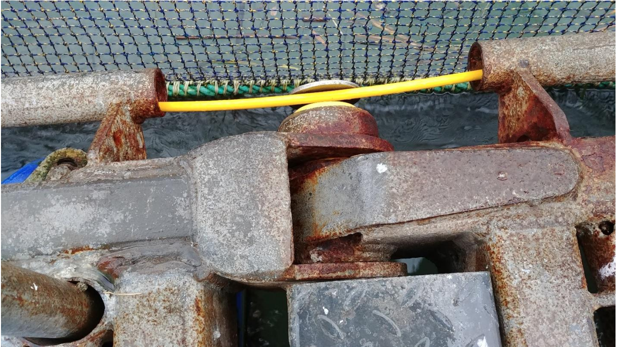
Figure C-106: Minor Corrosion of Walkway Hinge
