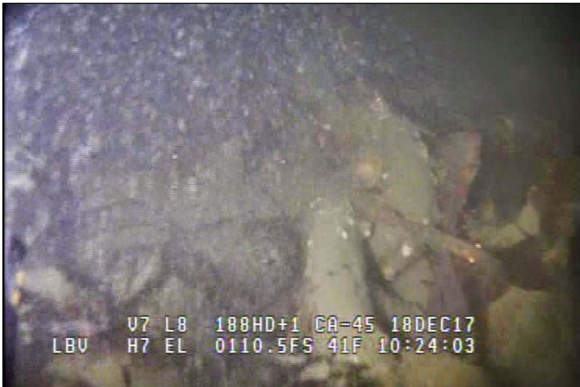
Photograph 44: View of the Lower Anchor Chain on the Channel Bottom at Anchor 1, Looking Southwest. Photo taken from an ROV.
