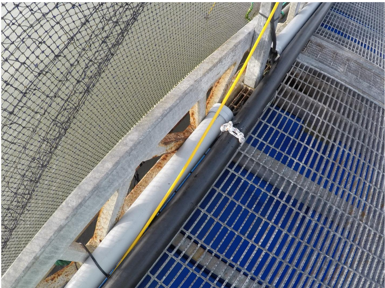
Figure C-111: Minor Corrosion of Central Walkway Bullrail
