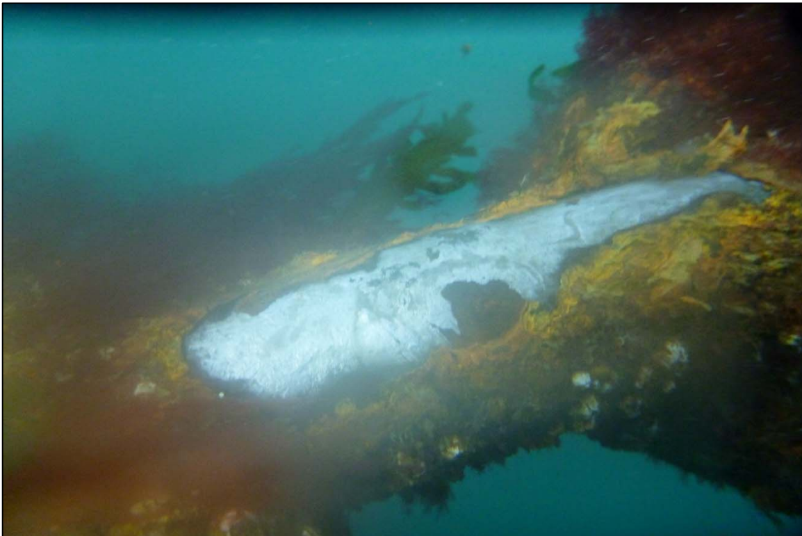
Photograph 54: View of the Light Surface Corrosion on the Upper Anchor Chain at Site 1 Anchor Chain 15, Looking North.
