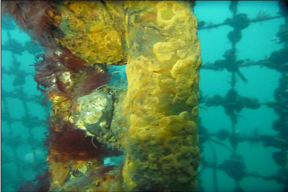
Photograph 35: View of Moderate Corrosion in the Buoy Chain at Site 1 Anchor Chain 8, Looking East.
