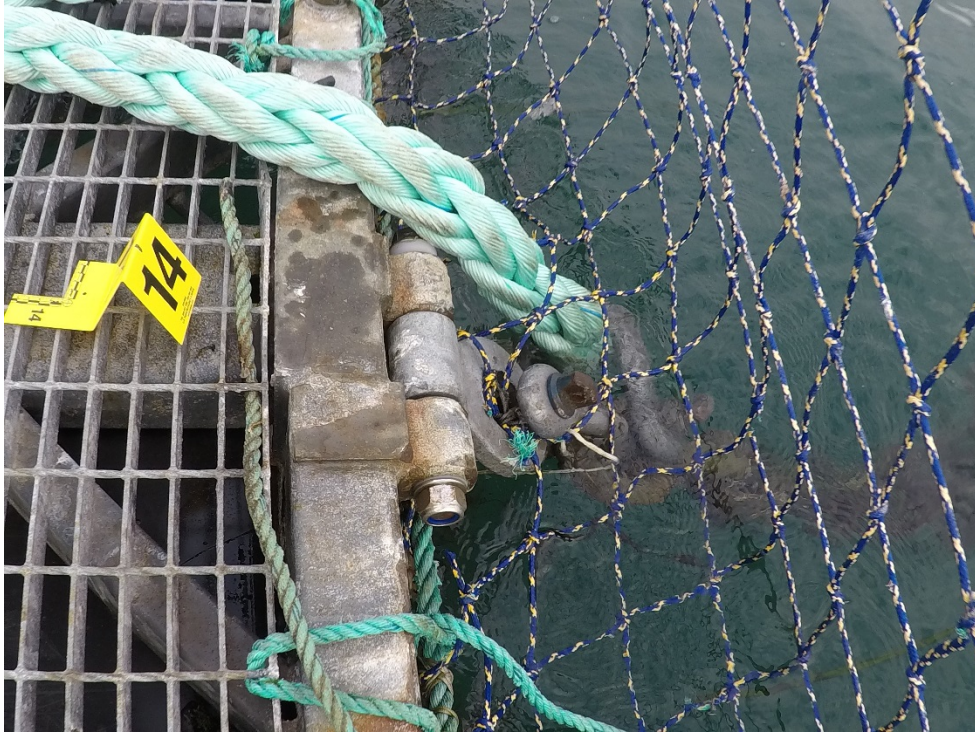
Figure C-13: Cypress Island Net Pen Site 1 – Connection at Anchor Line 14
