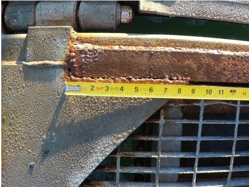
Figure C-26: Cypress Island Net Pen Site 1 – Crack in welded connection
