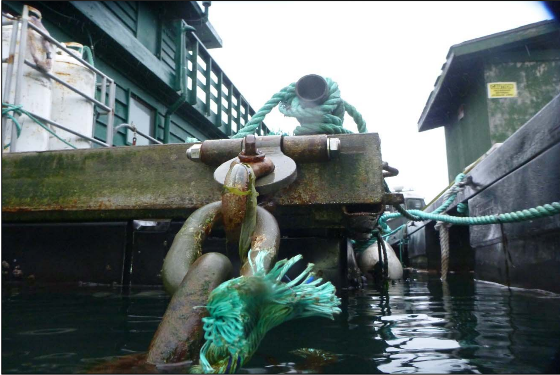
Photograph 13: View of the Float to Upper Anchor Chain Connection at Site 1 Anchor Line 1, Looking East.
