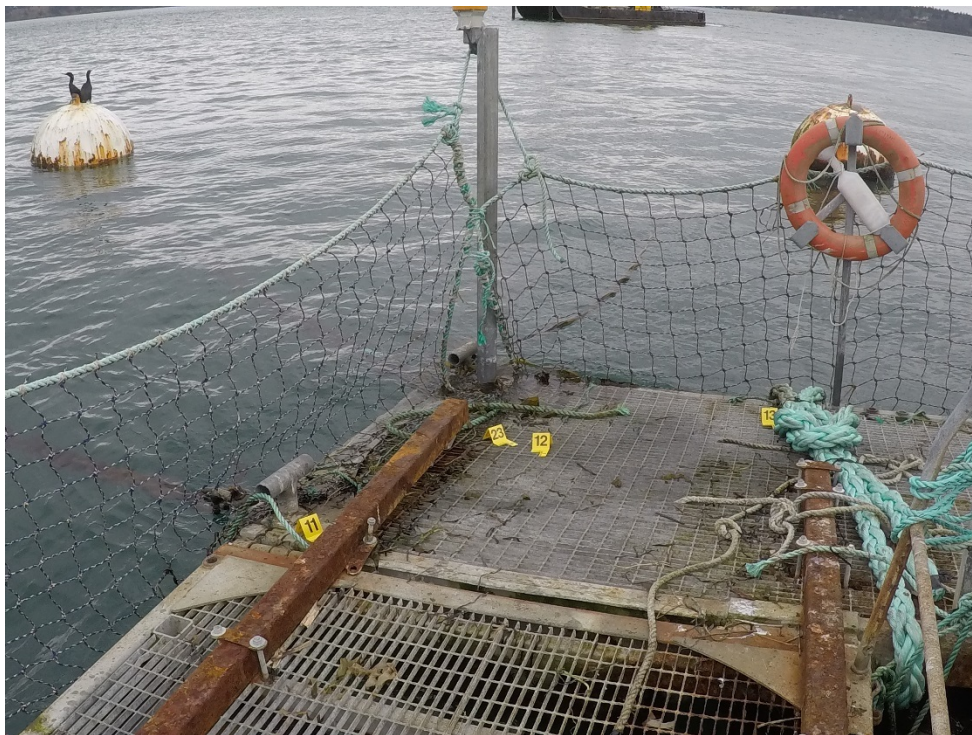
Figure C-12: Cypress Island Net Pen Site 1 – Northeast corner showing Anchor Lines 11, 12, 13, and 23 and inadequate flotation
