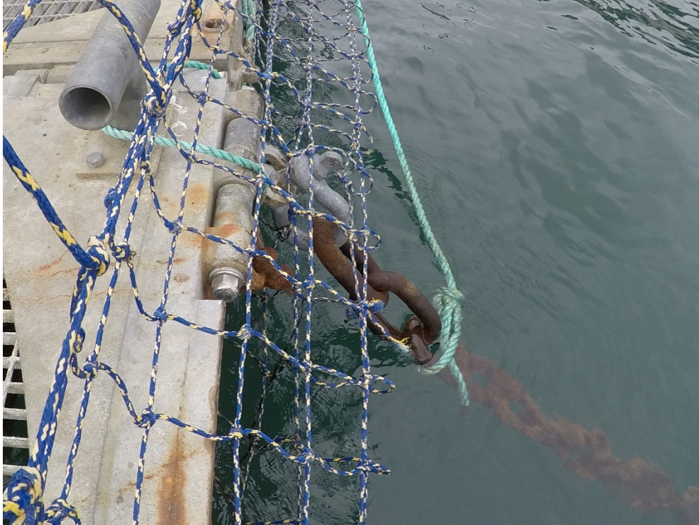
Figure C-11: Cypress Island Net Pen Site 1 – Connection at Anchor Line 10
