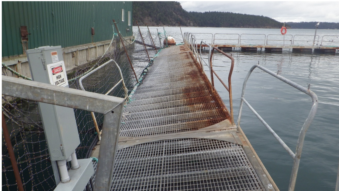
Figure C-20: Cypress Island Net Pen Site 1 – Severe listing of floats along west walkway
