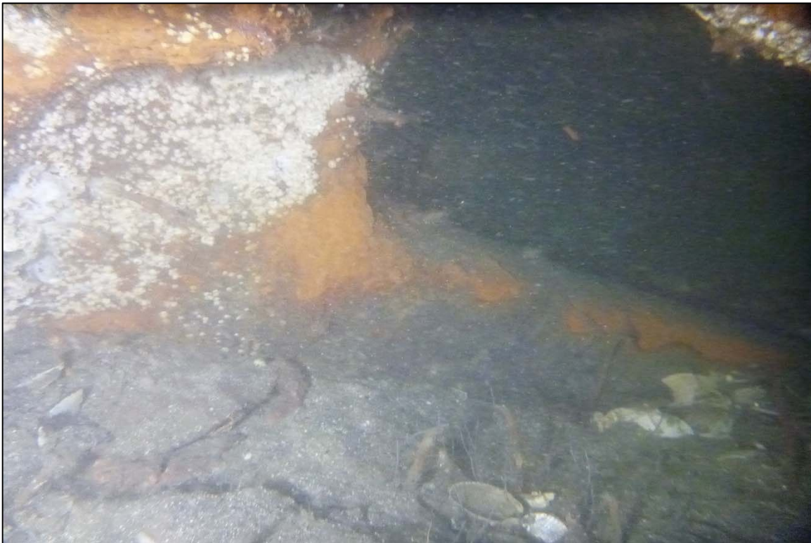
Photograph 34: View of the Anchor Embedment in the Channel Bottom at Site 1 Anchor Line 7, Looking East.
