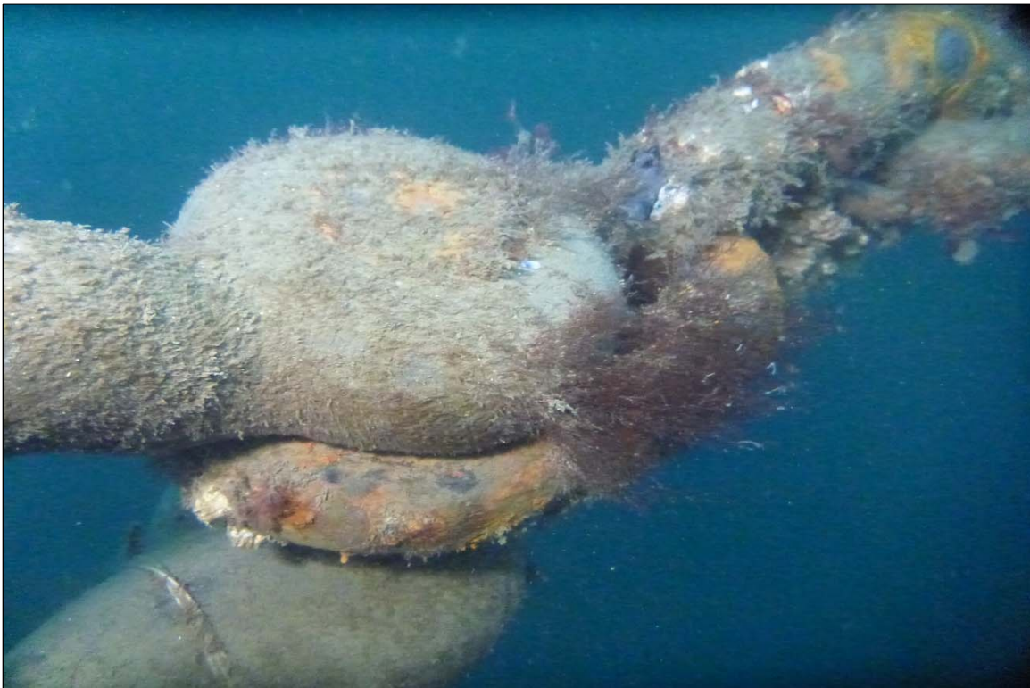
Photograph 28: View of the Upper Anchor Chain to Rope Connection (Shackle) at Site 1 Anchor Line 6, Looking North.
