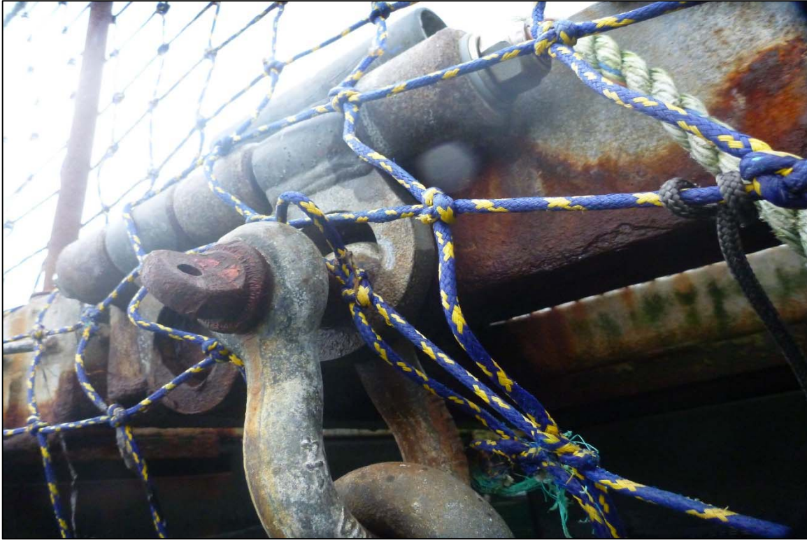
Photograph 41: View of Float to Upper Anchor Chain Connection at Site 1 Anchor Chain 10, Looking Southeast.
