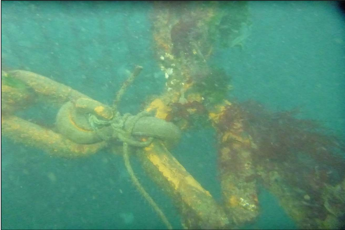
Photograph 75: View of the Upper Anchor Chain to Rope Connection (Thimble and Shackles) at Site 1 Anchor Chain 22, Looking North.
