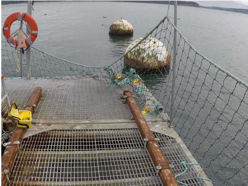
Figure C-15: Cypress Island Net Pen Site 1 – Southeast corner showing Anchor Lines 16, 17, and 18 and inadequate flotation
