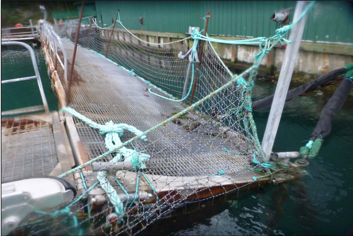
Photograph 7: View of the Uneven Walkway at the Northwest Corner of Site 1 Fish Net Pens System, Looking South.
