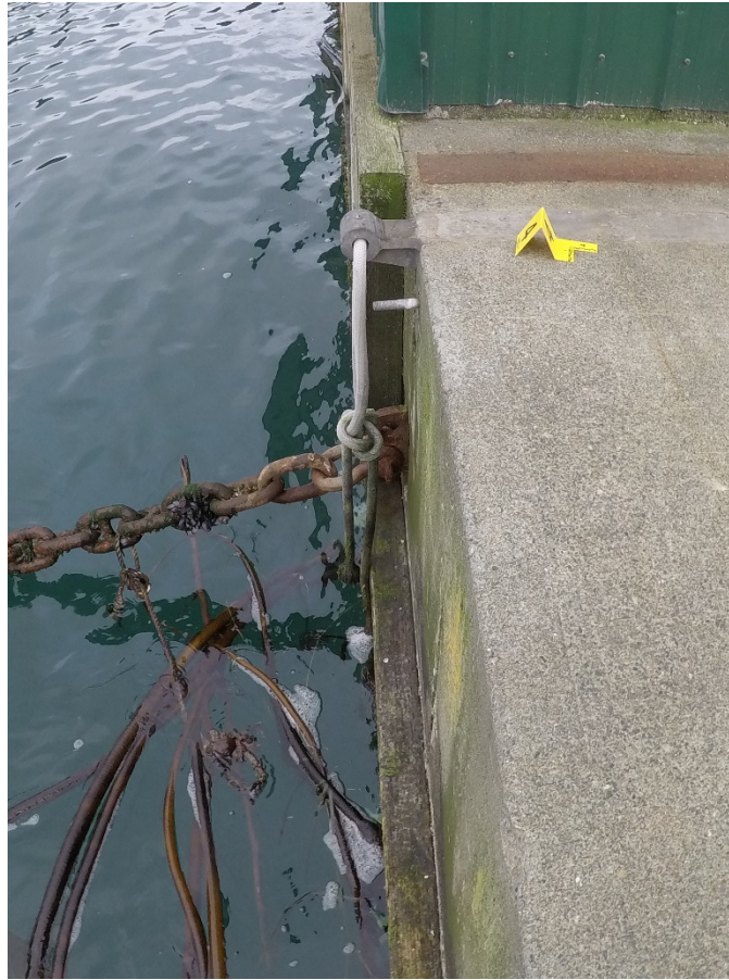
Figure C-7: Cypress Island Net Pen Site 1 – Anchor Line 4 at Concrete Barge
