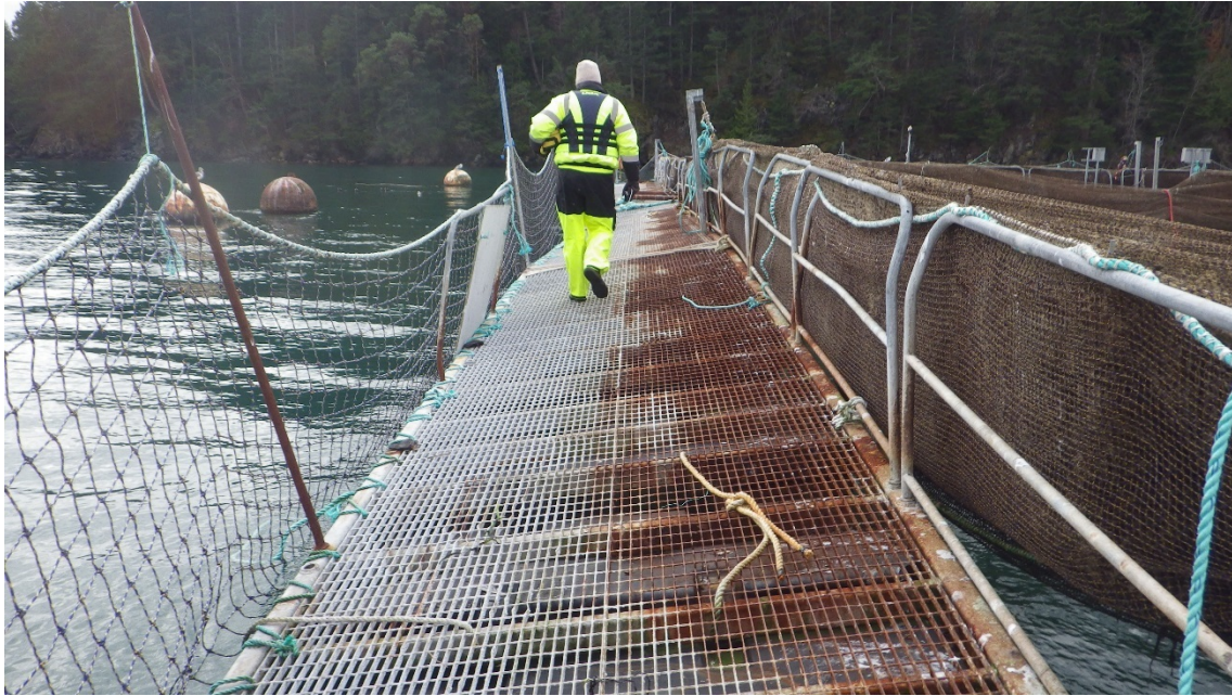
Figure C-22: Cypress Island Net Pen Site 1 – Severe listing of floats along east walkway
