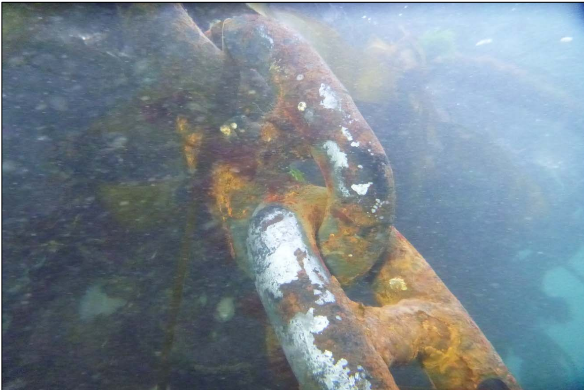
Photograph 50: View of Light Surface Corrosion Upper Anchor Chain at Site 1 Anchor Line 13, Looking Northwest.
