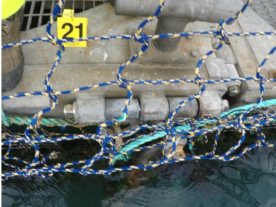
Figure C-18: Cypress Island Net Pen Site 1 – Connection at Anchor Line 21
