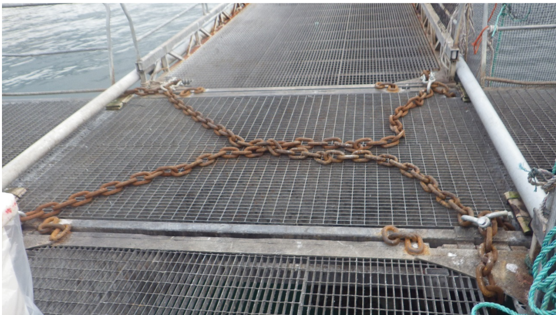
Figure C-23: Cypress Island Net Pen Site 1 – X-pattern chain repair to connect floats
