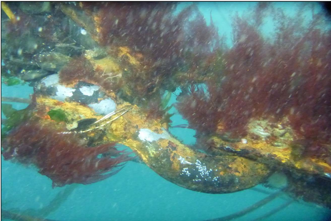
Photograph 44: View of Moderate Corrosion and Moderate Marine Growth on the Upper Anchor Chain to Rope Connection at Site 1 Anchor Line 11, Looking West.
