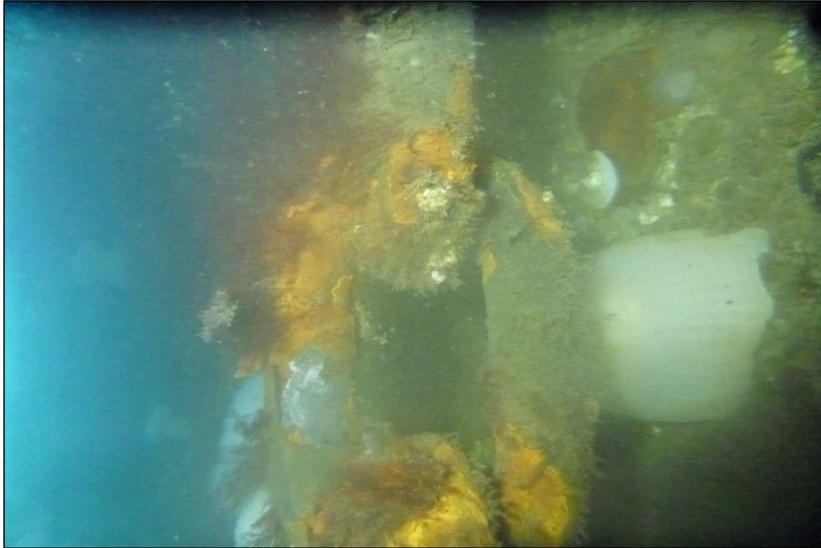
Photograph 9: View of the Severe Corrosion in the Upper Anchor Chain at Site 1 Feed Barge North Anchor Line, Looking East.
