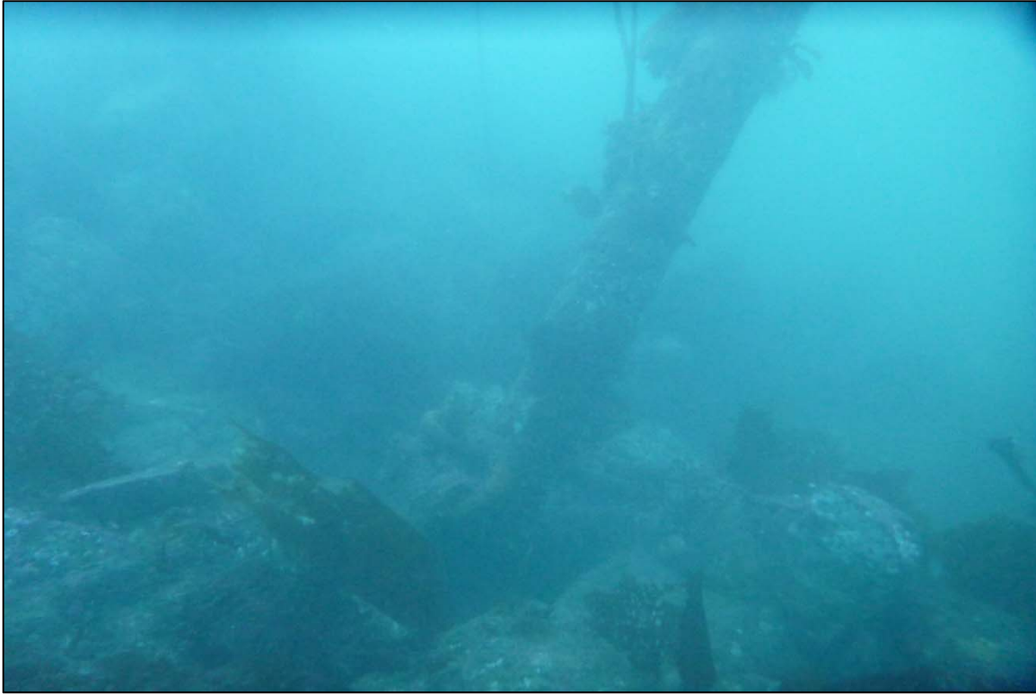
Photograph 71: View of the Tilt in the Pipe Anchor at Site 1 Anchor Line 20, Looking West.
