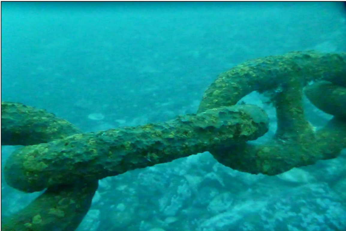
Photograph 70: View of Section Loss in the Lower Anchor Chain at Site 1 Anchor Chain 20, Looking East.
