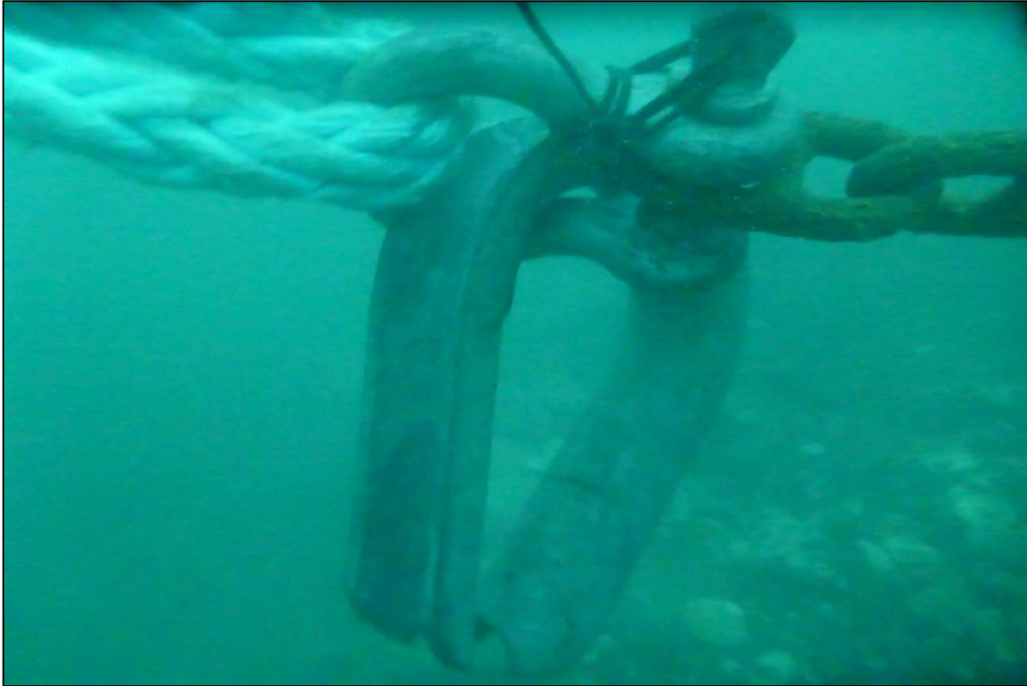
Photograph 69: View of the Failed Thimble at the Rope to Lower Anchor Chain Connection at Site 1 Anchor Line 20, Looking East.
