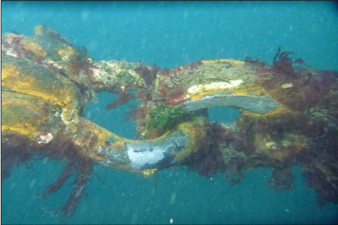
Photograph 61: View of the Upper Anchor Chain to Rope Connection (Shackle and Thimble) at Site 1 Anchor Chain 18, Looking North.
