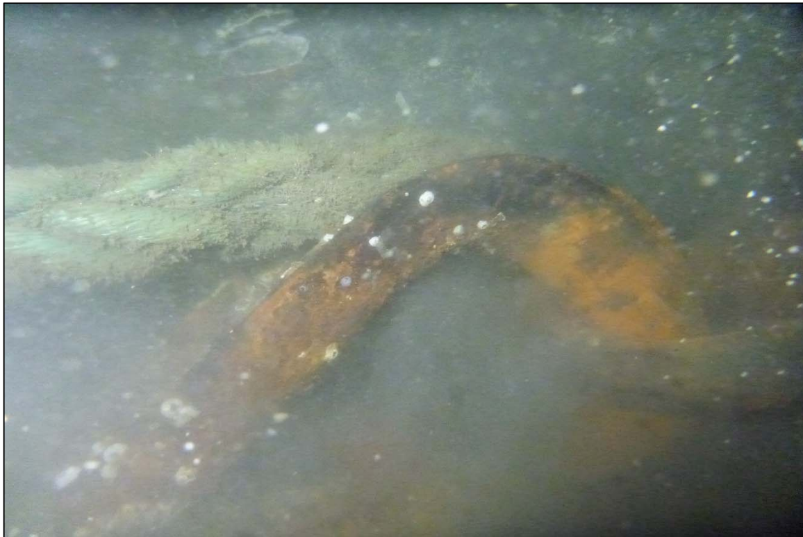
Photograph 32: View of the Loose Thimble at the Rope to Lower Anchor Chain Connection at Site 1 Anchor Line 7, Looking West.
