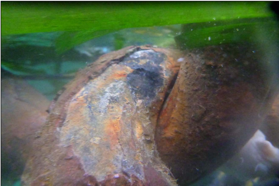
Photograph 68: View of Upper Anchor Chain at the Upper Connection with Corrosion and Pitting at Site 3 Anchor Line 20, Looking East.
