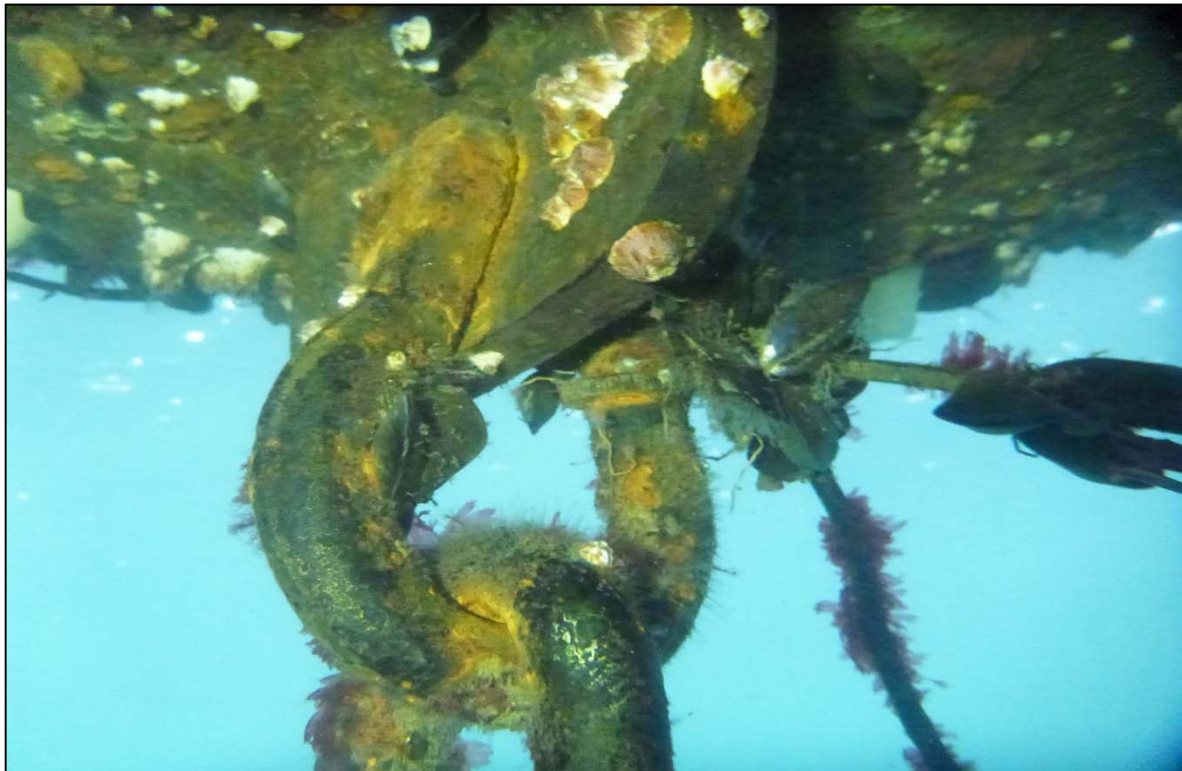
Photograph 34: View of Chain to Buoy (Shackle) at Fort Ward Anchor Line 7, Looking Southeast.
