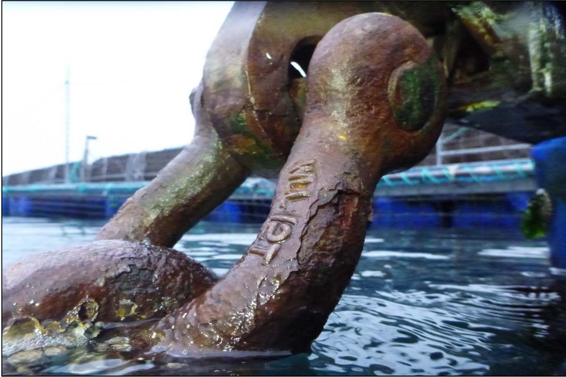
Photograph 21: View of Upper Chain to Float Connection Section Loss and Corrosion at Site 3 Anchor Line 4, Looking East.
