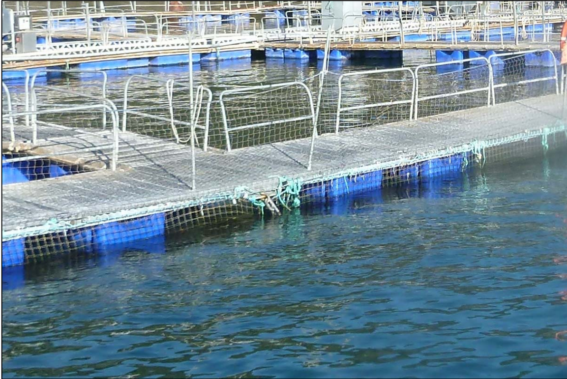
Photograph 9: View of Upper Anchor Chain to Float Connection at Site 3 Anchor Line 11, Looking Northeast.
