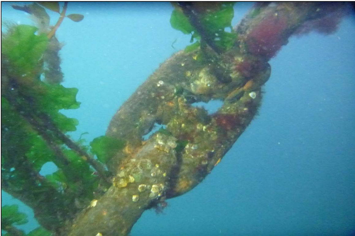
Photograph 22: View of Upper Chain with Marine Growth at Site 3 Anchor Line 4, Looking North.
