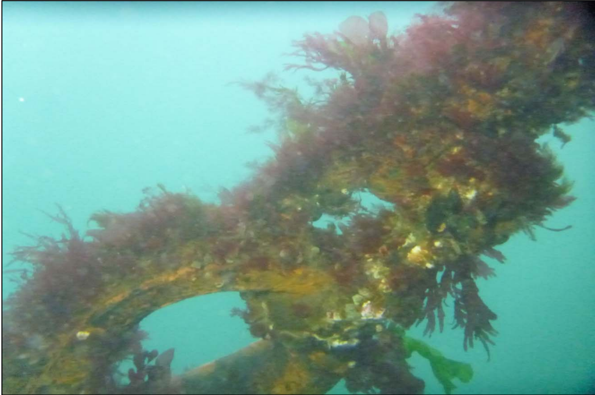
Photograph 13: View of Upper Anchor Chain to Anchor Rope Connection at Site 3 Anchor Line 1, Looking Northwest.
