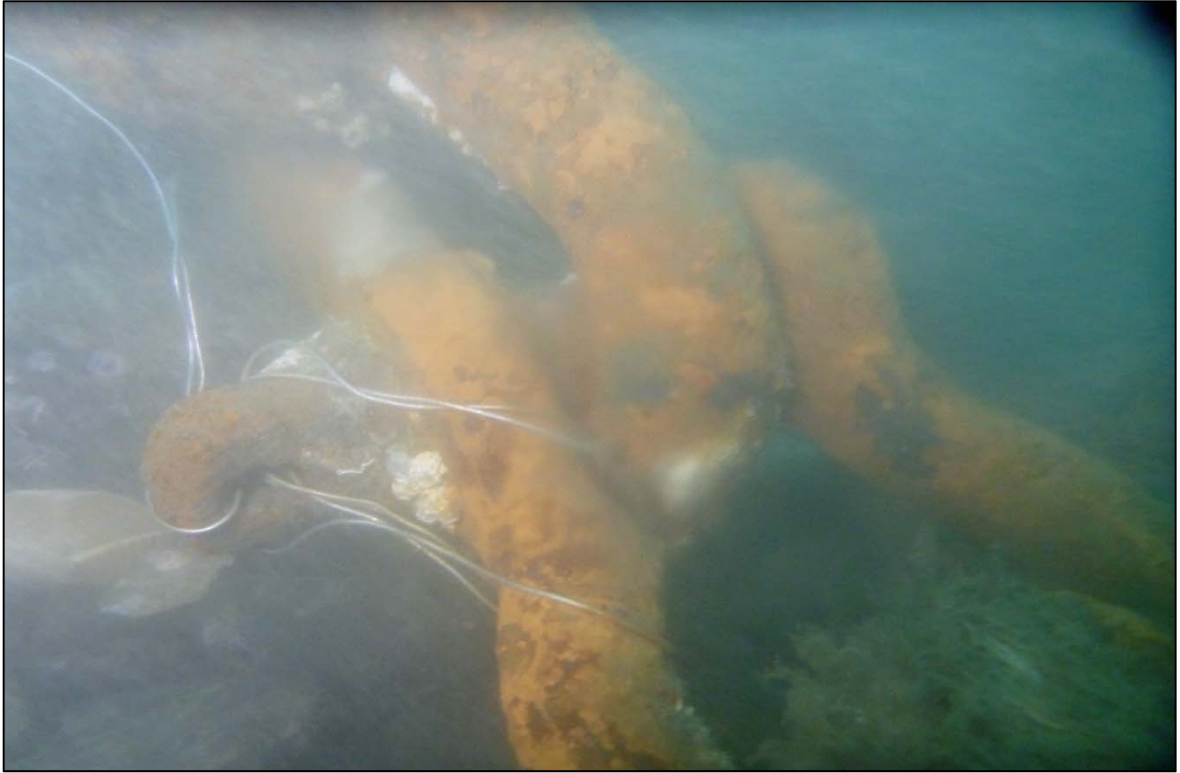
Photograph 79: View of Lower Anchor Chain to Anchor Rope Connection with Loose Safety Wire (Shackle) at Site 3 Anchor Line 24, Looking West.
