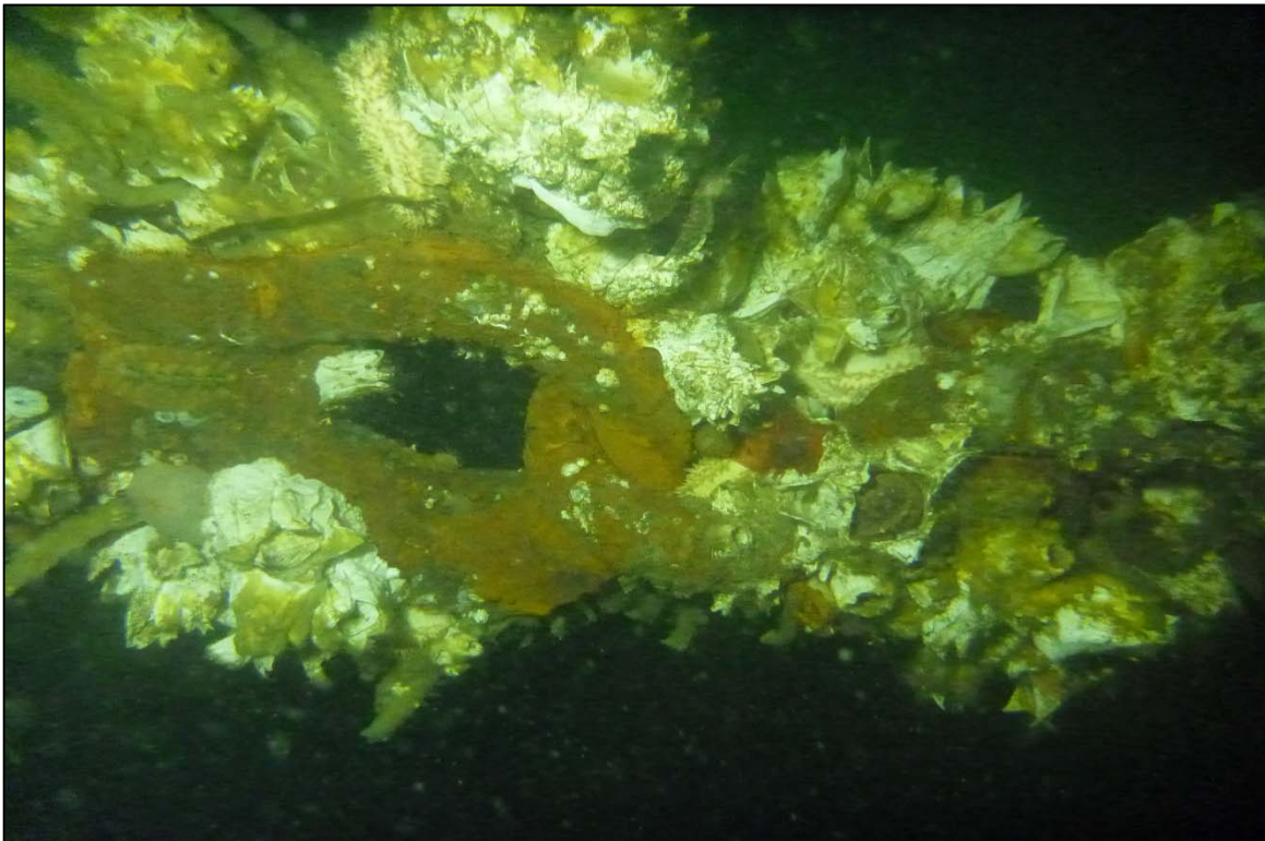
Photograph 72: View of Lower Anchor Chain to Anchor Rope Connection with Heavy Barnacle Growth (Thimble) at Site 3 Anchor Line 21, Looking Northeast.
