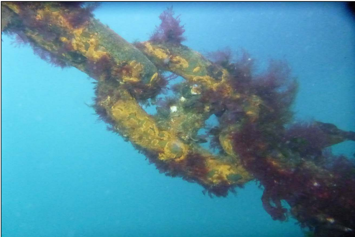
Photograph 12: View of Upper Anchor Chain Corrosion at Site 3 Anchor Line 1, Looking Northwest.
