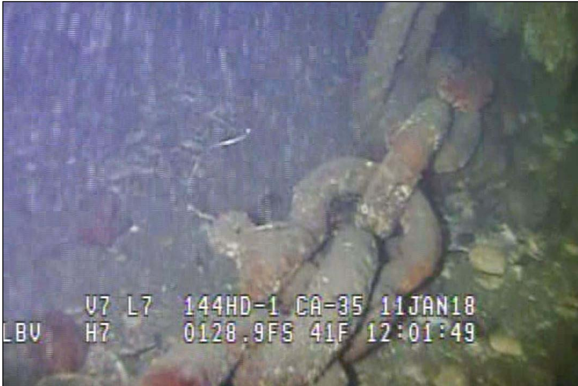
Photograph 23: View of Lower Chain to Chain Connection (Shackle) at Site 3 Anchor Line 4, Looking North.
