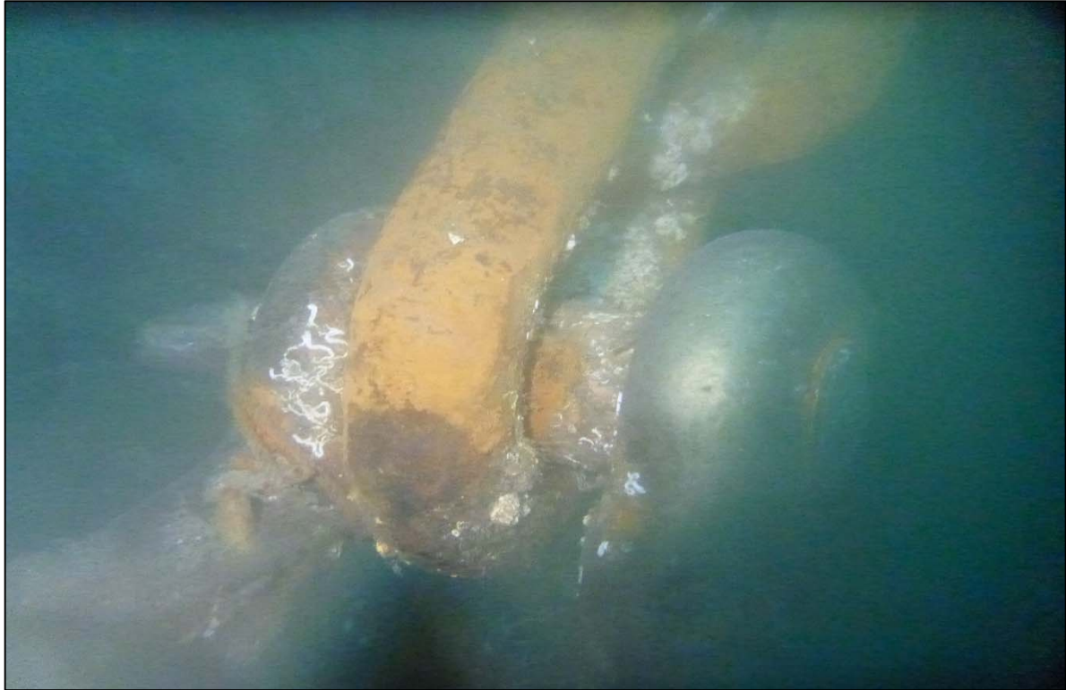
Photograph 83: View of Lower Anchor Chain to Anchor Rope Connection with Corrosion (Shackle) at Site 3 Anchor Line 27, Looking Northwest.
