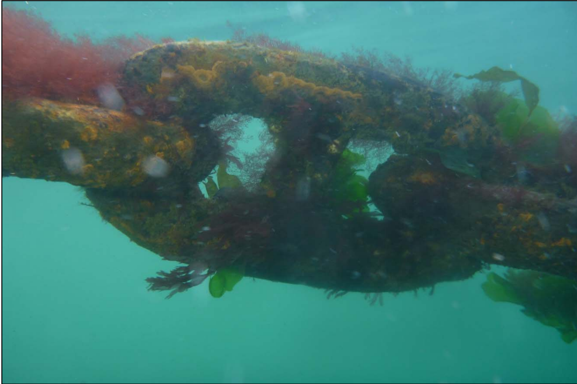
Photograph 55: View of Upper Anchor Chain Condition with Corrosion and Pitting at Site 3 Anchor Line 13A, Looking West.
