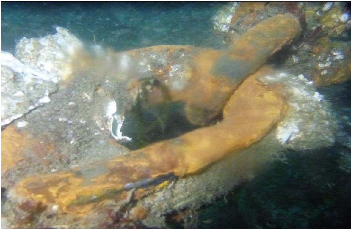
Photograph 82: View of Lower Anchor Chain to Anchor Rope Connection with Corrosion and Pitting (Thimble) at Site 3 Anchor Line 25, Looking Northwest.
