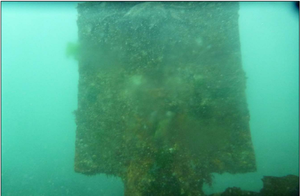
Photograph 80: View of Top of Anchor Pin at Site 3 Anchor Line 24, Looking Northwest.
