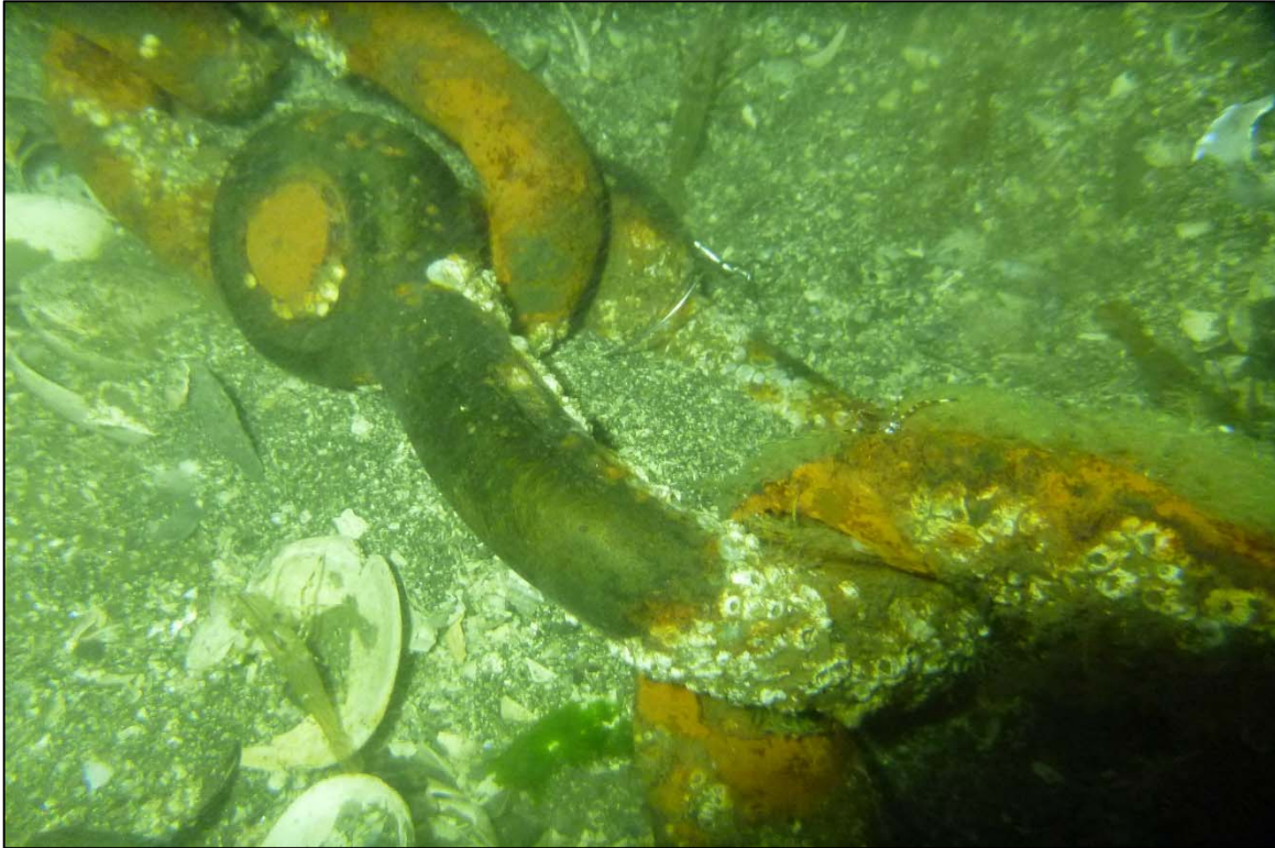
Photograph 31: View of Lower Anchor Rope to Anchor Chain Condition (Shackle and Thimble) at Site 3 Anchor Line 6A, Looking North.
