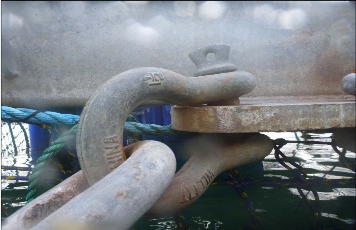
Photograph 85: View of Upper Anchor Chain to Float Connection with (Shackle) at Site 3 Anchor Line 28, Looking Southeast.
