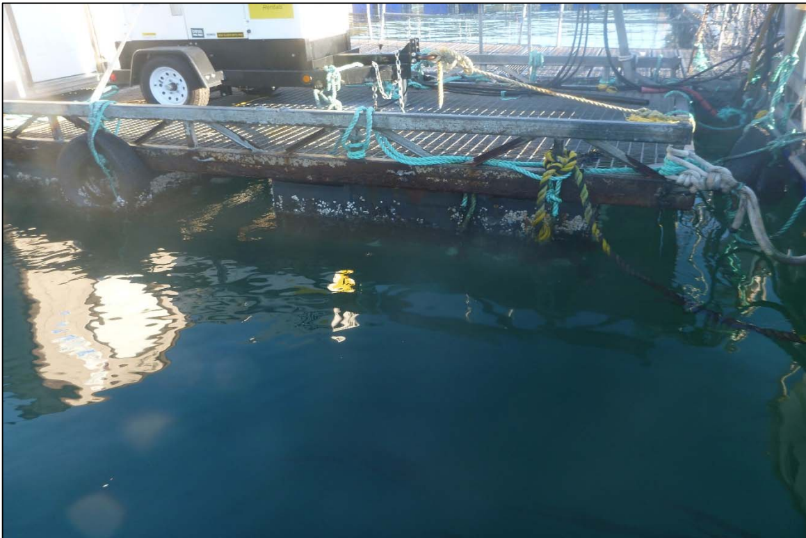
Photograph 8: View of the Float Condition at Site 3 Fish Net Pens System, Looking Northeast.
