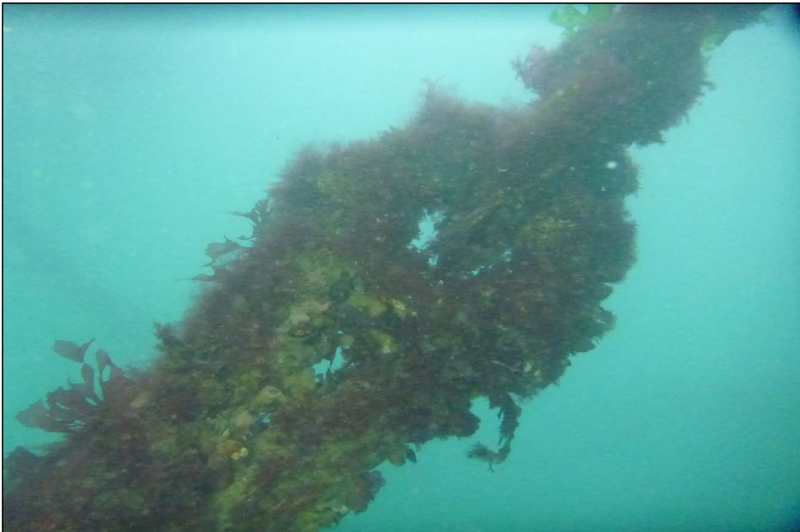
Photograph 20: View of Upper Anchor Chain to Rope Connection (Thimble) at Site 3 Anchor Line 3, Looking North.
