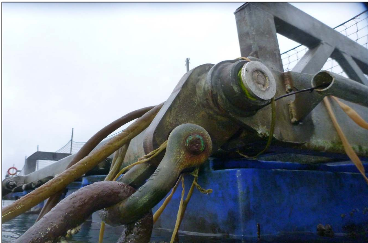
Photograph 18: View of Upper Chain to Float Connection at Site 3 Anchor Line 3, Looking Southeast.
