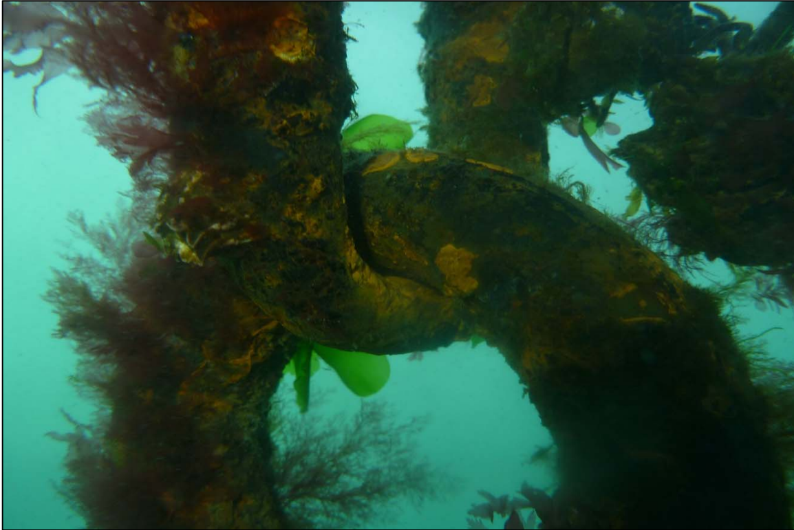
Photograph 61: View of Upper Anchor Chain Corrosion and Section Loss due to Abrasion at Site 3 Anchor Line 17, Looking Northwest.
