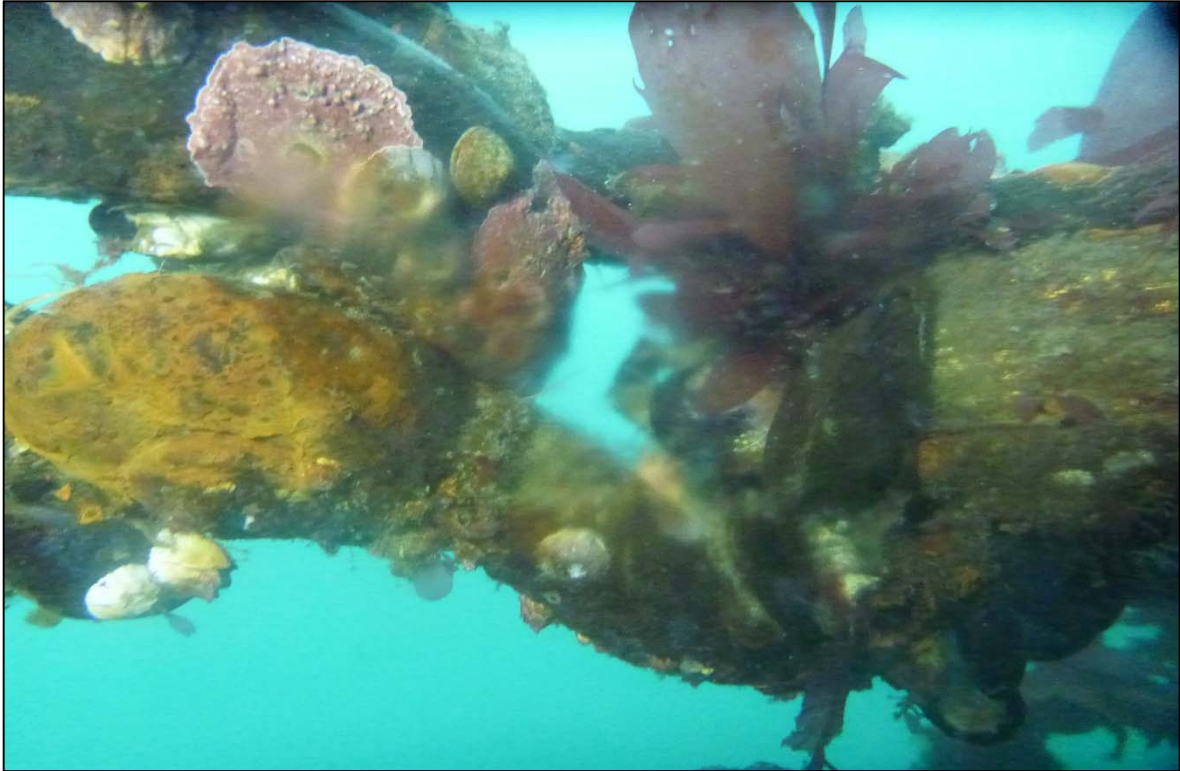
Photograph 81: View of Upper Anchor Chain to Anchor Rope Connection with Corrosion and Pitting (Shackle and Thimble) at Site 3 Anchor Line 25, Looking North.
