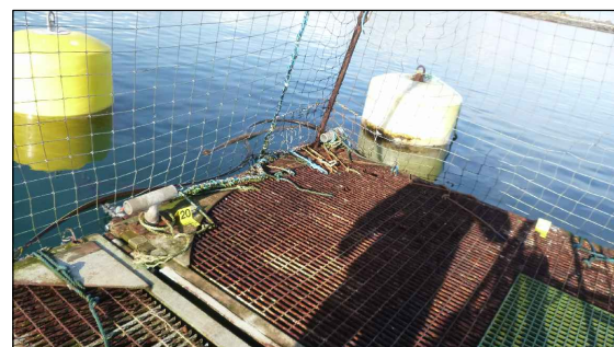
PHOTO 1 TYPICAL CORROSION ON EXTERIOR CORNER WALKWAY GRATING
