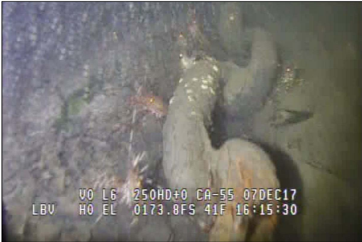
Photograph 54: View of Lower Anchor Chain Condition (Typical) at Primary System Anchor Line 15, Looking West.
