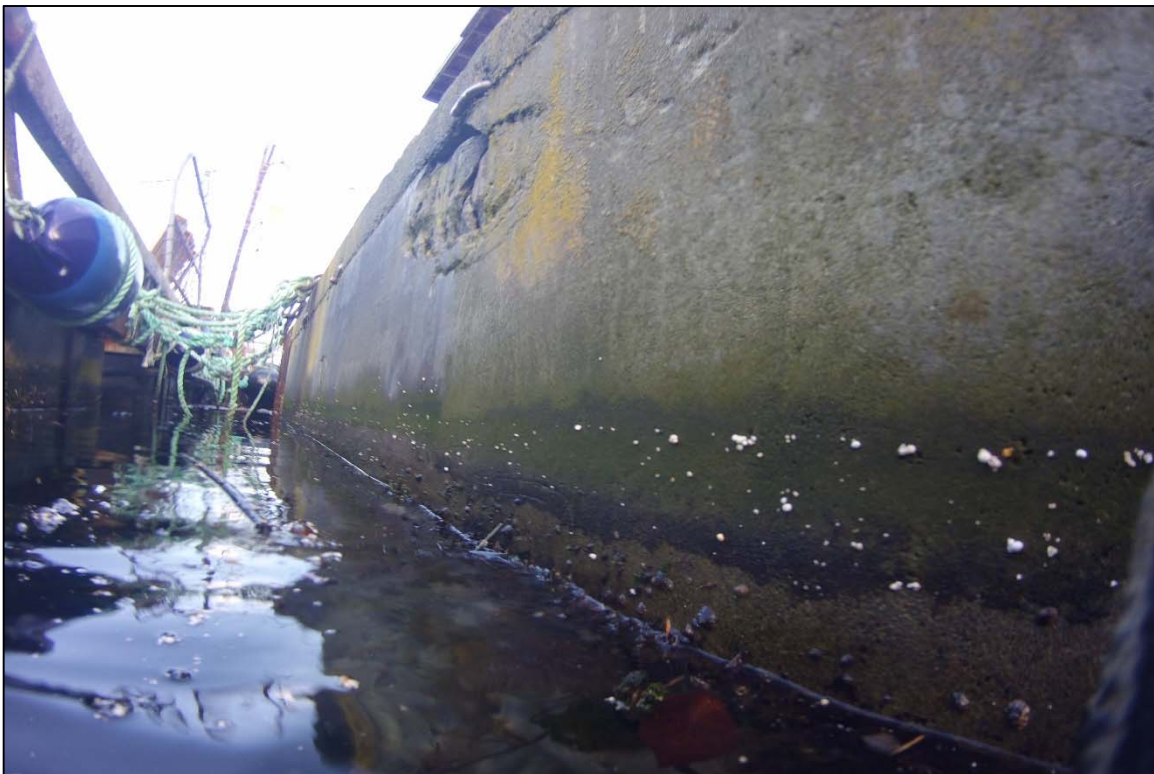
Photograph 24: View of the Typical Condition of the Office Building Float at the Waterline, Looking South.
