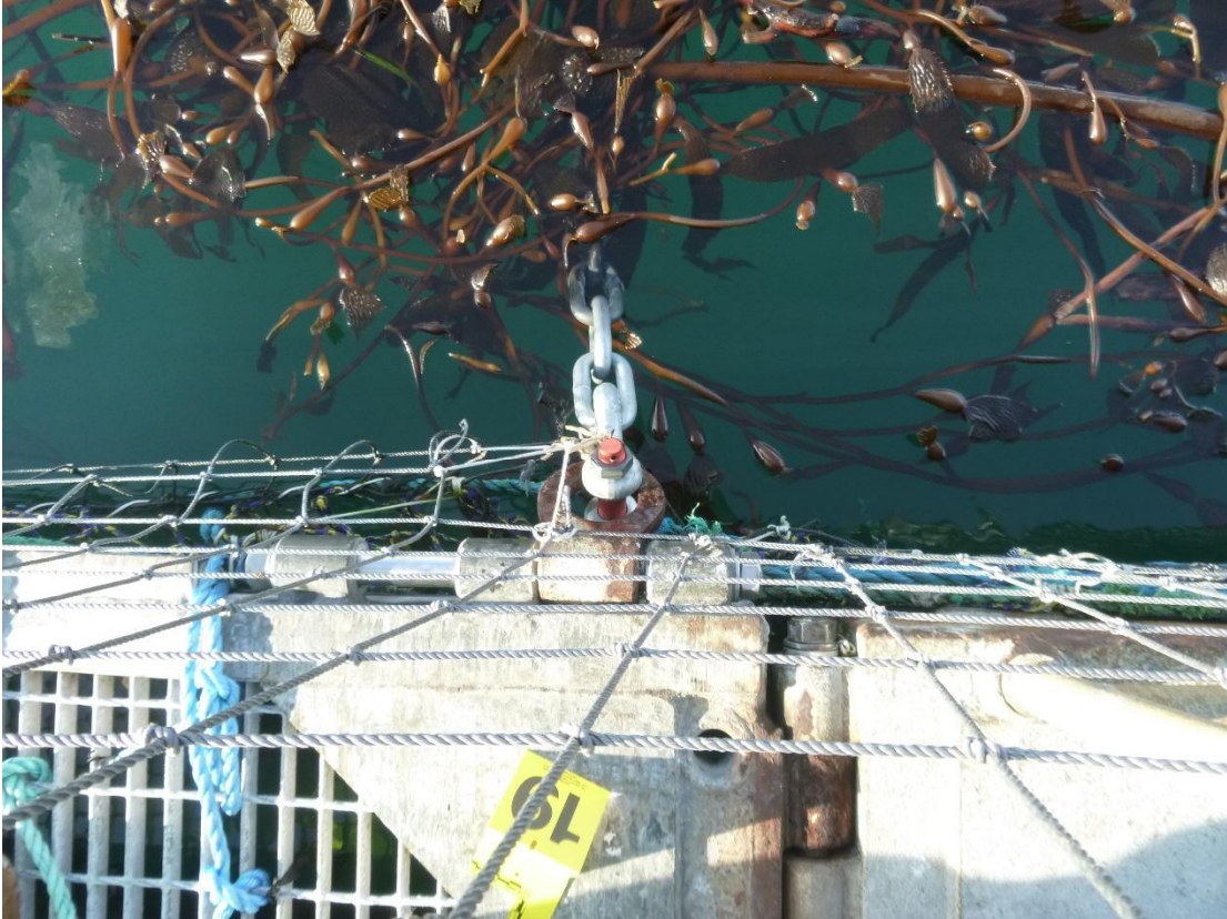
Figure C-64: Anchor 19 Right Padeye and Chain
