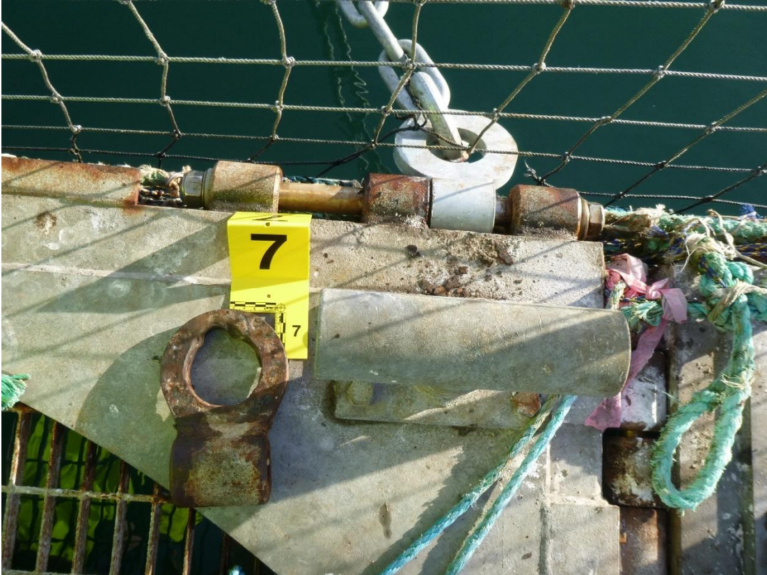
Figure C-22: Anchor 7 New Right Padeye Showing old Padeye
