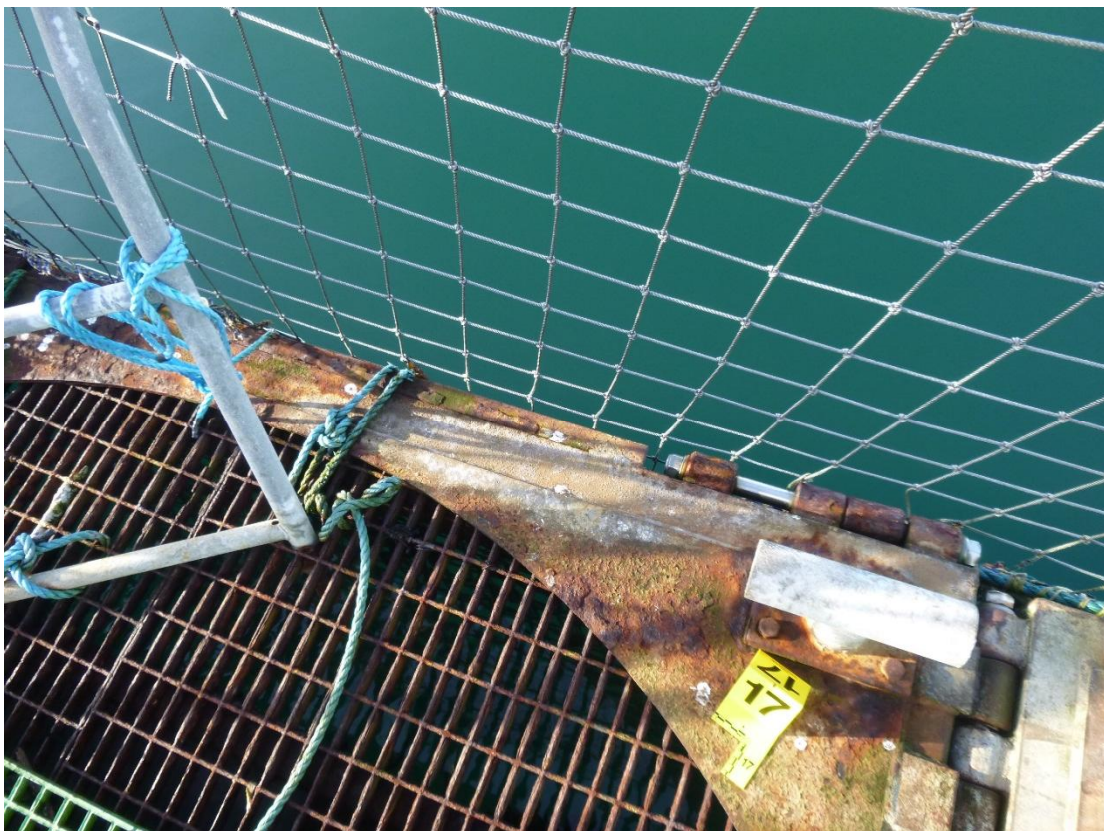
Figure C-57: Anchor 17 Missing - Right Padeye Hinge
