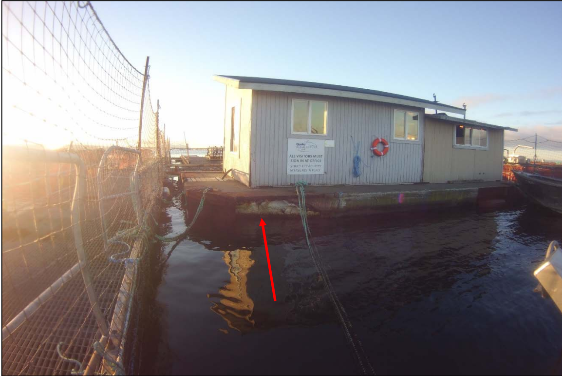
Photograph 21: View of the Storage Buildings Located between Pens 6 and 8 and Area of Deterioration at the Southeast Corner, Looking West.
