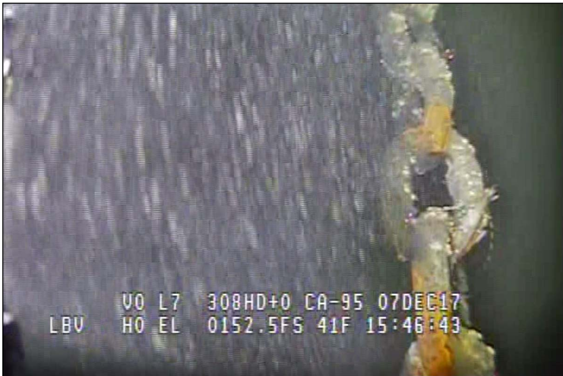
Photograph 56: View of Lower Anchor Chain Condition (Typical) at Primary System Anchor Line 16, Looking West.
