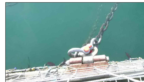
PHOTO 4 IMPROPER ASSEMBLY OF 2 SHACKLES TO ONE PADEYE
