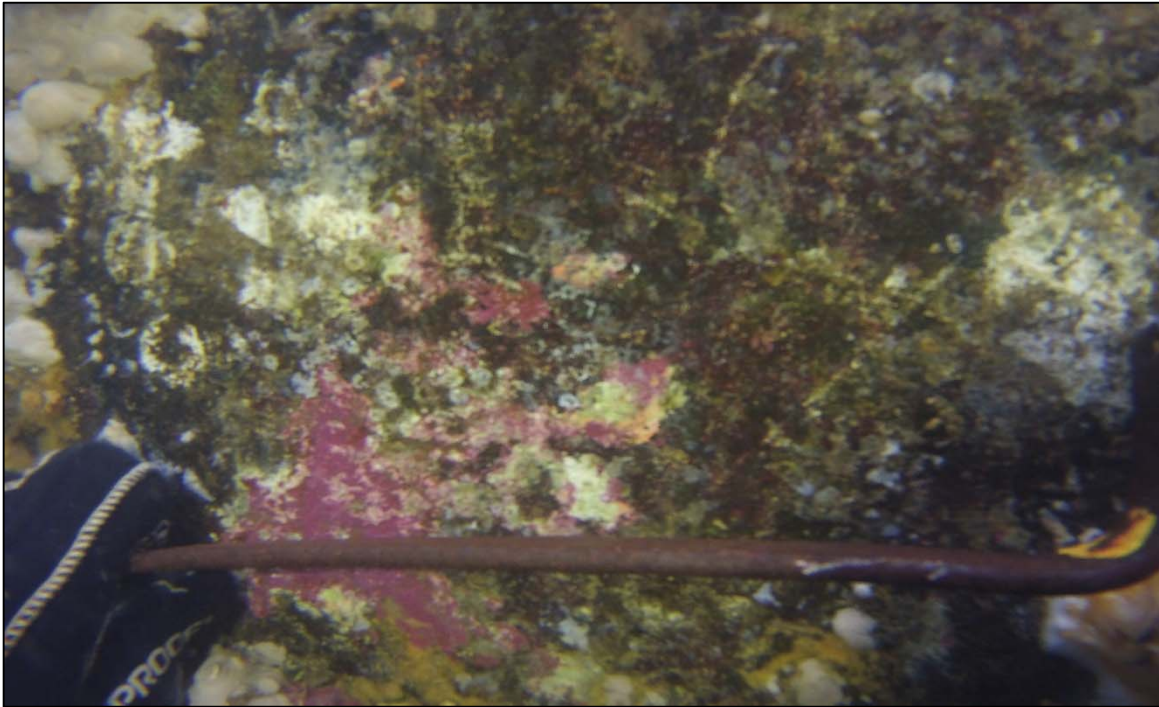
Photograph 25: View of Typical Concrete Condition of the Office Building Barge Float, Looking East.
