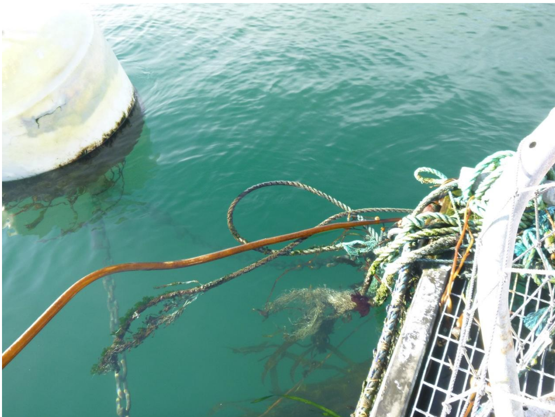
Figure C-37: Anchor 11 Buoy and Bridle Chains Unevenly Loaded
