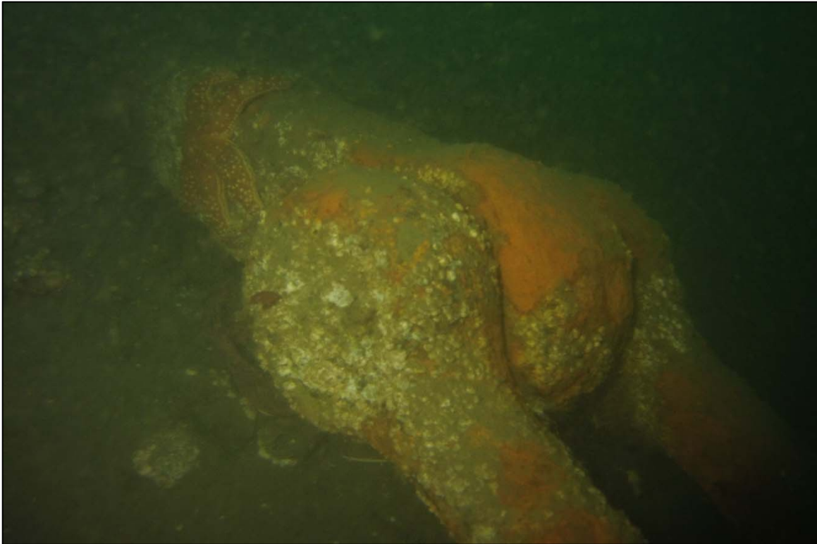
Photograph 36: View of Anchor Stem to Anchor Chain Connection at Anchor 22 (Typical Observed by Diver), Looking Southwest.
