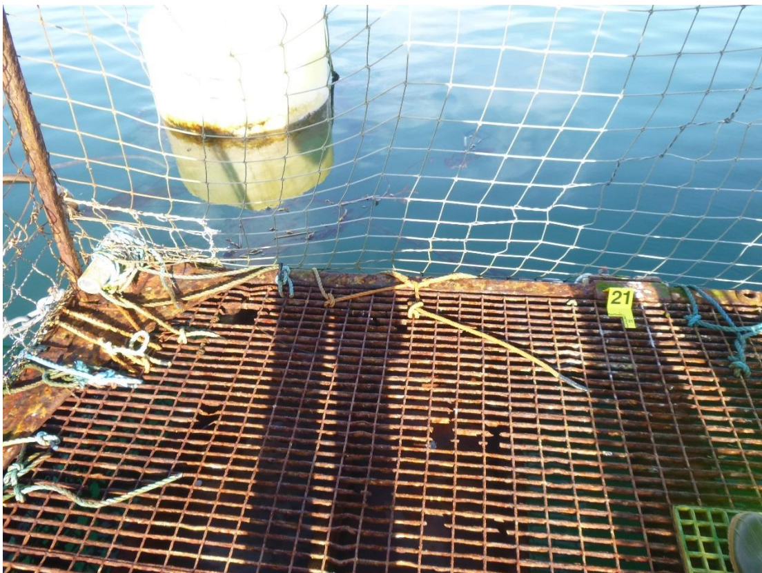
Figure C-69: Anchor 21 Showing Severe Corrosion in Grating
