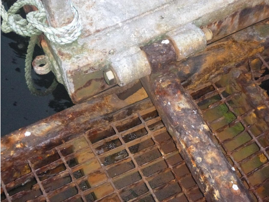
Figure C-54: Floating Dock Boarding Area, Damage to Dock Frame From Arms
