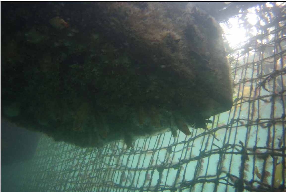
Photograph 12: View of the Typical Walkway float Condition.
