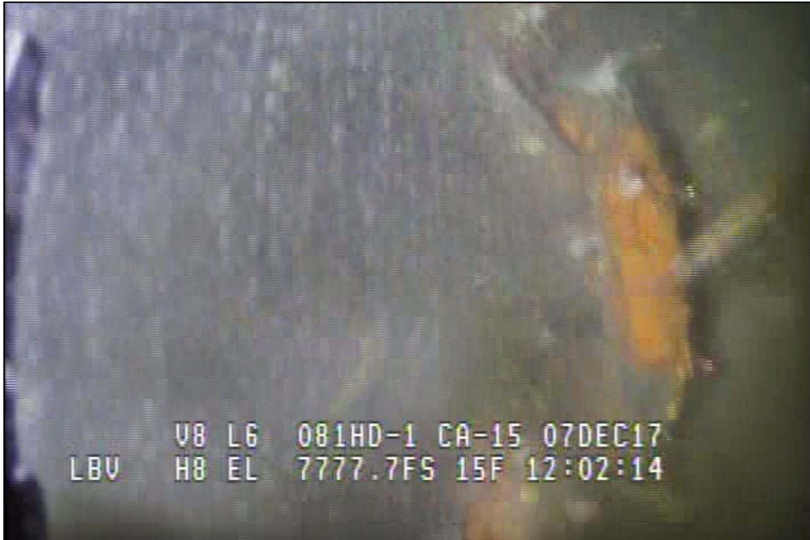
Photograph 41: View of Lower Anchor Chain Embedment in the Channel Bottom at Primary System Anchor Line 4, Looking East.
