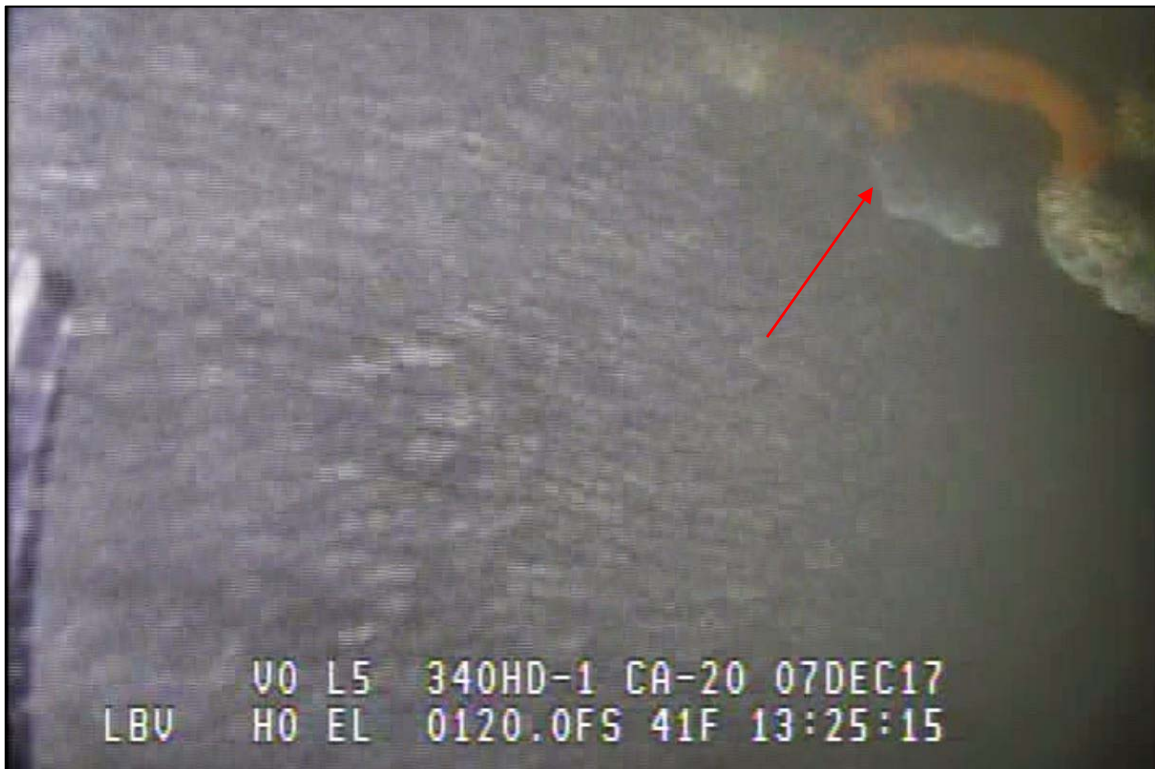
Photograph 61: View of Lower Anchor Chain Condition (Typical) at Primary System Anchor Line 18, Looking West.
