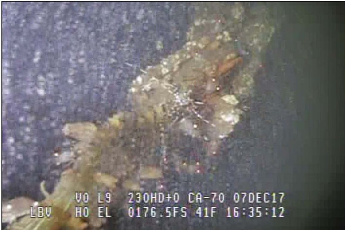
Photograph 48: View of Lower Anchor Chain to Rope Connection (Thimble and Shackle) at Primary System Anchor Line 14, Looking West.
