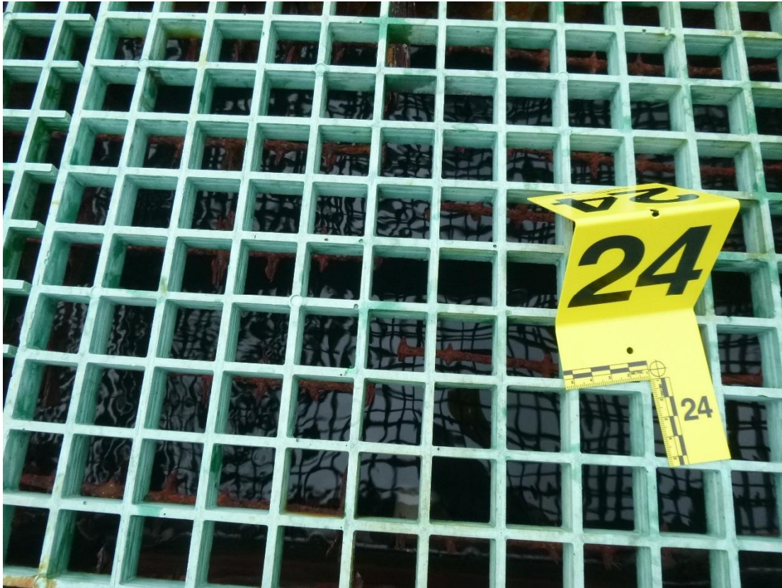
Figure C-78: Fiberglass Mesh Covers Severe Corrosion in Grating
