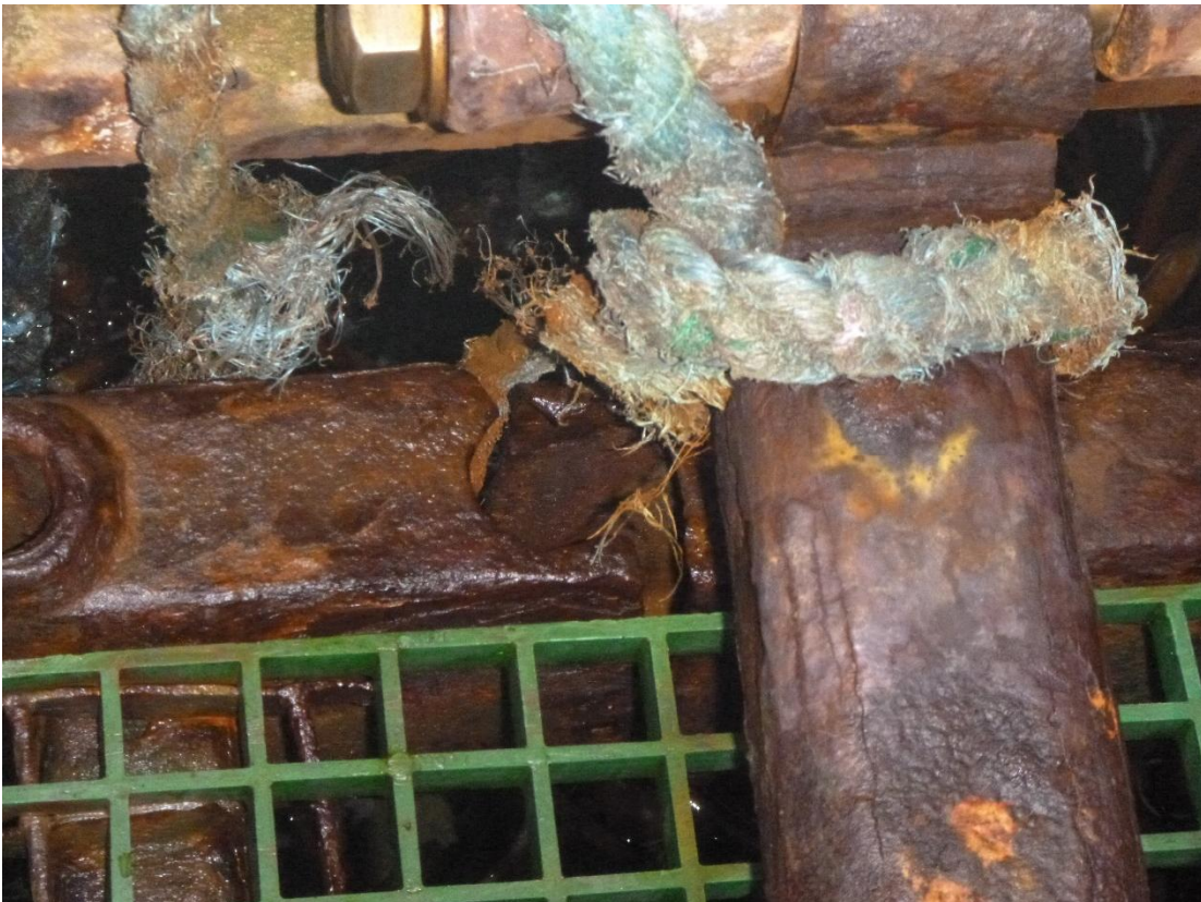
Figure C-55: Floating Dock Boarding Area, Broken Dock Frame From Arms
