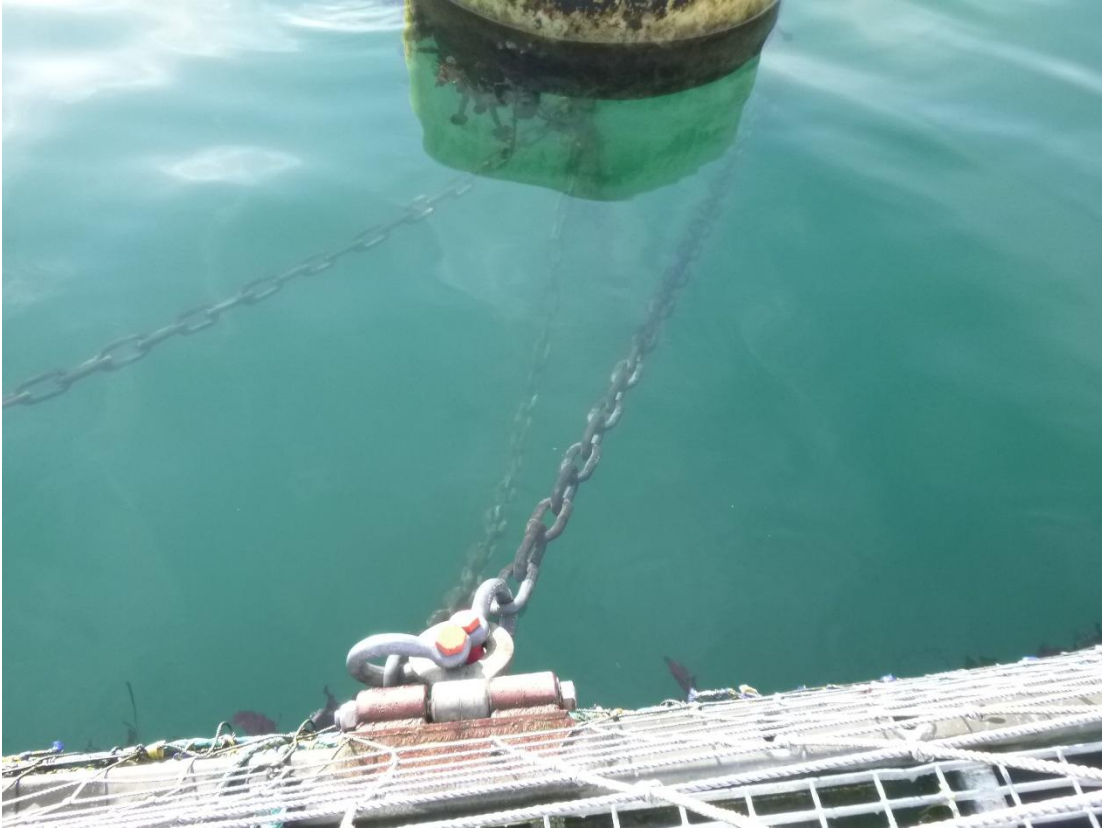
Figure C-30: Anchor 10 and Chain From Additional Unknown Anchor. Note Two Shackles in One Padeye
