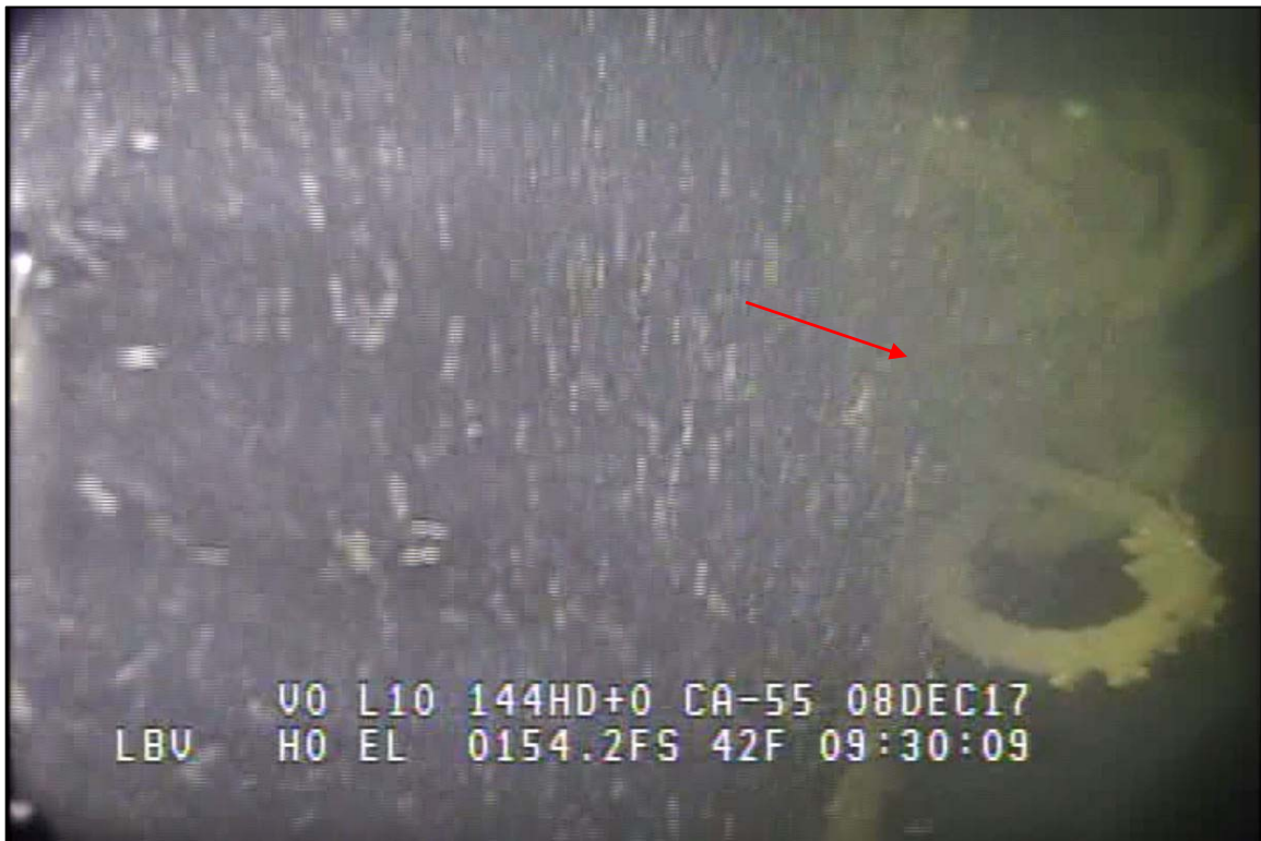
Photograph 42: View of Knots in the Anchor Line Rope at Primary System Anchor Line 10A1, Looking South.
