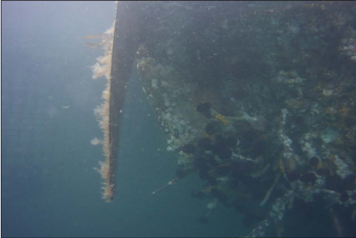
Photograph 23: View of the Area of Section Loss and Exposed Foam Floatation on the Southeast Corner of the Building Barge Float, Looking South.
