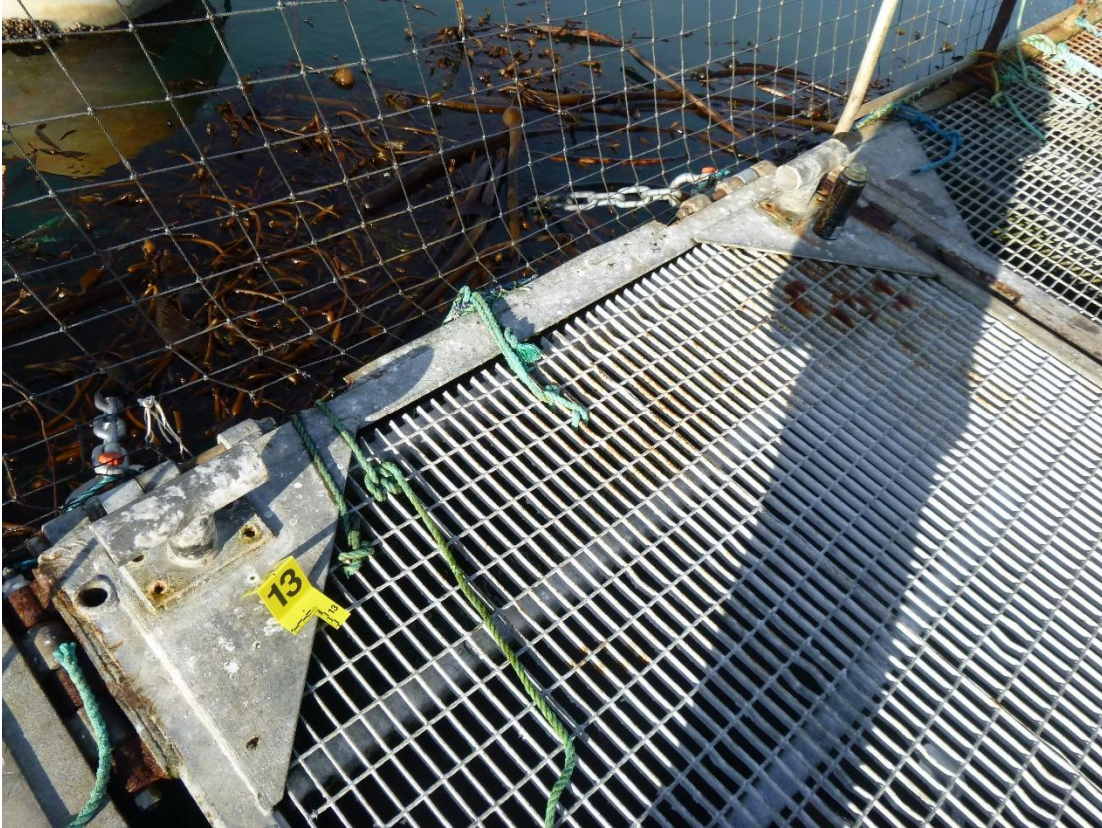
Figure C-42: Anchor 13 Bridle Chains
