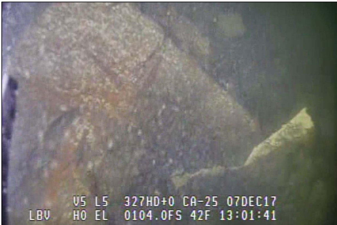
Photograph 67: View of Anchor North Fluke Embedment in the Channel Bottom at Primary System Anchor Line 19, Looking West.
