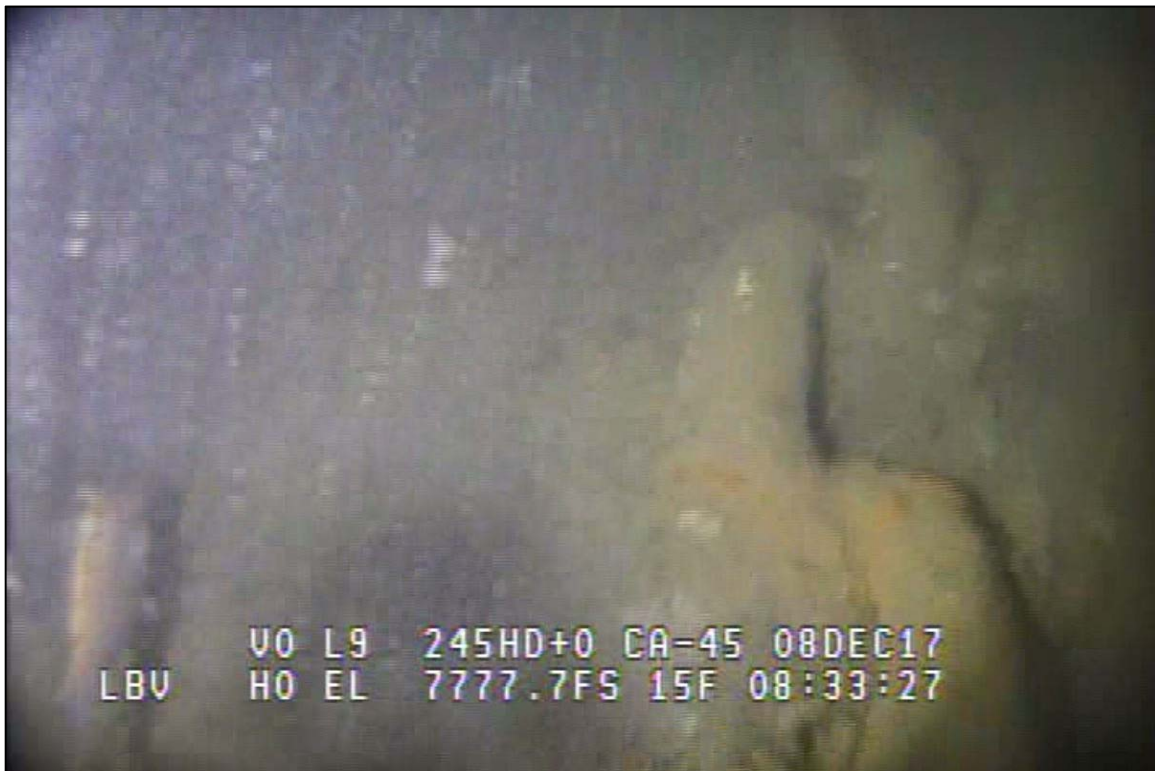
Photograph 46: View of Lower Anchor Chain Condition (Typical) at Primary System Anchor Line 12, Looking West.
