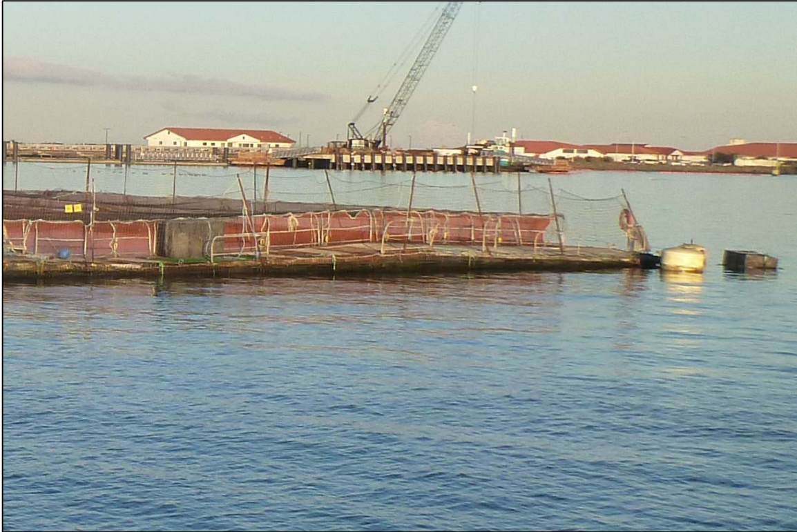
Photograph 11: View of the Depressed Pen Support Float at the Southeast Corner, Looking Northeast.
