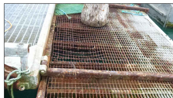
PHOTO 8 SEVERE CORROSION ON BOARDING FLOATS
