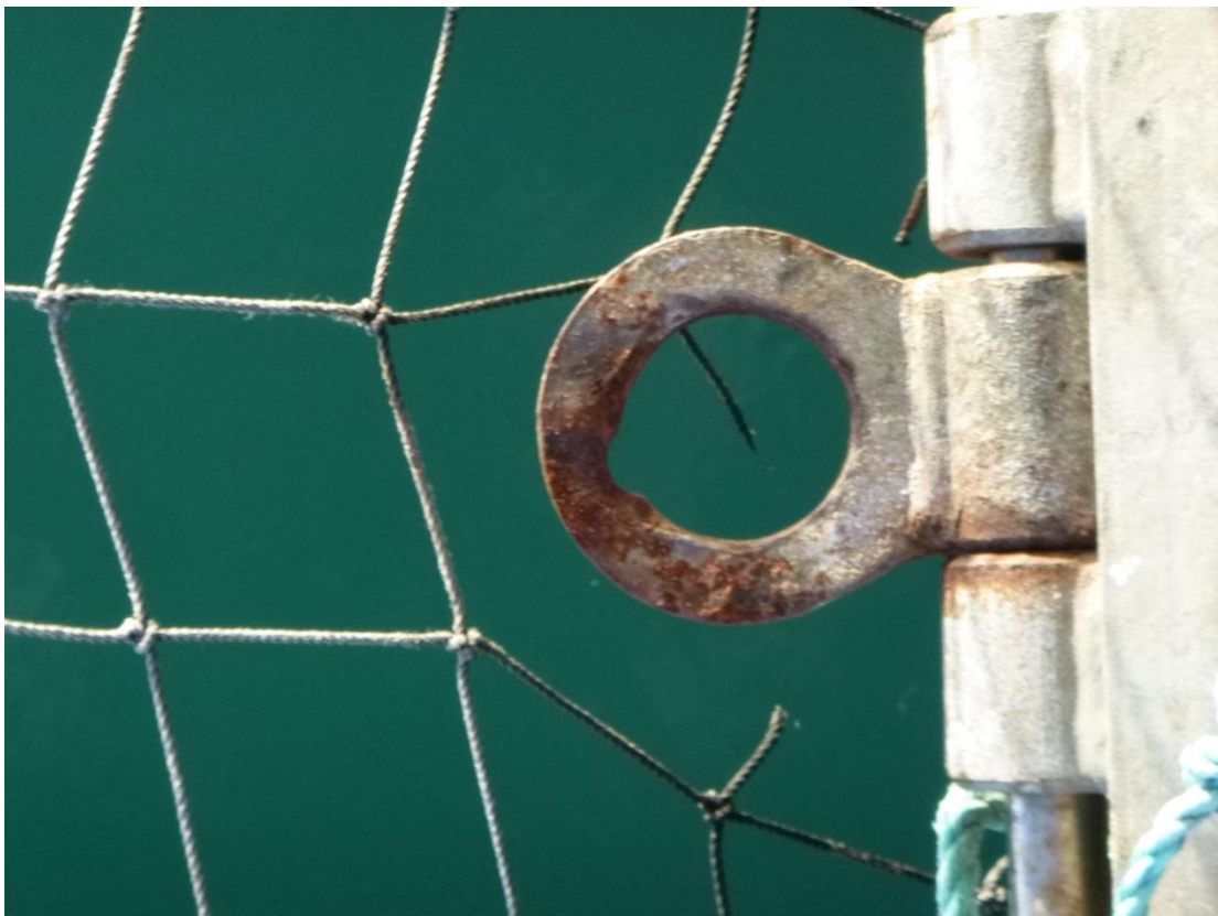
Figure C-19: Anchor 6 Right Padeye Showing Wear
