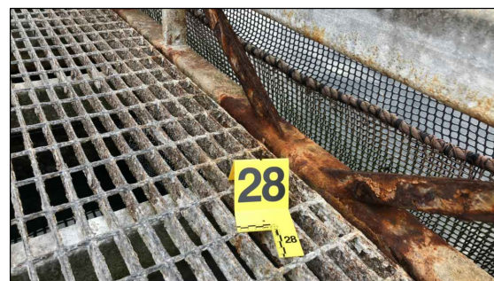
PHOTO 2 TYPICAL CORROSION ON 10 FT WIDE WALKWAY TRUSS MEMBER
