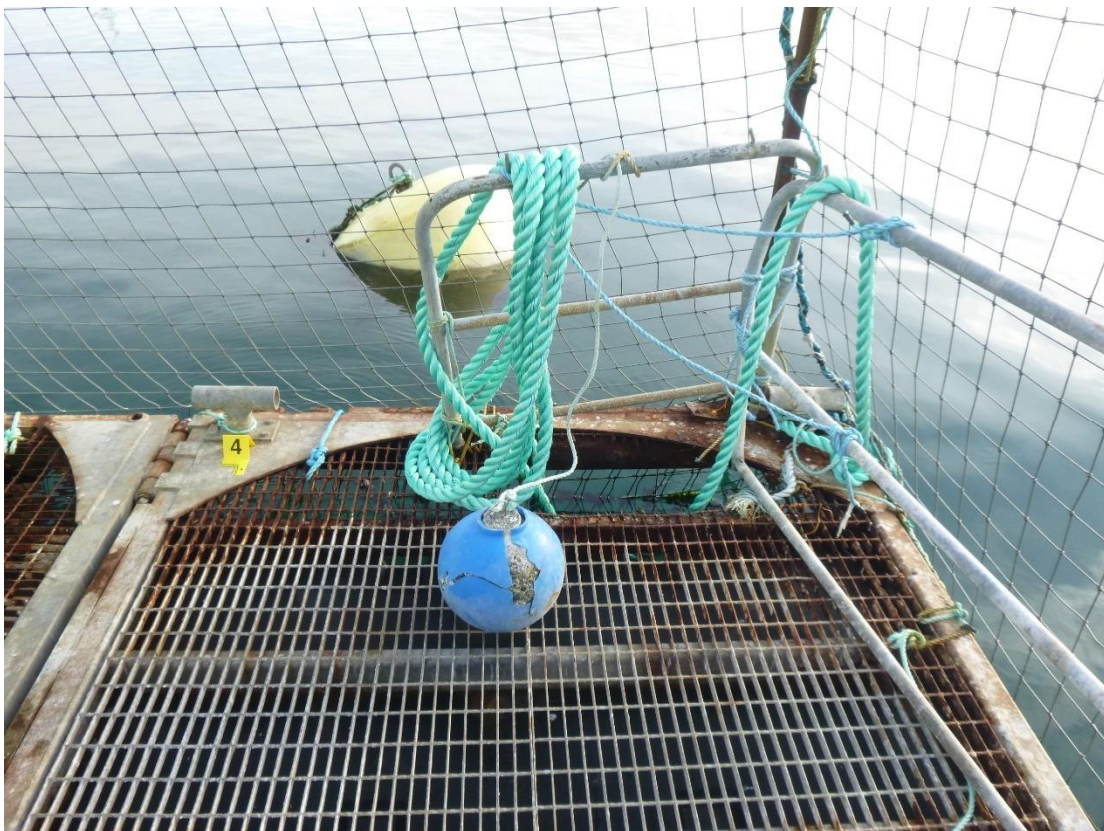
Figure C-11: Anchor 4 Showing Severe Corrosion of Grating in Corner
