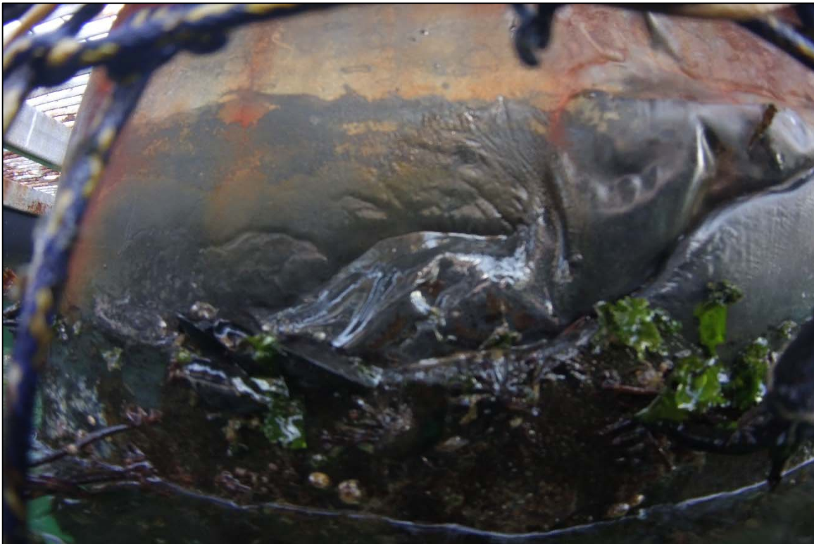
Photograph 18: View of the Heat Damage (Melted Plastic) Float 2 Shown, Looking North.
