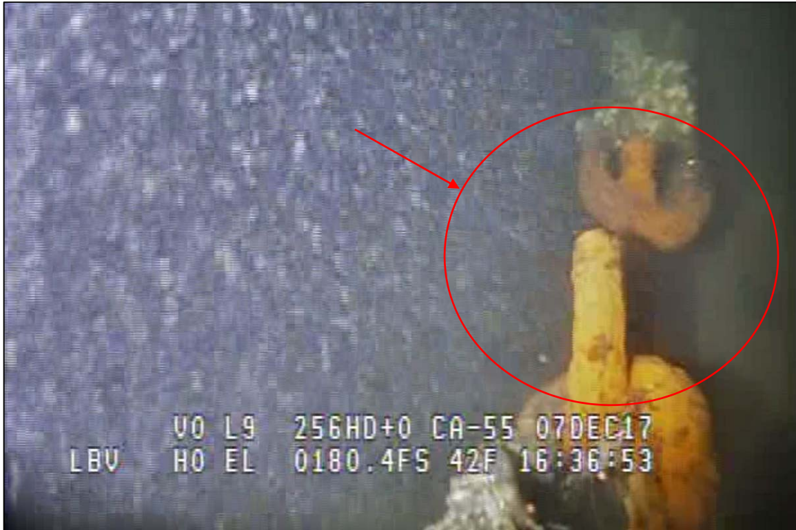
Photograph 49: View of a Broken Chain Link in the Lower Anchor Chain at Primary System Anchor Line 14, Looking West.
