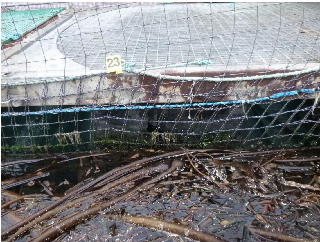
Figure C-75: Location 23 Damaged Pontoon (South Edge of Pen 5)
