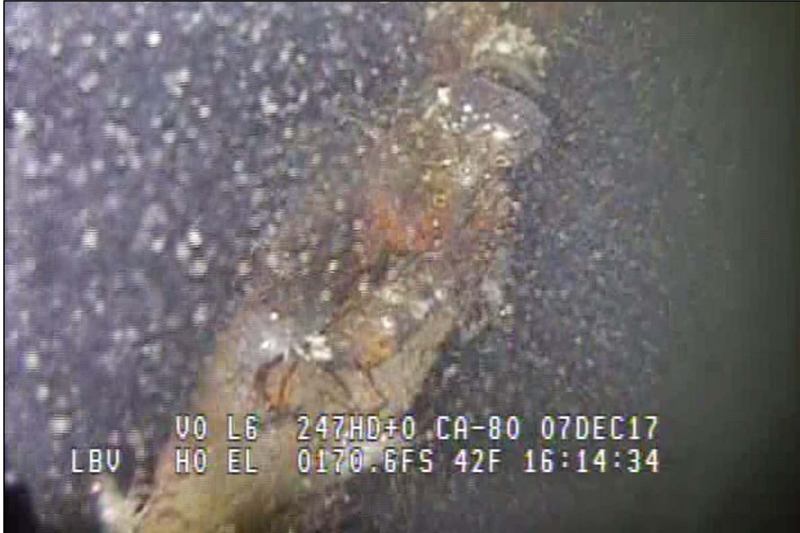
Photograph 53: View of Lower Anchor Chain to Rope Connection (Thimble and Shackle) at Primary System Anchor Line 15, Looking West.
