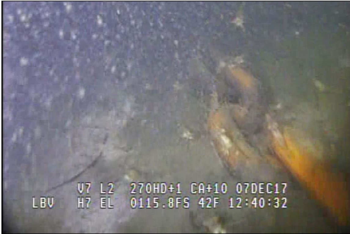
Photograph 70: View of Lower Anchor Chain Condition (Typical) at Primary System Anchor Line 20, Looking Southwest.
