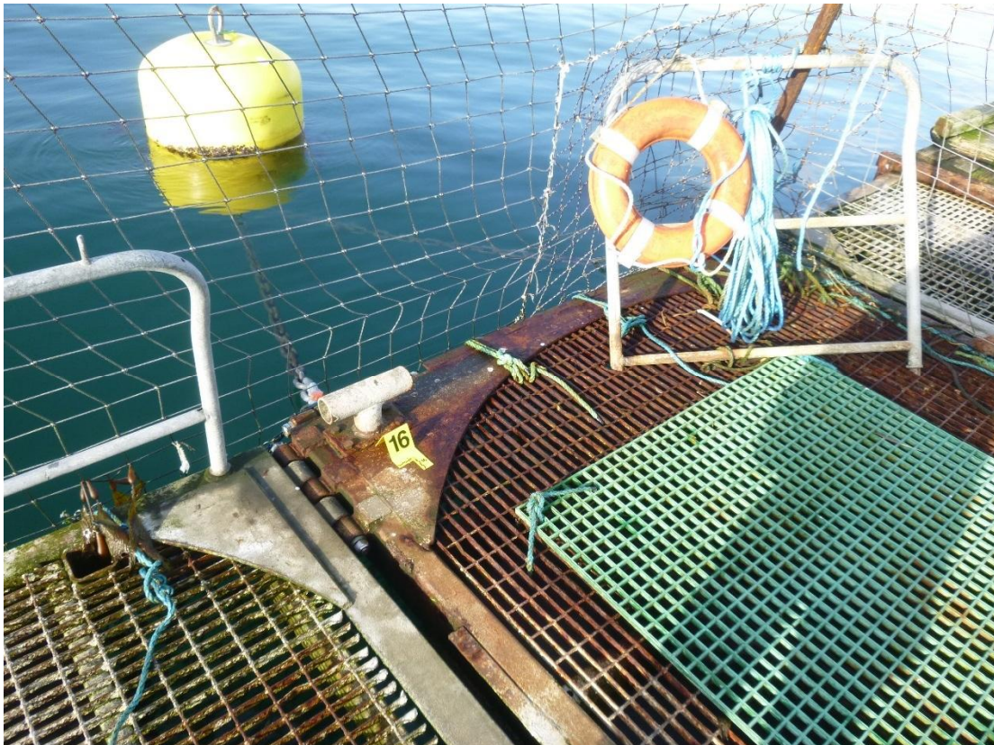
Figure C-49: Anchor 16 Showing Moderate to Severe Corrosion of Grating
