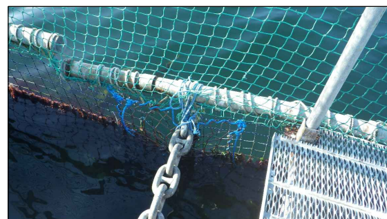
PHOTO 6 ANCHOR 10 MOORING CHAIN CAUSING BENDING TO PREDATOR NET SUPPORT PIPE
