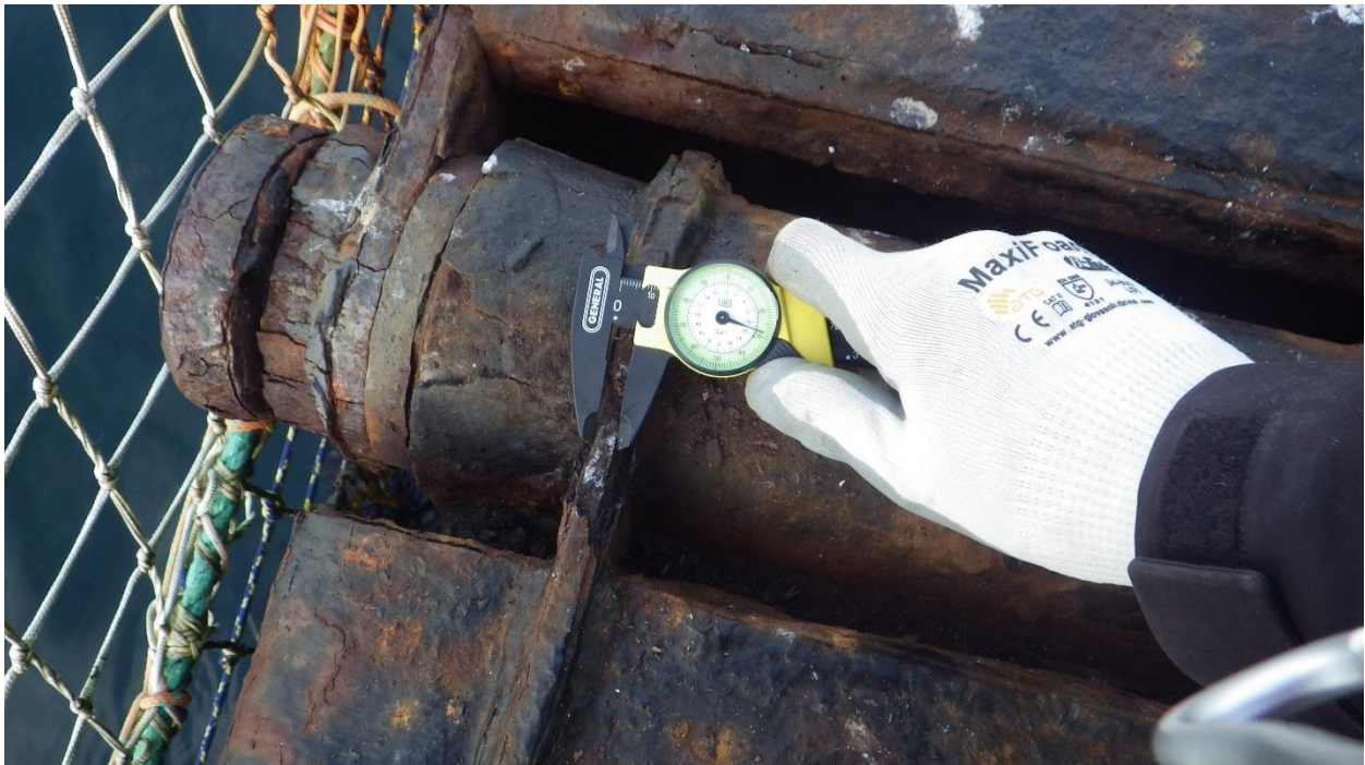
Figure D-58: Rusted Hinge Connection, Major Corrosion, Reduced Section of 40%.
