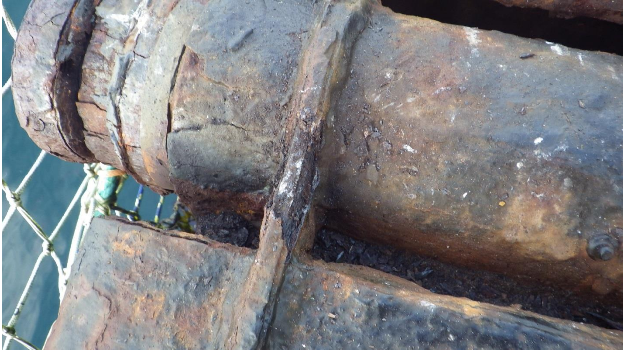
Figure D-59: Rusted Hinge Connection, Major Corrosion, Reduced Section of 40%.
