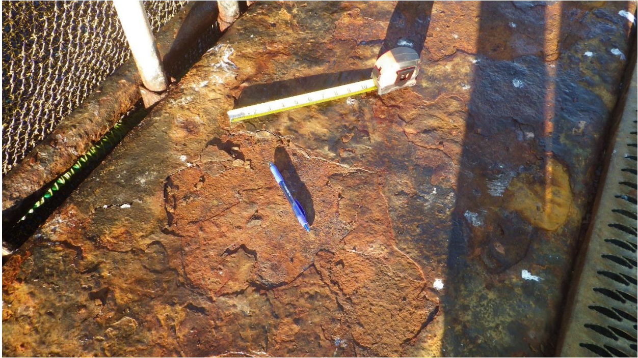
Figure C-42: Rusted Outer Steel Frame on North East side walkway. Moderate to major corrosion.
