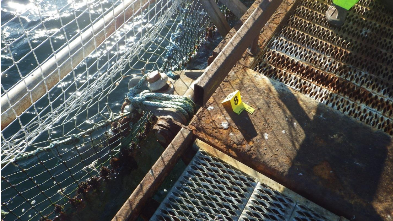
Figure D-19: Anchor #8, South Side of the South Net Pen. Hinge with moderate corrosion.
