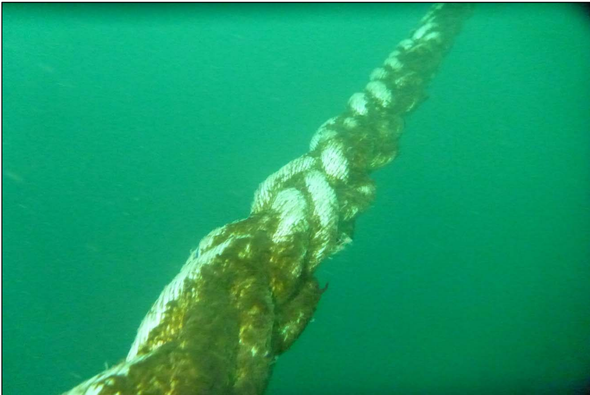
Photograph 14: View of Rope Condition with Light Marine Growth at Orchard Rocks North Anchor Line 1, Looking East.
