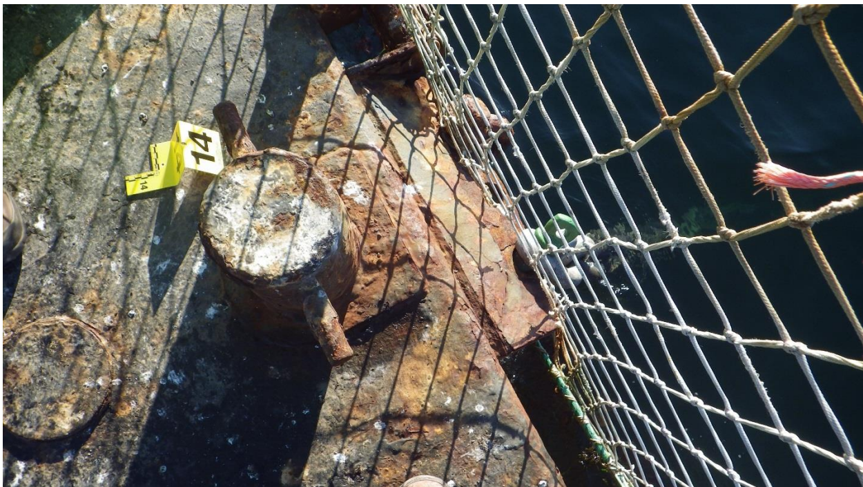
Figure D-32: Anchor #14, West Side of the South Net Pen
