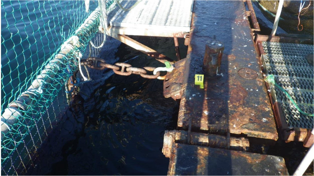
Figure C-24: Anchor #11, West Side of the North Net Pen. New shackle with old chain. Minor corrosion on chain. Chain tied to predator support pipe.
