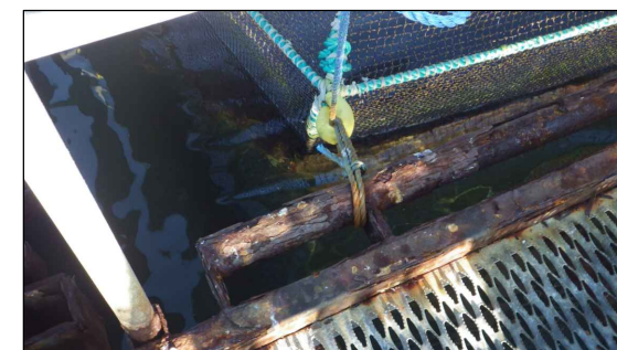
PHOTO 4 FISH NET CORRODED SUPPORT PIPE
