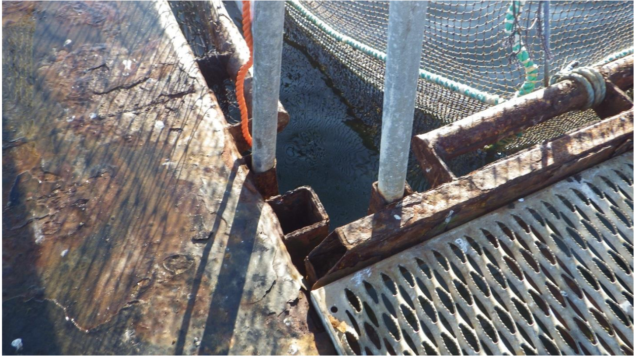
Figure D-51: Rusted Steel Framing, Handrail Brackets, and Net Pen Support Railings, moderate to major corrosion.
