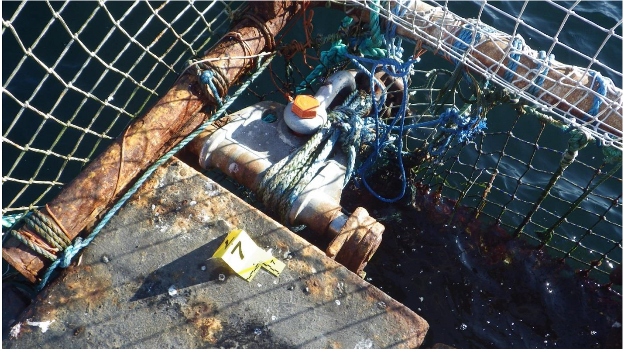
Figure D-17: Anchor #7, SE Corner of the South Net Pen. Hinge with minor to moderate corrosion.
