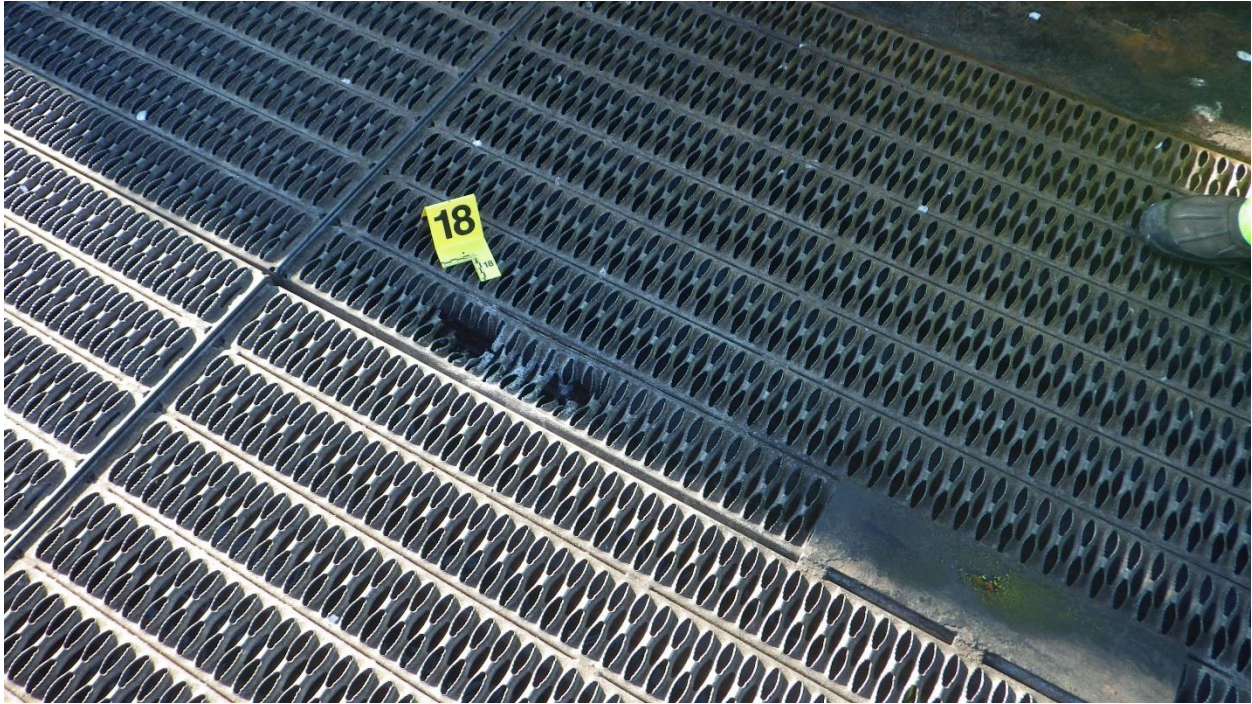
Figure C-52: Damaged Grating Panel at Center Bridge.
