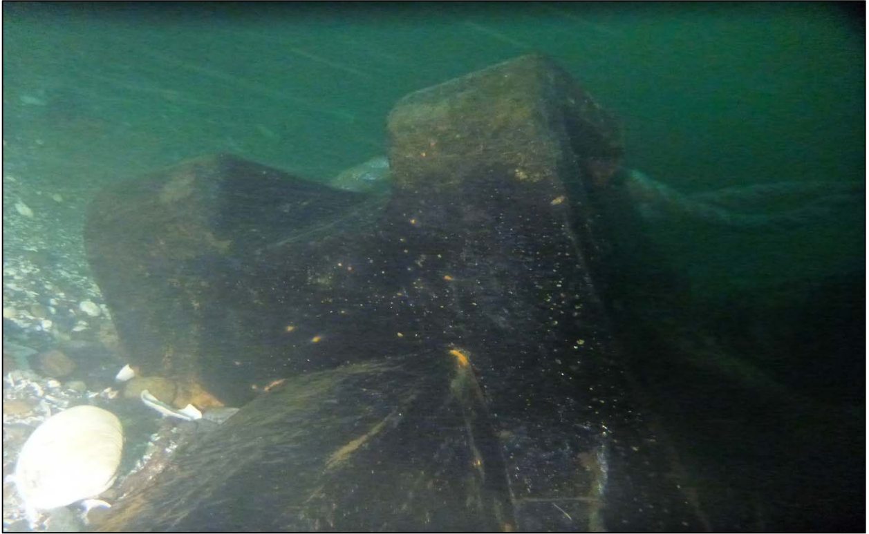
Photograph 93: View of Top of the New Anchor Rope at Orchard Rocks South Anchor Line 14, Looking West.
