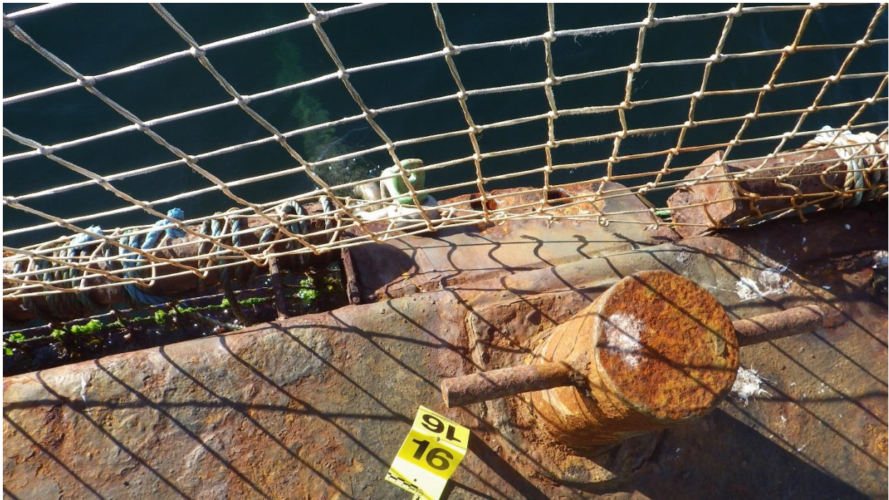
Figure D-37: Anchor #16, West Side of the South Net Pen, with new shackle and chain.
