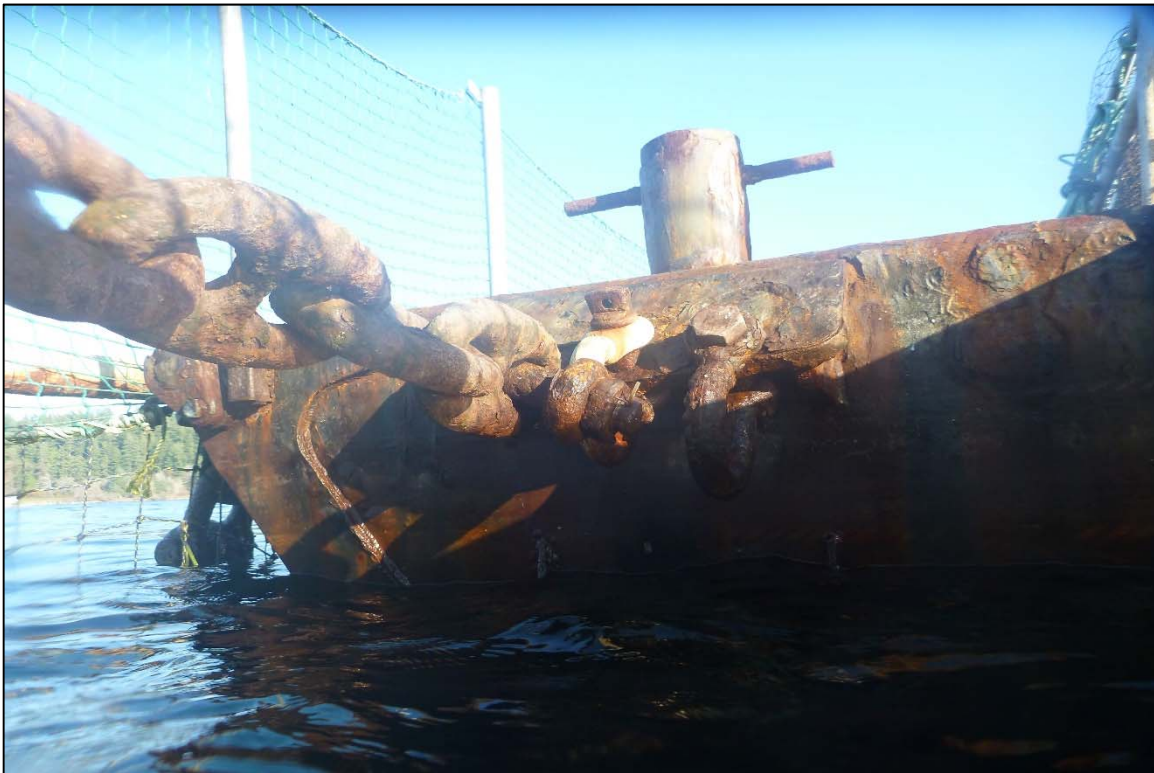
Photograph 12: View of Upper Anchor Chain to Float Connection at Orchard Rocks North Anchor Line 12, Looking East.
