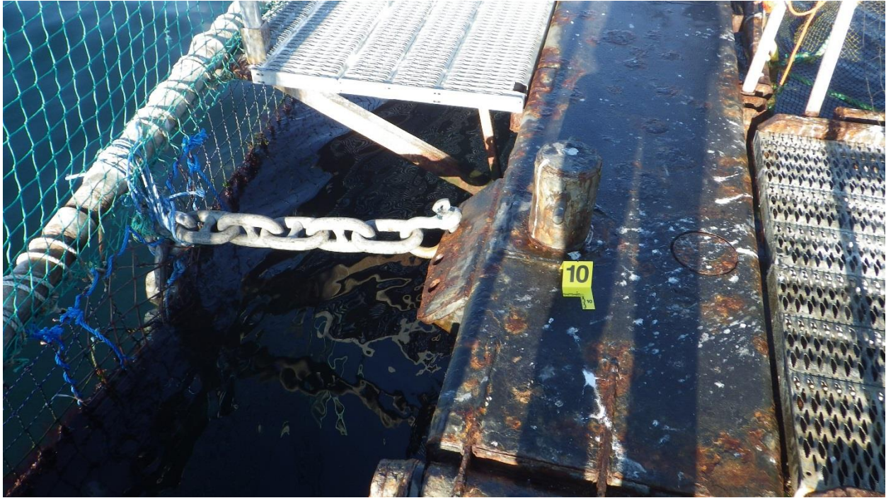
Figure C-22: Anchor #10, West Side of the North Net Pen. New shackle and chain. Chain tied to predator support pipe.
