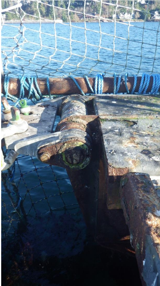
Figure D-39: South East Hinge connected to North pen with moderate corrosion.
