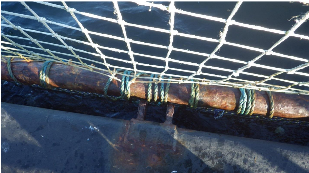
Figure D-52: Rusted Predator Net Support Railing with moderate corrosion.
