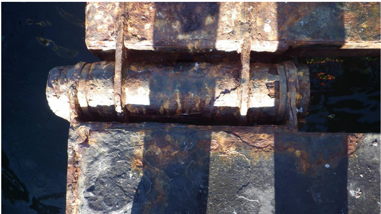
Figure C-61: Rusted Hinge between anchors 11 and 12. Moderate to major corrosion.
