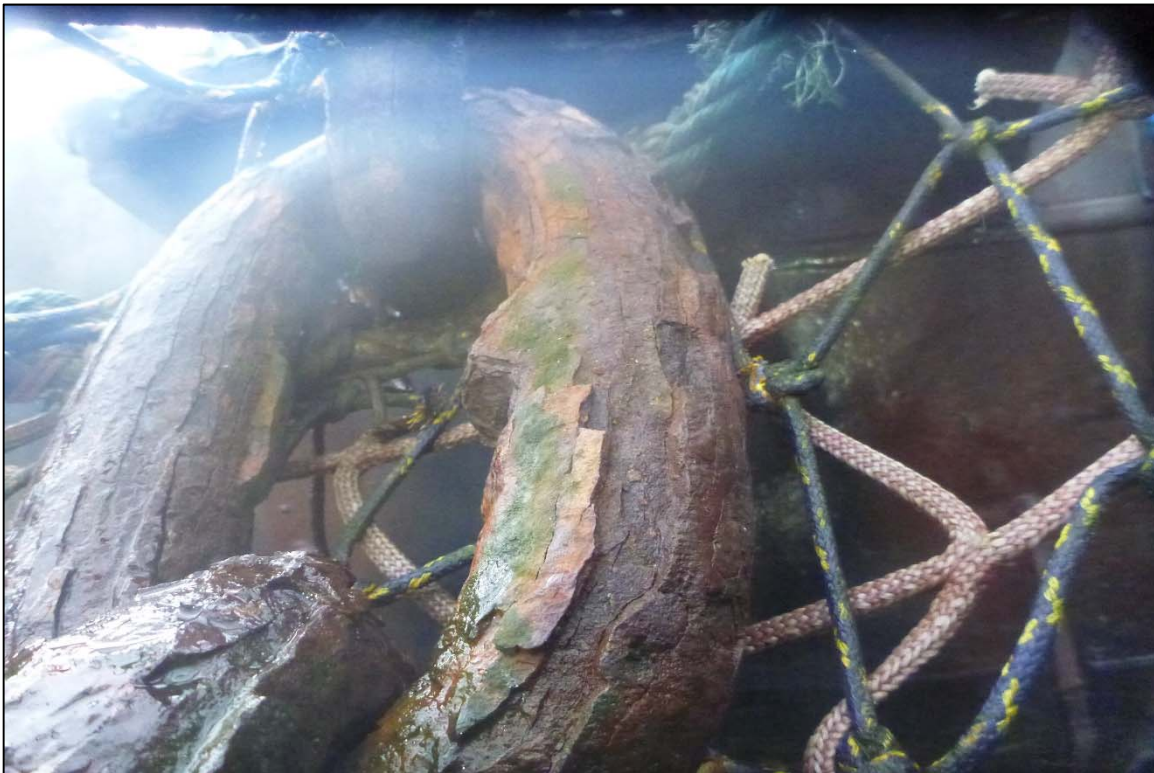
Photograph 24: View of Upper Anchor Chain Condition with Heavy Corrosion and Delamination at Orchard Rocks North Anchor Line 4, Looking West.
