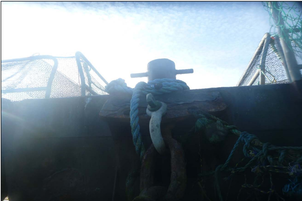
Photograph 20: View of Upper Anchor Chain to Float Connection with Severe Corrosion at Orchard Rocks North Anchor Line 3, Looking West.
