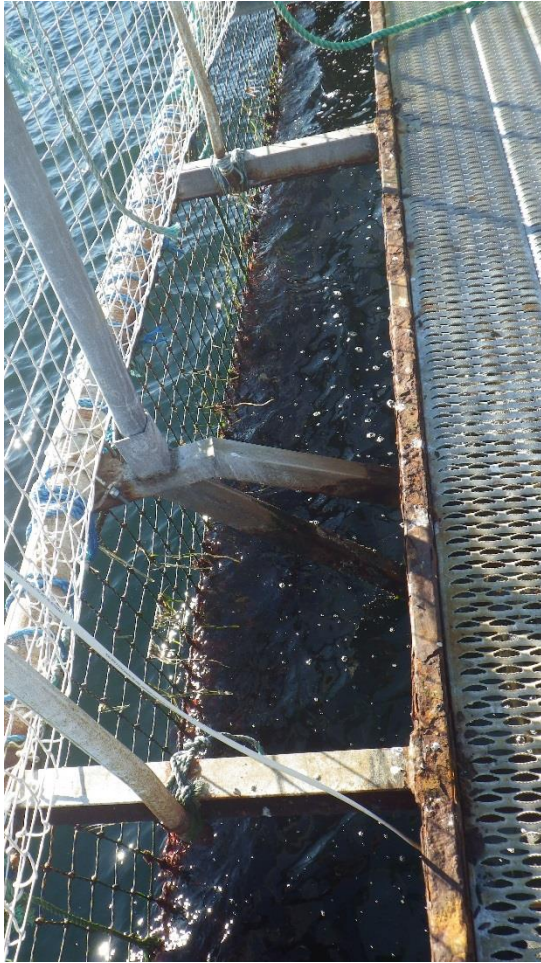
Figure D-53: Cantilevered Predator Net Supports - Moderate corrosion.
