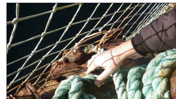
PHOTO 4 CORRODED SHACKLES AND MOORING BRACKET AT ANCHOR 13
