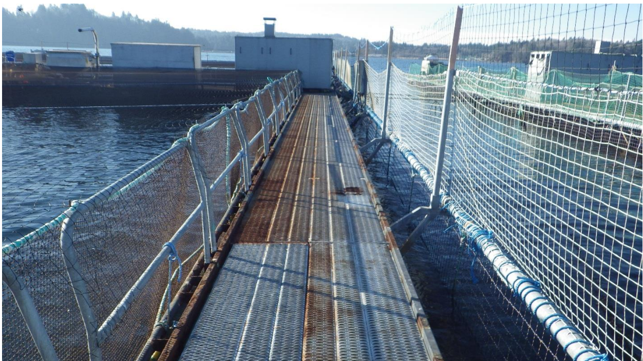
Figure D-50: Rusted Grated Walkway and Center Bridge and staff shed.
