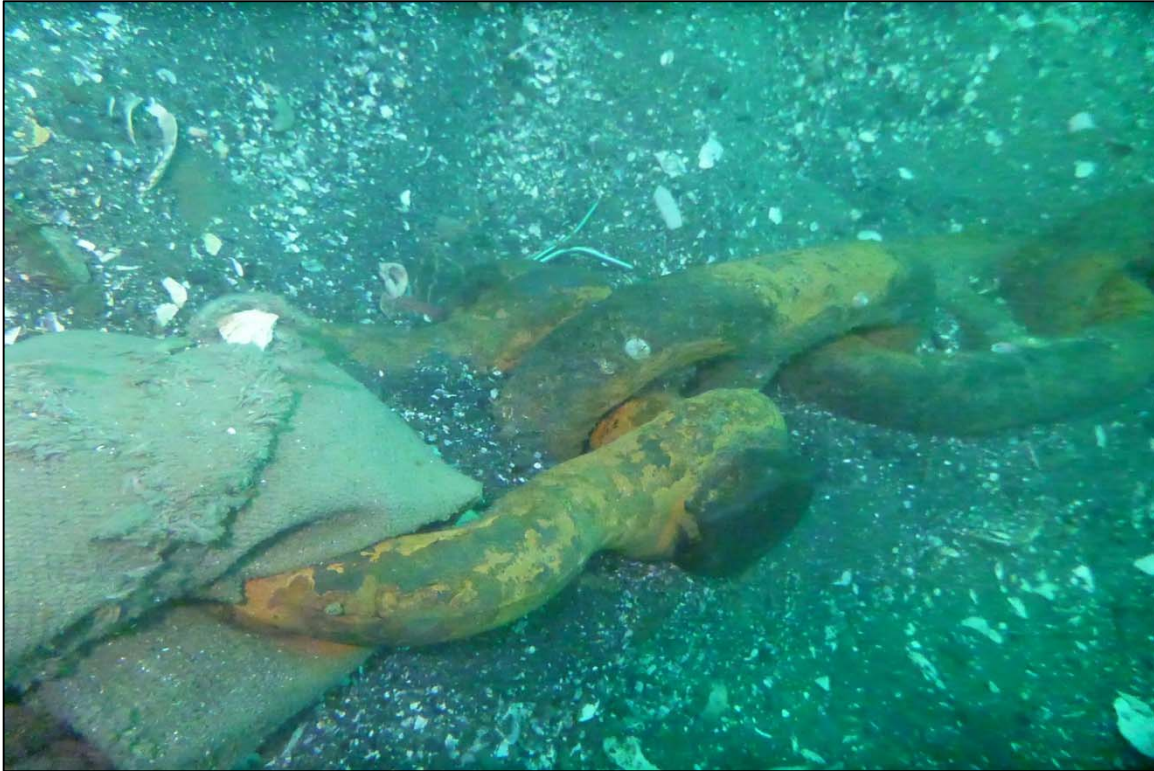
Photograph 31: View of Rope to Lower Anchor Chain Connection (Shackle and Sleeve) at Orchard Rocks North Anchor Line 9, Looking North.
