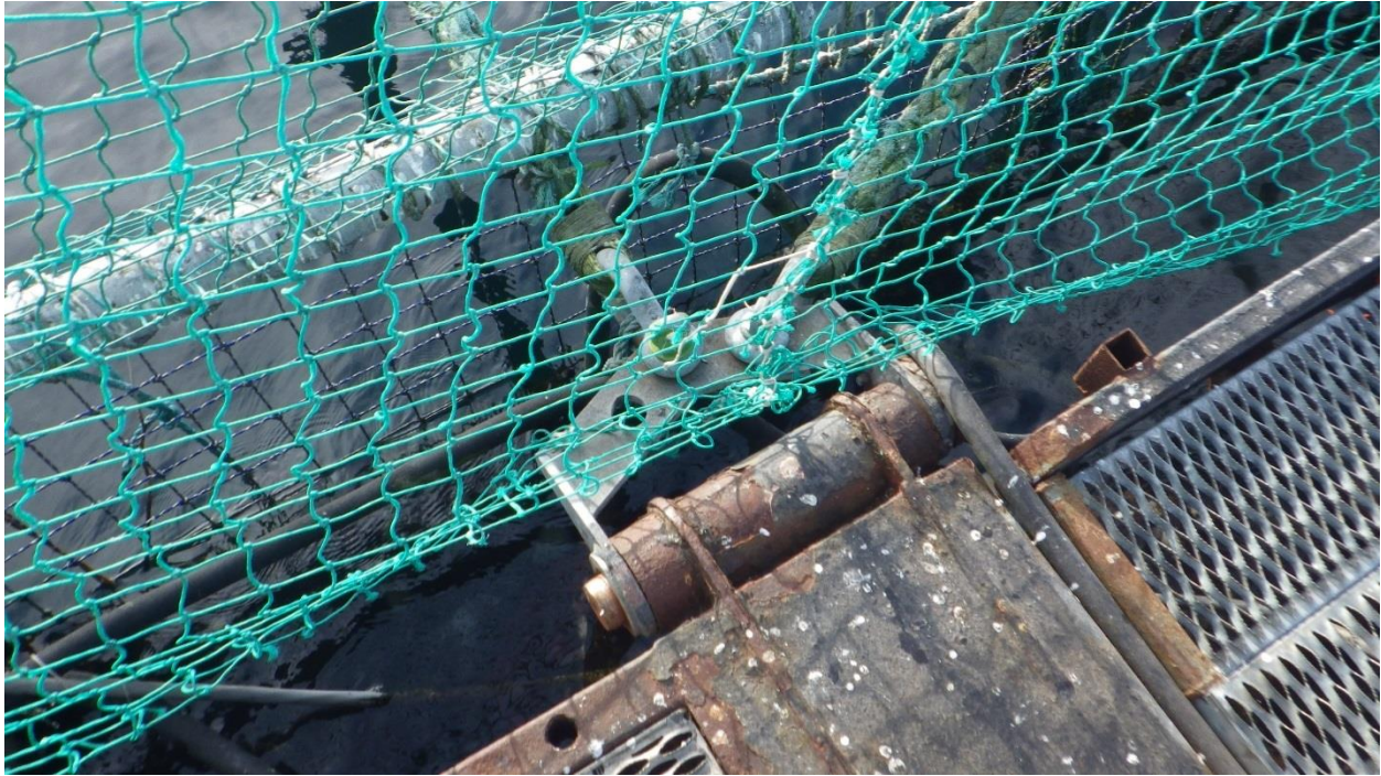
Figure C-38: North West Mid – Interconnection of North and South Net Pens. Hinge with moderate corrosion.
