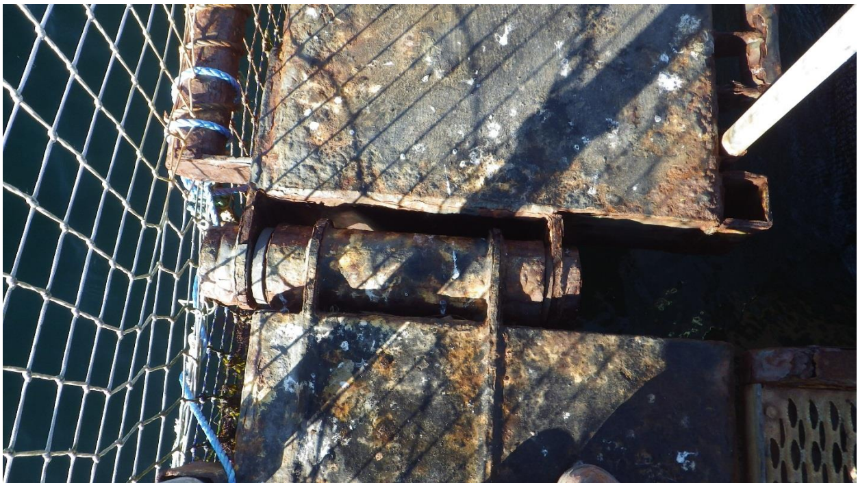
Figure D-46: Rusted Hinge Between Anchors #12 and #13 with moderate to major corrosion.
