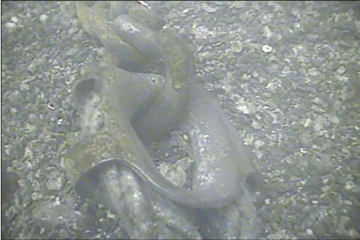
Photograph 55: View of Rope to Lower Anchor Chain Connection (Shackle and Thimble) at Orchard Rocks South Anchor Line 1, Looking East.
