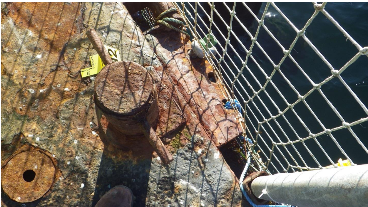
Figure D-30: Anchor #12, West Side of the South Net Pen
