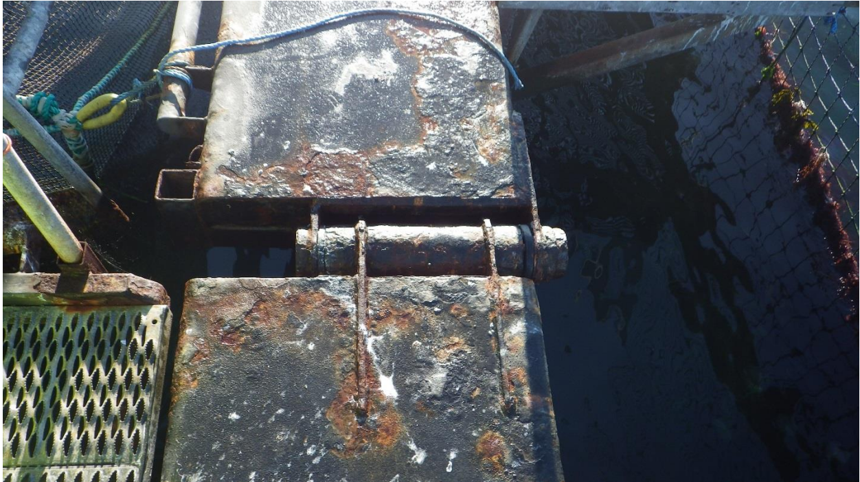
Figure C-60: Rusted Hinge between anchors 9 and 10. Moderate corrosion.
