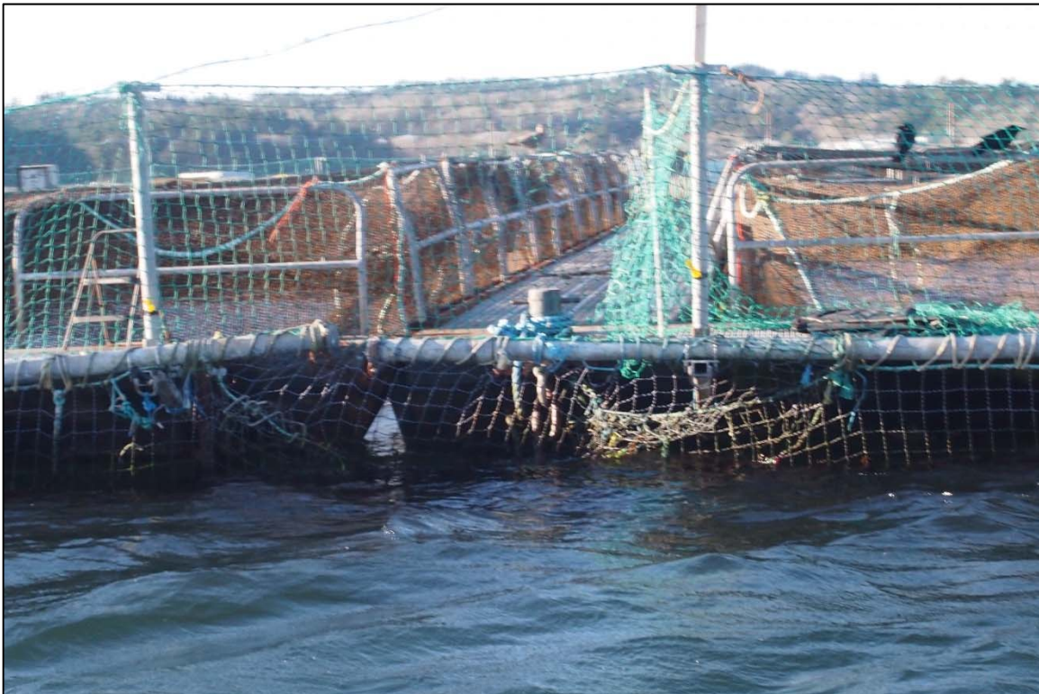
Photograph 10: View of Upper Anchor Chain to Float Connection at Orchard Rocks North Anchor Line 2, Looking West.
