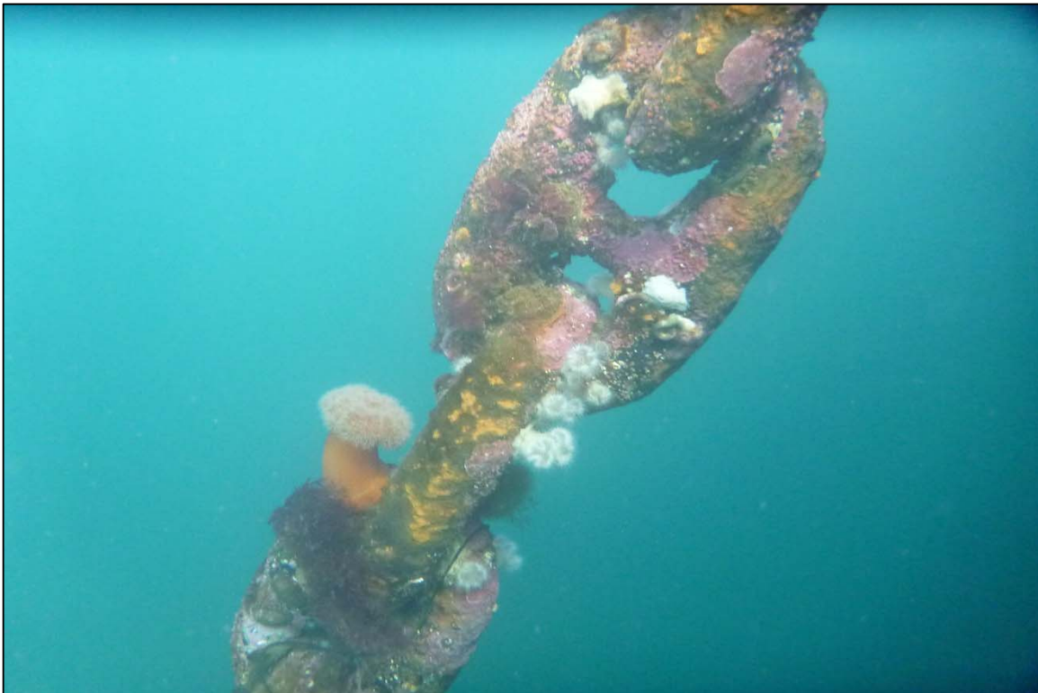
Photograph 40: View of Upper Anchor Chain Condition at Orchard Rocks North Anchor Line 13, Looking East.
