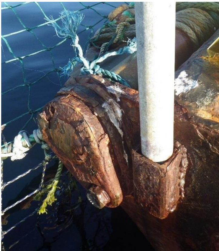
Figure C-29: Anchor #13, NW Corner of the North Net Pen. Moderate or major corrosion at hinge.
