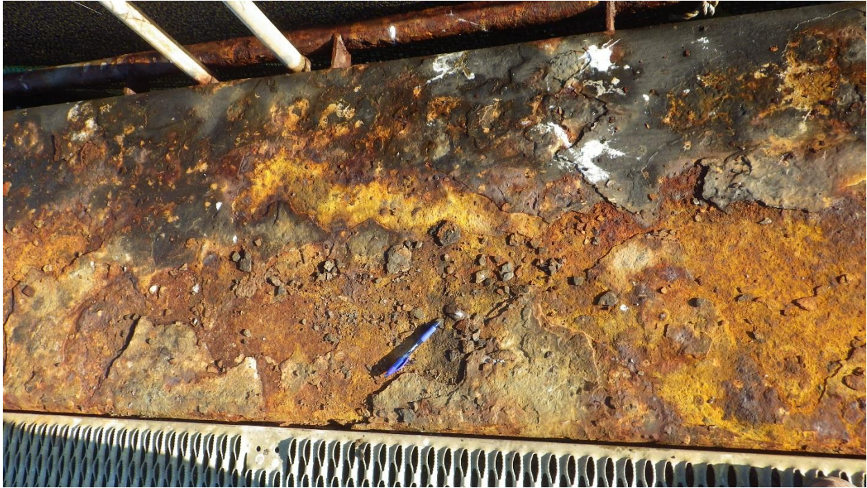
Figure C-62: Rusted walkway between anchors 11 and 12. Major corrosion.
