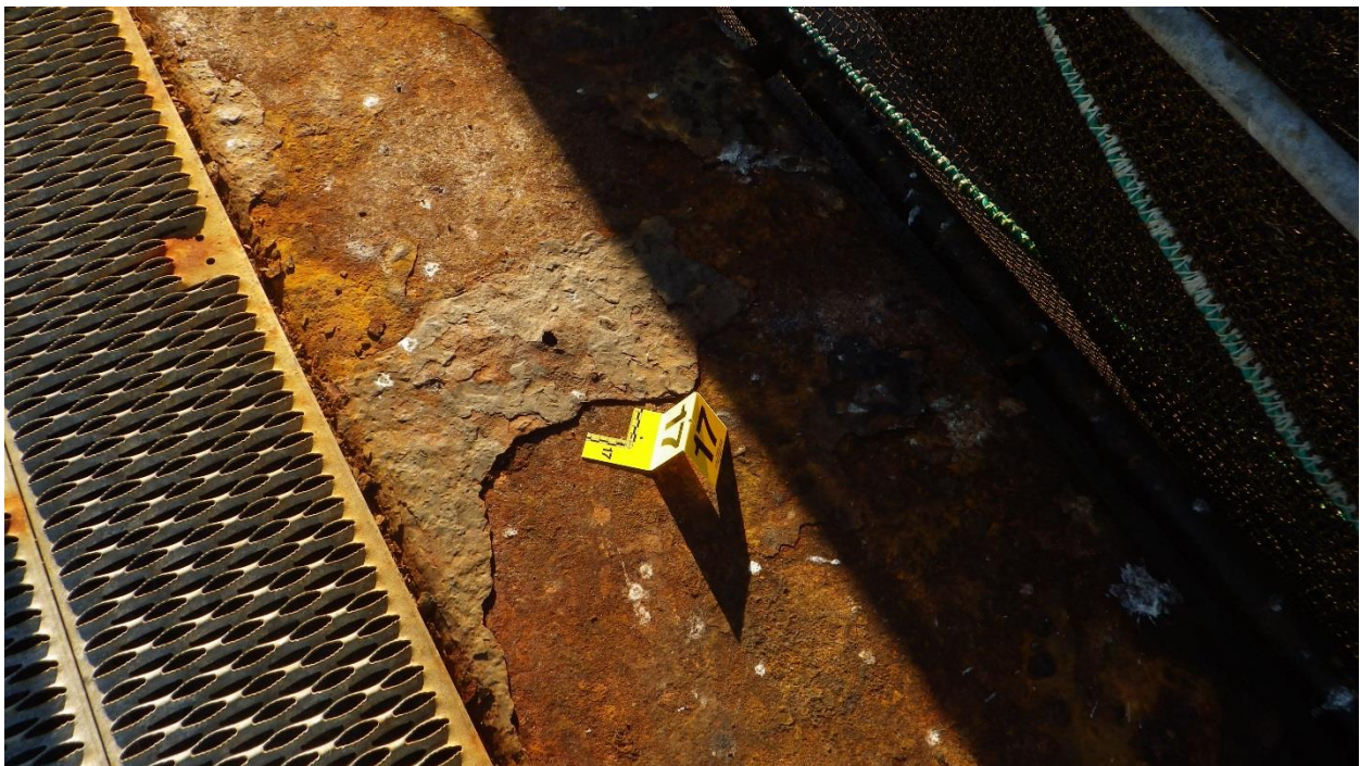
Figure C-51: Rusted Grating and Steel Walkway Framing. Major corrosion.
