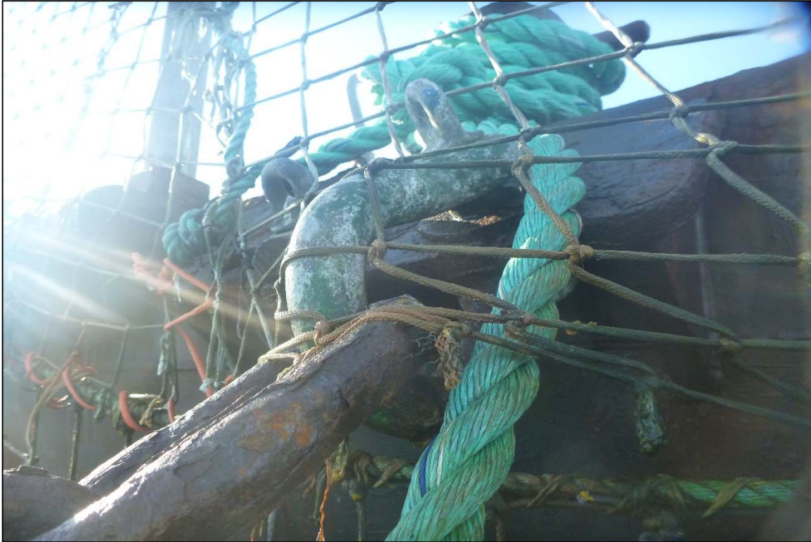
Photograph 53: View of Upper Anchor Chain to Float Connection at Orchard Rocks South Anchor Line 3, Looking West.
