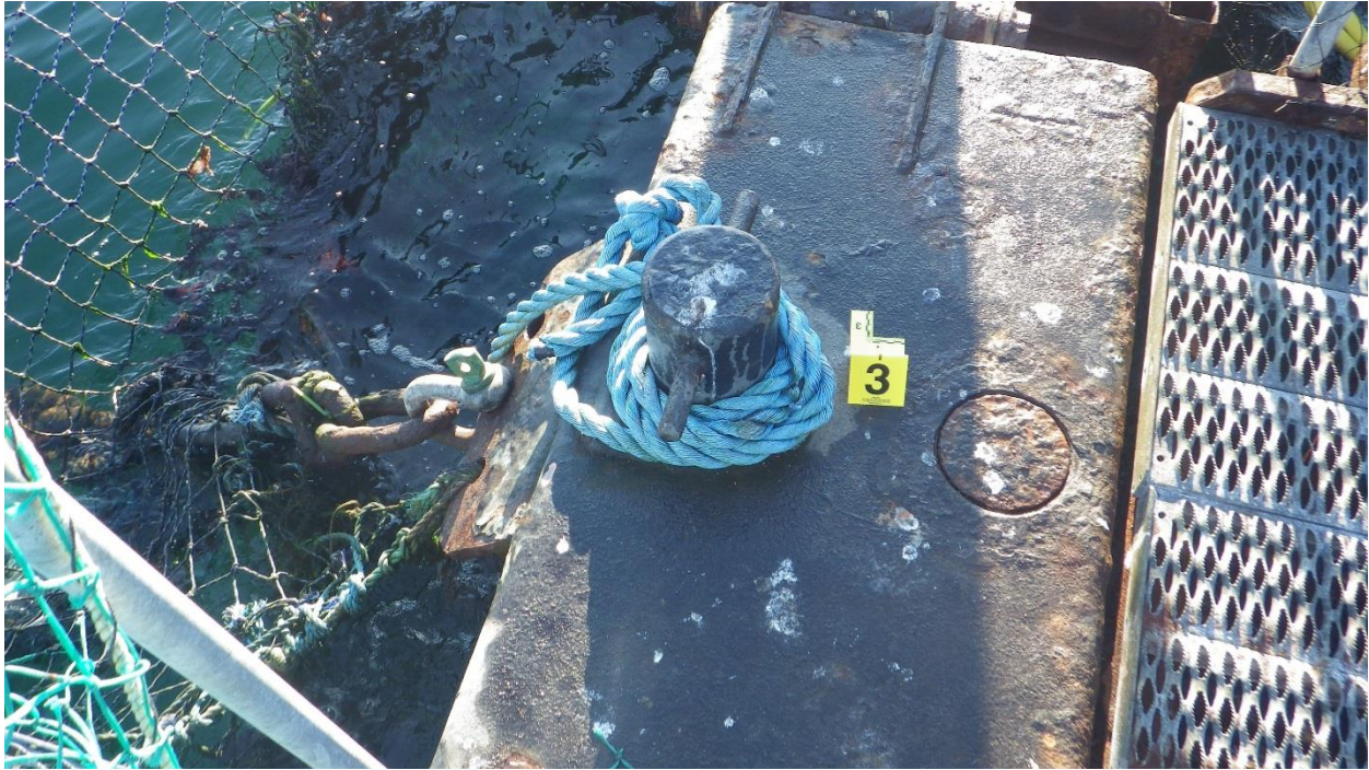
Figure C-10: Anchor #3, East Side of the North Net Pen. New shackle, old chain, moderate corrosion.
