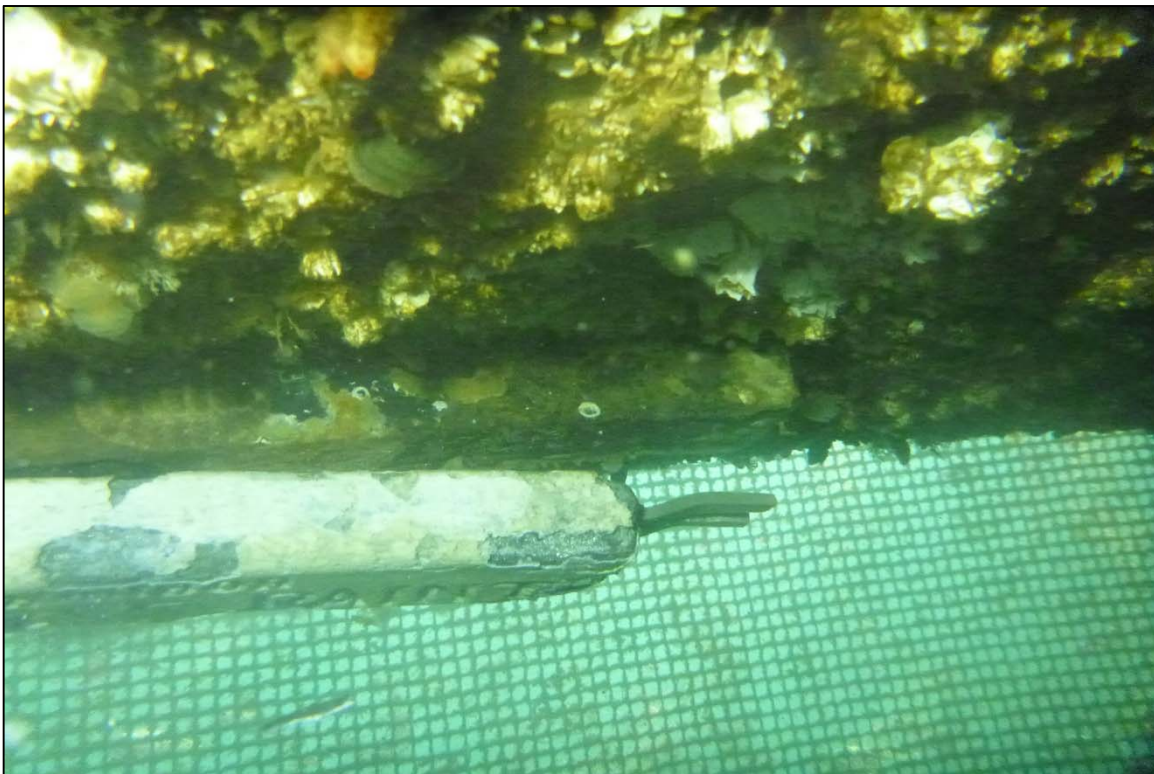
Photograph 8: View of Missing Connection of the Anode on the Steel pontoons at Orchard Rocks North Fish Net Pens System, Looking Northwest.
