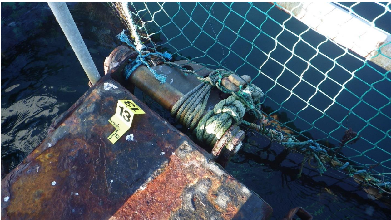
Figure C-27: Anchor #13, NW Corner of the North Net Pen. Hinge appears to be seized.
