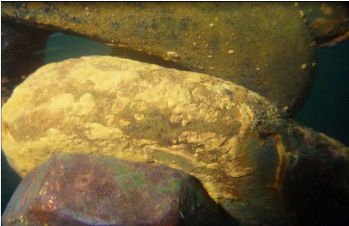
Photograph 76: View of Upper Anchor Chain to Float Connection Moderate Corrosion at Orchard Rocks South Anchor Line 7, Looking West.
