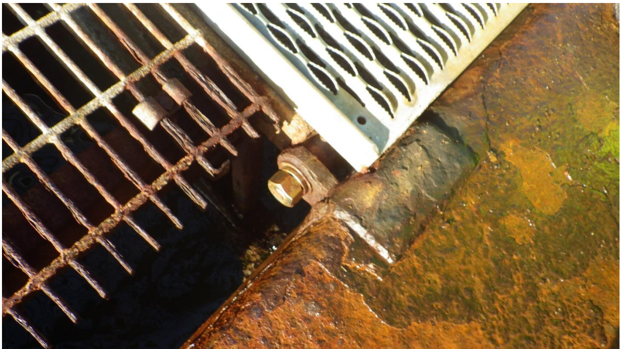
Figure C-49: Rusted Grating and Steel Walkway Framing. Old grating has lost section. New grating not bolted down.
