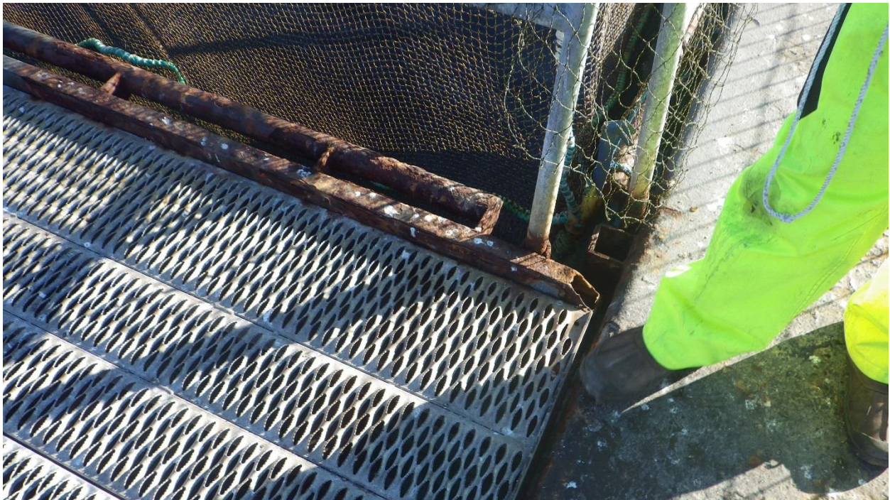
Figure D-56: Rusted Steel Framing, Handrail Brackets, and Net Pen Support Railings with moderate to major corrosion.
