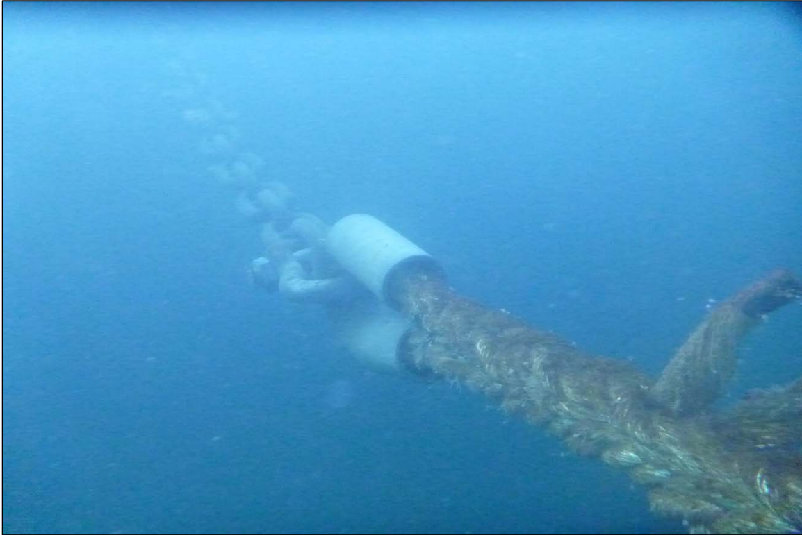
Photograph 17: View of Upper Anchor Chain to Rope Connection (Shackle and Thimble) at Orchard Rocks North Anchor Line 2, Looking West.
