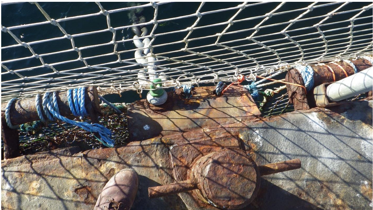
Figure D-28: Anchor #11, SW Corner of the South Net Pen. Reinforced hole on mooring bracket.
