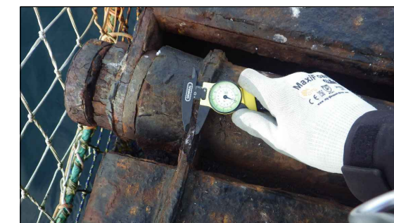
PHOTO 5 PEN HINGE WITH MAJOR CORROSION / 40% LOSS IN SECTION
