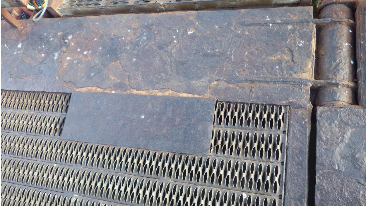
Figure C-54: Steel Plates Welded on Top of Rusted Grating. Moderate corrosion.
