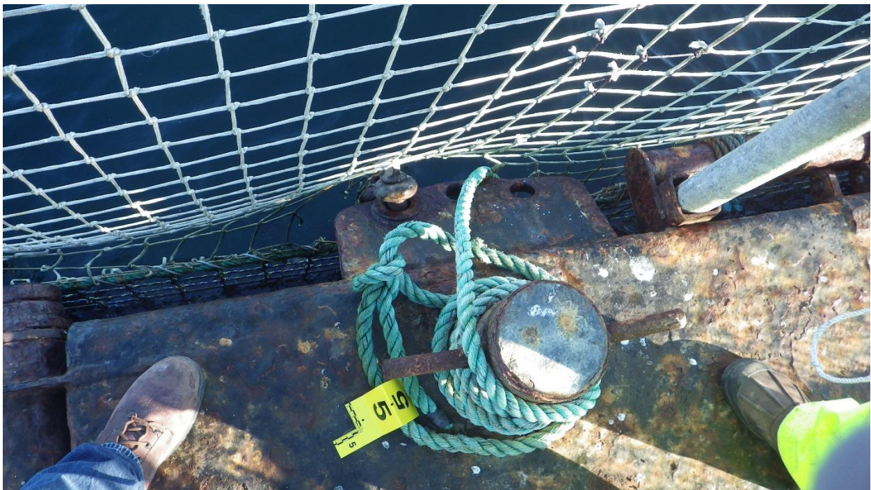
Figure D-14: Anchor #5, East Side of the South Net Pen. Mooring bracket hole reinforced.
