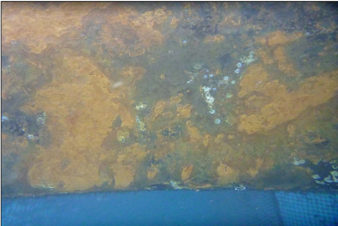
Photograph 50: View of the Steel Pontoon Condition at Orchard Rocks South Fish Net Pens System, Looking South.
