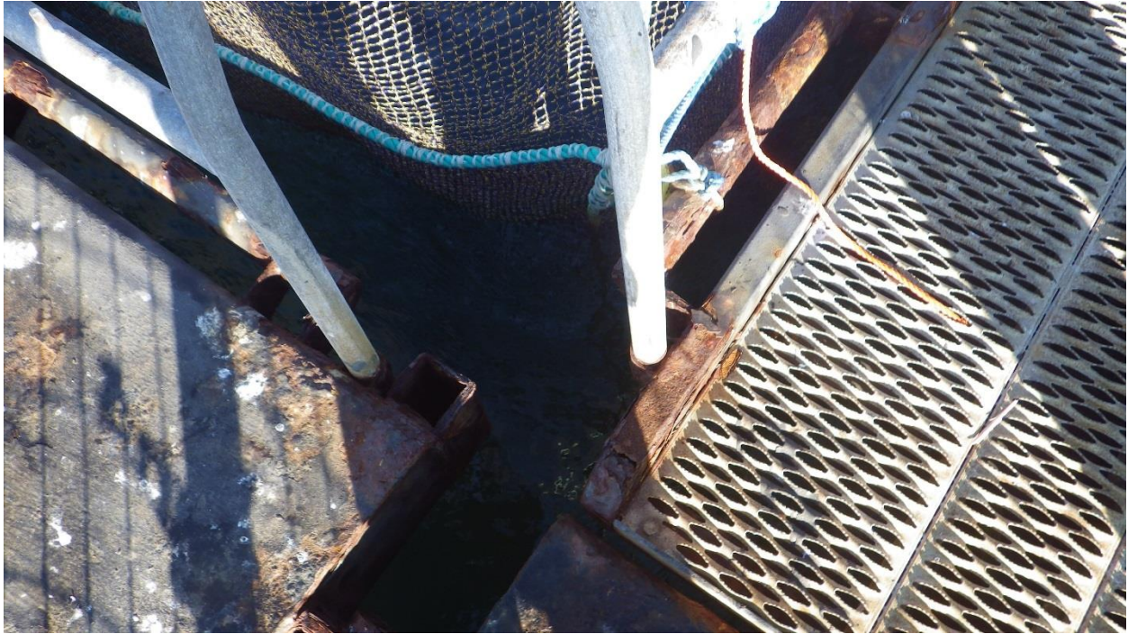
Figure D-55: Rusted Steel Framing, Handrail Brackets, and Net Pen Support Railings with moderate to major corrosion.
