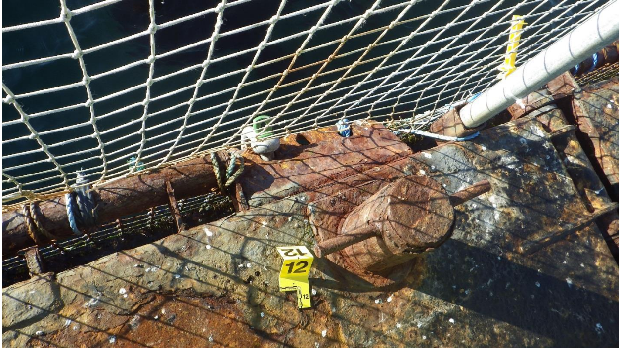
Figure D-29: Anchor #12, West Side of the South Net Pen
