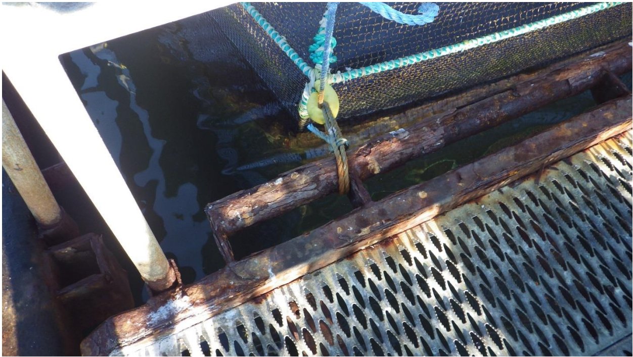
Figure C-50: Rusted Net Pen Support Railing. Major corrosion.
