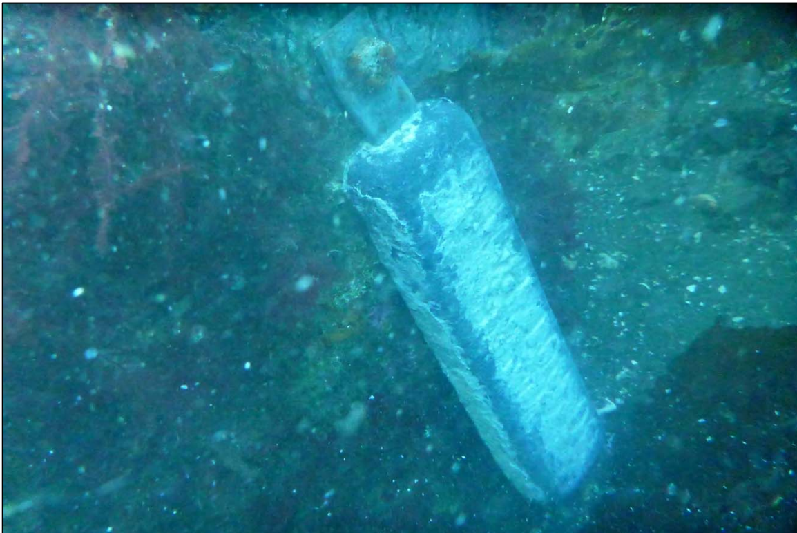
Photograph 44: View of Anode at the Pipe Anchor at Orchard Rocks North Anchor Line 14, Looking West.
