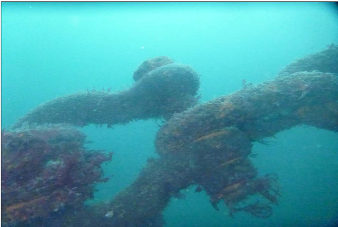
Photograph 64: View of Upper Anchor Chain to Anchor Rope Connection (Shackle) at Orchard Rocks South Anchor Line 4, Looking West.
