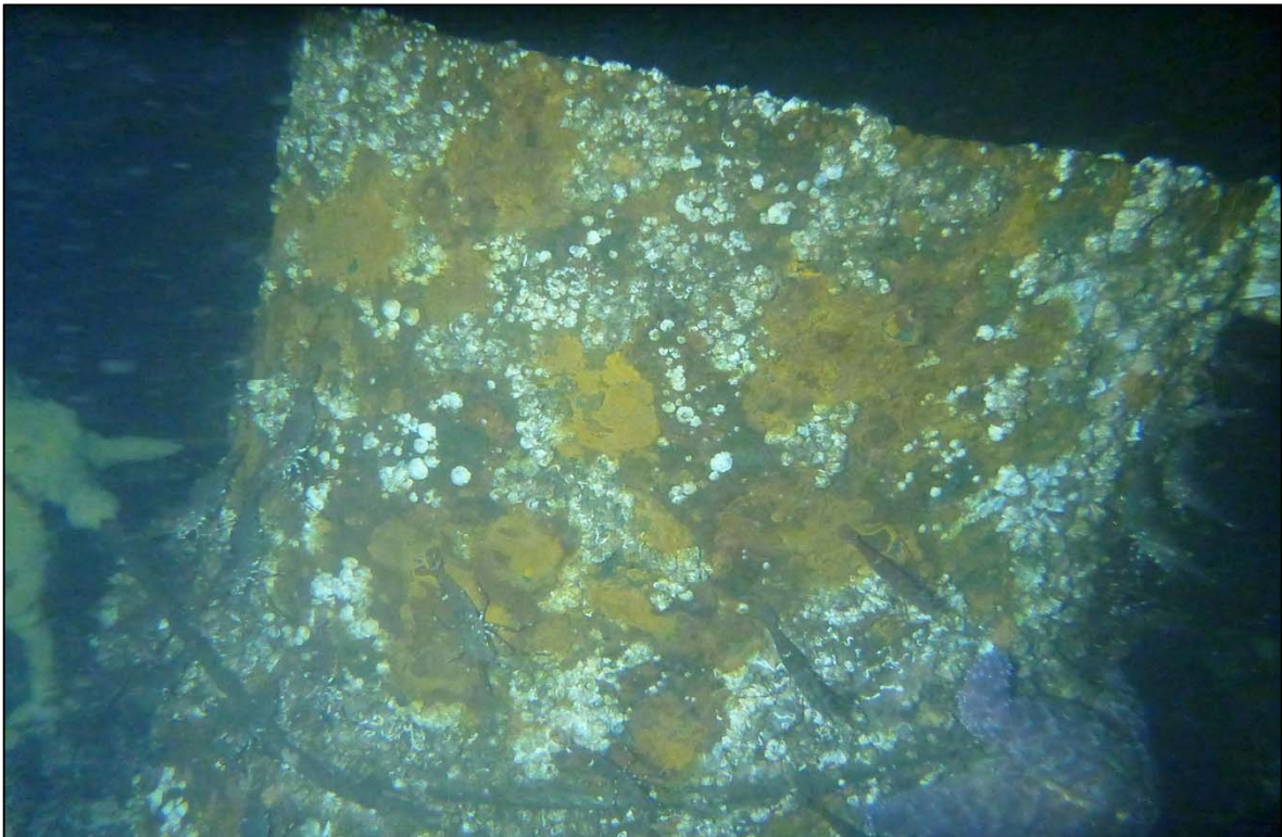
Photograph 72: View of Pipe Anchor at Orchard Rocks South Anchor Line 6, Looking East.
