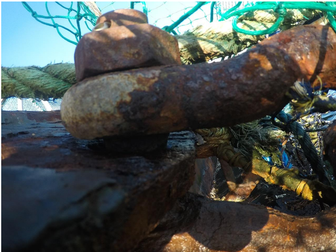
Figure D-48: Rusted Anchor Shackle at Anchor 13. Note Reduced Edge Bolt Hole on Mooring Bracket.
