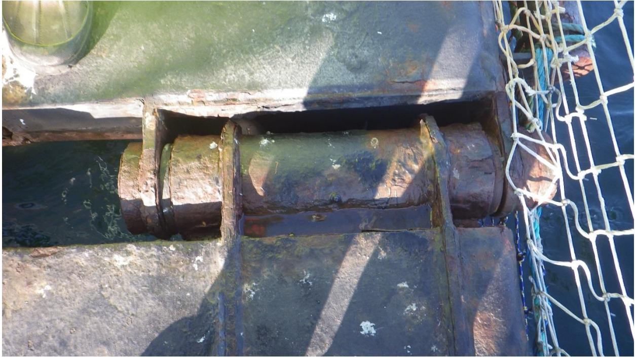
Figure D-45: Rusted Hinge Between Anchors #2 and #3 with moderate corrosion.
