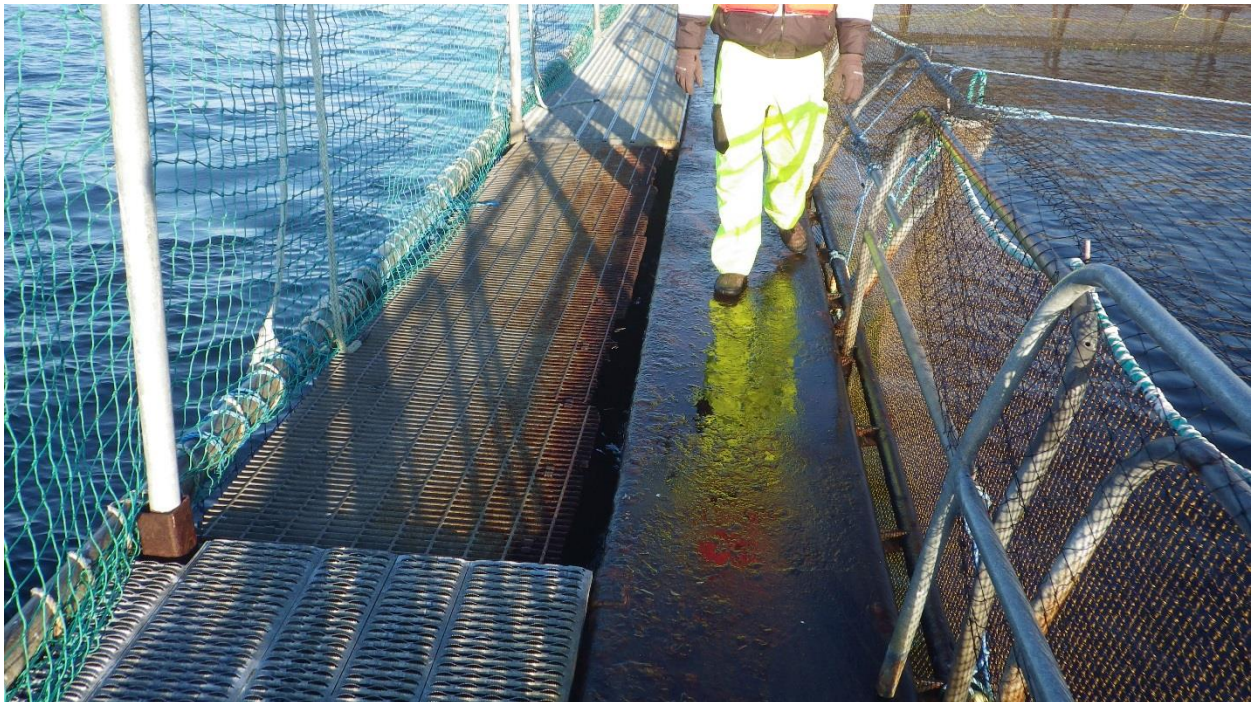
Figure C-41: Old Walkway Grating on west side. Note gap in grating.
