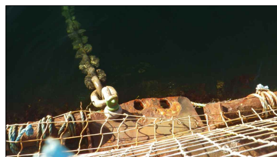
PHOTO 6 NEW SHACKLE AND CHAIN WITH MAJOR CORROSION ON MOORING BRACKET
