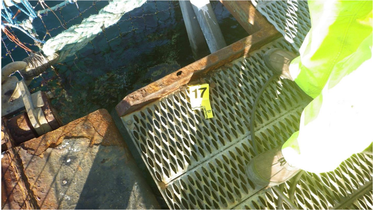
Figure D-57: Rusted Steel Framing, Hole in Framing Member with total section loss, major to severe corrosion.
