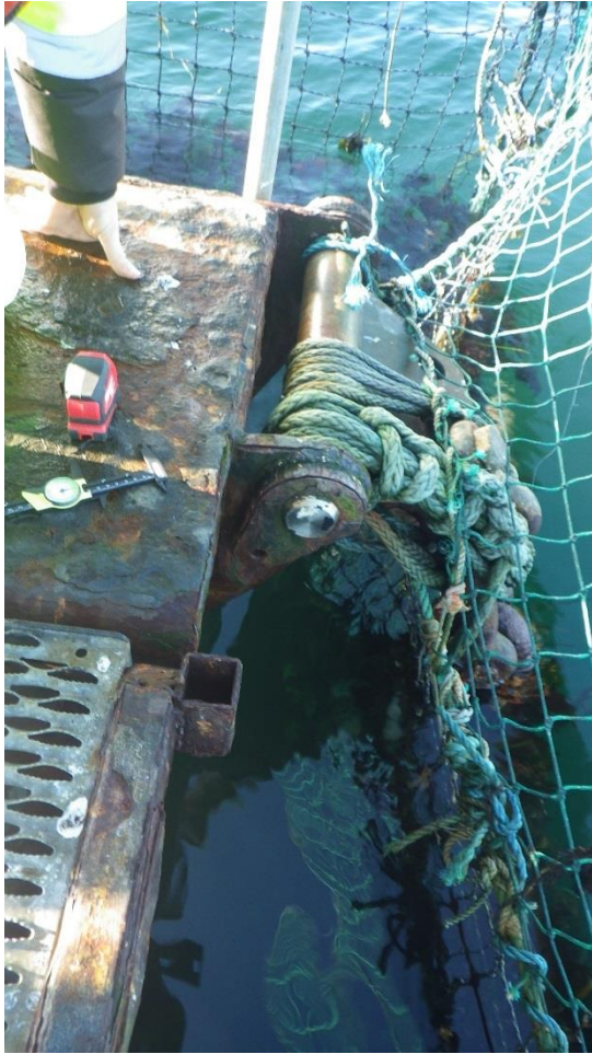
Figure C-30: Anchor #13, NW Corner of the North Net Pen. Hinge at different angle than chain.
