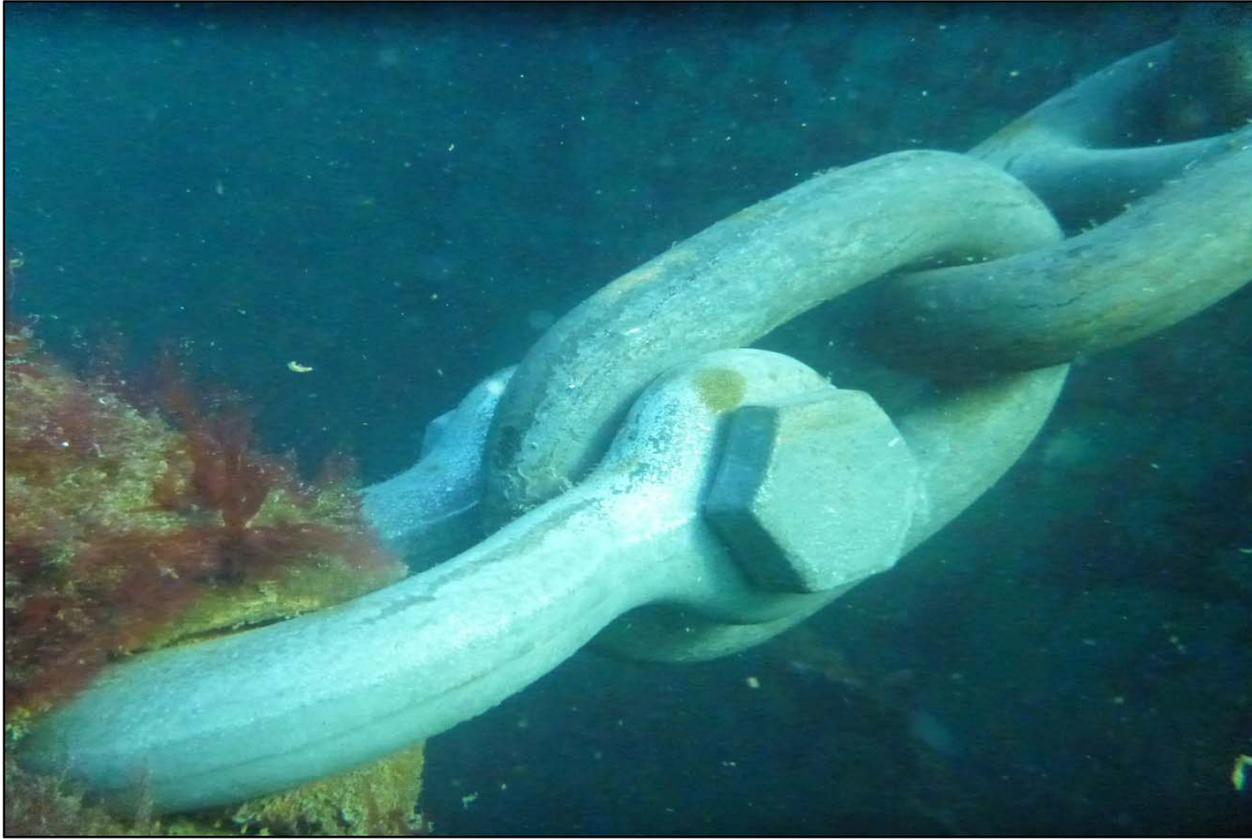
Photograph 29: View of Upper Anchor Chain Condition at Orchard Rocks North Anchor Line 9, Looking North.
