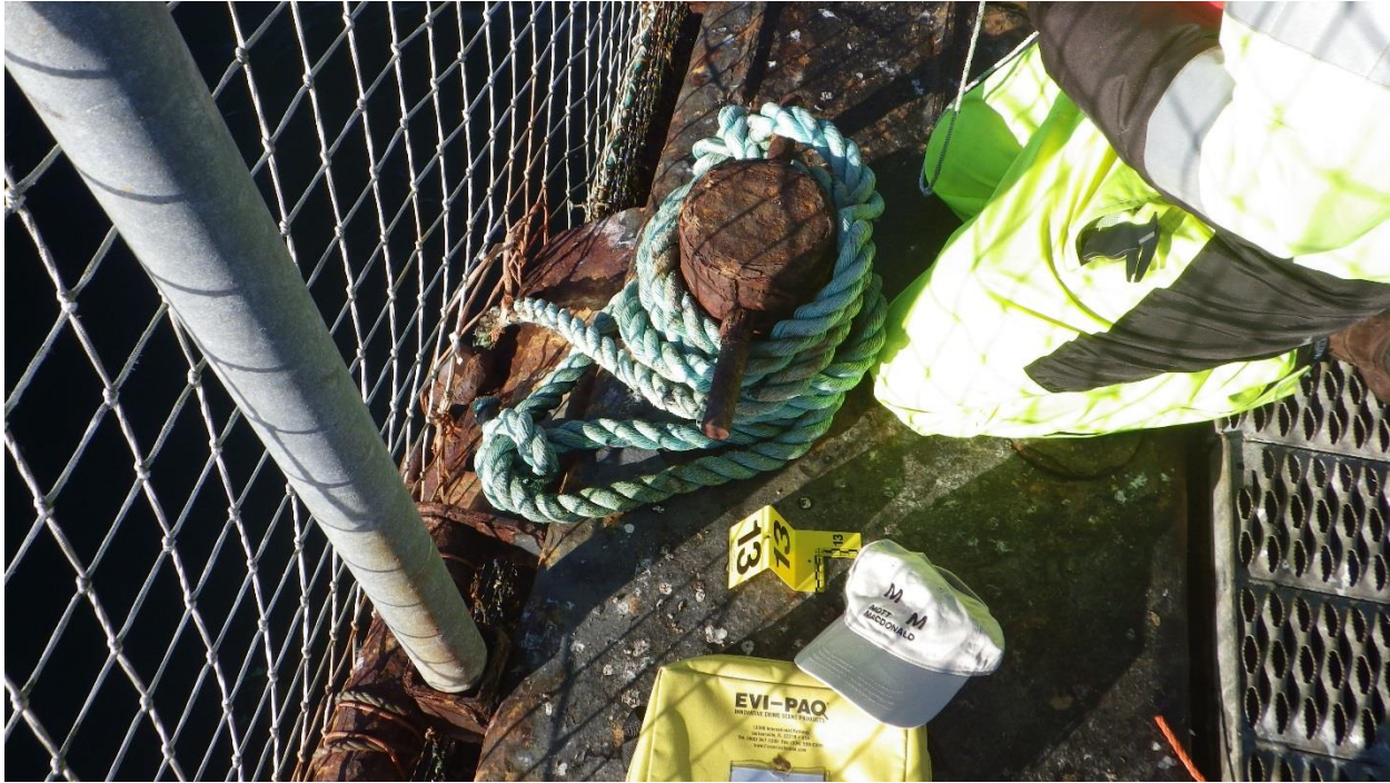
Figure D-31: Anchor #13, West Side of the South Net Pen. Moderate corrosion on shackle.
