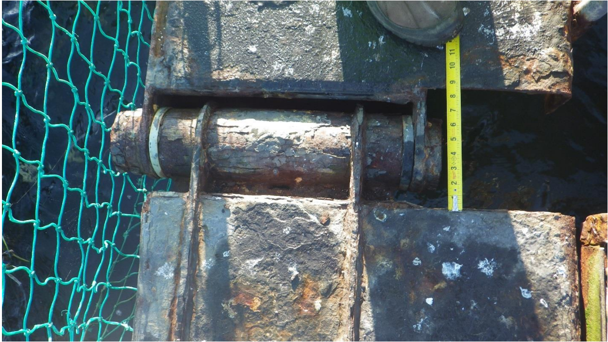
Figure C-58: Rusted Hinge between anchors 2 and 3. Major corrosion.
