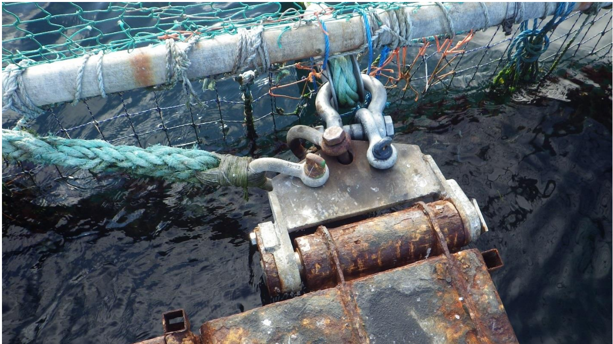
Figure C-37: North West Hinge – Connection of North and South Net Pens. Hinge with moderate corrosion.
