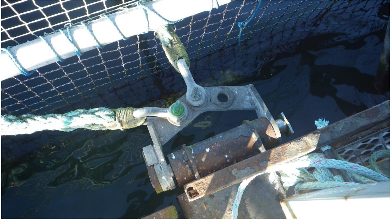
Figure D-41: South East Mid Hinge connected to North pen with minor corrosion.
