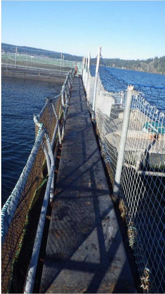
Figure D-49: Steel Framing Walkway. Note that Grating is Absent.
