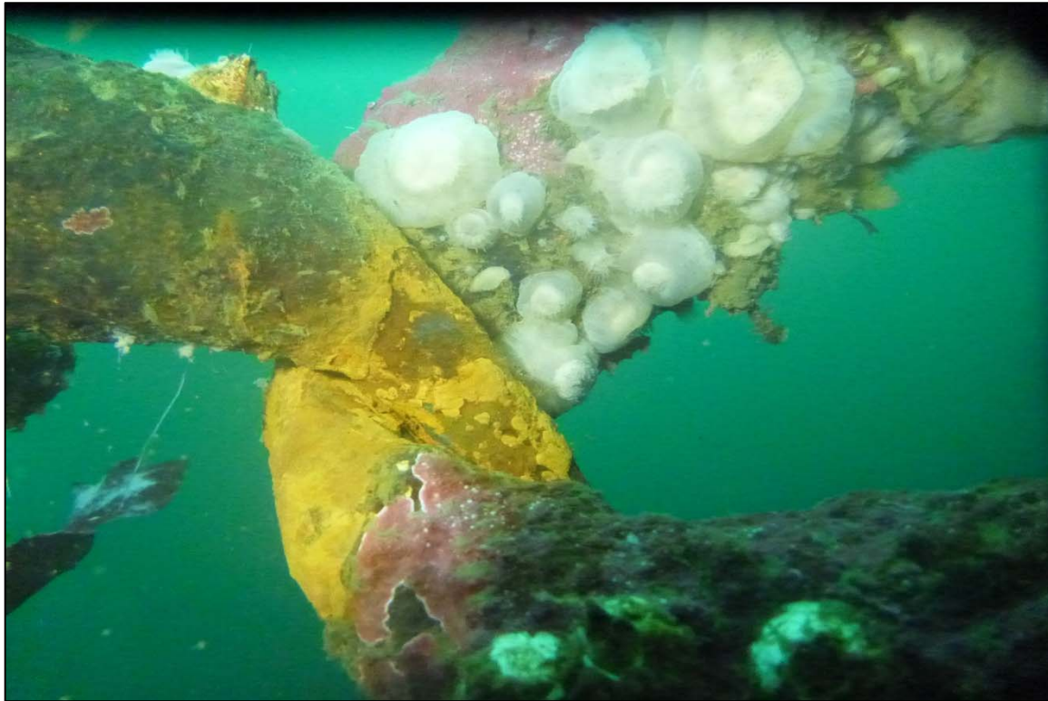
Photograph 25: View of Upper Anchor Chain Shackle with up to 75% Section Loss at Orchard Rocks North Anchor Line 4, Looking North.
