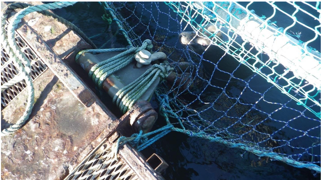
Figure C-33: Anchor #15, North Side of the North Net Pen. Hinge at different angle than chain.
