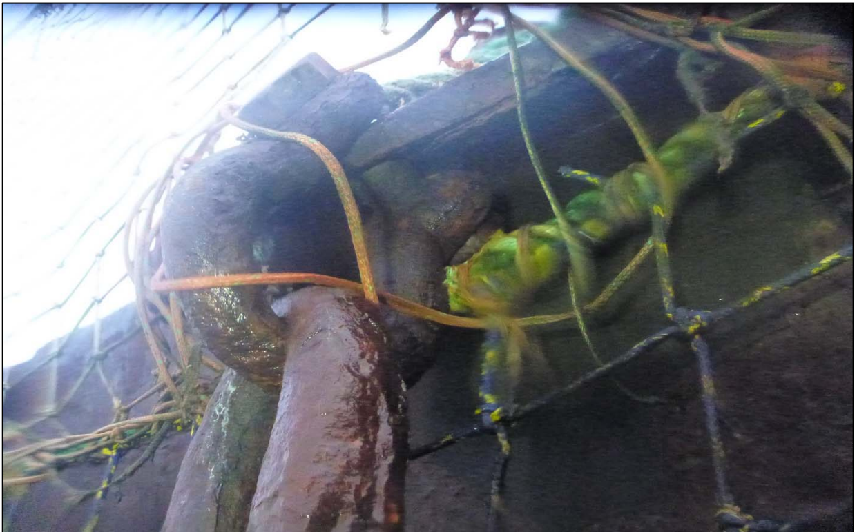
Photograph 88: View of Upper Anchor Chain Connection at Orchard Rocks South Anchor Line 13, Looking North.
