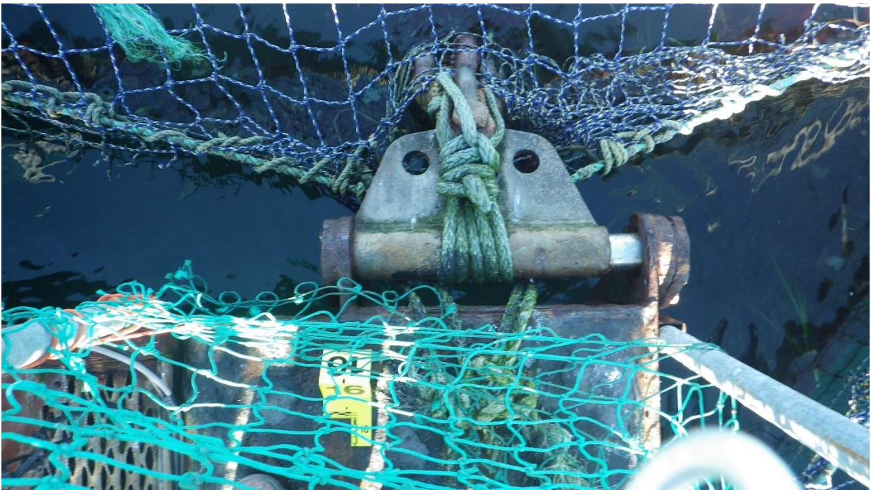
Figure C-35: Anchor #16, NE Corner of the North Net Pen. Hinge at different angle than chain.
