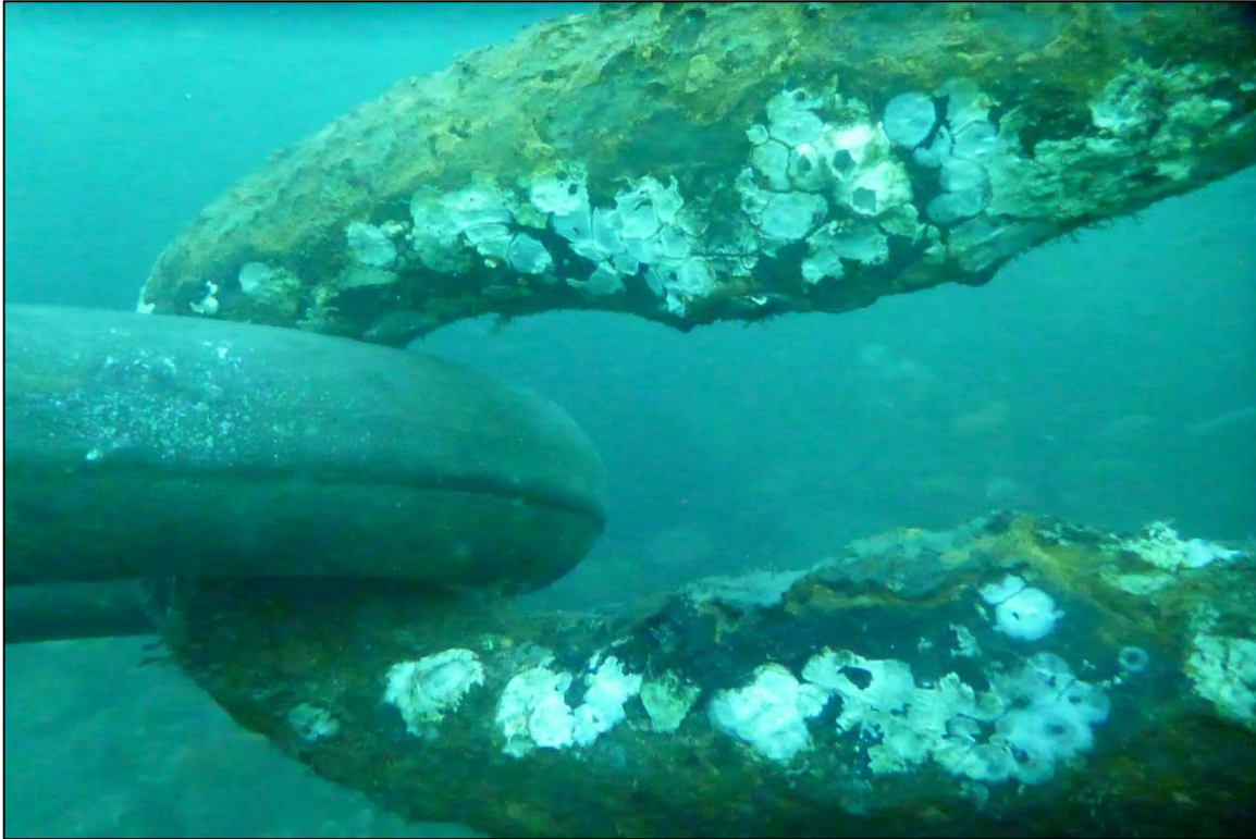
Photograph 45: View of Section Loss and Missing Stud in the Anchor Chain at Orchard Rocks North Anchor Line 15, Looking East.
