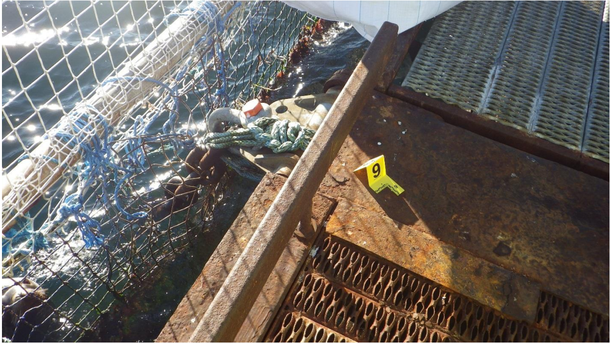
Figure D-23: Anchor #9, South Side of the South Net Pen. Hinge with moderate corrosion.
