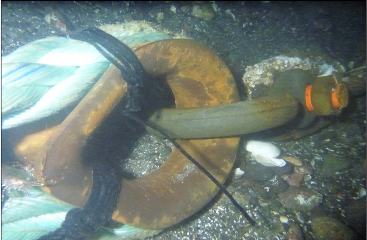
Photograph 71: View of Lower Anchor Chain to Anchor Rope Connection at Orchard Rocks South Anchor Line 6, Looking West.
