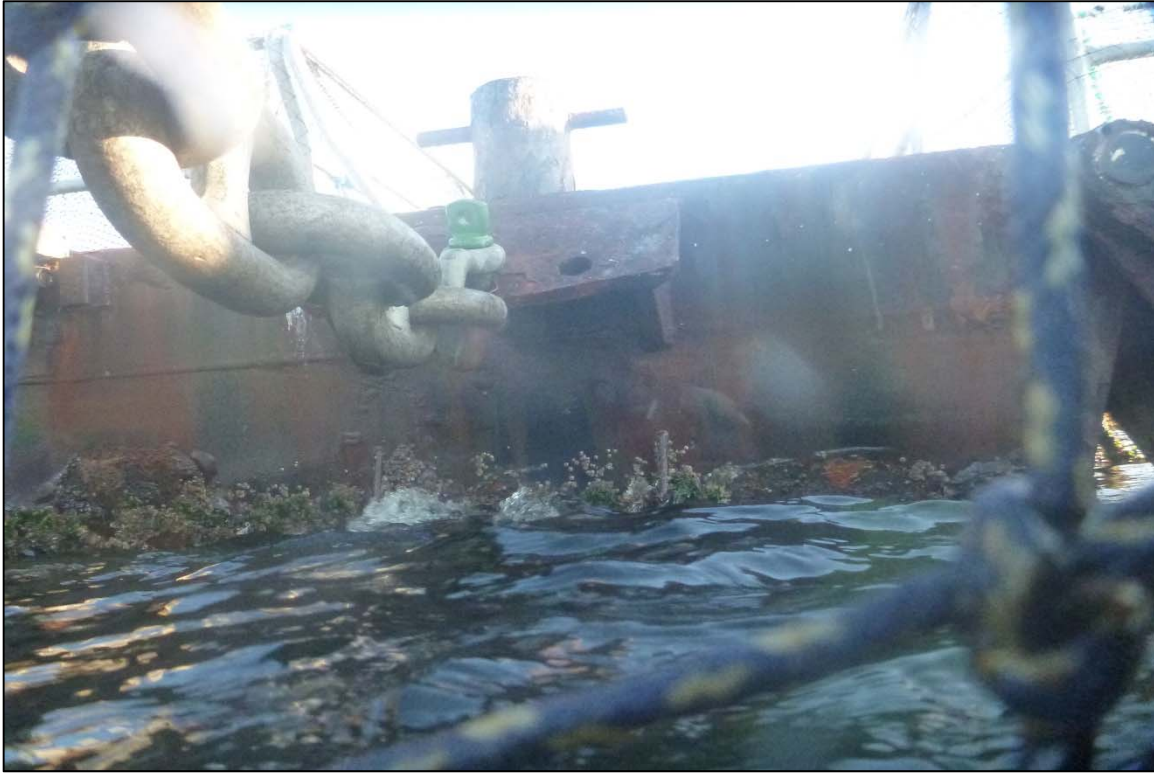
Photograph 11: View of Upper Anchor Chain to Float Connection at Orchard Rocks North Anchor Line 9, Looking East.
