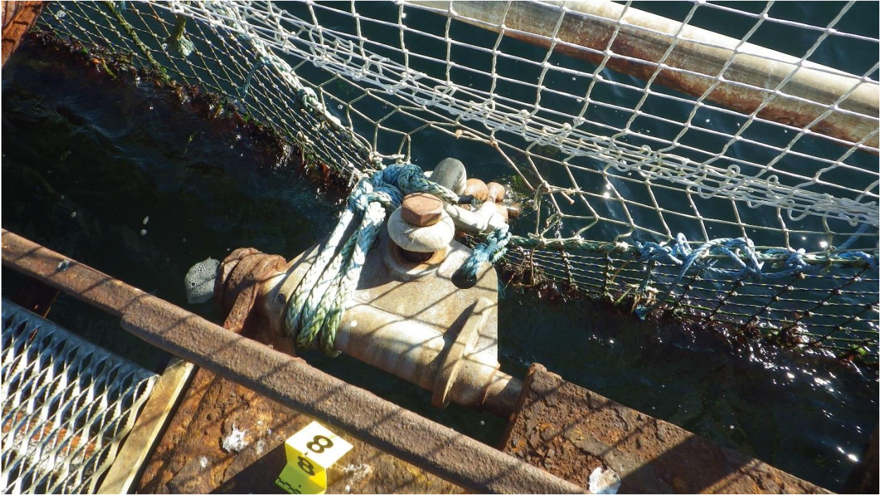
Figure D-21: Anchor #8, South Side of the South Net Pen. Hinge with moderate corrosion.
