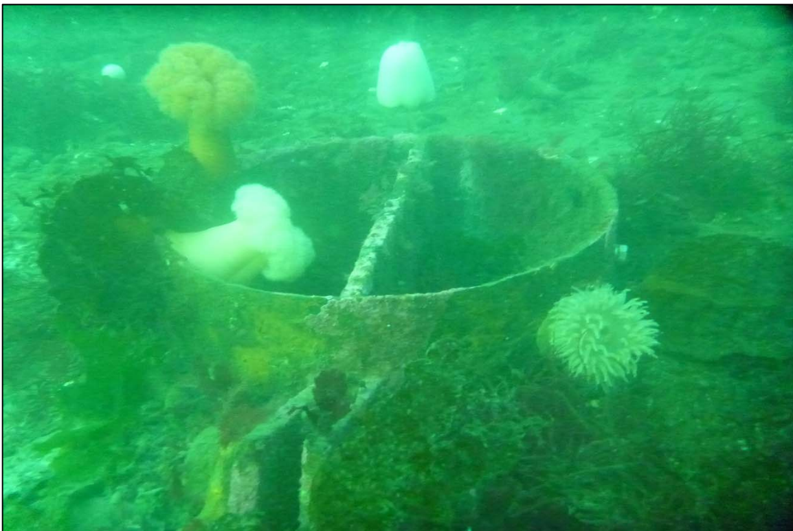
Photograph 42: View of Pipe Anchor Condition at Orchard Rocks North Anchor Line 13, Looking North.
