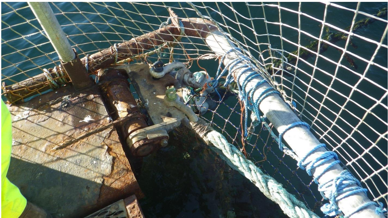
Figure D-42: South West Hinge connected to North pen with moderate to major corrosion.
