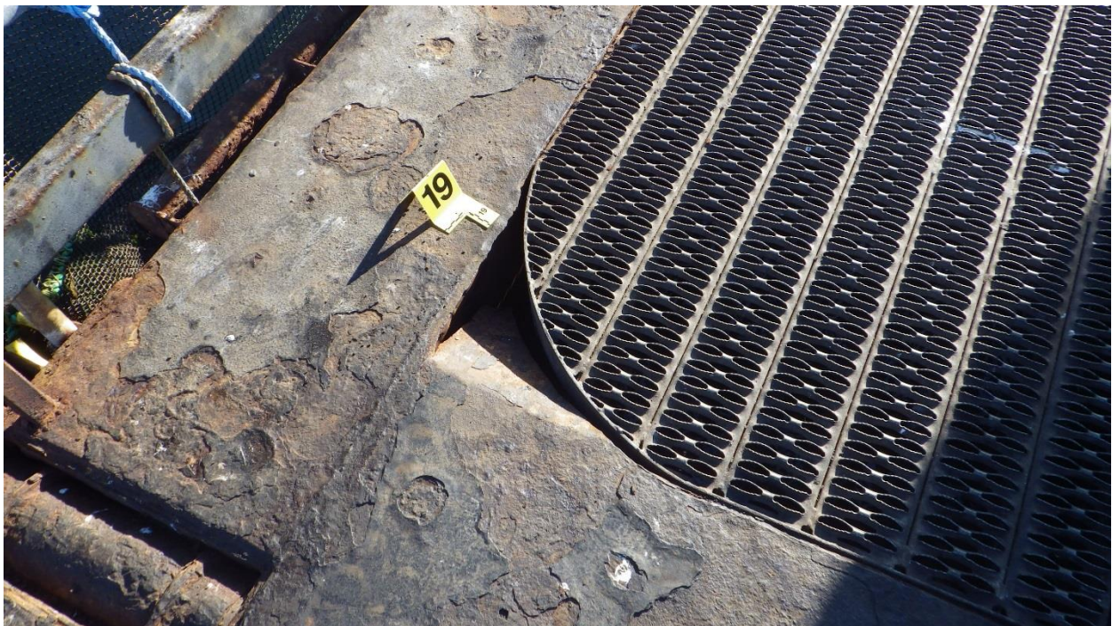
Figure C-53: Damaged Walkway on Center Bridge due to corrosion
