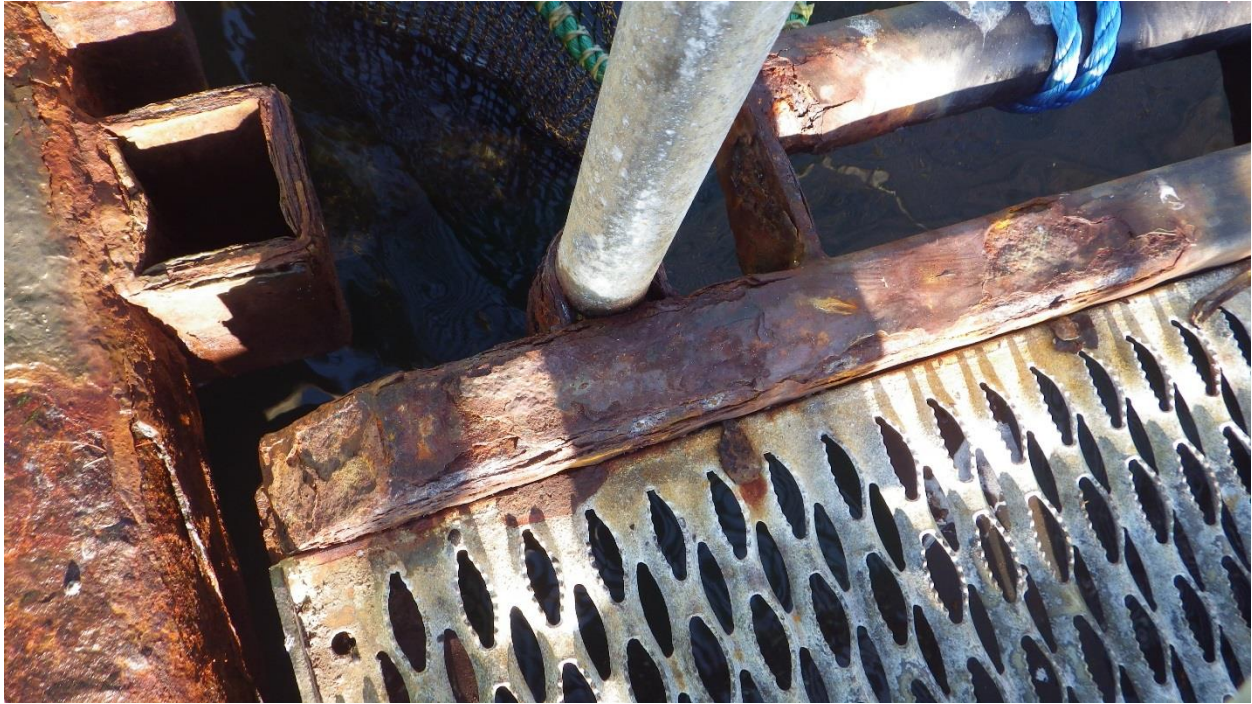
Figure C-48: Rusted Handrail Bracket and Structural Framing. Major corrosion.
