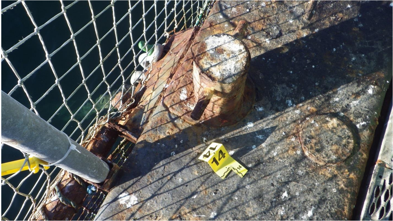
Figure D-33: Anchor #14, West Side of the South Net Pen. New shackle and chain.
