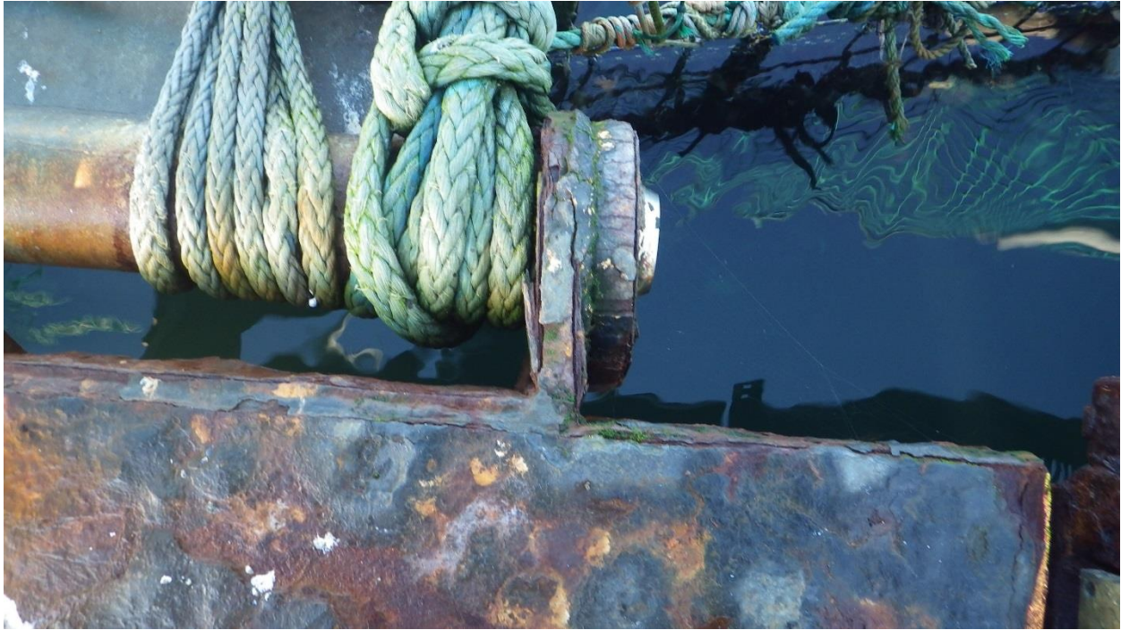
Figure C-28: Anchor #13, NW Corner of the North Net Pen. Moderate corrosion at hinge.
