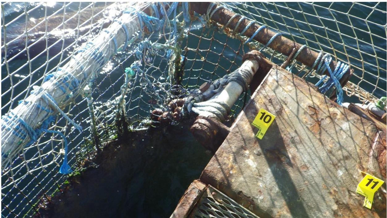
Figure D-26: Anchors #10 and #11, SW Corner of the South Net Pen. Hinge with moderate corrosion.
