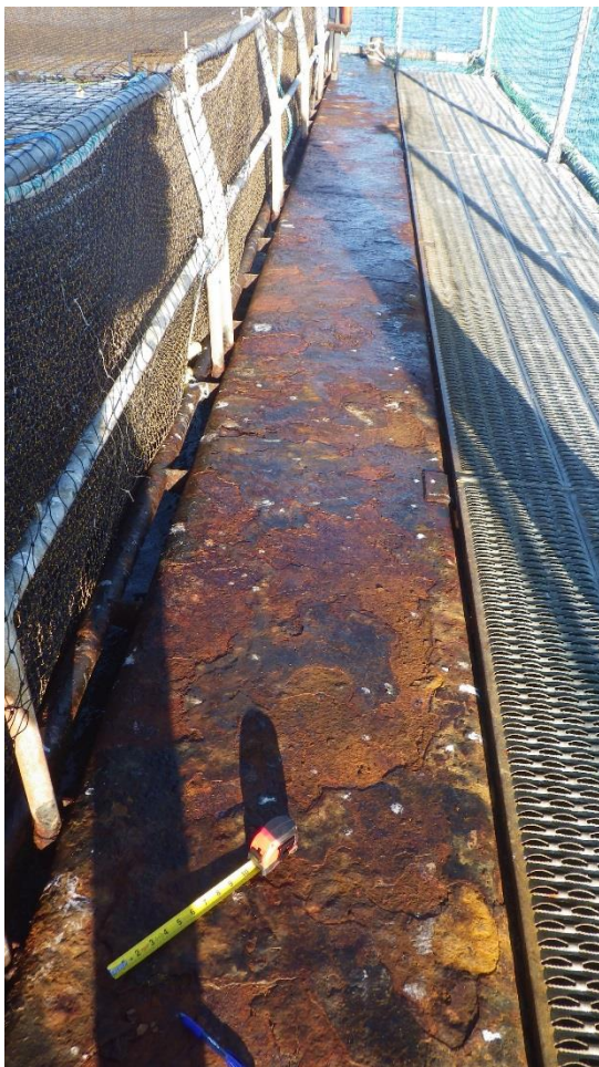
Figure C-43: Rusted Outer Steel Frame on North East side walkway. Moderate to major corrosion.
