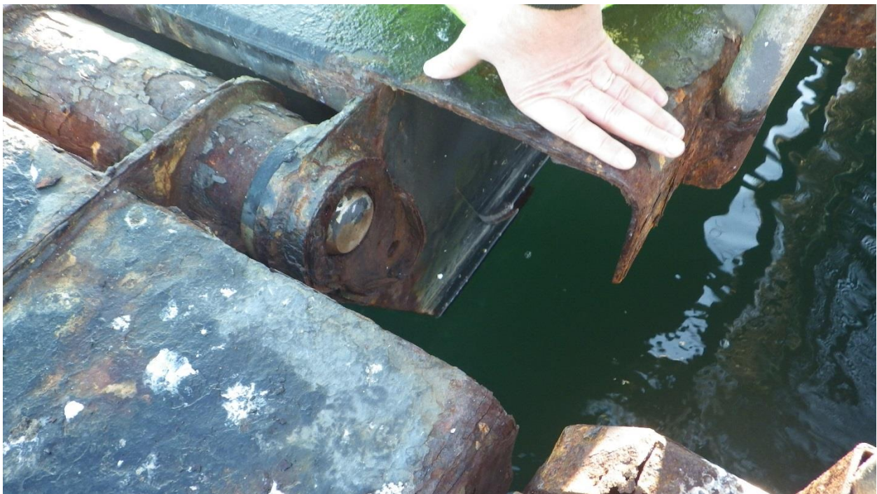
Figure C-59: Rusted Hinge between anchors 2 and 3. Major corrosion.
