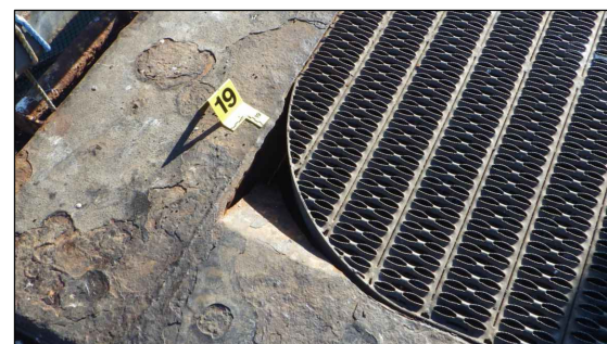
PHOTO 3 DAMAGE DUE TO CORROSION ON CENTER BRIDGE
