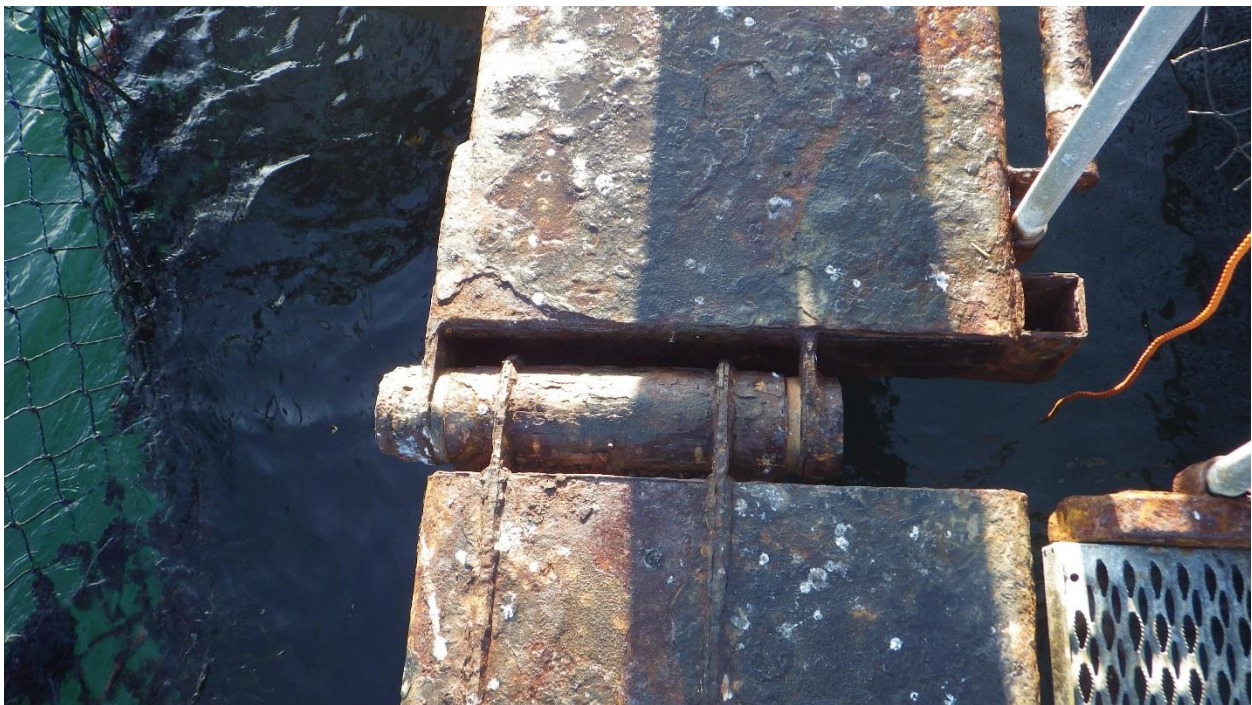
Figure C-57: Rusted Hinge between anchors 5 and 6. Major corrosion.
