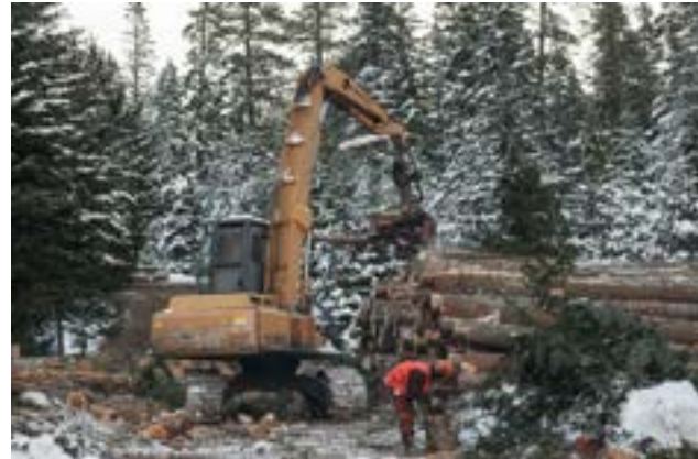
Restoration has lowered the risk of wildfire for the Ridge and 3 communities (Photo by TNC)
