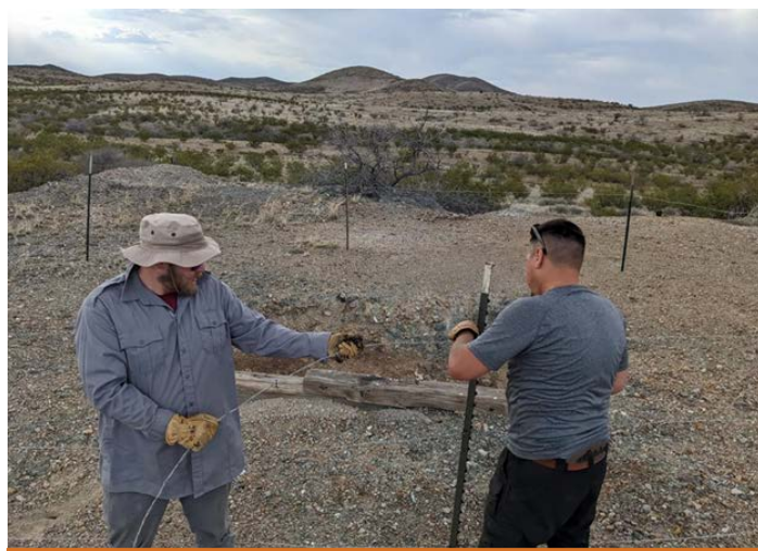
AML staff construct a temporary fence around an abandoned mine shaft near Lordsburg.
